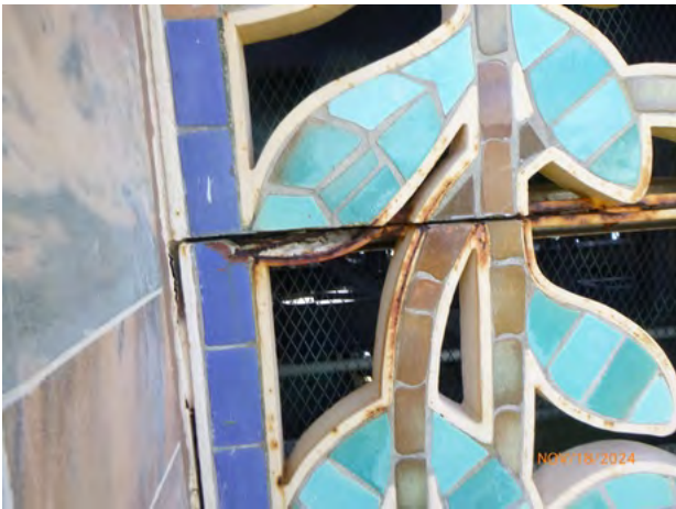
9-164 TerraCotta_Spall Missing + Steel 2024-3.jpg
