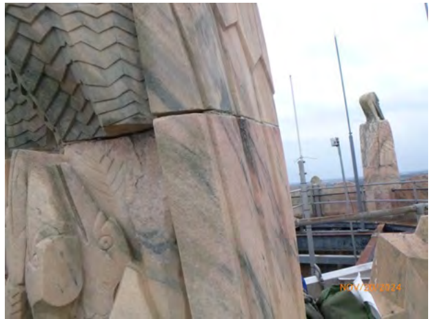
136-200 Stone_Joints Mortar Missing 2024-3.jpg
