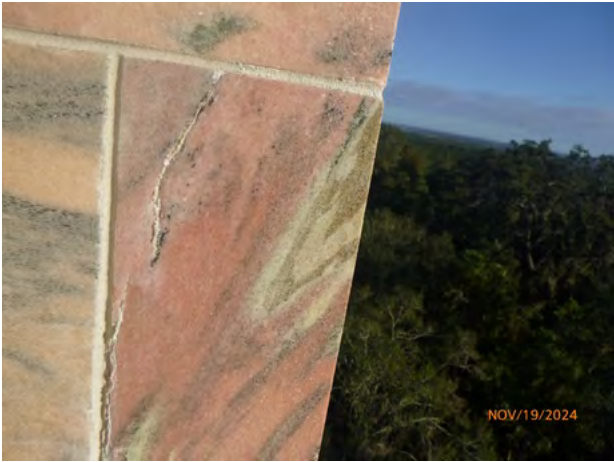
355-78 Stone_Crack Single unit 2024-2.jpg
