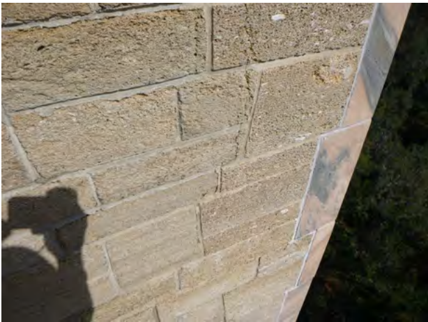
264-132 Stone_Crack System units and joints 2024-3.jpg
