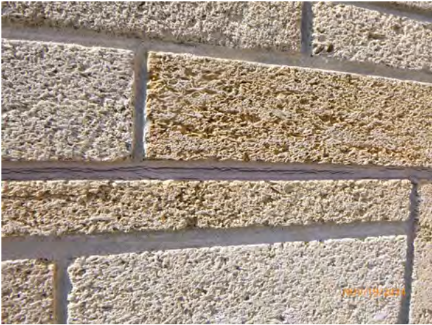
340-80 Stone_Joints Sealant Failed 2024-2.jpg
