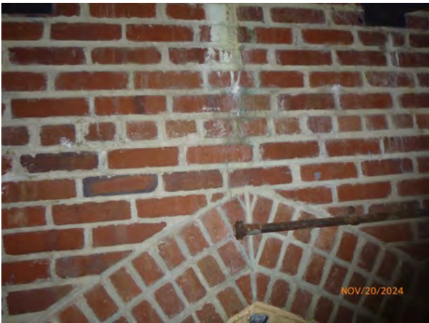
651-179 Brick_Crack System units and joints 2024-1.jpg
