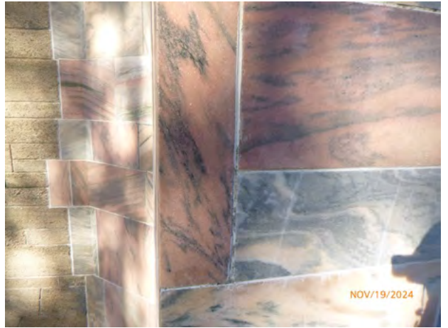
342-16 Stone_Joints Mortar Failed 2024-1.jpg
