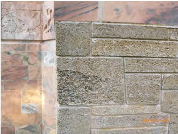
234-26 Stone_Crack System units and joints 2024-2.jpg
