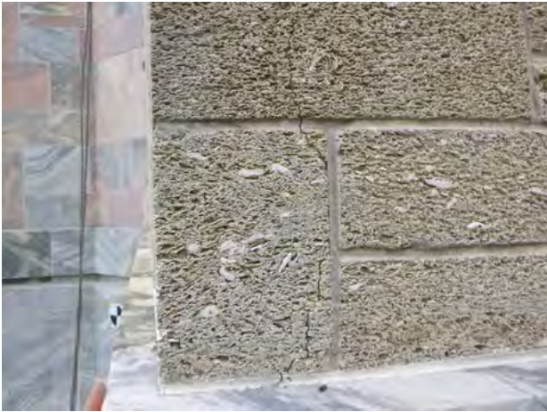
135-10 Stone_Crack System units and joints 2024-2.jpg
