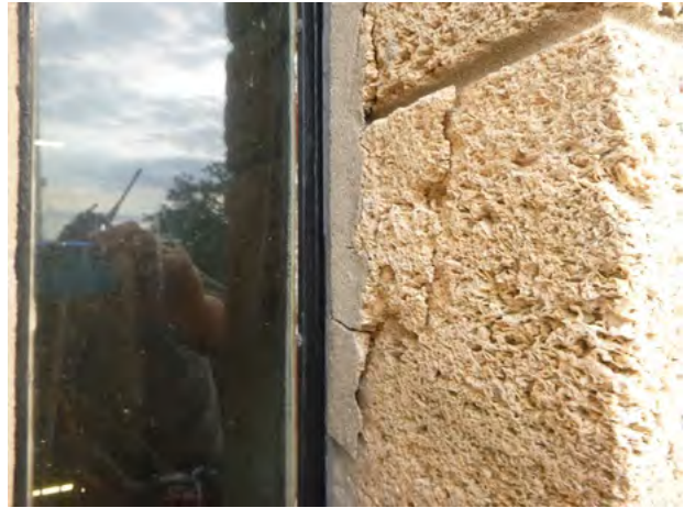
164-55 Stone_Spall Removed 2024-2.jpg
