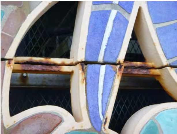
16-149 ArchMetal_Corrosion Pitted 2024-1.jpg
