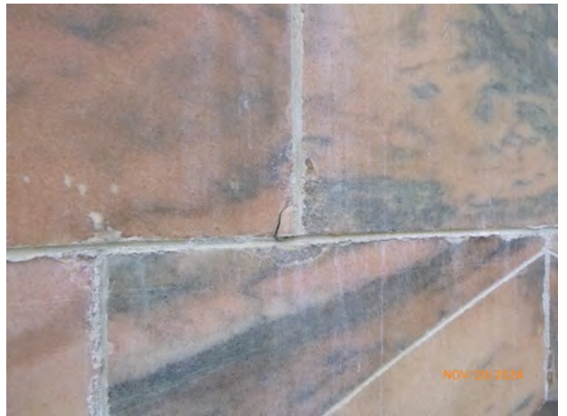
137-182 Stone_Spall Removed 2024-1.jpg
