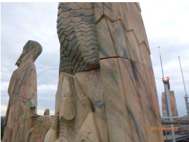
134-200 Stone_Spall Missing 2024-3.jpg
