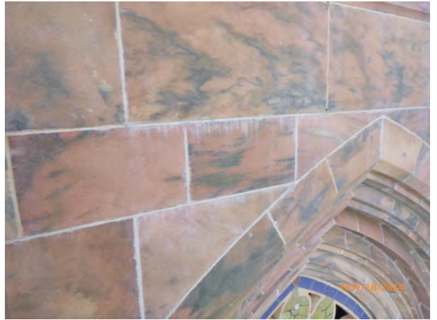
37-182 Stone_SoilStain Leached Salts 2024-3.jpg
