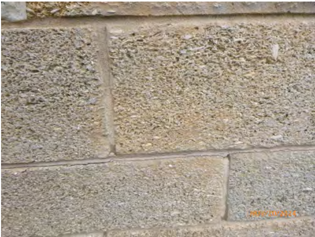
61-71 Stone_Joints Sealant Failed 2024-3.jpg
