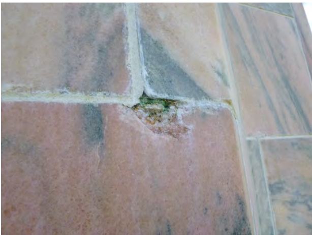
41-163 Stone_Spall Missing 2024-1.jpg
