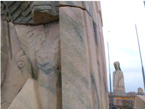
134-200 Stone_Spall Missing 2024-1.jpg
