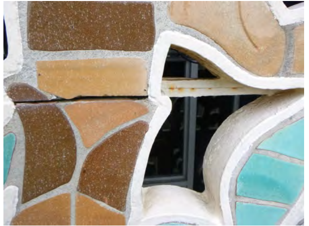
87-133 ArchMetal_Corrosion Surface 2024-2.jpg
