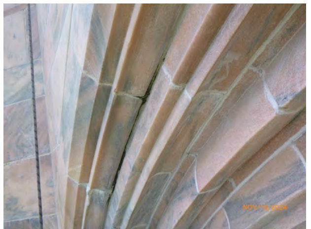
38-181 Stone_Joints Mortar Failed 2024-3.jpg
