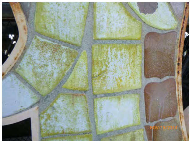
13-163 TerraCotta_Crack Single unit 2024-1.jpg
