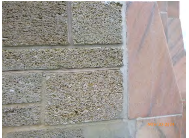
61-121 Stone_Joints Sealant Failed 2024-5.jpg
