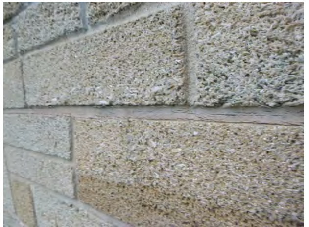
137-51 Stone_Joints Sealant Failed 2024-1.jpg
