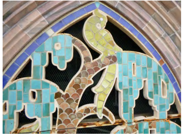
392-174 ArchMetal_Coating Coating Failed 2024-2.jpg
