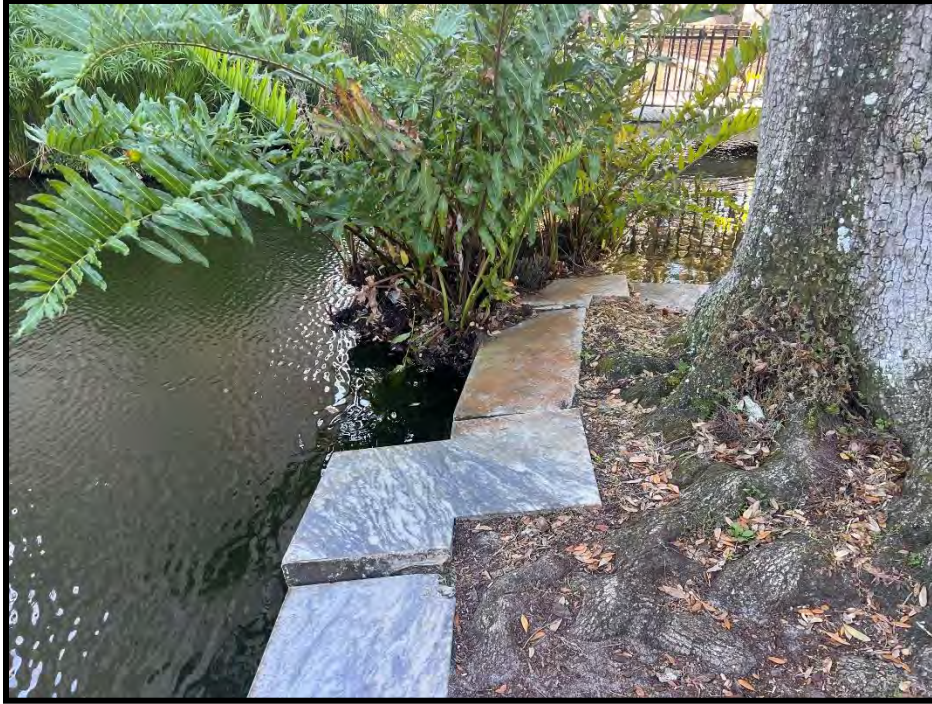
Figure 43 Displaced coping stones around the moat perimeter
