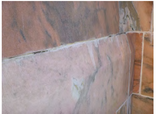
251-138 Stone_SoilStain Leached Salts 2024-1.jpg
