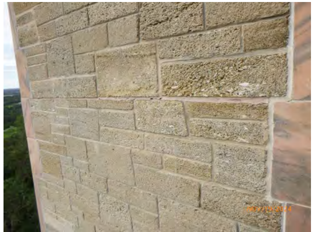
240-112 Stone_Joints Sealant Failed 2024-1.jpg
