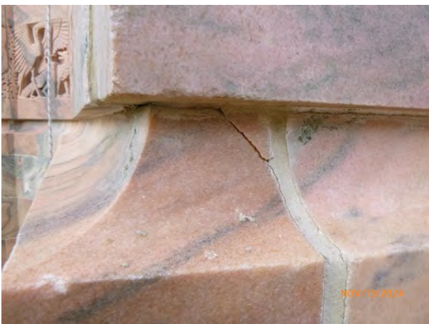
235-28 Stone_Crack Single unit 2024-1.jpg
