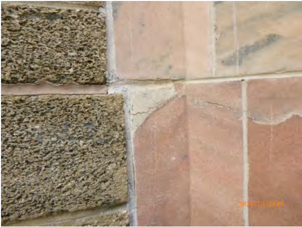
240-70 Stone_Repair Patch Failed 2024-1.jpg
