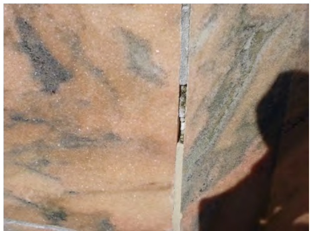
334-186 Stone_Joints Mortar Failed 2024-2.jpg
