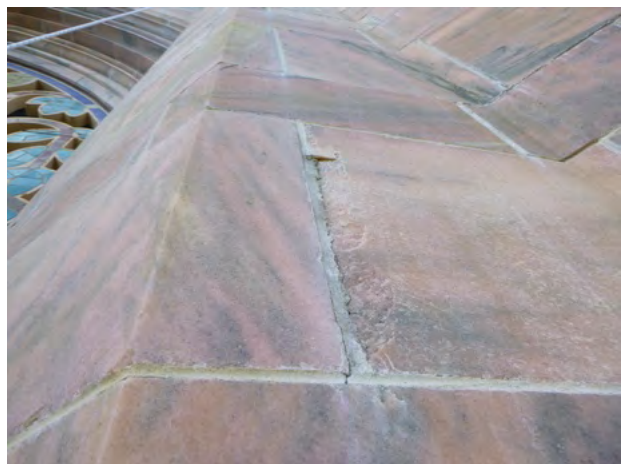
42-169 Stone_SurfLoss Chipped 2024-1.jpg
