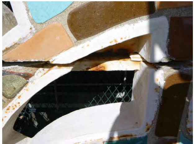
311-172 ArchMetal_Coating Coating Failed 2024-2.jpg
