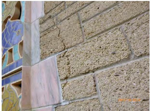
355-108 Stone_Crack System units and joints 2024-2.jpg
