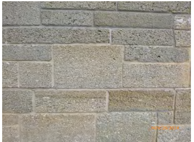
61-109 Stone_Joints Sealant Failed 2024-3.jpg
