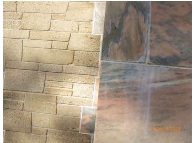
358-37 Stone_SoilStain Leached Salts 2024-2.jpg
