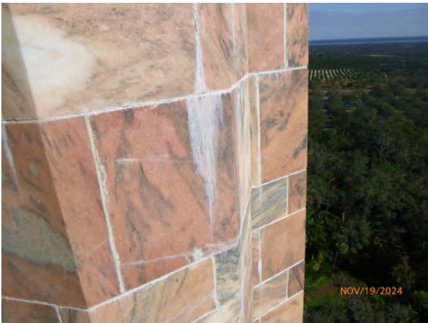
269-169 Stone_SoilStain Leached Salts 2024-1.jpg
