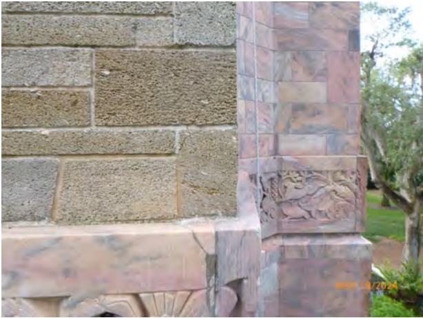
368-32 Stone_Crack Repair failed 2024-2.jpg
