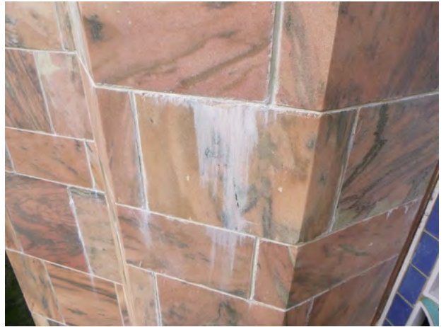
204-157 Stone_SoilStain Leached Salts 2024-2.jpg
