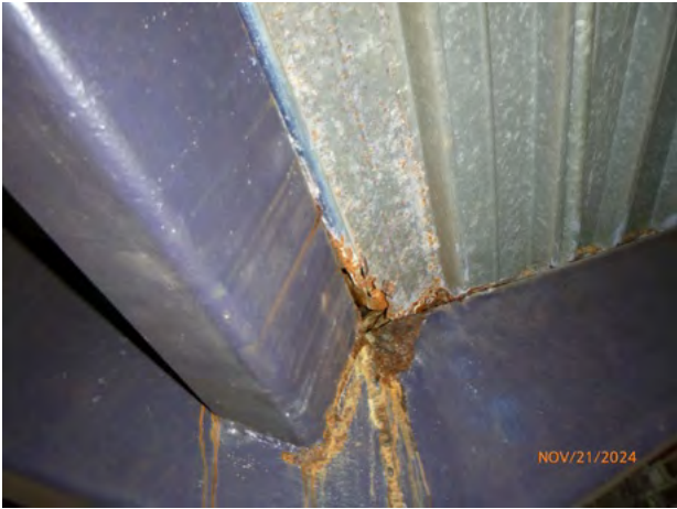
765-182 SheetMetal_Corrosion Perforated 2024-1.jpg
