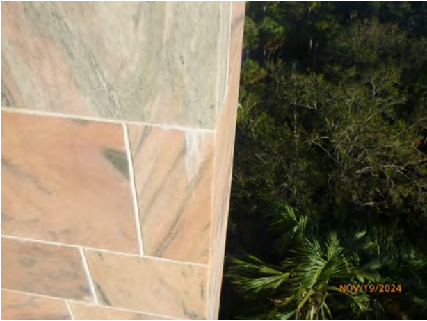
356-71 Stone_SoilStain Leached Salts 2024-2.jpg
