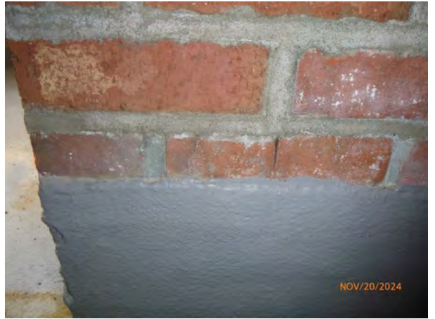
537-138 Brick_Crack Single unit 2024-1.jpg
