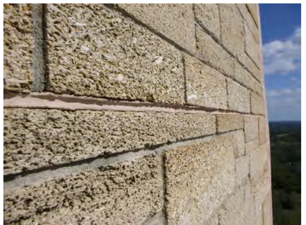
262-121 Stone_Joints Sealant Failed 2024-1.jpg
