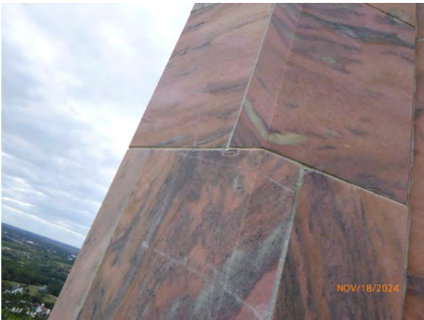
344-186 Stone_SurfLoss Chipped 2024-1.jpg
