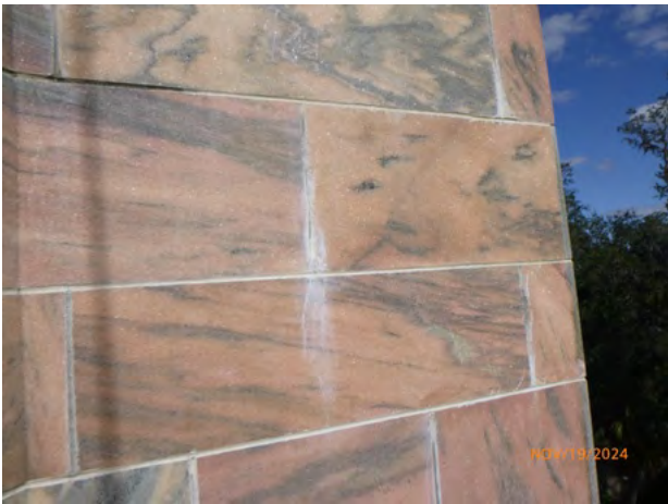
272-35 Stone_SoilStain Leached Salts 2024-2.jpg
