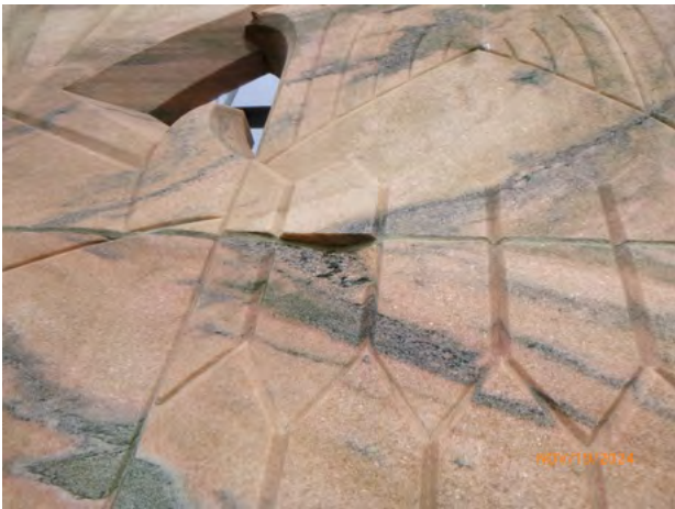
237-193 Stone_Spall Missing 2024-3.jpg
