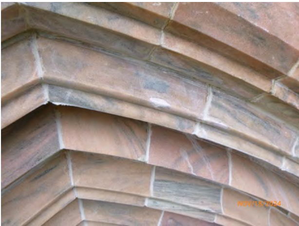
351-181 Stone_Repair Patch Failed 2024-2.jpg
