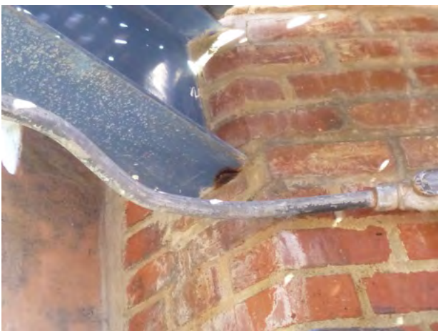
549-193 ArchMetal_Corrosion Surface 2024-2.jpg
