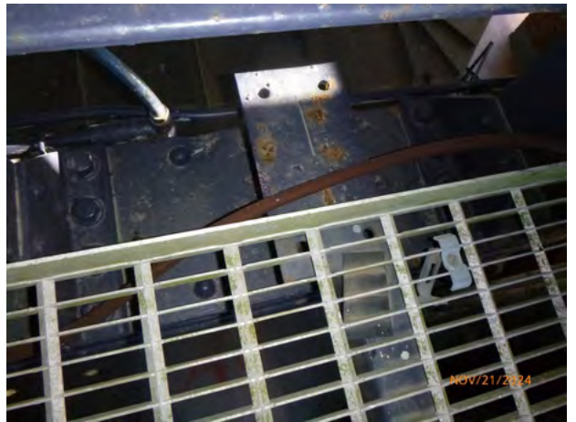
763-147 ArchMetal_Coating Coating Failed 2024-4.jpg
