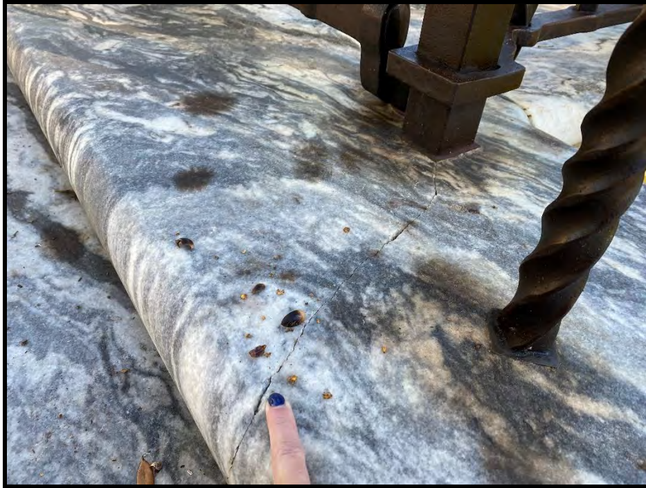
Figure 45 Crack in Creole marble steps of the moat bridge
