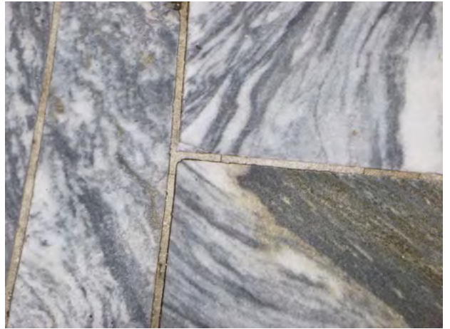
149-0 Stone_Joints Mortar Failed 2024-3.jpg
