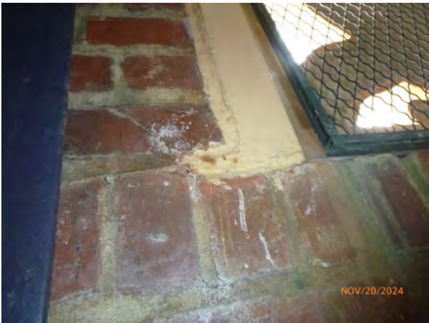
745-143 ArchMetal_Corrosion Surface 2024-1.jpg
