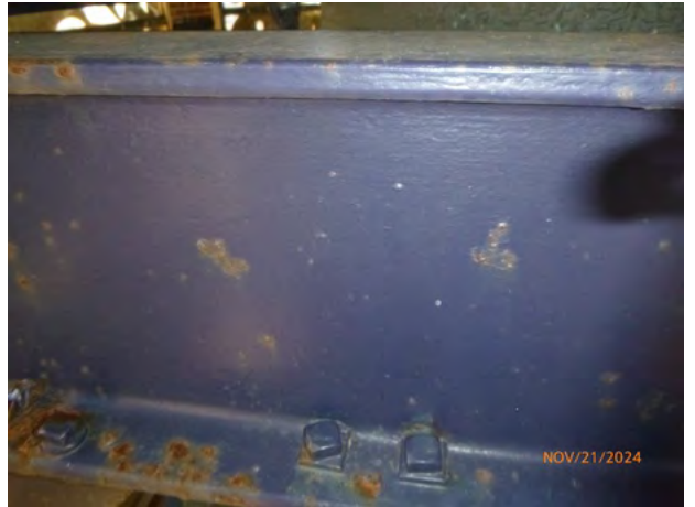
561-157 ArchMetal_Coating Coating Failed 2024-8.jpg
