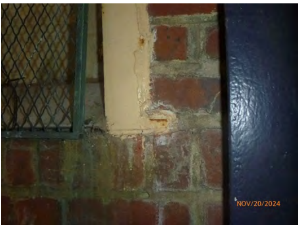
755-143 ArchMetal_Corrosion Surface 2024-2.jpg
