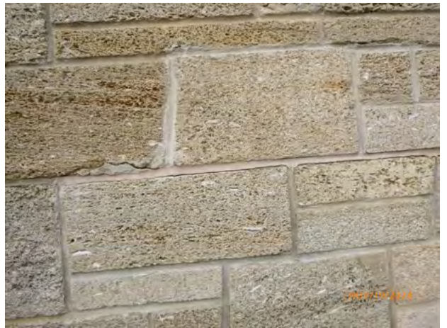
241-80 Stone_Joints Sealant Failed 2024-4.jpg
