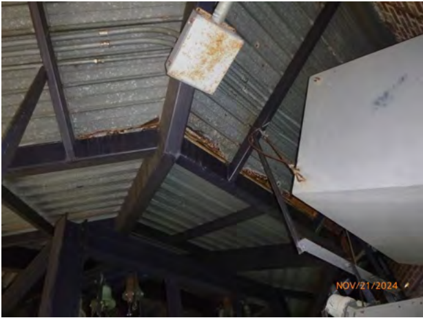
848-180 ArchMetal_Corrosion Perforated 2024-1.jpg
