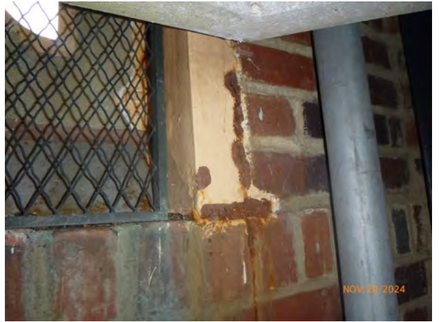
560-143 ArchMetal_Corrosion Pitted 2024-1.jpg
