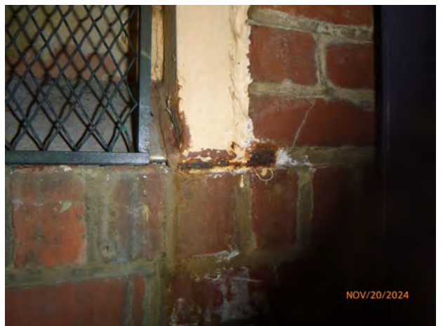
551-144 ArchMetal_Corrosion Pitted 2024-1.jpg
