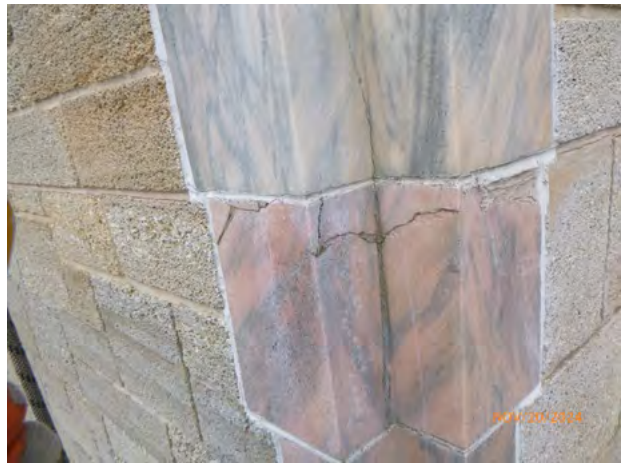
134-102 Stone_Spall Removed 2024-1.jpg
