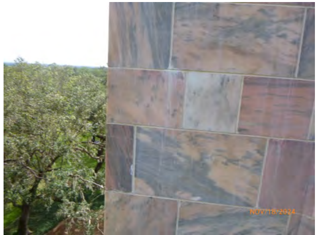
31-59 Stone_SoilStain Leached Salts 2024-1.jpg
