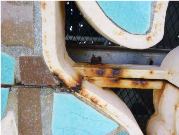
17-163 ArchMetal_Corrosion Fastener rusted 2024-1.jpg
