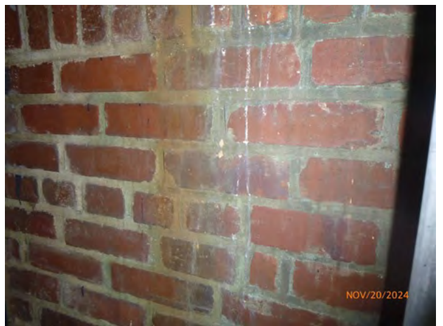
759-141 Brick_SoilStain Rust 2024-2.jpg
