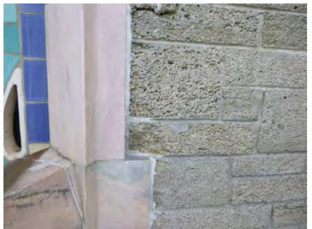
54-105 Stone_Spall Missing 2024-1.jpg
