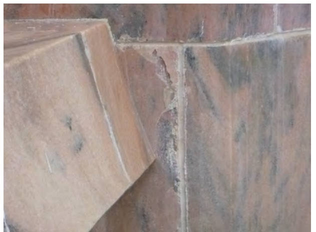
141-140 Stone_SurfLoss Chipped 2024-1.jpg
