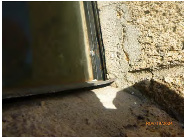
351-86 Stone_Joints Mortar Failed 2024-3.jpg
