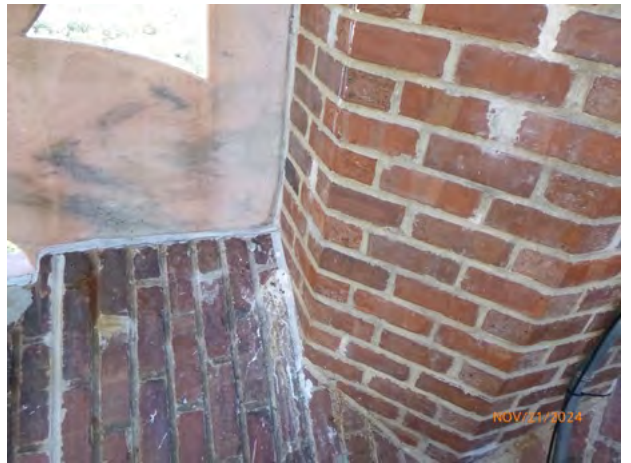
860-184 Brick_Joints Sealant Failed 2024-1.jpg
