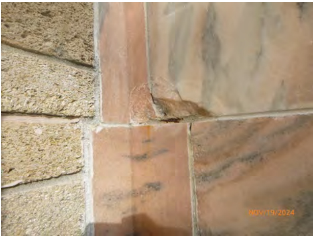
355-38 Stone_Spall Missing + Steel 2024-1.jpg
