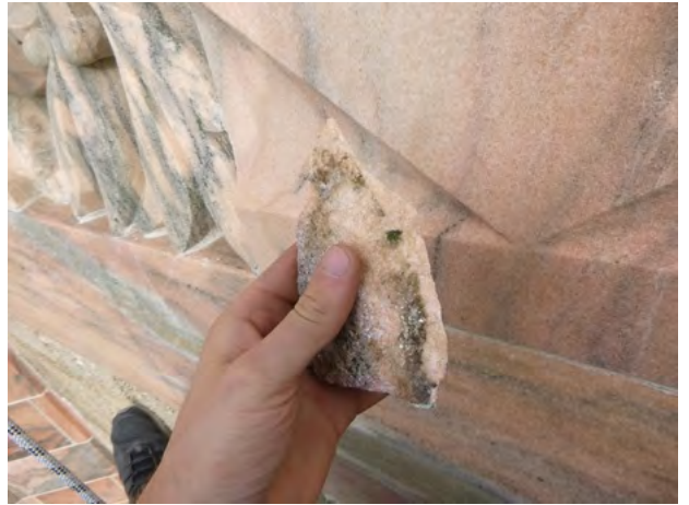
164-142 Stone_Spall Removed 2024-2.jpg
