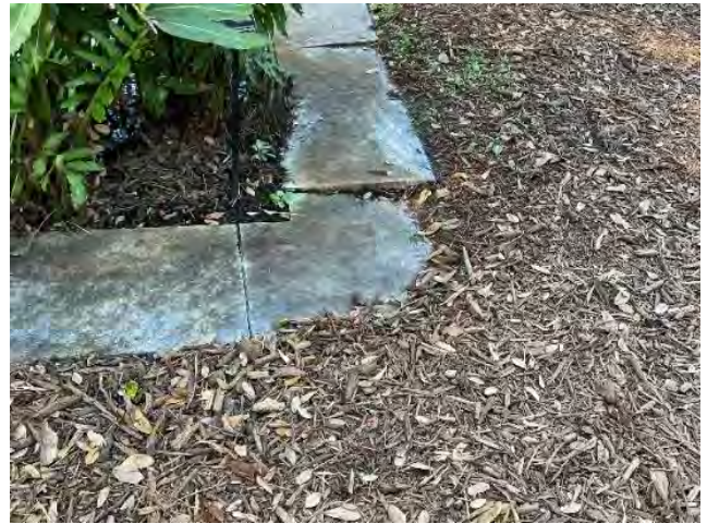
25 Moat coping stones out of plumb.
