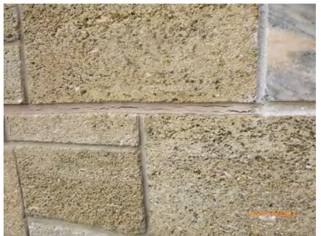
240-57 Stone_Joints Sealant Failed 2024-2.jpg
