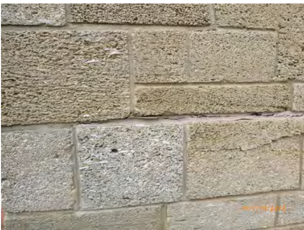
241-44 Stone_Joints Sealant Failed 2024-3.jpg
