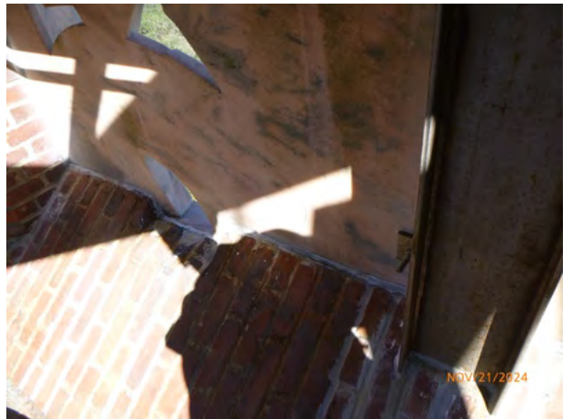
844-184 Brick_Joints Sealant Failed 2024-4.jpg
