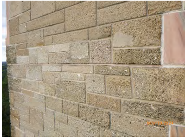
240-90 Stone_Joints Sealant Failed 2024-1.jpg
