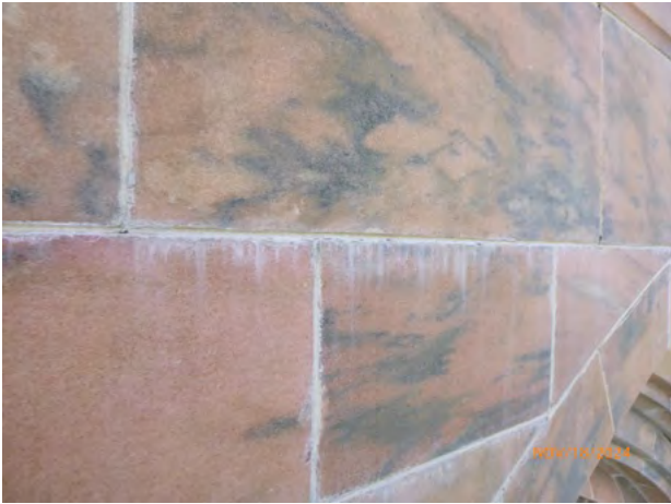
37-182 Stone_SoilStain Leached Salts 2024-2.jpg
