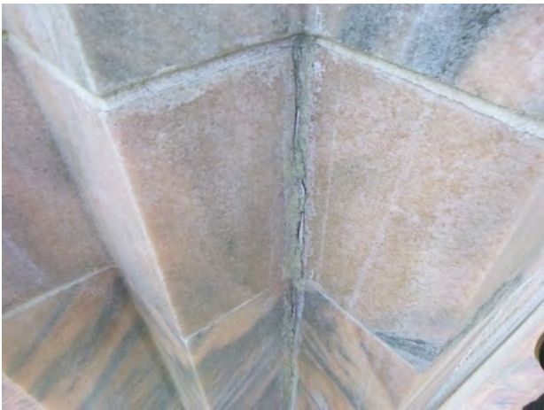
35-124 Stone_Crack Repair failed 2024-1.jpg
