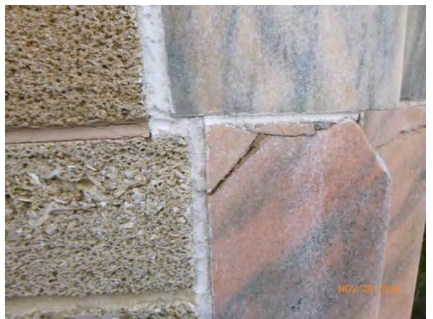
67-101 Stone_Crack Repair failed 2024-1.jpg
