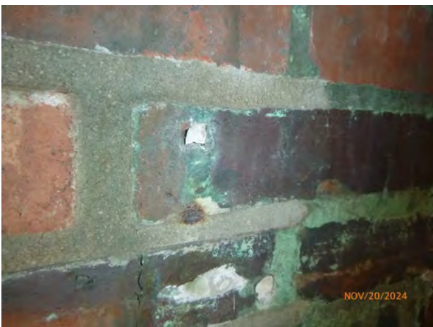
866-141 Brick_Joints Sealant Failed 2024-2.jpg
