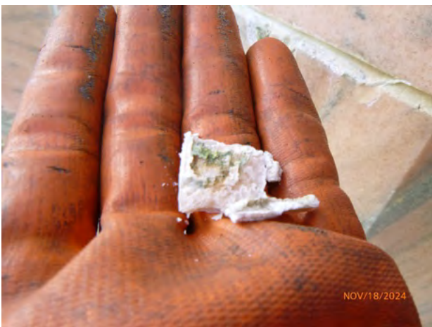
33-176 Stone_SurfLoss Chipped 2024-3.jpg
