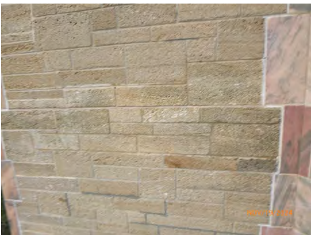
241-130 Stone_Joints Sealant Failed 2024-1.jpg
