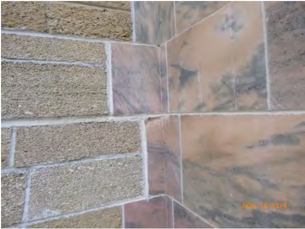
355-90 Stone_Spall Missing 2024-2.jpg
