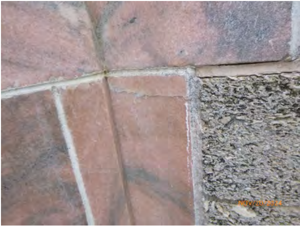
59-128 Stone_Crack Single unit 2024-1.jpg
