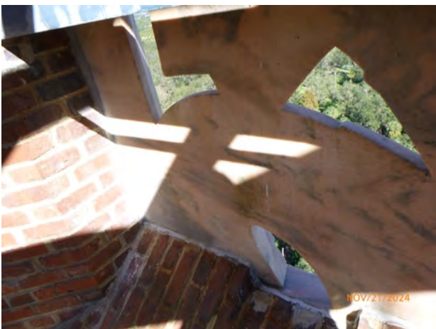
844-184 Brick_Joints Sealant Failed 2024-5.jpg
