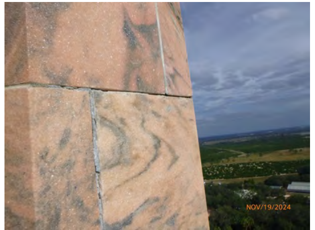
245-185 Stone_Joints Mortar Failed 2024-3.jpg
