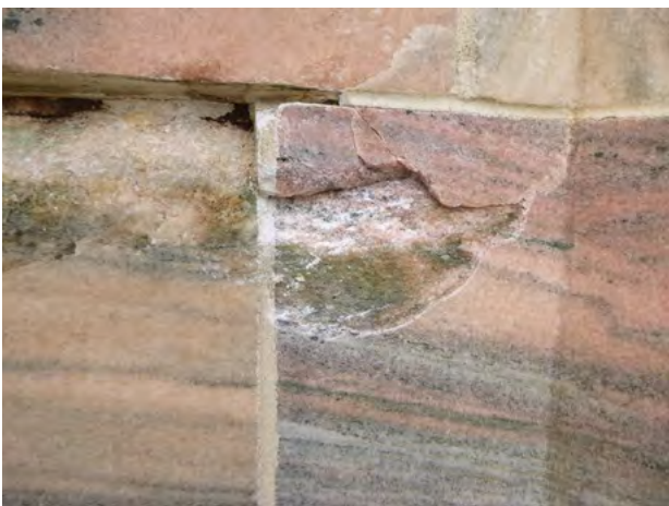
161-46 Stone_Spall Removed 2024-2.jpg
