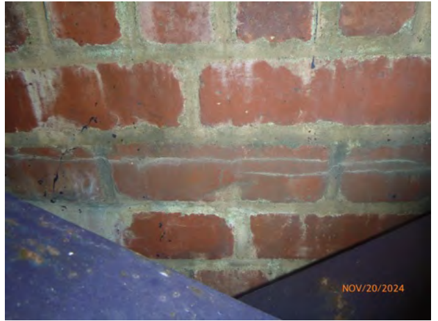
651-142 Brick_Crack System units and joints 2024-3.jpg
