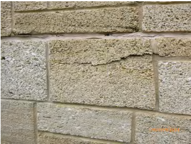
236-42 Stone_Crack Single unit 2024-1.jpg
