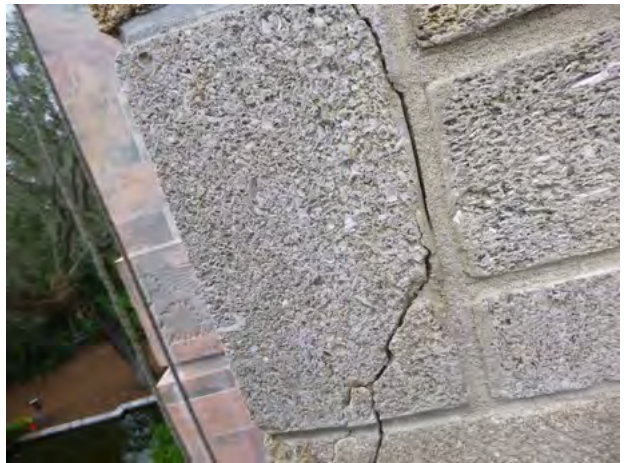
135-32 Stone_Crack System units and joints 2024-2.jpg
