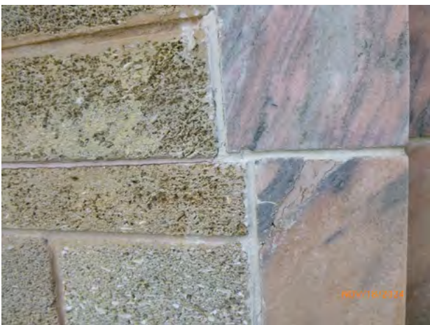
366-97 Stone_Crack Repair failed 2024-2.jpg
