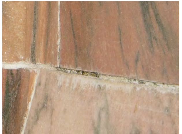
248-138 Stone_Joints Mortar Failed 2024-2.jpg
