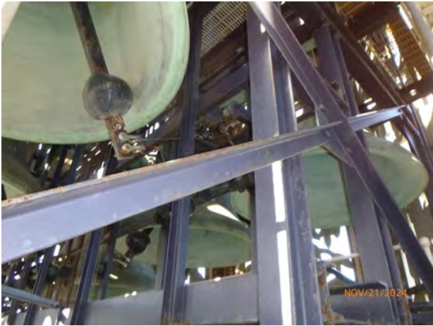
841-150 ArchMetal_Coating Coating Failed 2024-1.jpg
