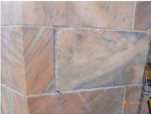
33-181 Stone_SurfLoss Chipped 2024-1.jpg
