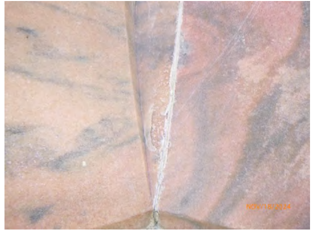
35-184 Stone_SurfLoss Chipped 2024-1.jpg
