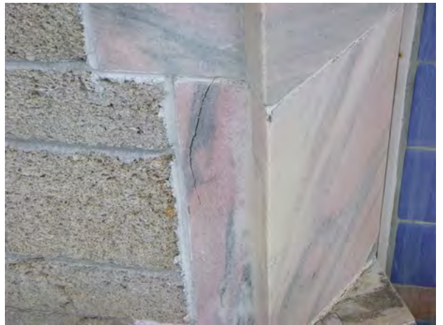
48-105 Stone_Crack Single unit 2024-1.jpg
