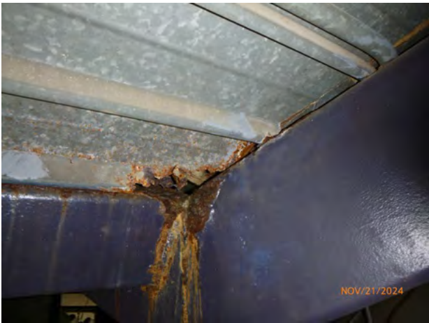
765-182 SheetMetal_Corrosion Perforated 2024-3.jpg
