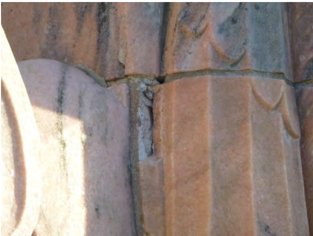
255-195 Stone_Spall Missing 2024-1.jpg
