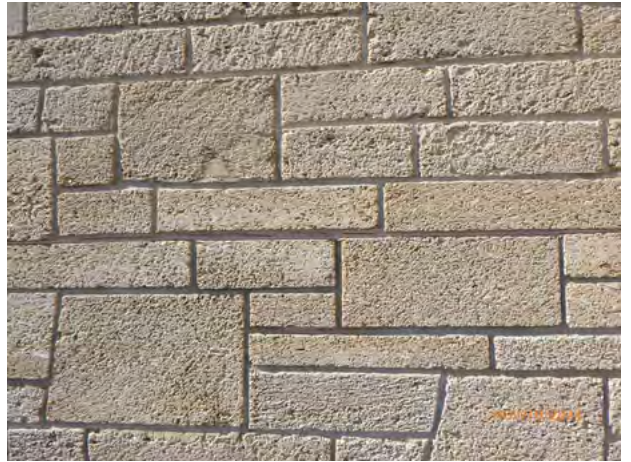
340-106 Stone_Joints Sealant Failed 2024-2.jpg
