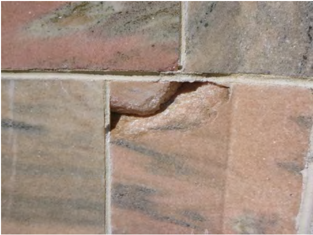
331-48 Stone_Spall Removed 2024-2.jpg
