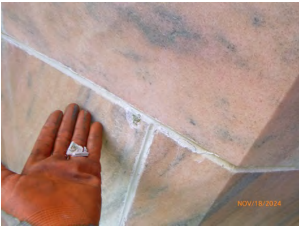
33-176 Stone_SurfLoss Chipped 2024-1.jpg
