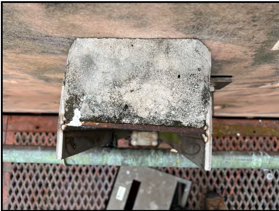
Figure 18 Minor corrosion observed at ends of stainless-steel parapet columns
