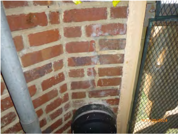
847-152 Brick_Crack System units and joints 2024-1.jpg
