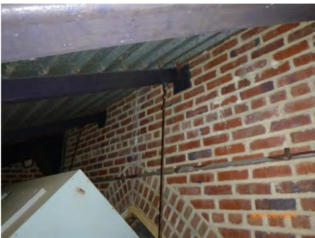
538-179 Brick_SoilStain Leached Salts 2024-1.jpg
