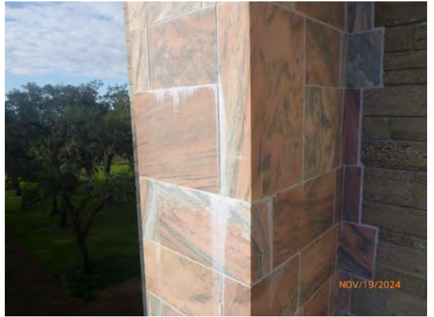
344-52 Stone_SoilStain Leached Salts 2024-1.jpg
