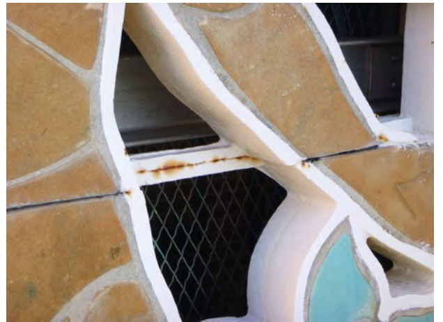
287-133 ArchMetal_Corrosion Surface 2024-2.jpg
