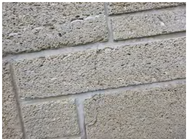
138-118 Stone_Crack System units and joints 2024-1.jpg
