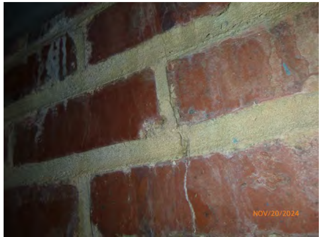
546-181 Brick_Crack System units and joints 2024-3.jpg
