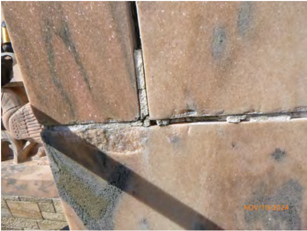
344-141 Stone_Joints Mortar Failed 2024-4.jpg
