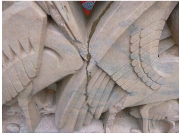
49-30 Stone_Crack Repair failed 2024-2.jpg
