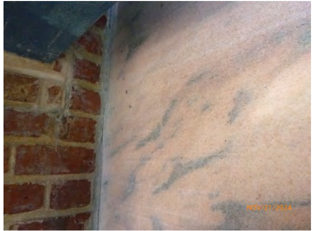
734-190 Brick_Joints Mortar Failed 2024-4.jpg
