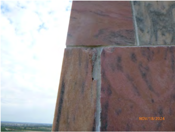
345-148 Stone_Repair Patch Failed 2024-2.jpg
