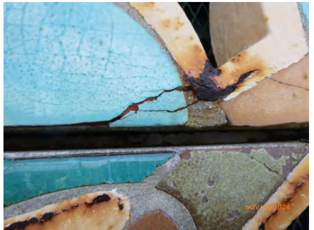
10-173 TerraCotta_Crack System units and joints 2024-1.jpg
