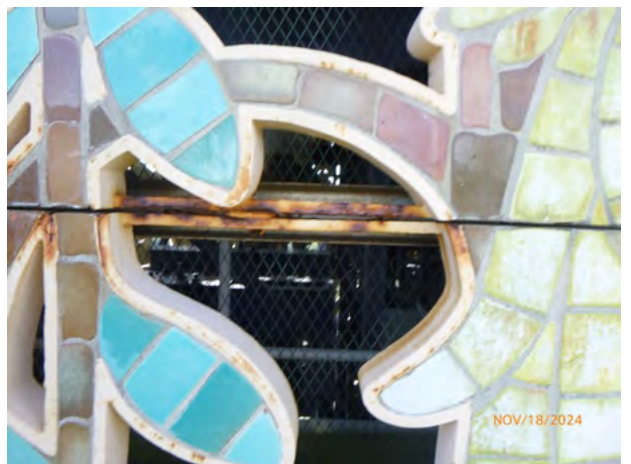
12-163 ArchMetal_Corrosion Pitted 2024-1.jpg
