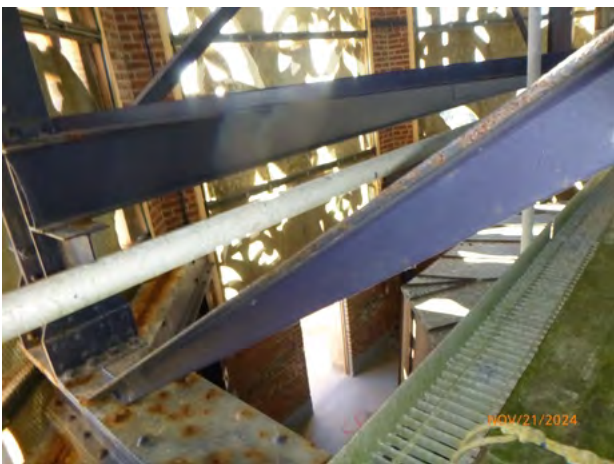
841-150 ArchMetal_Coating Coating Failed 2024-5.jpg
