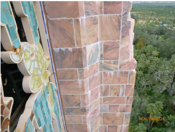
397-156 Stone_SoilStain Leached Salts 2024-1.jpg
