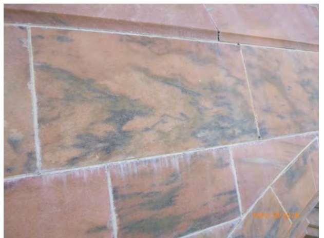
37-182 Stone_SoilStain Leached Salts 2024-1.jpg
