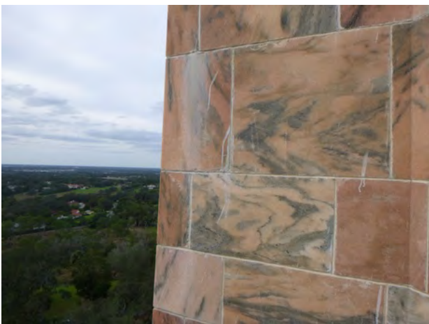
230-138 Stone_SoilStain Leached Salts 2024-1.jpg
