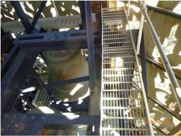
741-169 ArchMetal_Coating Coating Failed 2024-4.jpg
