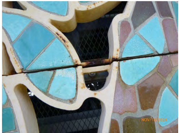
12-168 ArchMetal_Corrosion Pitted 2024-2.jpg
