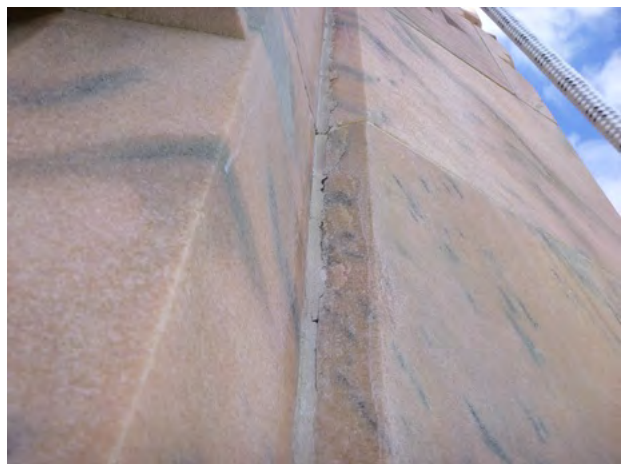
41-190 Stone_SurfLoss Chipped 2024-1.jpg
