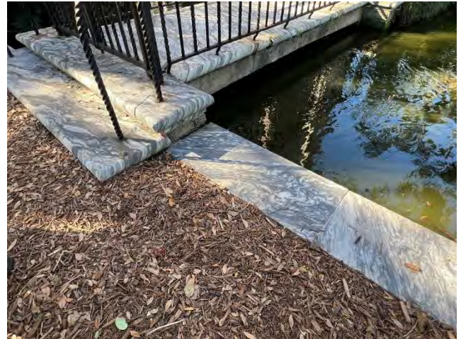
23 Cracked stone at moat edge.
