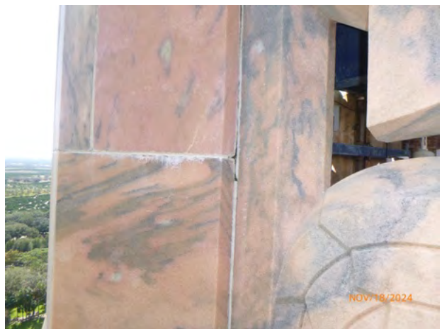
36-185 Stone_Joints Mortar Failed 2024-4.jpg
