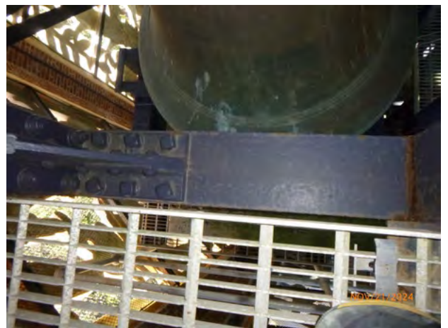
562-170 ArchMetal_Coating Coating Failed 2024-6.jpg
