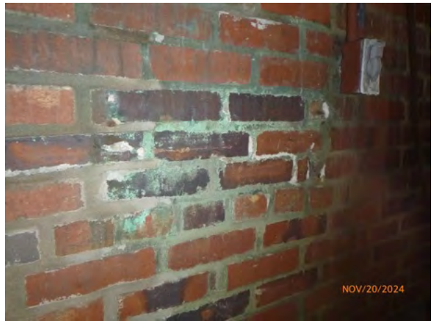
866-141 Brick_Joints Sealant Failed 2024-1.jpg
