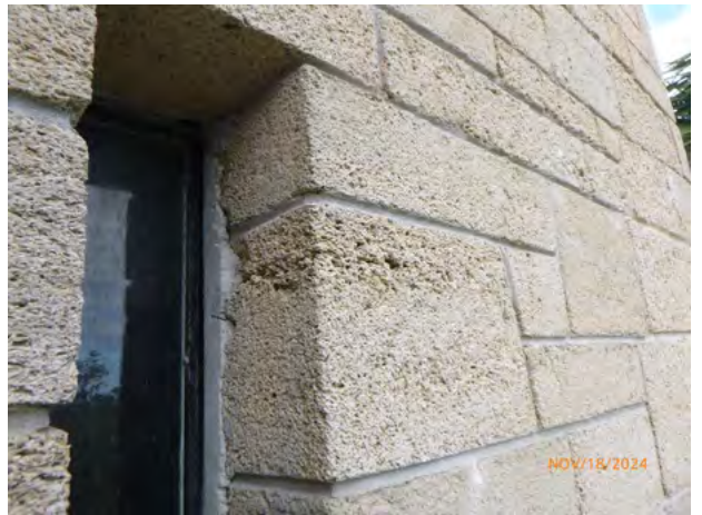
34-56 Stone_Joints Mortar Failed 2024-3.jpg
