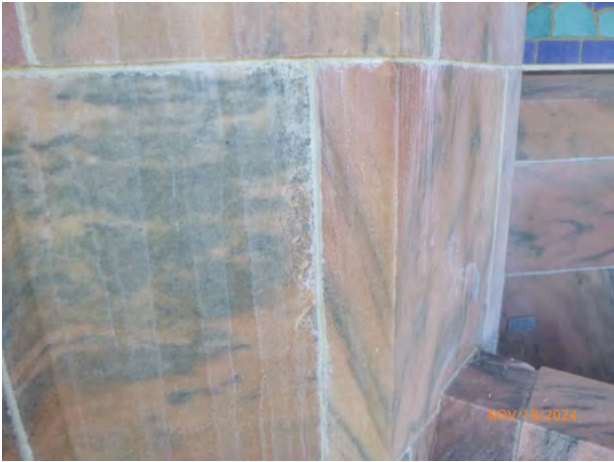
33-142 Stone_SurfLoss Chipped 2024-1.jpg
