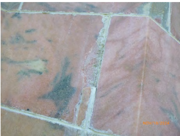
35-163 Stone_Spall Missing 2024-3.jpg
