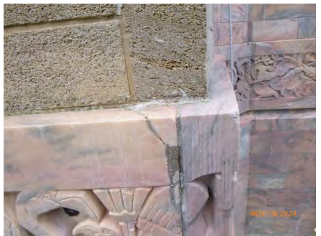
368-32 Stone_Crack Repair failed 2024-1.jpg
