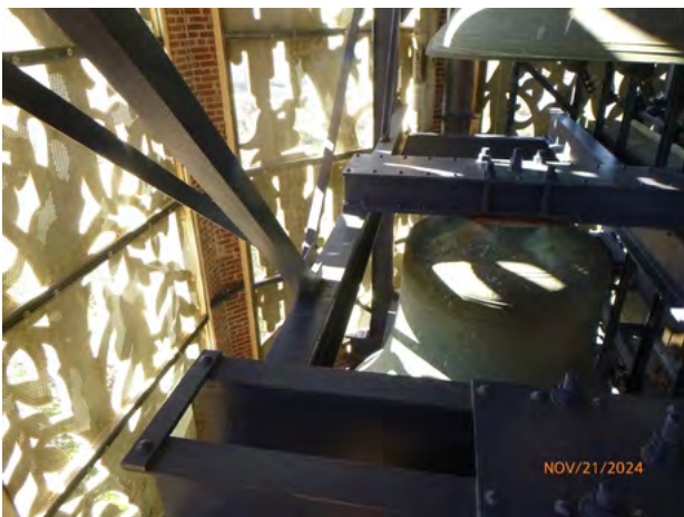
743-157 ArchMetal_Coating Coating Failed 2024-3.jpg
