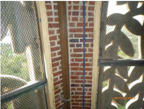
656-168 Brick_SurfLoss Face spalled 2024-1.jpg
