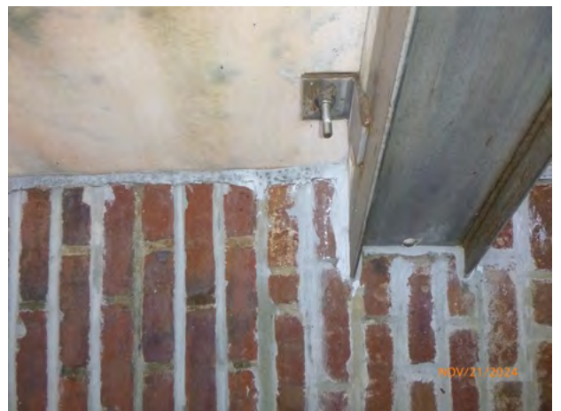
741-184 Brick_Joints Sealant Failed 2024-4.jpg
