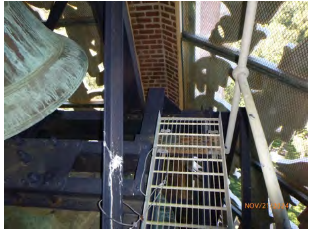
538-170 ArchMetal_Coating Coating Failed 2024-2.jpg
