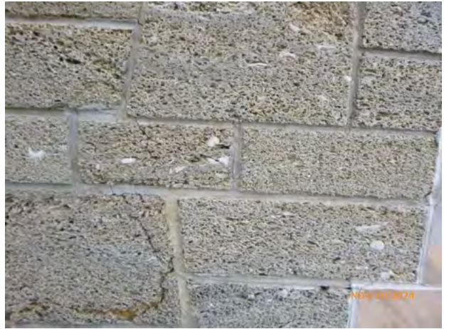
65-116 Stone_Crack System units and joints 2024-6.jpg
