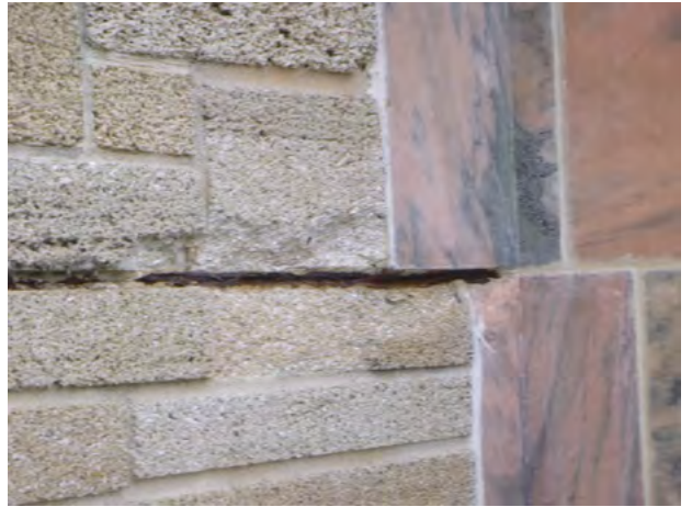
154-91 Stone_Spall Missing + Steel 2024-1.jpg
