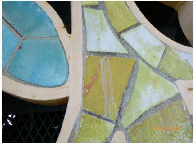
13-175 TerraCotta_Crack Single unit 2024-1.jpg
