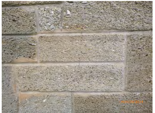
66-77 Stone_Crack Single unit 2024-3.jpg
