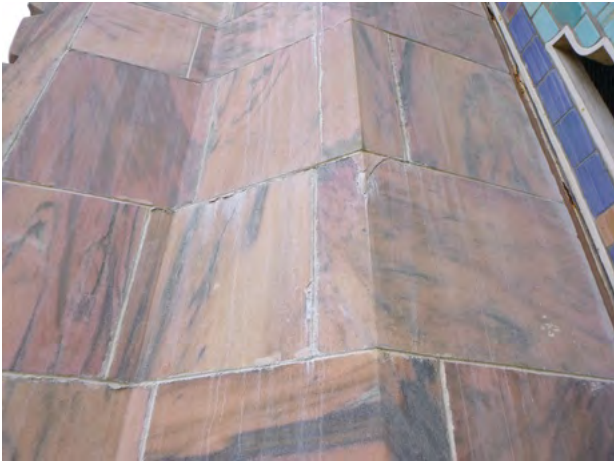
80-162 Stone_SoilStain Leached Salts 2024-1.jpg
