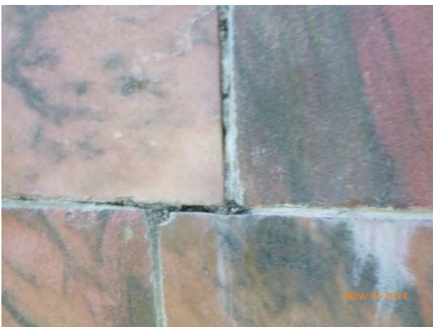
31-158 Stone_Joints Mortar Failed 2024-5.jpg
