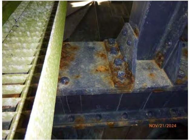
844-147 ArchMetal_Corrosion Fastener rusted 2024-3.jpg
