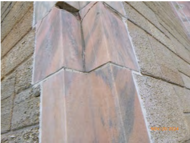
136-101 Stone_Crack Repair failed 2024-2.jpg
