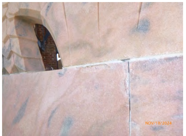
37-184 Stone_SurfLoss Chipped 2024-2.jpg
