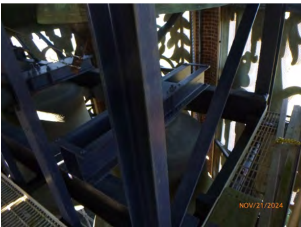
559-162 ArchMetal_Coating Coating Failed 2024-2.jpg
