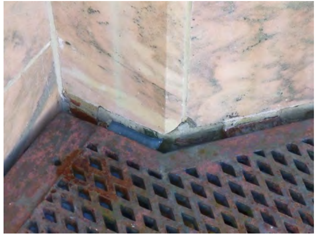
866-193 Stone_Joints Mortar Failed 2024-1.jpg
