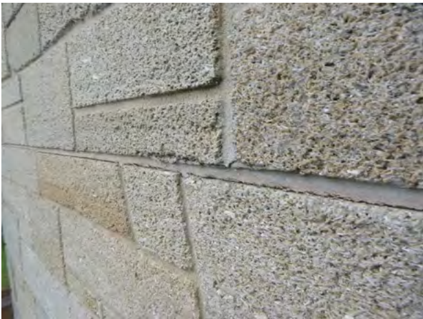
137-42 Stone_Joints Sealant Failed 2024-1.jpg
