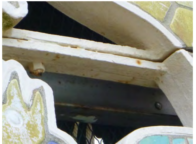
186-168 ArchMetal_Corrosion Surface 2024-2.jpg
