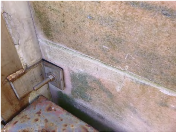
545-193 Stone_Repair Patch Failed 2024-1.jpg
