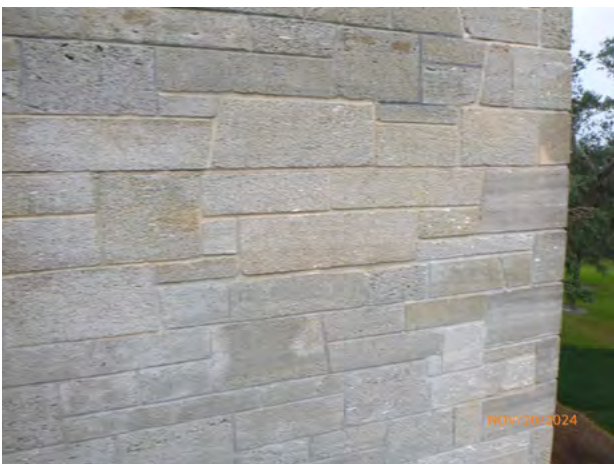
62-46 Stone_Joints Sealant Failed 2024-1.jpg
