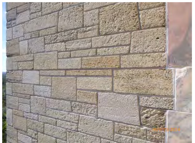
340-80 Stone_Joints Sealant Failed 2024-1.jpg
