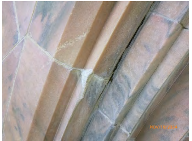
37-180 Stone_SoilStain Leached Salts 2024-1.jpg
