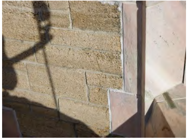
247-104 Stone_Crack System units and joints 2024-2.jpg
