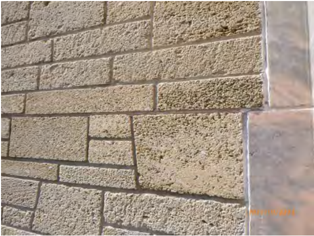
340-106 Stone_Joints Sealant Failed 2024-1.jpg
