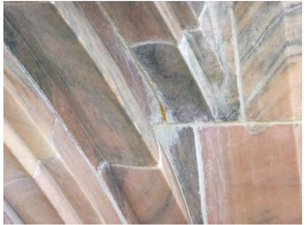
187-180 Stone_SoilStain Leached Salts 2024-3.jpg
