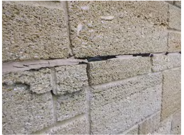
150-90 Stone_Joints Sealant Failed 2024-2.jpg
