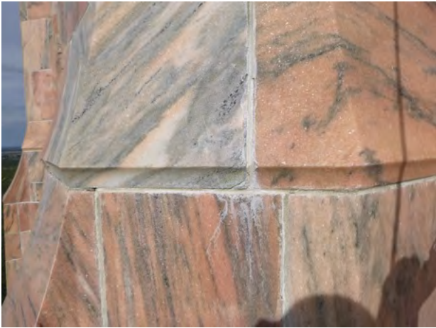
234-183 Stone_SoilStain Leached Salts 2024-1.jpg
