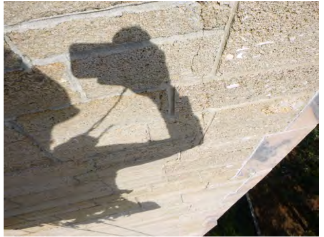
264-132 Stone_Crack System units and joints 2024-2.jpg
