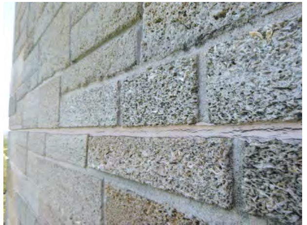
37-90 Stone_Joints Sealant Failed 2024-1.jpg
