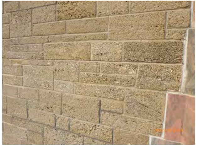
240-122 Stone_Joints Sealant Failed 2024-1.jpg
