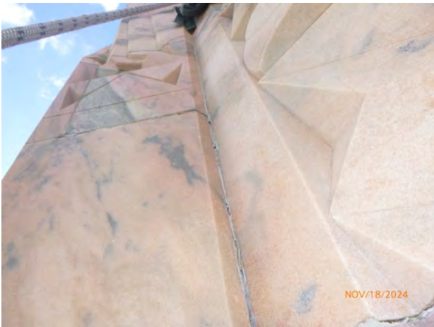
36-185 Stone_Joints Mortar Failed 2024-1.jpg
