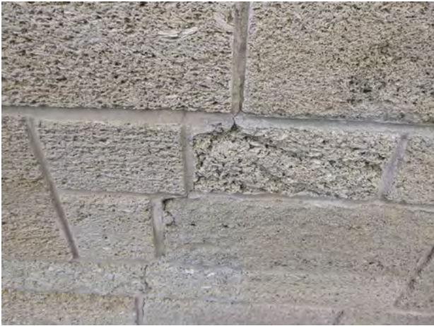
138-118 Stone_Crack System units and joints 2024-2.jpg
