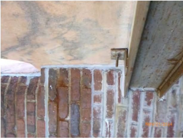
860-184 Brick_Joints Sealant Failed 2024-4.jpg
