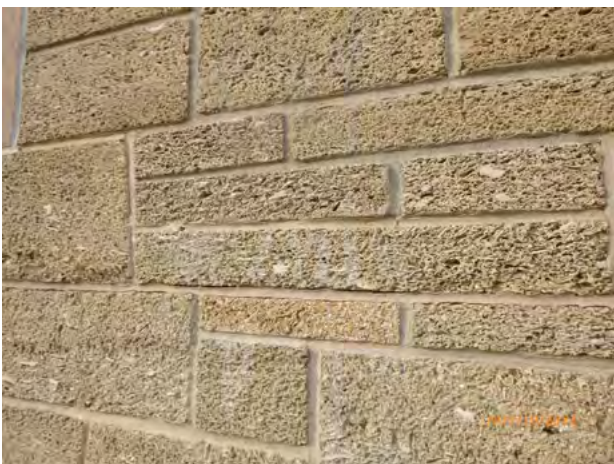
240-122 Stone_Joints Sealant Failed 2024-4.jpg
