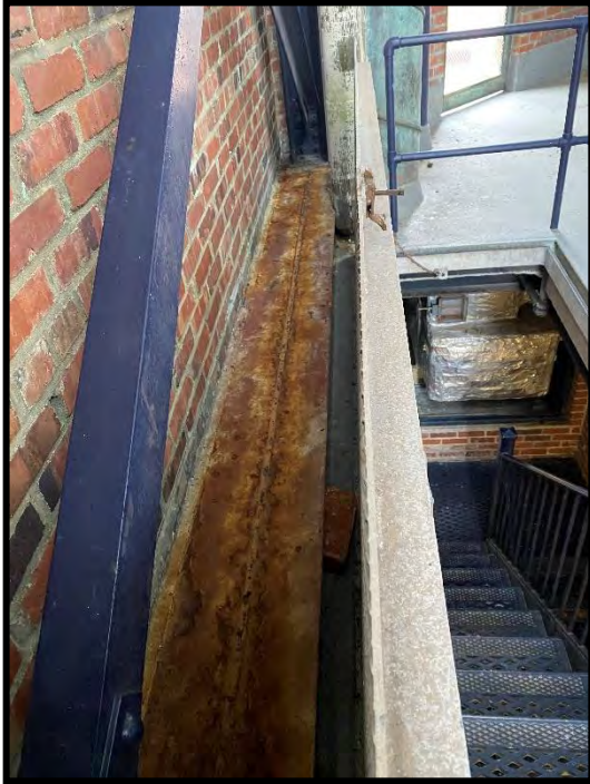
Figure 28 Corrosion of Carillon framing transfer girder at Level 7.
