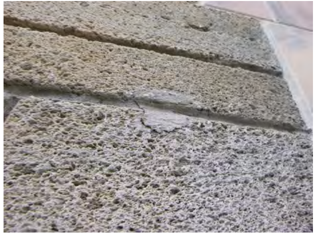
138-17 Stone_Repair Patch Failed 2024-1.jpg
