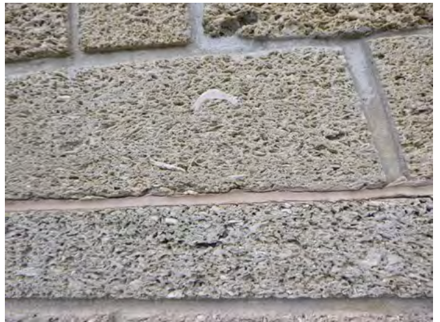
139-128 Stone_Joints Sealant Failed 2024-1.jpg
