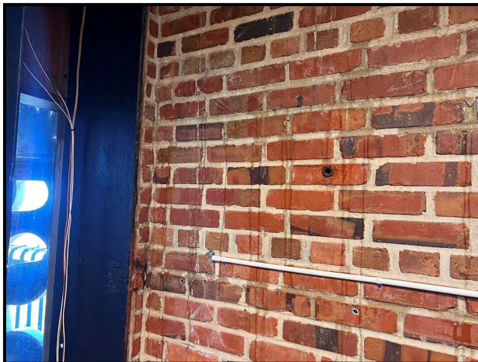
Figure 11 Leaks on the interior masonry aligned with the spray rackVisual Conditions Assessment
