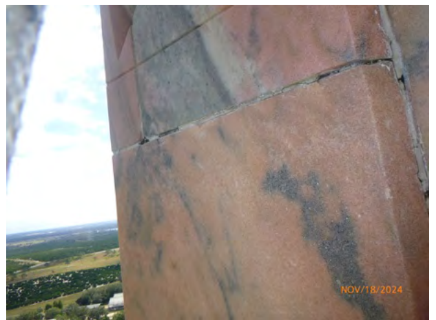
35-191 Stone_Joints Mortar Failed 2024-3.jpg
