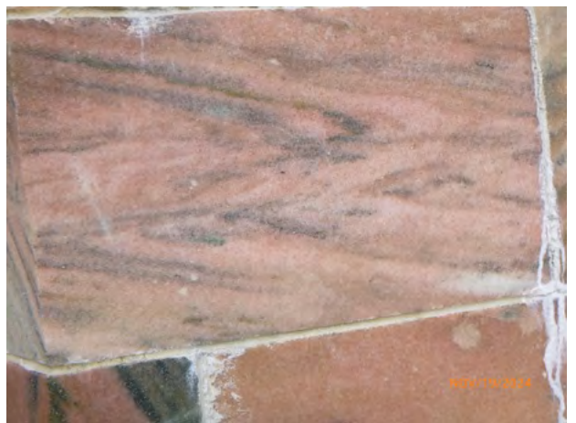
242-164 Stone_SoilStain Leached Salts 2024-3.jpg
