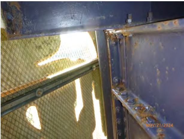
561-157 ArchMetal_Coating Coating Failed 2024-9.jpg
