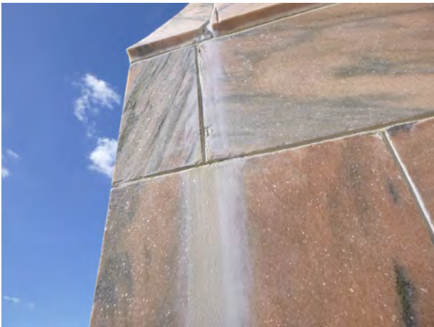
330-115 Stone_SoilStain Leached Salts 2024-1.jpg
