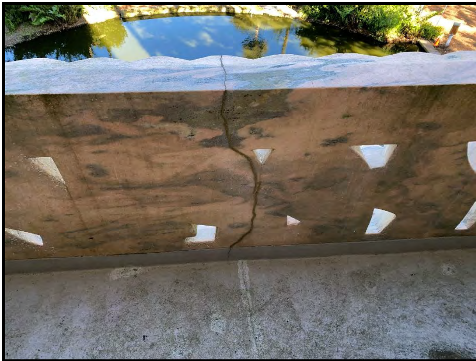
Figure 34 Crack in stone guardrail at 2 nd level balcony
