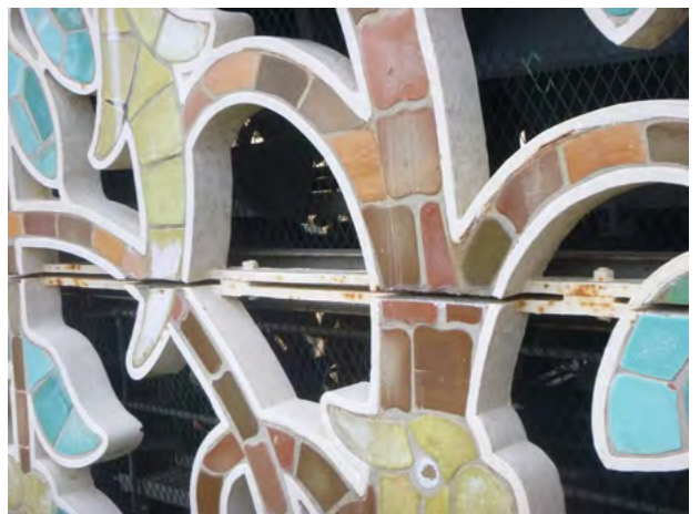
114-172 ArchMetal_Corrosion Surface 2024-1.jpg
