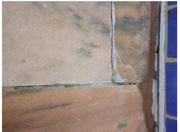
336-174 Stone_Joints Mortar Failed 2024-2.jpg
