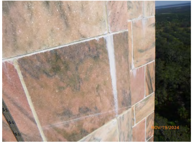
342-175 Stone_SoilStain Leached Salts 2024-1.jpg
