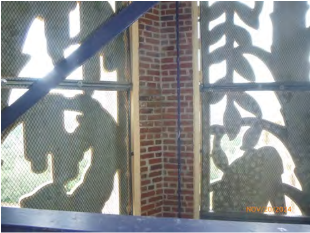
858-151 Brick_Repair Patch Failed 2024-1.jpg
