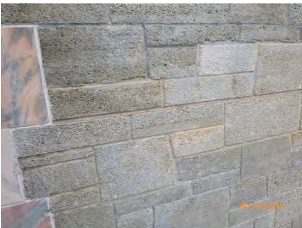
61-59 Stone_Joints Sealant Failed 2024-1.jpg
