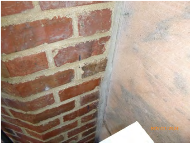
734-190 Brick_Joints Mortar Failed 2024-3.jpg
