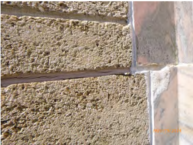
340-80 Stone_Joints Sealant Failed 2024-4.jpg
