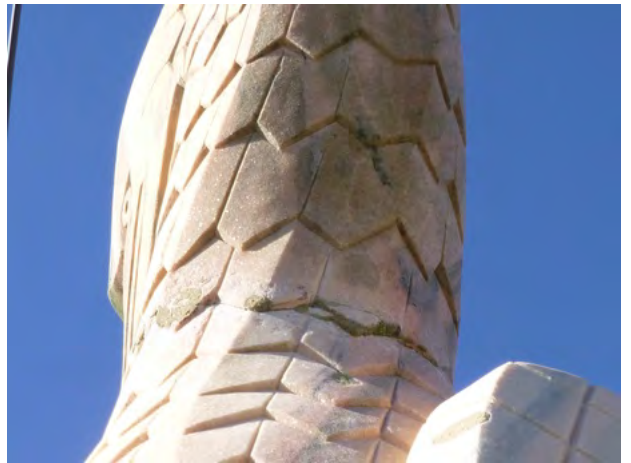
644-206 Stone_Crack Repair failed 2024-1.jpg
