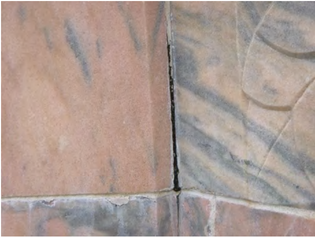
45-185 Stone_Joints Mortar Failed 2024-1.jpg
