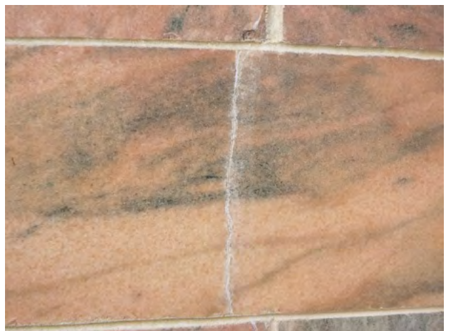
230-51 Stone_Crack System units and joints 2024-1.jpg
