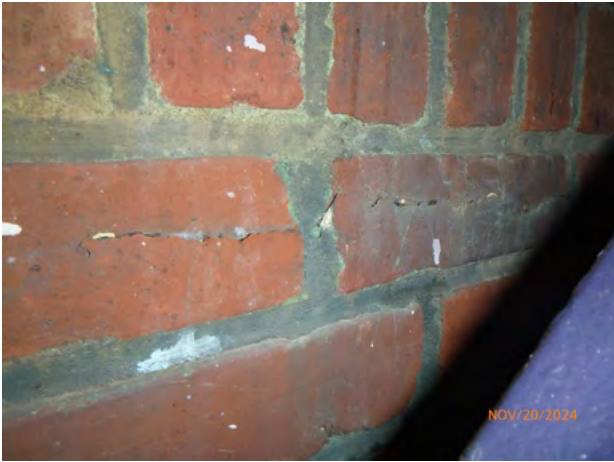
547-143 Brick_Crack System units and joints 2024-3.jpg
