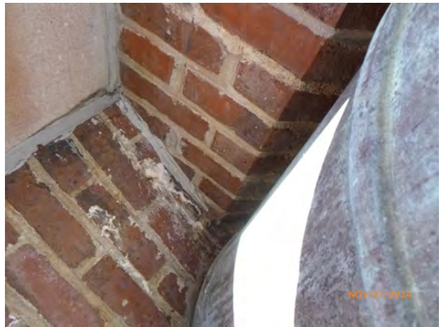
757-184 Brick_Joints Sealant Failed 2024-1.jpg
