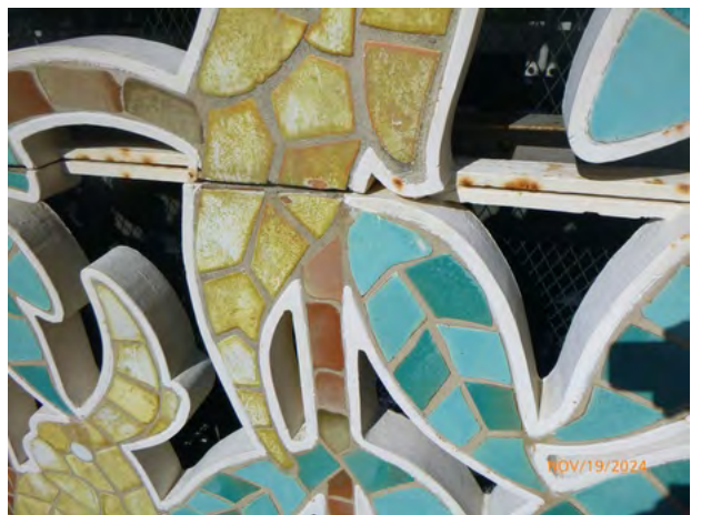
315-168 TerraCotta_SurfLoss Glaze loss 2024-1.jpg
