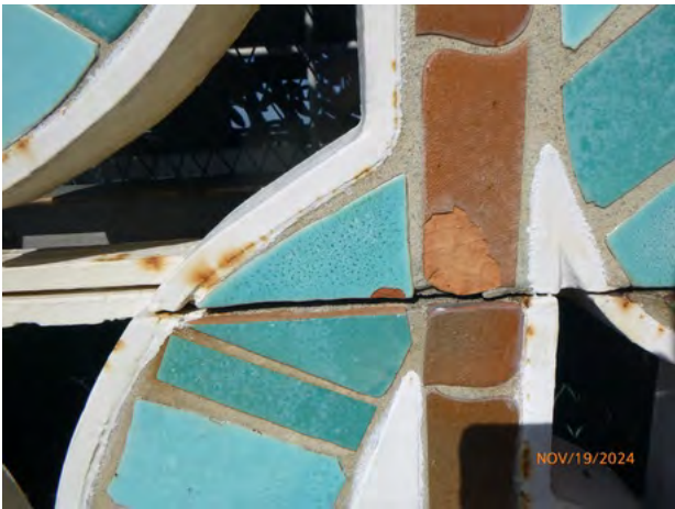
317-168 TerraCotta_SurfLoss Glaze loss 2024-2.jpg
