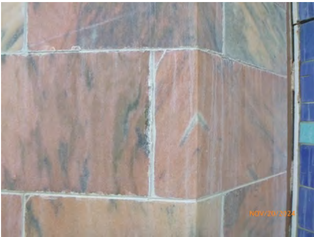
137-157 Stone_SurfLoss Chipped 2024-1.jpg
