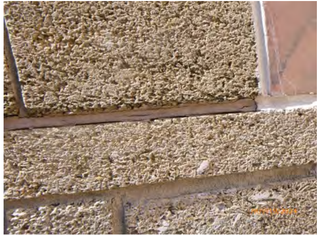
341-45 Stone_Joints Sealant Failed 2024-2.jpg
