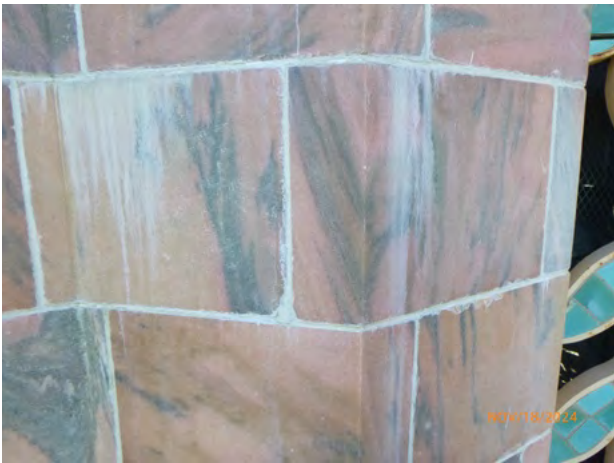
32-157 Stone_SurfLoss Chipped 2024-2.jpg
