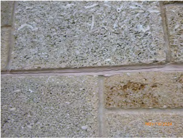
361-96 Stone_Joints Sealant Failed 2024-3.jpg
