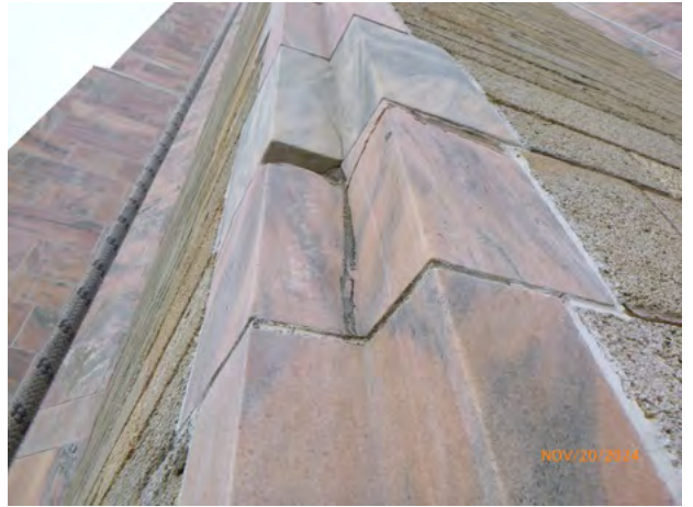
136-101 Stone_Crack Repair failed 2024-1.jpg
