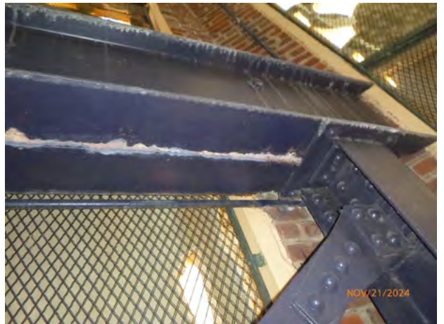
861-145 ArchMetal_Coating Coating Failed 2024-1.jpg
