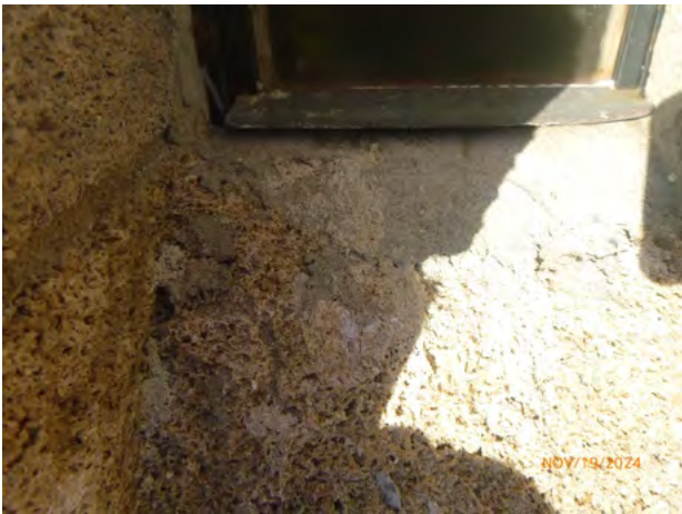
351-86 Stone_Joints Mortar Failed 2024-2.jpg
