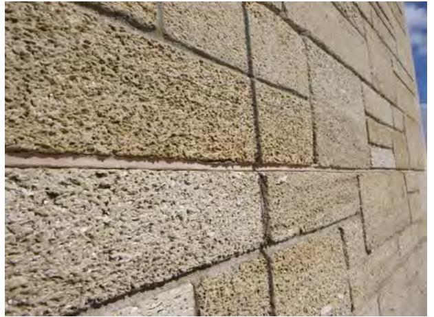
263-100 Stone_Joints Sealant Failed 2024-1.jpg
