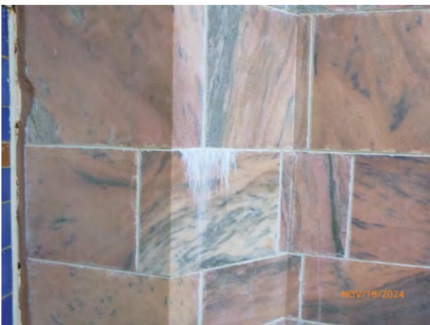
357-152 Stone_SoilStain Leached Salts 2024-1.jpg
