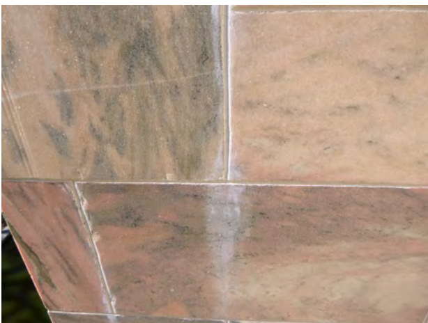
329-32 Stone_SoilStain Leached Salts 2024-1.jpg
