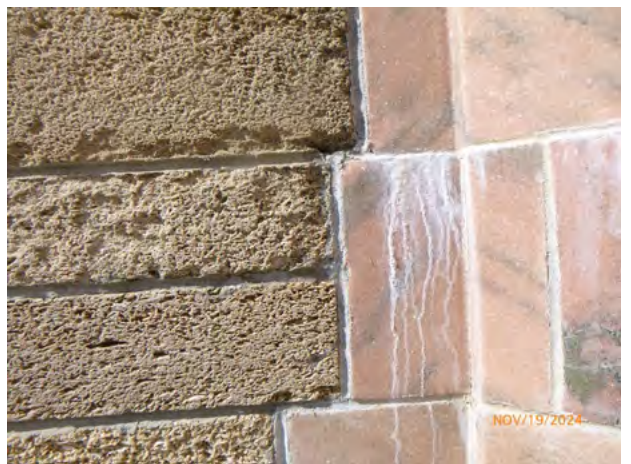
342-131 Stone_SoilStain Leached Salts 2024-2.jpg
