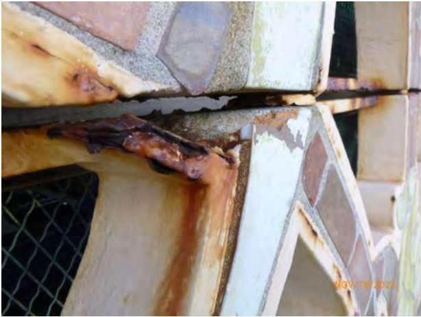
13-173 TerraCotta_Spall Missing 2024-3.jpg
