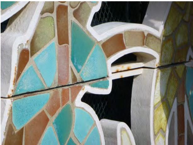
313-168 ArchMetal_Corrosion Surface 2024-1.jpg
