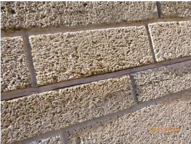
341-45 Stone_Joints Sealant Failed 2024-3.jpg
