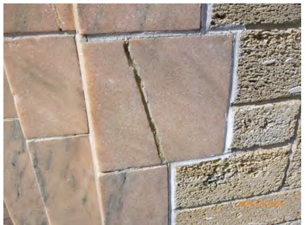
336-132 Stone_Crack Repair failed 2024-1.jpg
