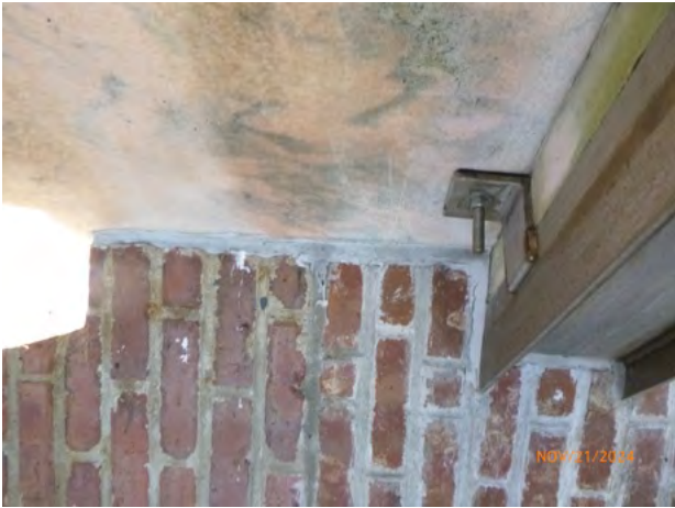
757-184 Brick_Joints Sealant Failed 2024-4.jpg
