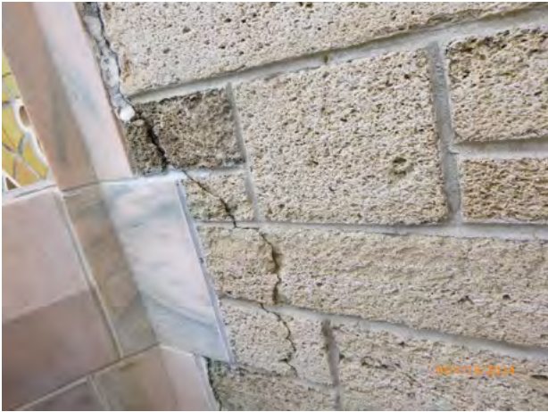
355-108 Stone_Crack System units and joints 2024-5.jpg
