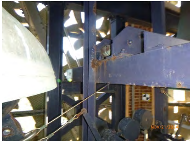
664-151 ArchMetal_Coating Coating Failed 2024-1.jpg
