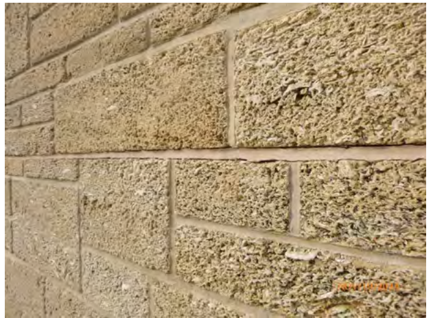
240-122 Stone_Joints Sealant Failed 2024-3.jpg
