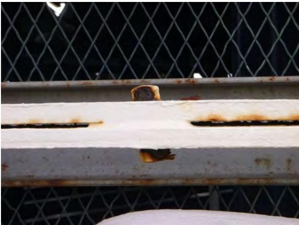
85-154 ArchMetal_Corrosion Fastener rusted 2024-1.jpg
