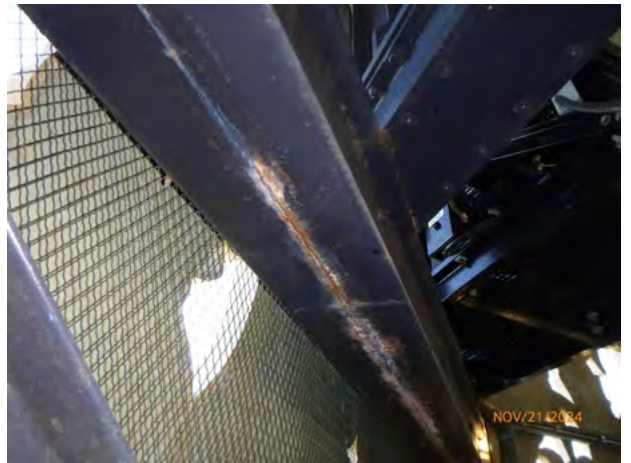
657-144 ArchMetal_Coating Coating Failed 2024-5.jpg
