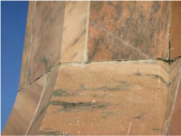
245-184 Stone_Joints Mortar Failed 2024-1.jpg
