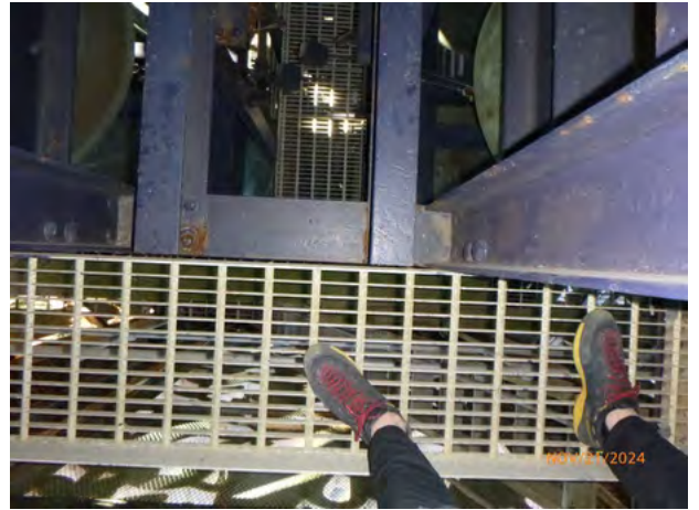
562-170 ArchMetal_Coating Coating Failed 2024-2.jpg
