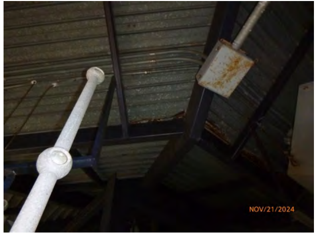
848-180 ArchMetal_Corrosion Perforated 2024-2.jpg
