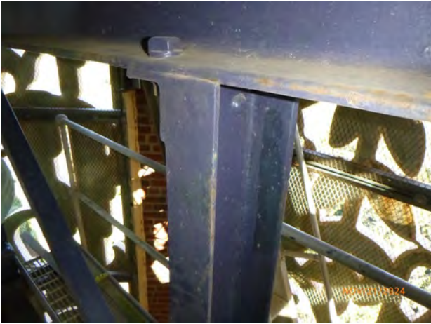
559-162 ArchMetal_Coating Coating Failed 2024-4.jpg
