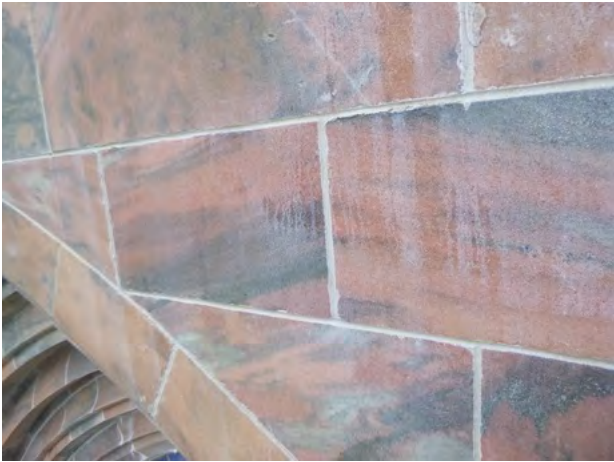
141-182 Stone_SoilStain Leached Salts 2024-1.jpg
