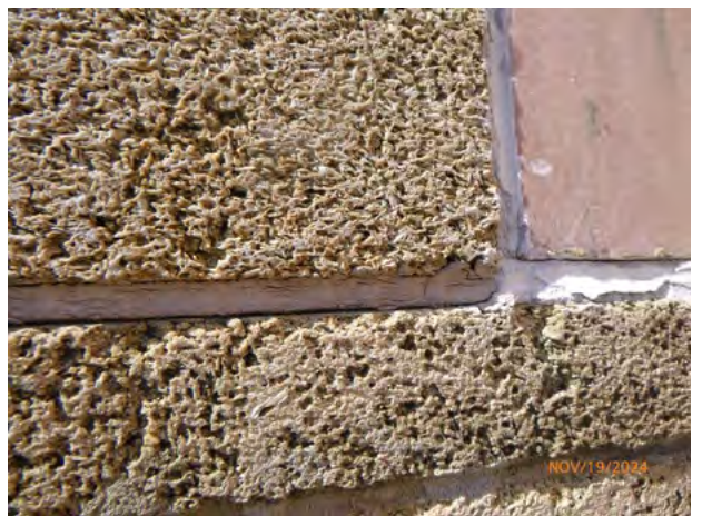
341-89 Stone_Joints Sealant Failed 2024-3.jpg
