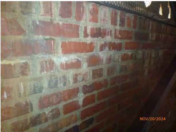
646-139 Brick_SoilStain Leached Salts 2024-2.jpg
