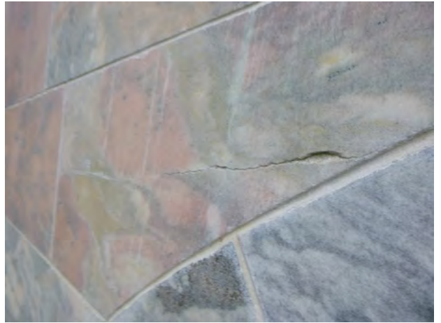
48-14 Stone_Crack Single unit 2024-1.jpg
