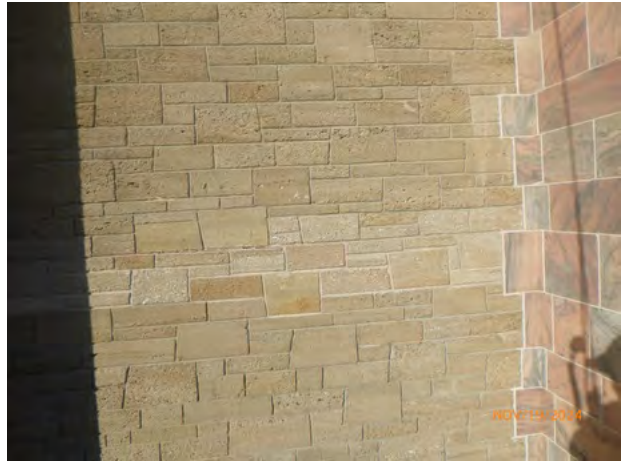
355-68 Stone_Joints Sealant Failed 2024-3.jpg
