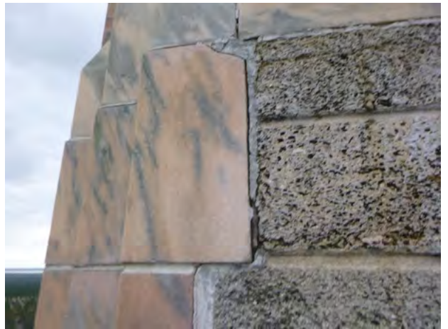
135-133 Stone_Joints Mortar Failed 2024-1.jpg
