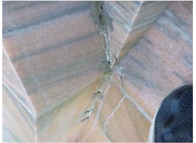
35-122 Stone_Crack Repair failed 2024-2.jpg
