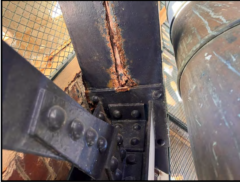
Figure 30 Close up view of deterioration of Carillon framing
