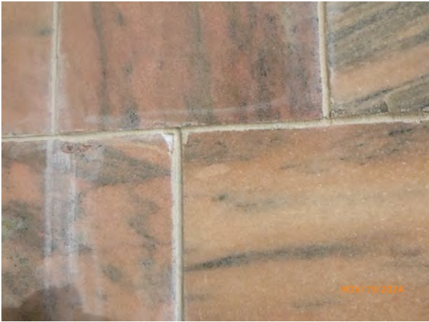
357-45 Stone_SoilStain Leached Salts 2024-4.jpg
