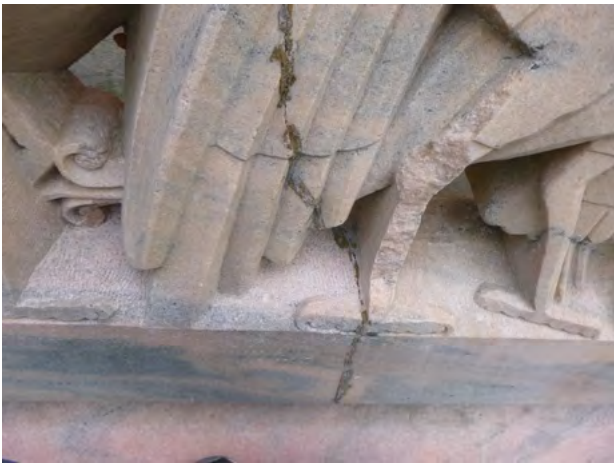
49-30 Stone_Crack Repair failed 2024-3.jpg
