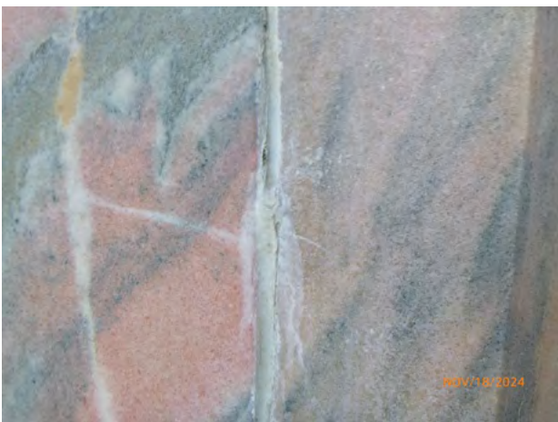
36-165 Stone_SoilStain Leached Salts 2024-2.jpg
