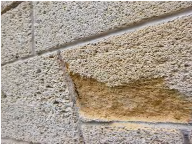
137-17 Stone_Spall Removed 2024-2.jpg
