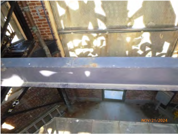
663-148 ArchMetal_Coating Coating Failed 2024-1.jpg
