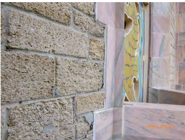
346-104 Stone_Crack System units and joints 2024-3.jpg
