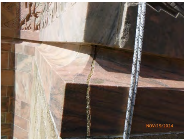
334-28 Stone_Crack Repair failed 2024-1.jpg
