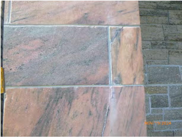
344-88 Stone_Crack System units and joints 2024-1.jpg
