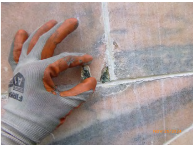
137-182 Stone_Spall Removed 2024-2.jpg
