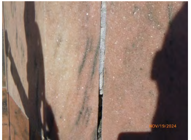
343-185 Stone_Joints Mortar Failed 2024-5.jpg
