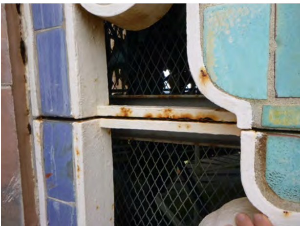
85-154 ArchMetal_Corrosion Surface 2024-2.jpg
