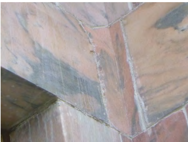
94-138 Stone_SurfLoss Chipped 2024-1.jpg
