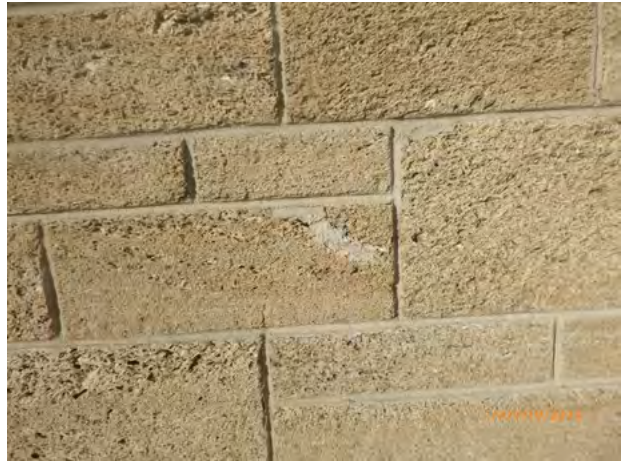
354-71 Stone_Repair Patch Failed 2024-1.jpg
