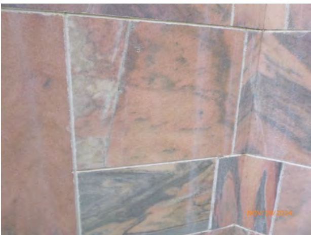
130-20 Stone_Crack Single unit 2024-1.jpg
