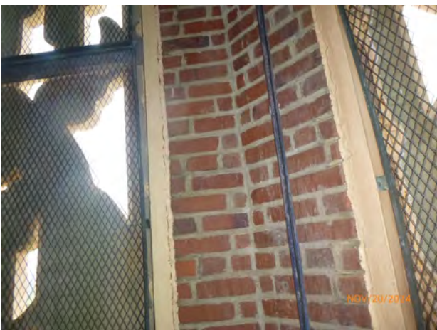
553-156 Brick_Joints Mortar Failed 2024-1.jpg
