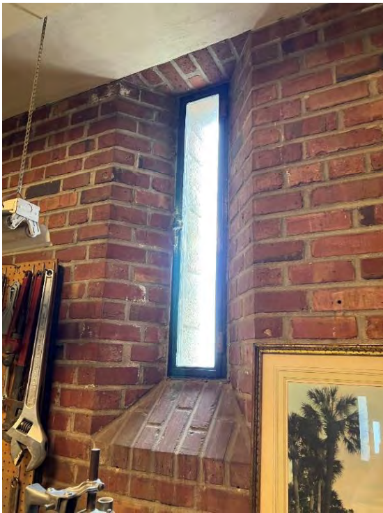
27 Slot window with reported leaks
