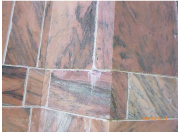
345-168 Stone_SoilStain Leached Salts 2024-1.jpg
