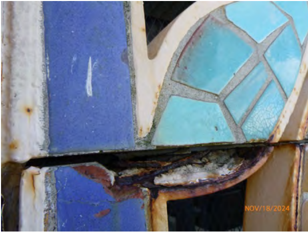
9-164 TerraCotta_Spall Missing + Steel 2024-1.jpg
