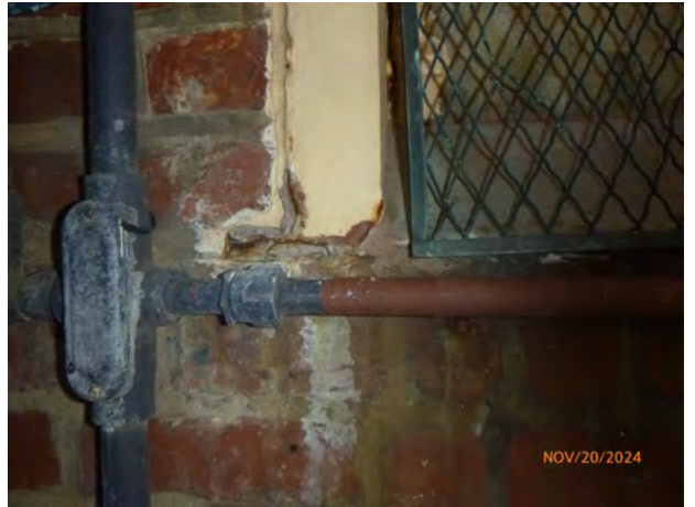
861-143 ArchMetal_Corrosion Pitted 2024-2.jpg
