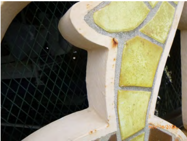
392-174 ArchMetal_Coating Coating Failed 2024-3.jpg
