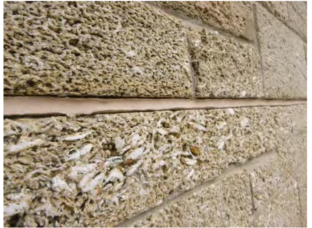
163-115 Stone_Joints Sealant Failed 2024-1.jpg
