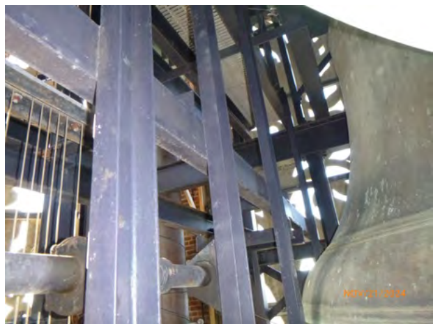
664-151 ArchMetal_Coating Coating Failed 2024-3.jpg
