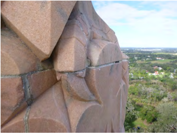
42-192 Stone_Joints Mortar Failed 2024-2.jpg
