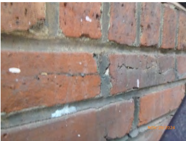
547-143 Brick_Crack System units and joints 2024-1.jpg
