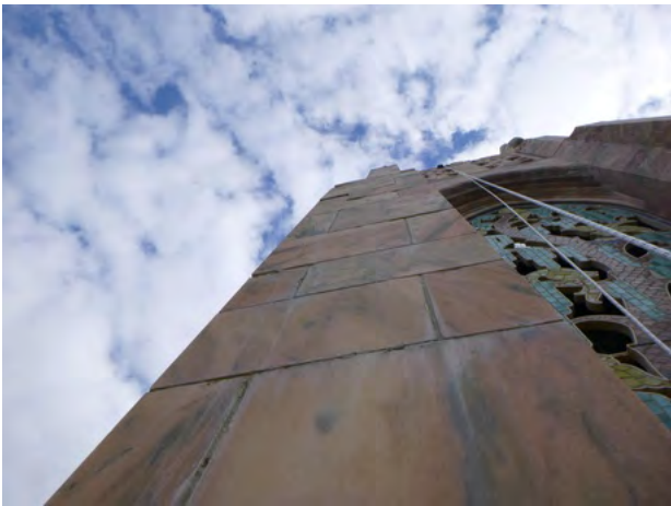
43-154 Stone_Joints Mortar Failed 2024-1.jpg
