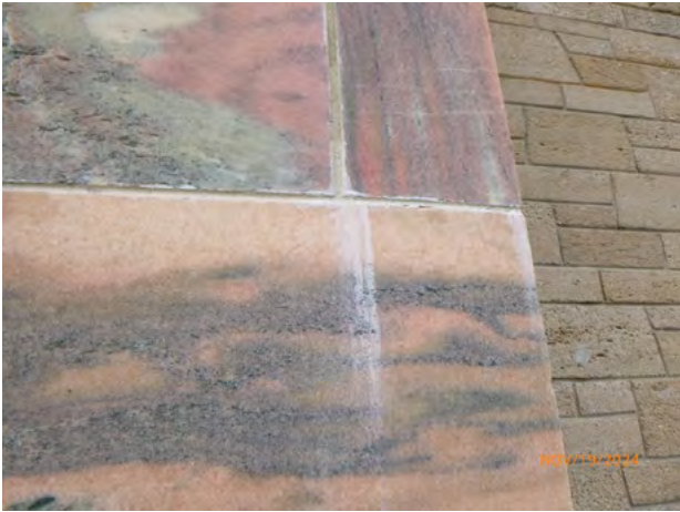
244-72 Stone_SoilStain Leached Salts 2024-1.jpg
