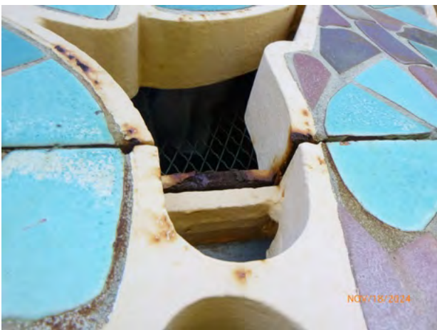
12-168 ArchMetal_Corrosion Pitted 2024-3.jpg
