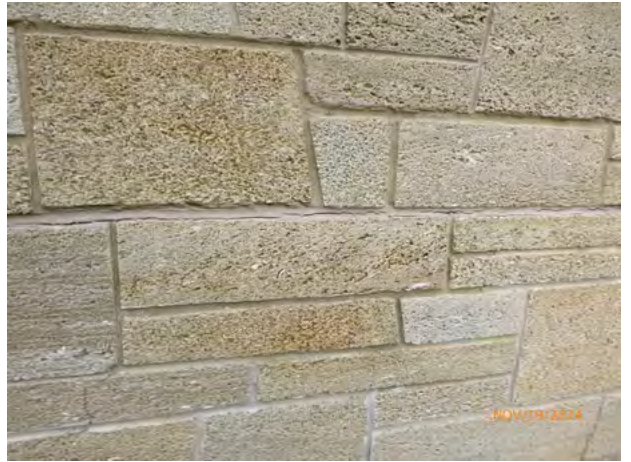
241-37 Stone_Joints Sealant Failed 2024-4.jpg
