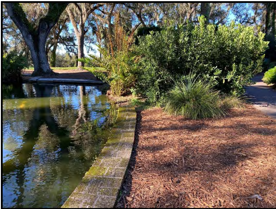
Figure 44 Alternate material coping stone and unfinished edge of moat
