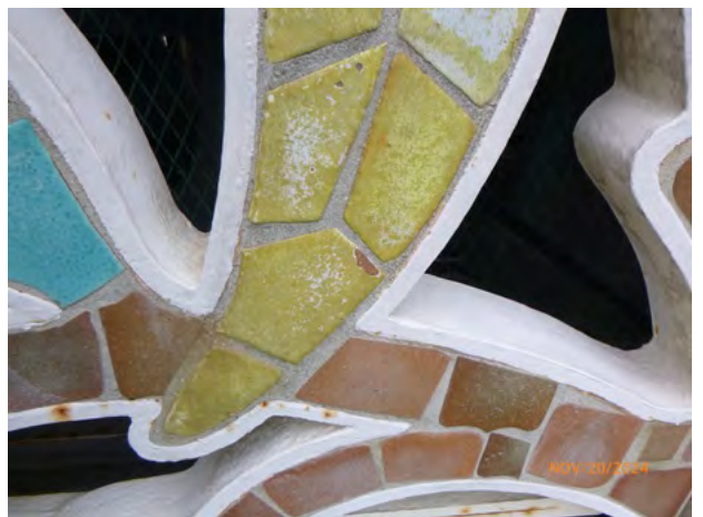
114-159 TerraCotta_SurfLoss Glaze loss 2024-1.jpg
