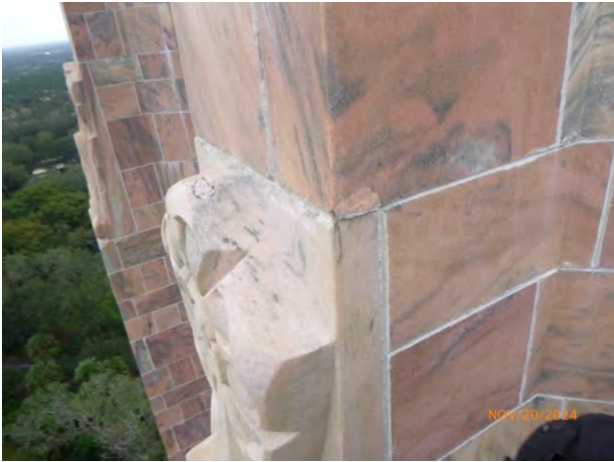
131-162 Stone_SurfLoss Chipped 2024-1.jpg
