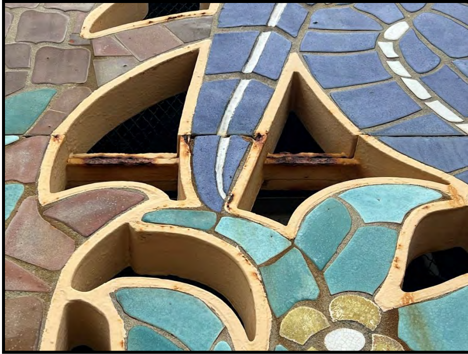
Figure 37 Terra cotta screens with cast iron frames. Corrosion is visible at the joint between cast iron frames pieces
