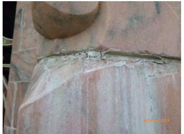
58-157 Stone_Joints Mortar Failed 2024-2.jpg
