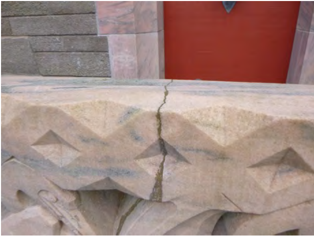
49-30 Stone_Crack Repair failed 2024-1.jpg
