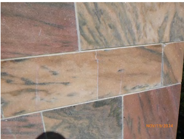
271-75 Stone_Crack Single unit 2024-1.jpg
