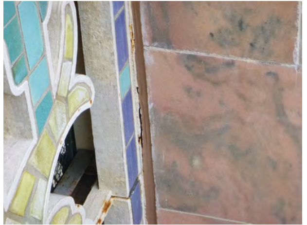
92-166 ArchMetal_Corrosion Pitted 2024-1.jpg
