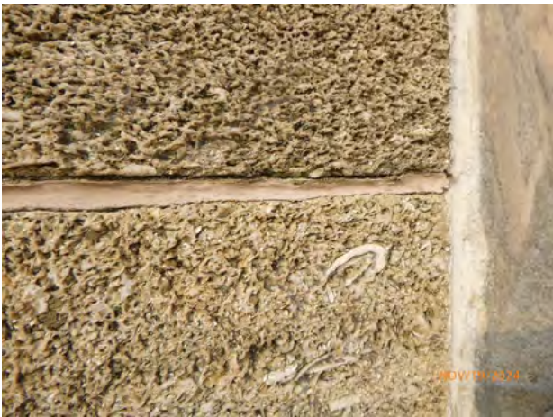
240-122 Stone_Joints Sealant Failed 2024-2.jpg
