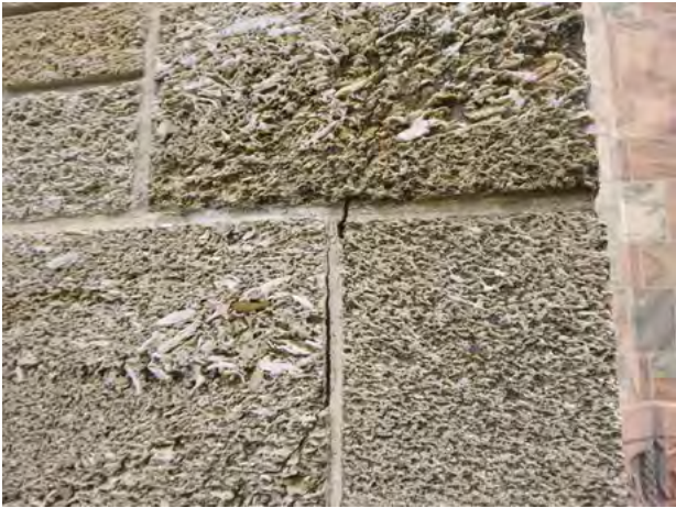
166-33 Stone_Crack System units and joints 2024-2.jpg
