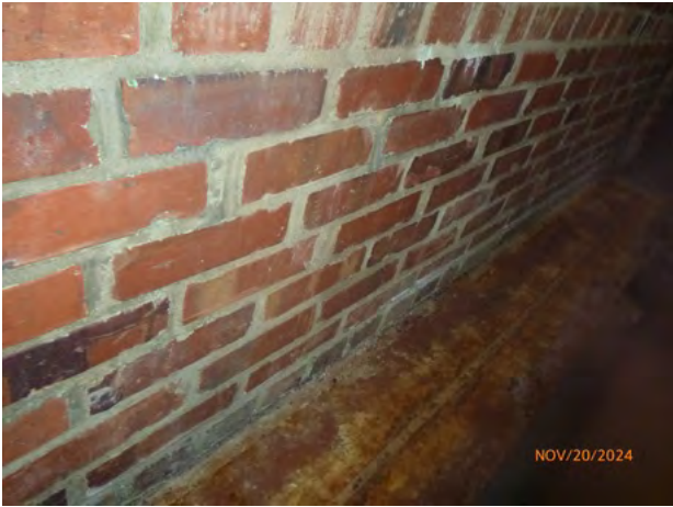
746-139 Brick_Spall Missing 2024-1.jpg
