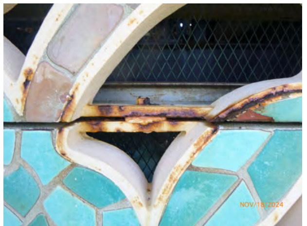
14-158 ArchMetal_Corrosion Pitted 2024-3.jpg
