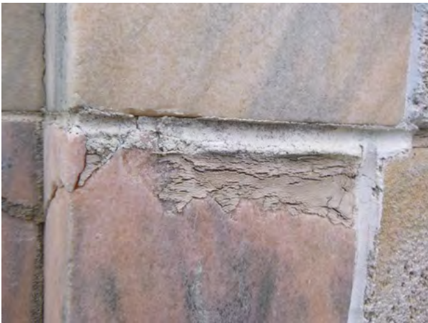
135-107 Stone_Repair Patch Failed 2024-1.jpg
