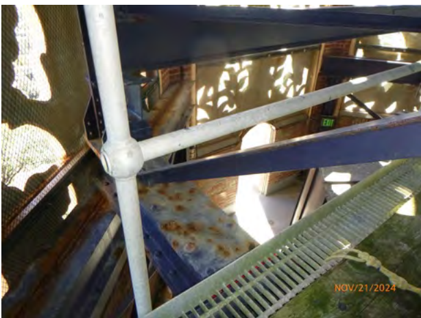
560-148 ArchMetal_Corrosion Surface 2024-3.jpg
