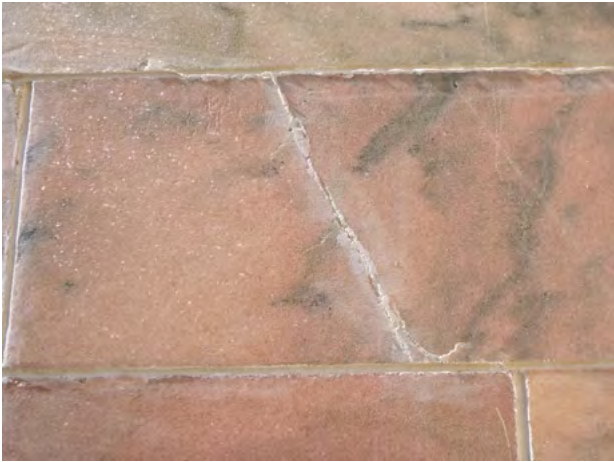
330-23 Stone_Crack Single unit 2024-1.jpg
