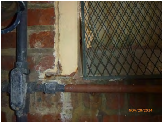
861-143 ArchMetal_Corrosion Pitted 2024-3.jpg
