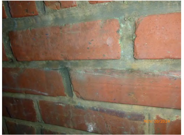
854-143 Brick_Crack System units and joints 2024-3.jpg
