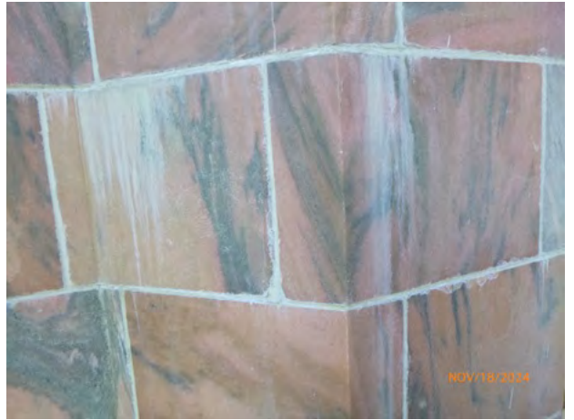
32-157 Stone_SurfLoss Chipped 2024-1.jpg
