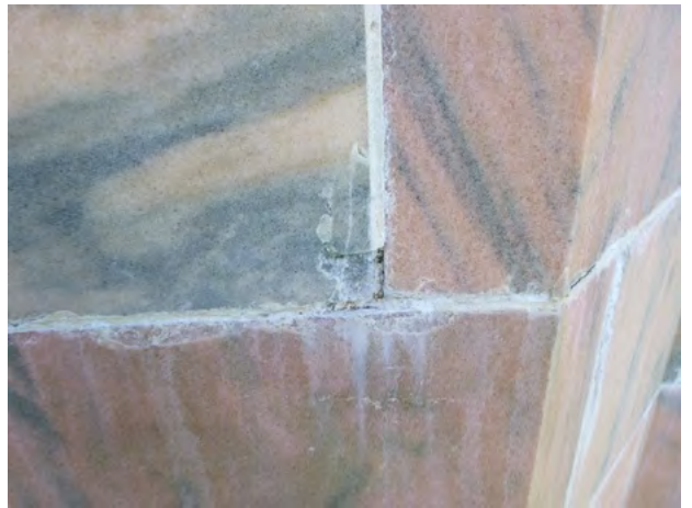
41-160 Stone_SurfLoss Chipped 2024-1.jpg
