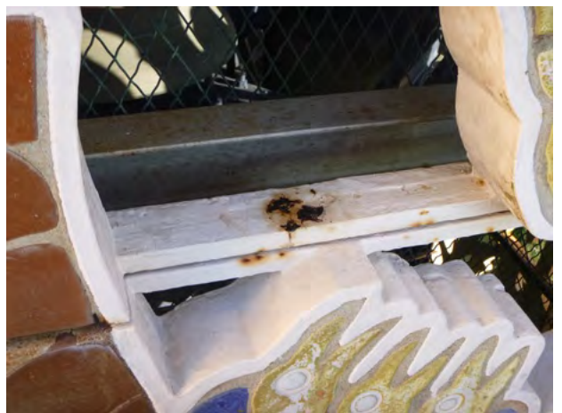
288-169 ArchMetal_Coating Coating Failed 2024-1.jpg
