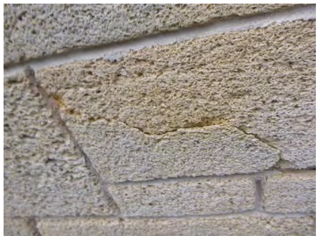
137-17 Stone_Spall Removed 2024-1.jpg
