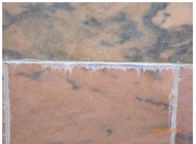
350-182 Stone_SoilStain Leached Salts 2024-2.jpg
