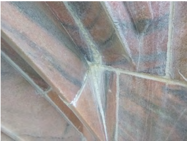
140-178 Stone_SoilStain Leached Salts 2024-3.jpg
