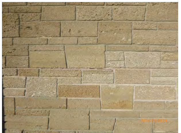
355-68 Stone_Joints Sealant Failed 2024-1.jpg
