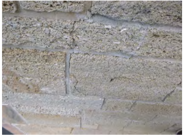
138-118 Stone_Crack System units and joints 2024-3.jpg
