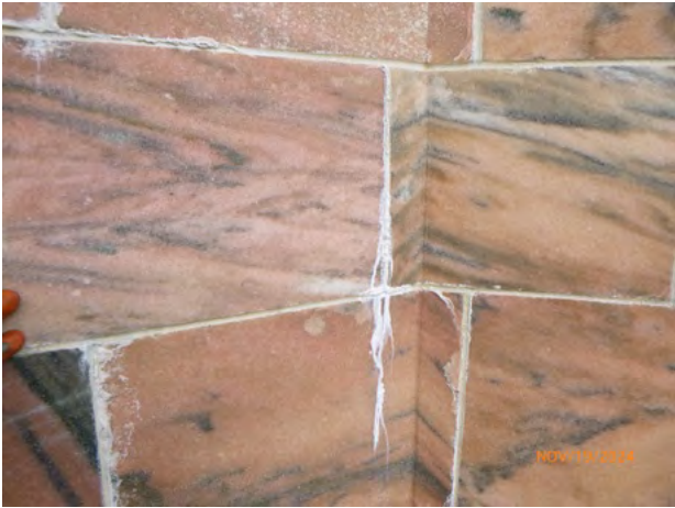
242-164 Stone_SoilStain Leached Salts 2024-4.jpg
