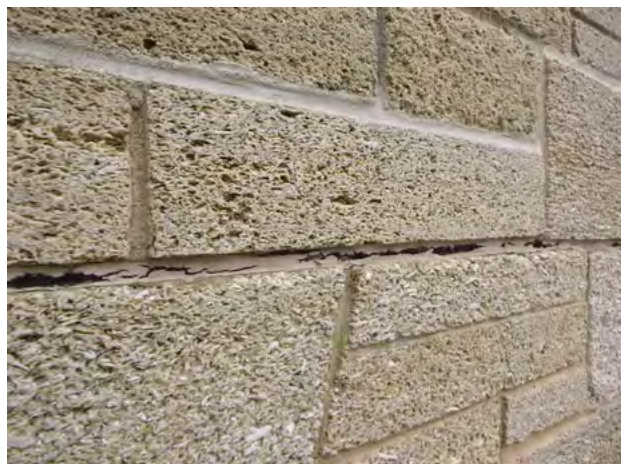
164-40 Stone_Joints Sealant Failed 2024-2.jpg
