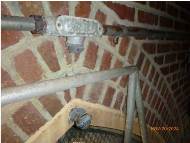
547-178 Brick_Joints Mortar Failed 2024-2.jpg
