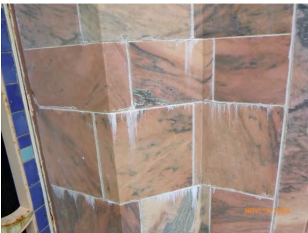
397-156 Stone_SoilStain Leached Salts 2024-3.jpg
