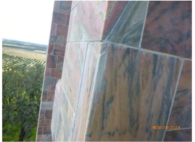
28-102 Stone_SoilStain Leached Salts 2024-1.jpg
