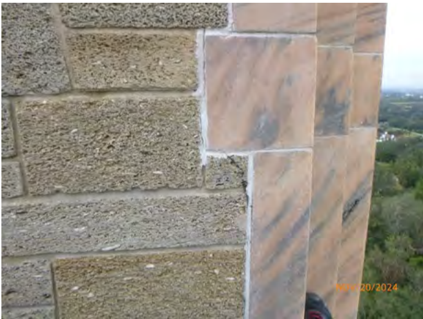
66-132 Stone_Crack System units and joints 2024-4.jpg
