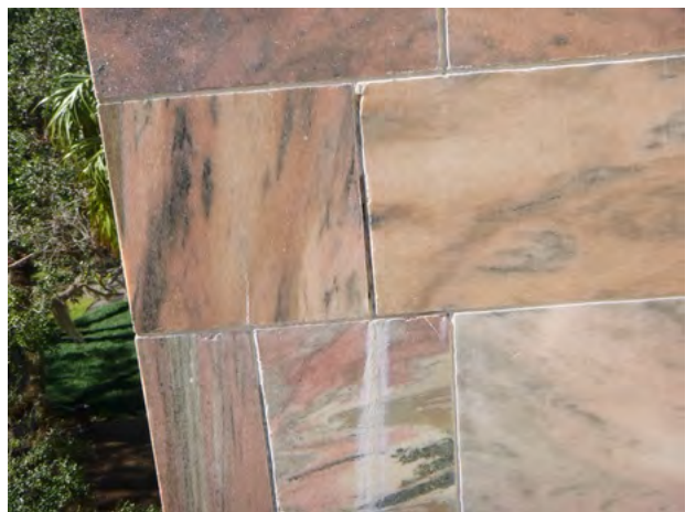
329-41 Stone_Joints Mortar Failed 2024-1.jpg
