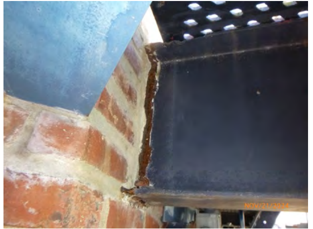
743-190 ArchMetal_Corrosion Surface 2024-2.jpg
