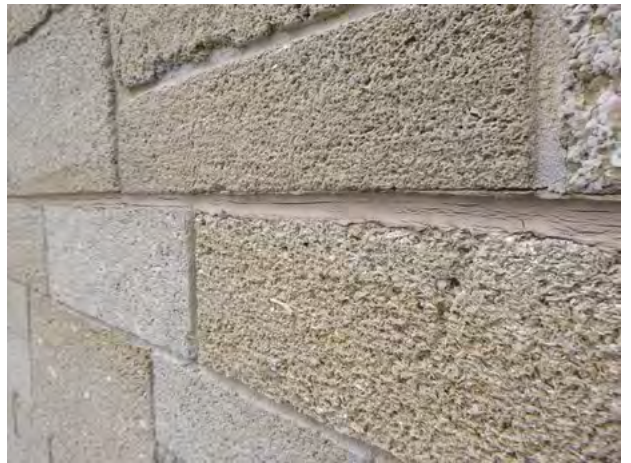
138-106 Stone_Joints Sealant Failed 2024-1.jpg
