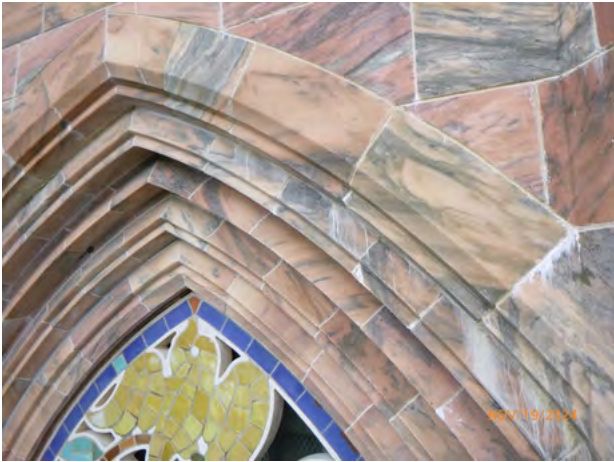
241-178 Stone_SoilStain Leached Salts 2024-1.jpg
