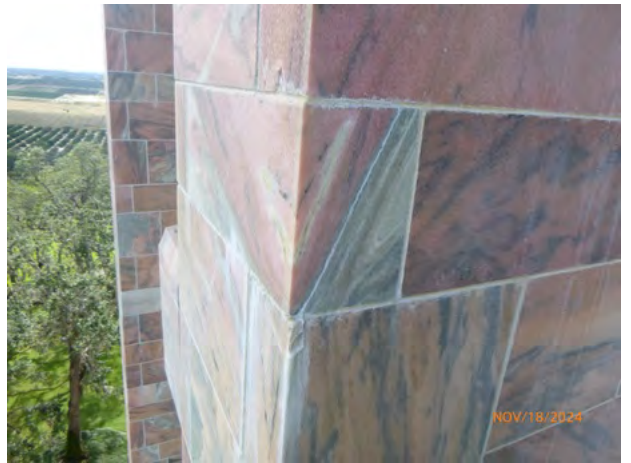
28-103 Stone_Crack Single unit 2024-2.jpg
