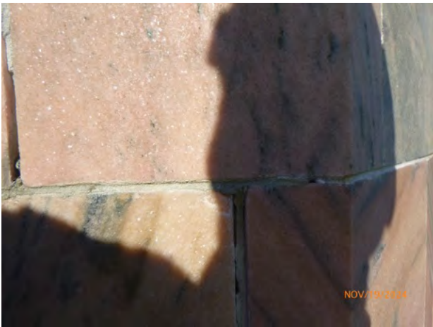
343-185 Stone_Joints Mortar Failed 2024-4.jpg
