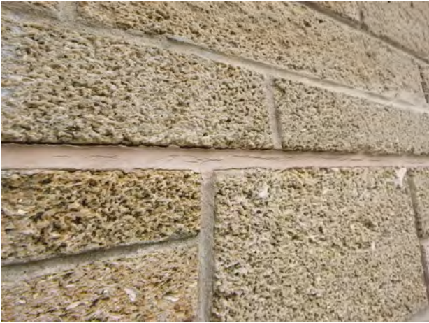
163-109 Stone_Joints Sealant Failed 2024-1.jpg
