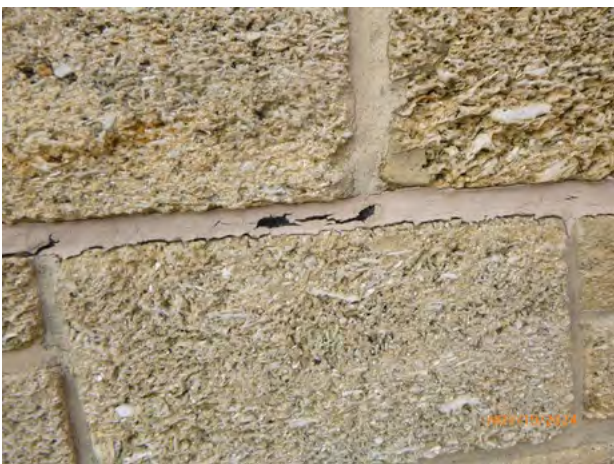
240-112 Stone_Joints Sealant Failed 2024-2.jpg
