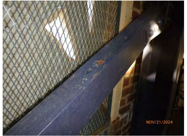
656-144 ArchMetal_Coating Coating Failed 2024-2.jpg
