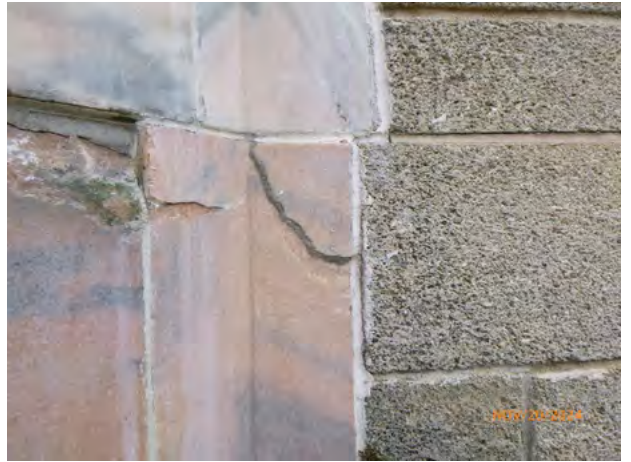
60-70 Stone_Crack Single unit 2024-1.jpg
