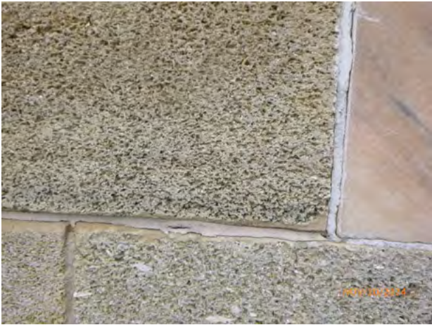
61-127 Stone_Joints Sealant Failed 2024-3.jpg
