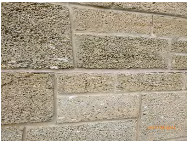
240-69 Stone_Joints Sealant Failed 2024-3.jpg
