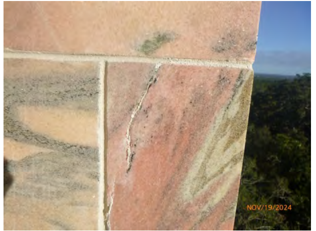
355-78 Stone_Crack Single unit 2024-3.jpg
