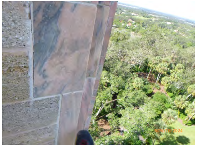
365-107 Stone_Crack System units and joints 2024-4.jpg
