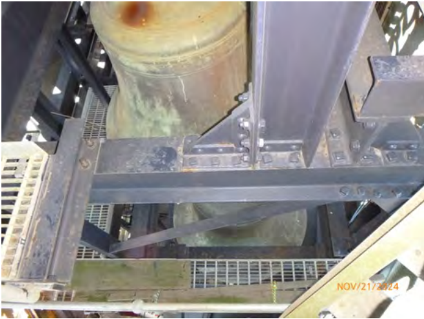
562-170 ArchMetal_Coating Coating Failed 2024-1.jpg
