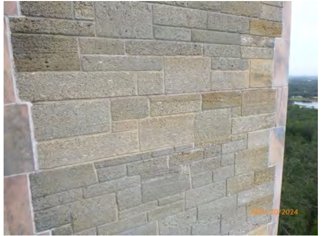
61-109 Stone_Joints Sealant Failed 2024-1.jpg
