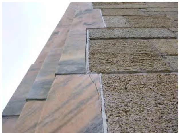
135-123 Stone_Crack System units and joints 2024-1.jpg
