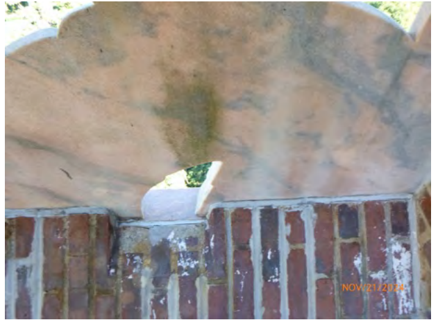
844-184 Brick_Joints Sealant Failed 2024-2.jpg
