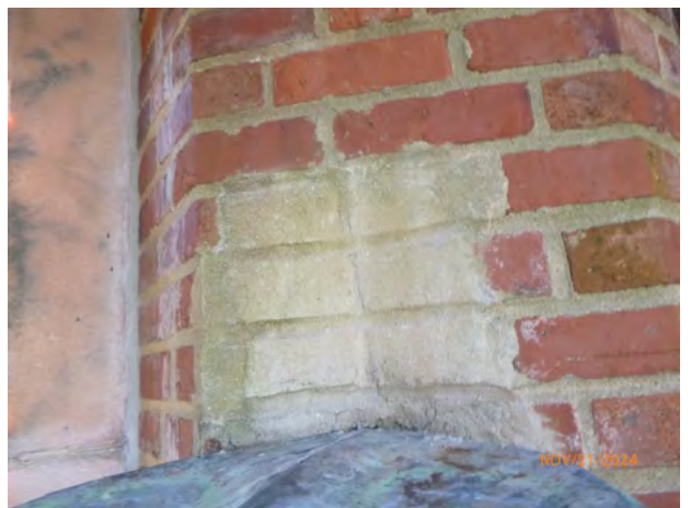
756-190 Brick_Repair Patch Failed 2024-4.jpg
