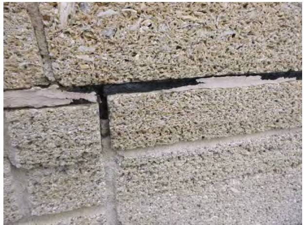
150-90 Stone_Joints Sealant Failed 2024-4.jpg
