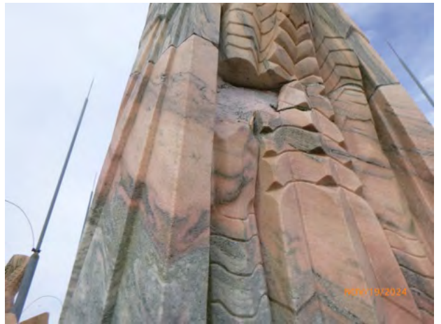
244-201 Stone_Spall Missing 2024-1.jpg
