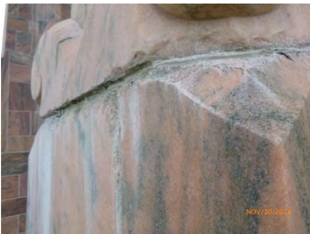
58-157 Stone_Joints Mortar Failed 2024-3.jpg
