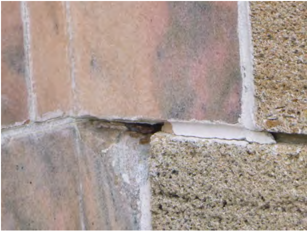
145-91 Stone_Spall Missing + Steel 2024-1.jpg
