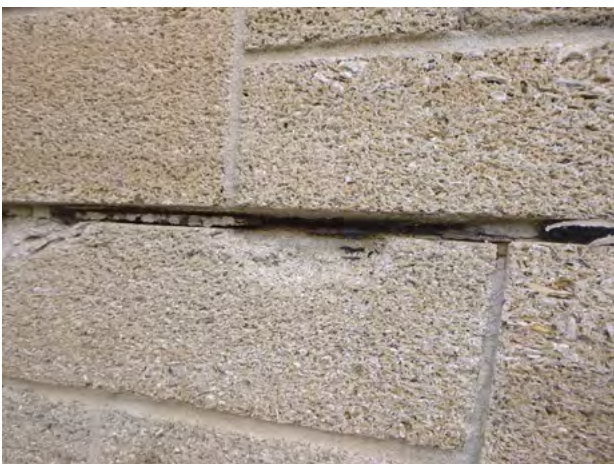
147-91 Stone_Spall Missing + Steel 2024-1.jpg
