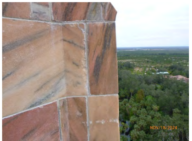
355-181 Stone_SurfLoss Chipped 2024-3.jpg
