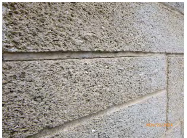
62-46 Stone_Joints Sealant Failed 2024-2.jpg
