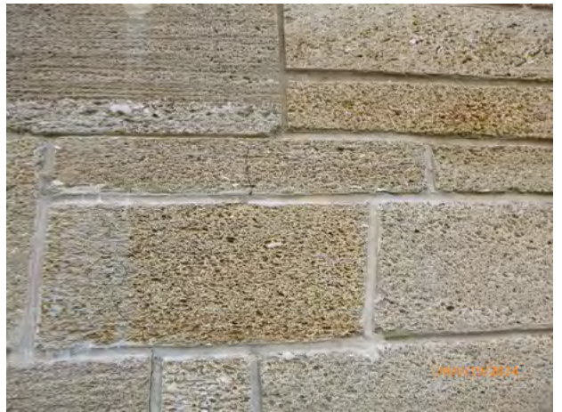
235-33 Stone_Crack System units and joints 2024-4.jpg
