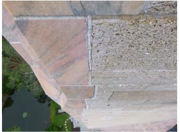
135-123 Stone_Crack System units and joints 2024-3.jpg
