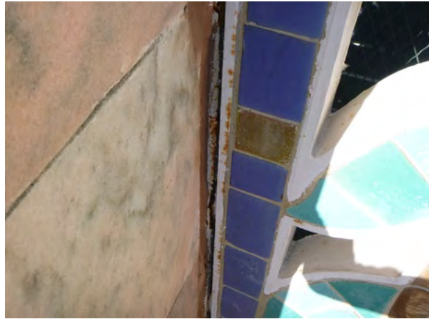
336-160 ArchMetal_Corrosion Pitted 2024-1.jpg
