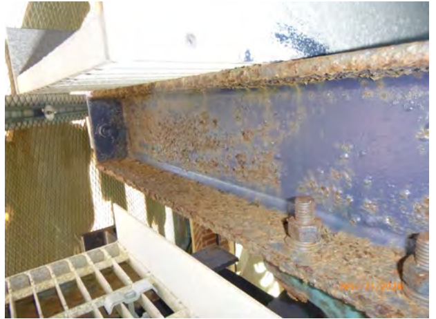
562-172 ArchMetal_Corrosion Surface 2024-2.jpg
