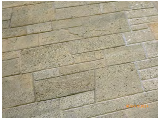
364-13 Stone_Crack System units and joints 2024-1.jpg
