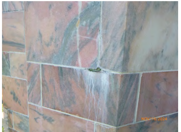
36-165 Stone_SoilStain Leached Salts 2024-1.jpg
