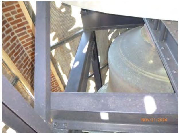
764-157 ArchMetal_Coating Coating Failed 2024-2.jpg
