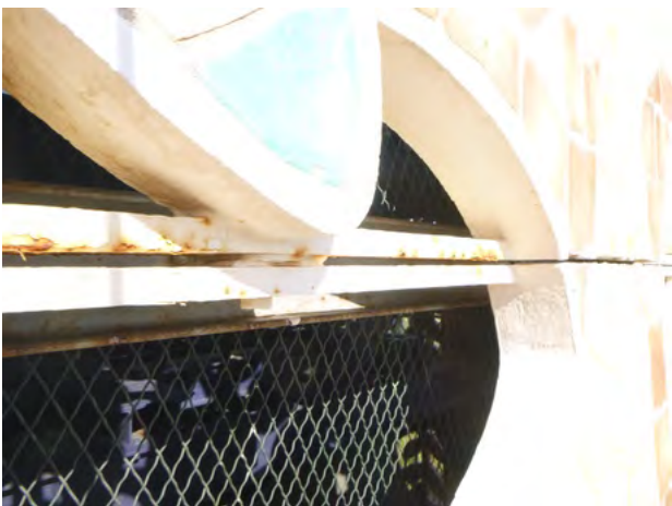
313-158 ArchMetal_Corrosion Surface 2024-1.jpg
