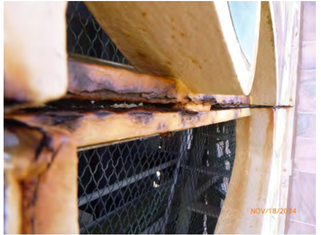
12-163 ArchMetal_Corrosion Pitted 2024-3.jpg
