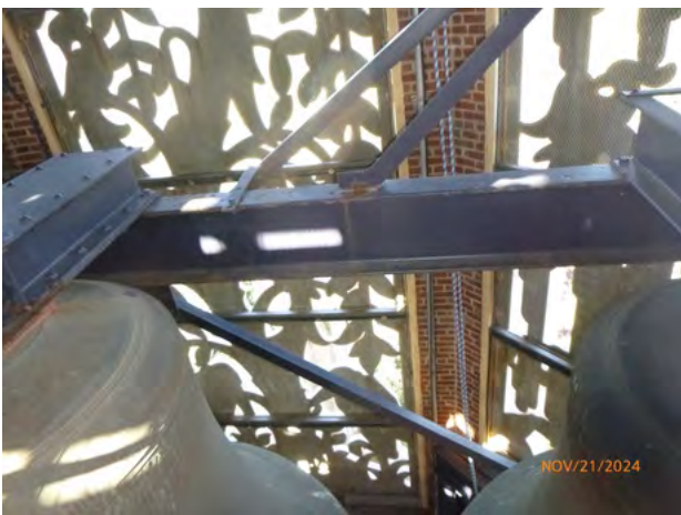
540-158 ArchMetal_Coating Coating Failed 2024-1.jpg
