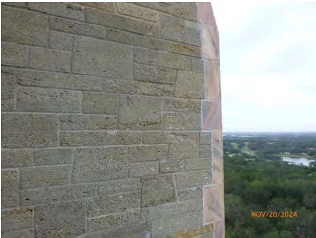
65-116 Stone_Crack System units and joints 2024-1.jpg
