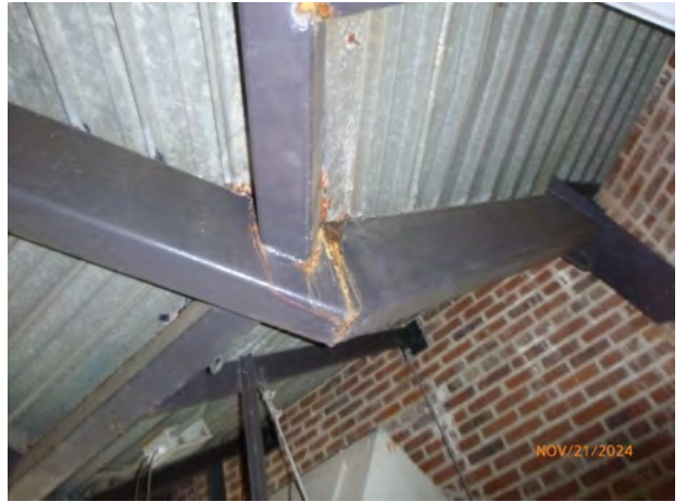
763-180 ArchMetal_Corrosion Surface 2024-2.jpg
