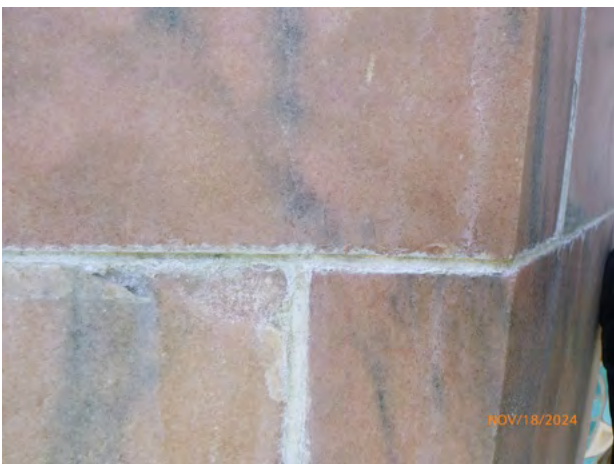
32-169 Stone_SurfLoss Chipped 2024-2.jpg
