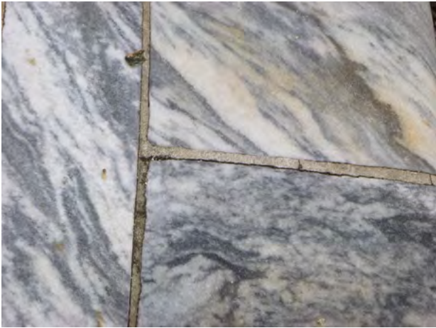
149-0 Stone_Joints Mortar Failed 2024-2.jpg
