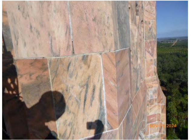
343-185 Stone_Joints Mortar Failed 2024-3.jpg
