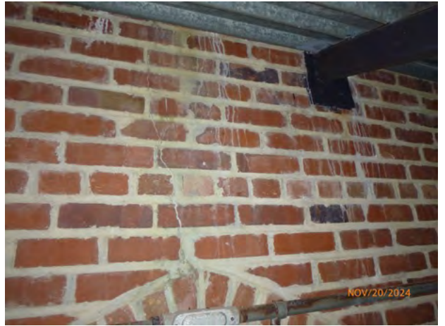
548-180 Brick_SoilStain Leached Salts 2024-1.jpg
