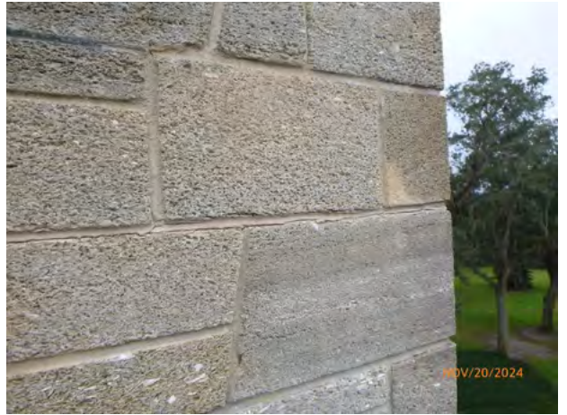
62-46 Stone_Joints Sealant Failed 2024-4.jpg
