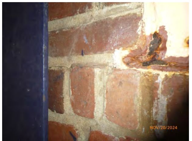
541-144 Brick_Crack Repair failed 2024-1.jpg
