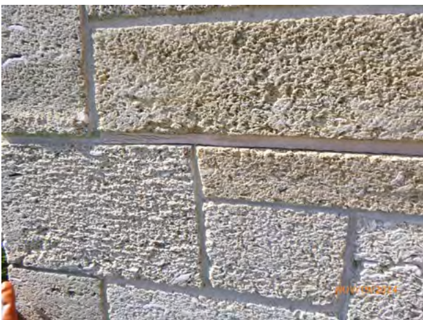
340-68 Stone_Joints Sealant Failed 2024-4.jpg
