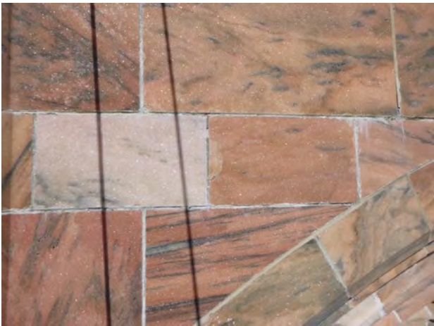
337-181 Stone_Joints Mortar Failed 2024-1.jpg
