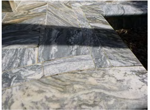
225-1 Stone_Joints Mortar Failed 2024-1.jpg
