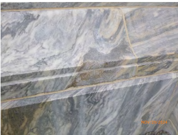
128-4 Stone_Spall Missing 2024-1.jpg
