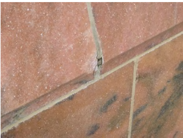
338-184 Stone_Joints Mortar Failed 2024-2.jpg
