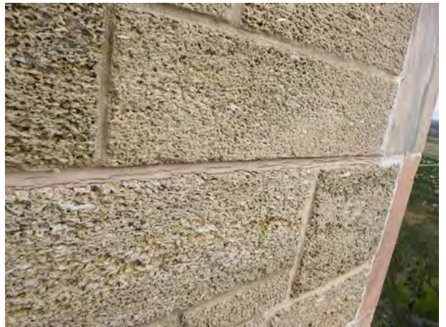
163-130 Stone_Joints Sealant Failed 2024-2.jpg
