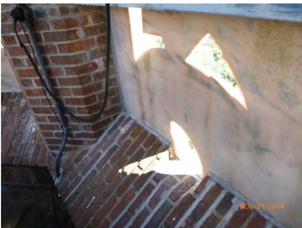
741-184 Brick_Joints Sealant Failed 2024-3.jpg
