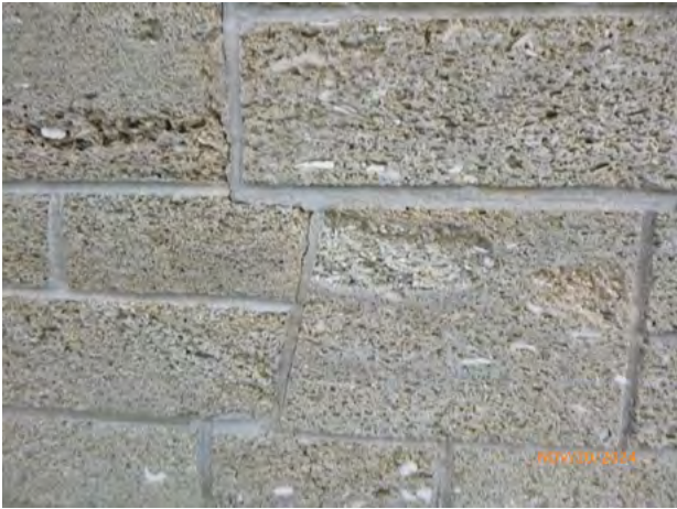
65-116 Stone_Crack System units and joints 2024-5.jpg
