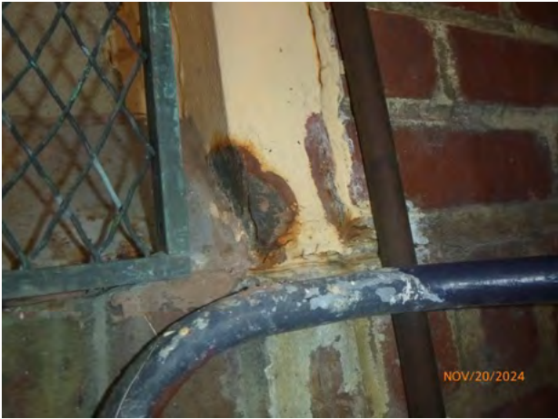
742-144 ArchMetal_Corrosion Pitted 2024-1.jpg
