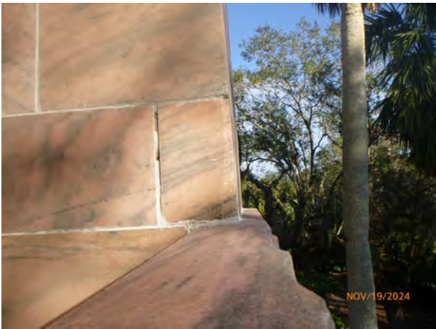
356-32 Stone_Spall Missing 2024-2.jpg
