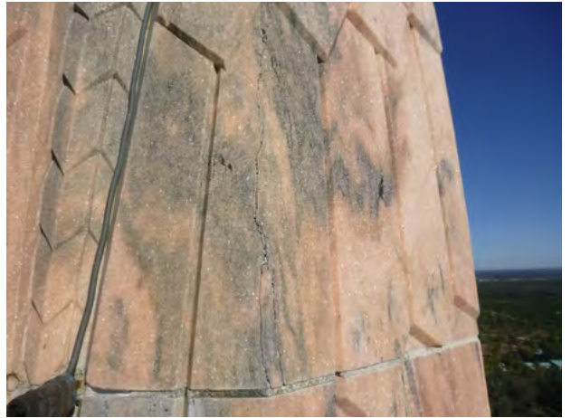
538-201 Stone_Crack Repair failed 2024-3.jpg
