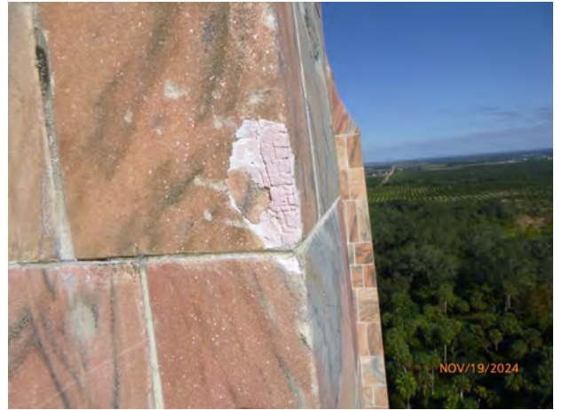
342-183 Stone_Repair Patch Failed 2024-1.jpg
