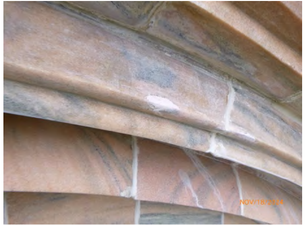
351-181 Stone_Repair Patch Failed 2024-1.jpg
