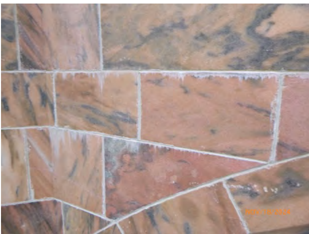
350-182 Stone_SoilStain Leached Salts 2024-1.jpg
