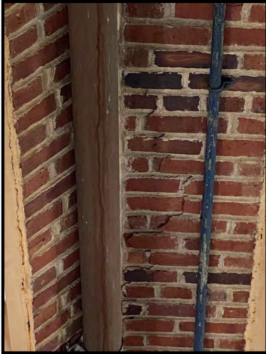
Figure 25 Spalled interior masonry within the Carillon chamber
