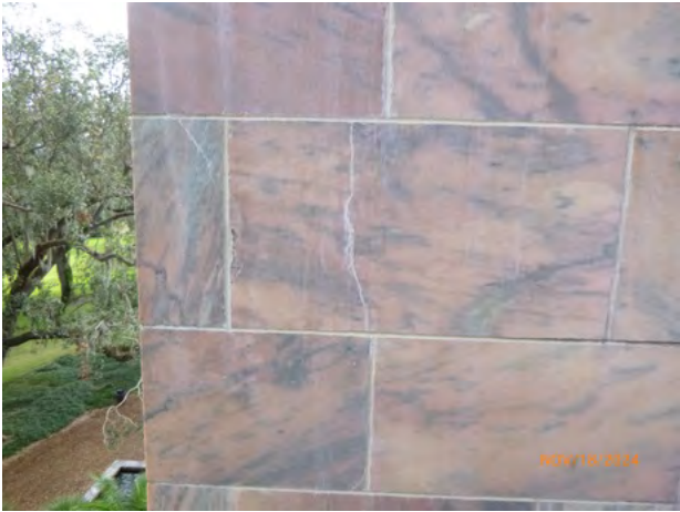
30-44 Stone_Crack Single unit 2024-1.jpg
