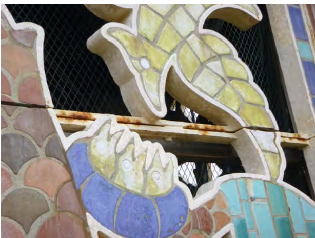
90-168 ArchMetal_Corrosion Surface 2024-1.jpg
