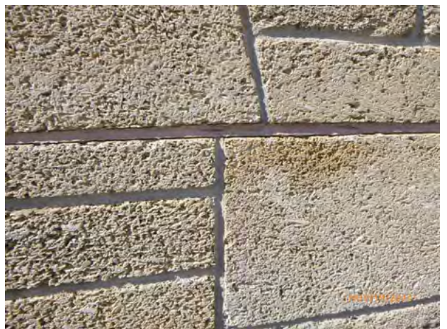
341-122 Stone_Joints Sealant Failed 2024-4.jpg
