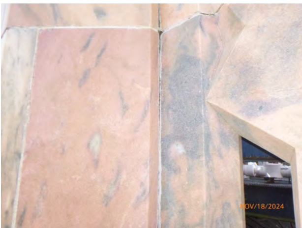
36-185 Stone_Joints Mortar Failed 2024-3.jpg
