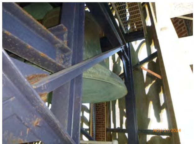
560-148 ArchMetal_Corrosion Surface 2024-4.jpg
