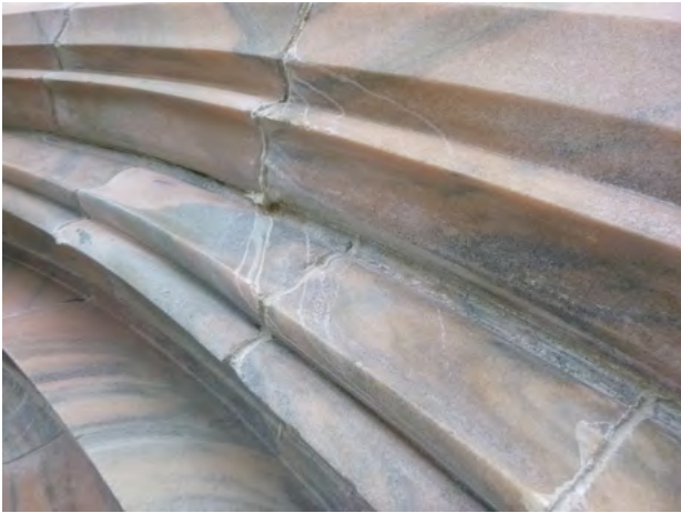
140-178 Stone_SoilStain Leached Salts 2024-1.jpg
