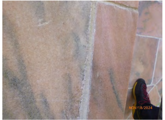
33-180 Stone_SurfLoss Chipped 2024-3.jpg
