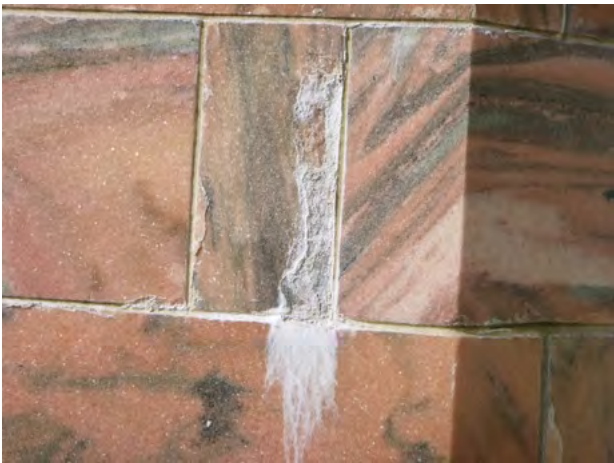
237-170 Stone_SoilStain Leached Salts 2024-1.jpg
