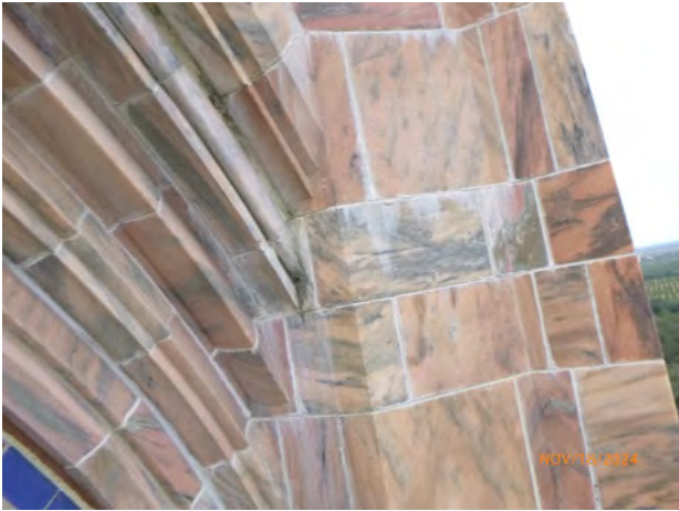
355-176 Stone_SoilStain Leached Salts 2024-1.jpg
