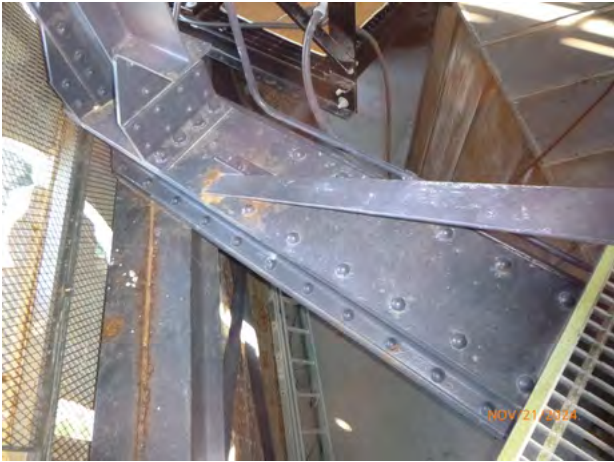
763-147 ArchMetal_Coating Coating Failed 2024-1.jpg
