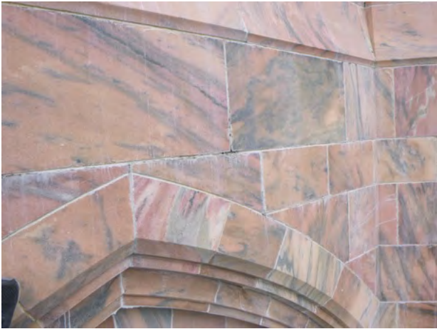
90-181 Stone_SoilStain Leached Salts 2024-1.jpg
