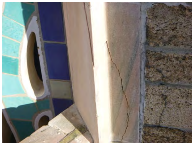
253-105 Stone_Crack Single unit 2024-2.jpg
