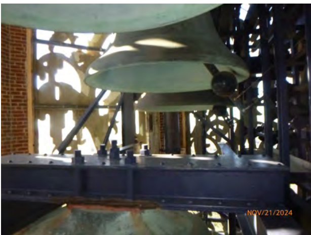
561-160 ArchMetal_Coating Coating Failed 2024-2.jpg
