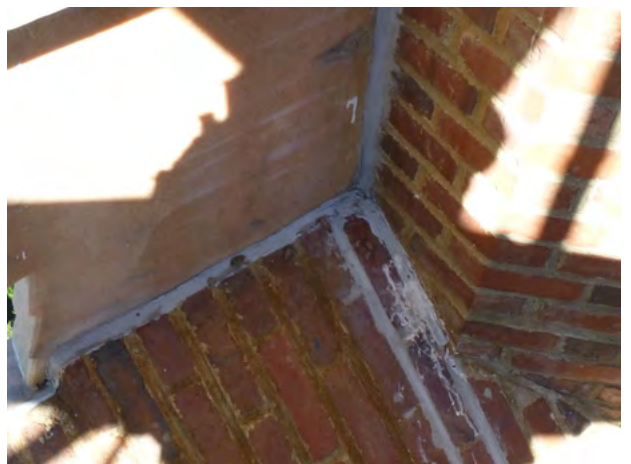
535-185 Brick_Joints Sealant Failed 2024-1.jpg
