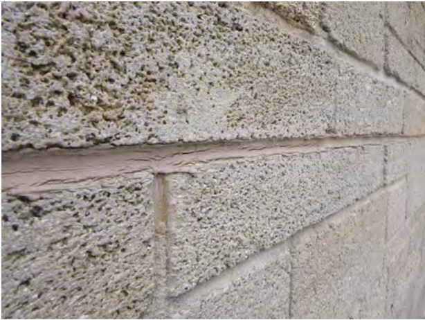
139-89 Stone_Joints Sealant Failed 2024-2.jpg
