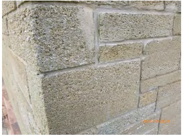
235-33 Stone_Crack System units and joints 2024-2.jpg
