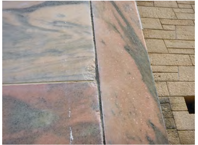
158-11 Stone_Spall Missing 2024-1.jpg
