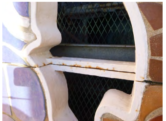
287-149 ArchMetal_Corrosion Surface 2024-1.jpg
