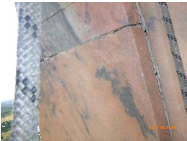
35-191 Stone_Joints Mortar Failed 2024-2.jpg
