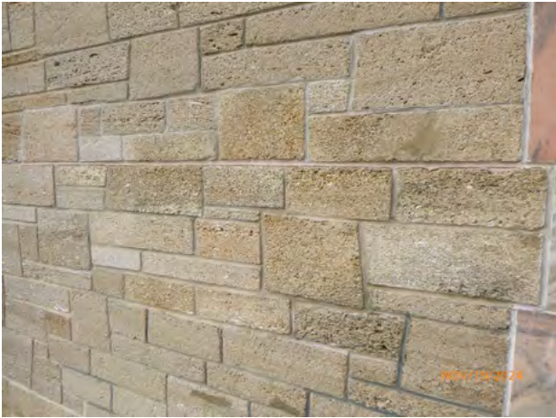
241-80 Stone_Joints Sealant Failed 2024-1.jpg
