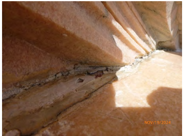
341-139 Stone_Joints Mortar Failed 2024-4.jpg
