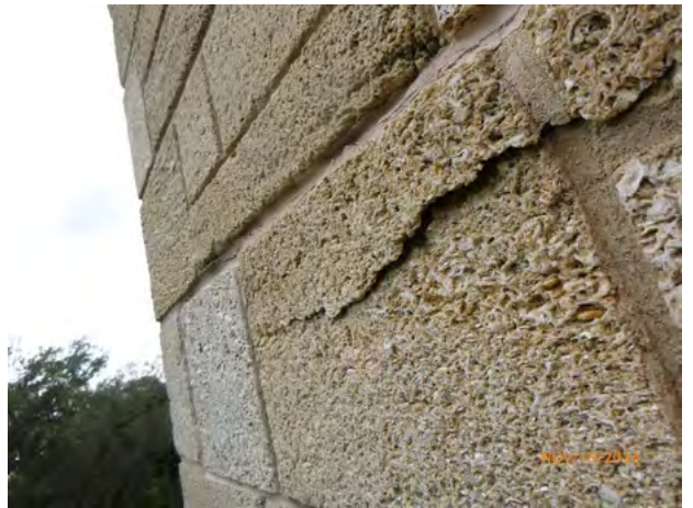
236-42 Stone_Crack Single unit 2024-2.jpg
