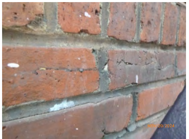
547-143 Brick_Crack System units and joints 2024-2.jpg
