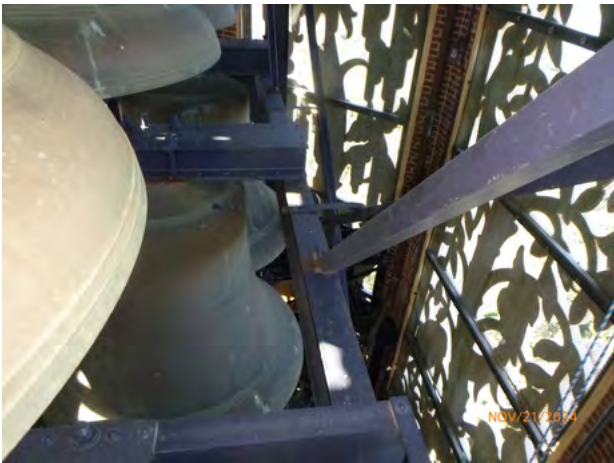
540-158 ArchMetal_Coating Coating Failed 2024-5.jpg
