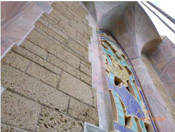
346-104 Stone_Crack System units and joints 2024-1.jpg
