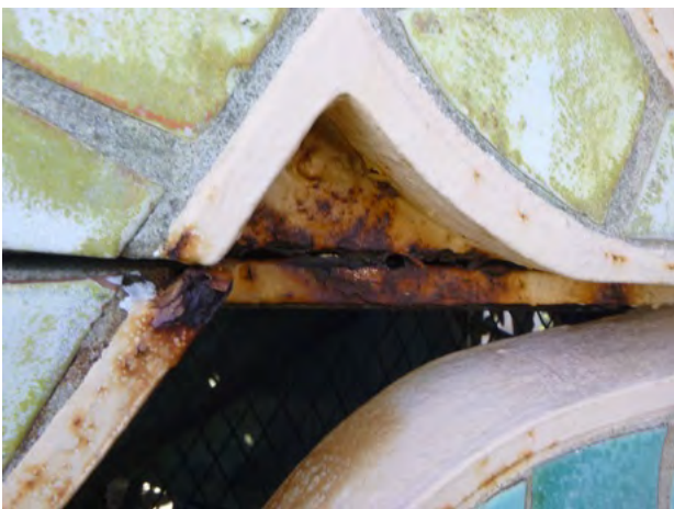
16-158 ArchMetal_Corrosion Pitted 2024-2.jpg
