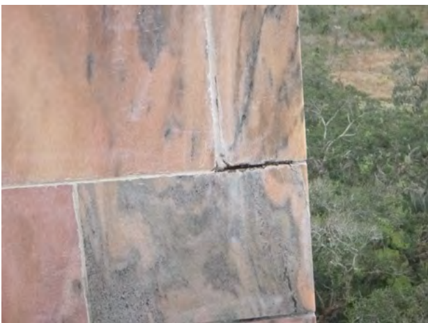
196-138 Stone_Joints Mortar Failed 2024-1.jpg
