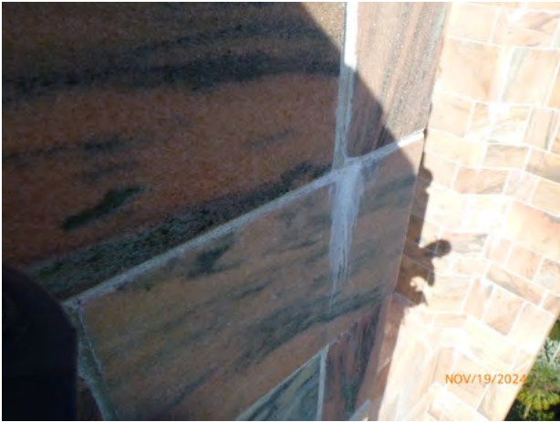
343-154 Stone_SoilStain Leached Salts 2024-1.jpg
