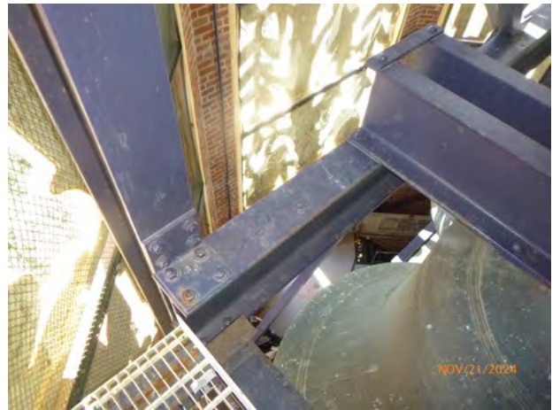
743-157 ArchMetal_Coating Coating Failed 2024-2.jpg
