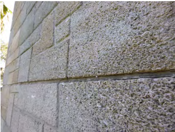
37-43 Stone_Joints Sealant Failed 2024-1.jpg
