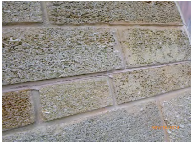
361-96 Stone_Joints Sealant Failed 2024-4.jpg
