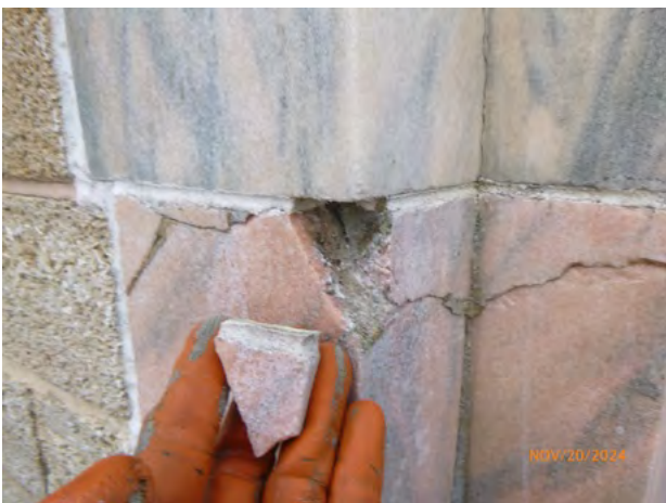
134-102 Stone_Spall Removed 2024-2.jpg
