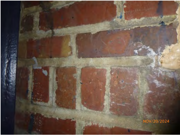
759-143 Brick_Joints Mortar Failed 2024-1.jpg
