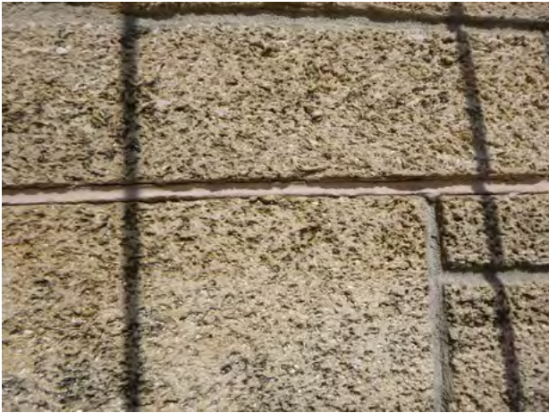
262-121 Stone_Joints Sealant Failed 2024-2.jpg
