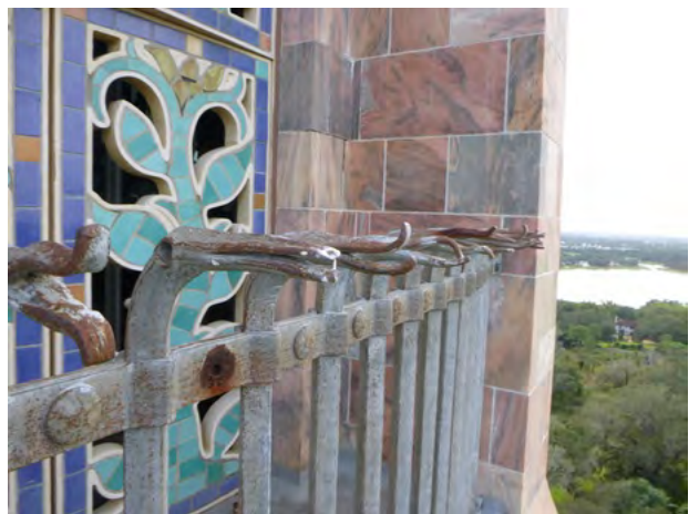
87-127 ArchMetal_Corrosion Surface 2024-2.jpg
