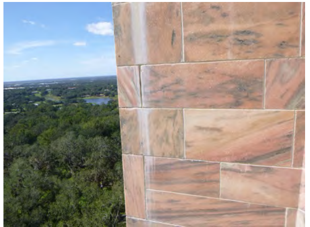
330-115 Stone_SoilStain Leached Salts 2024-2.jpg
