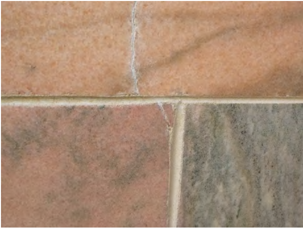
230-51 Stone_Crack System units and joints 2024-2.jpg
