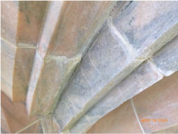
36-179 Stone_SoilStain Leached Salts 2024-1.jpg
