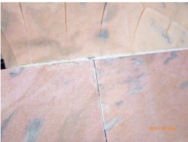
37-184 Stone_SurfLoss Chipped 2024-1.jpg
