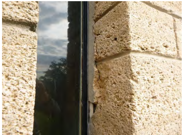
164-55 Stone_Spall Removed 2024-4.jpg
