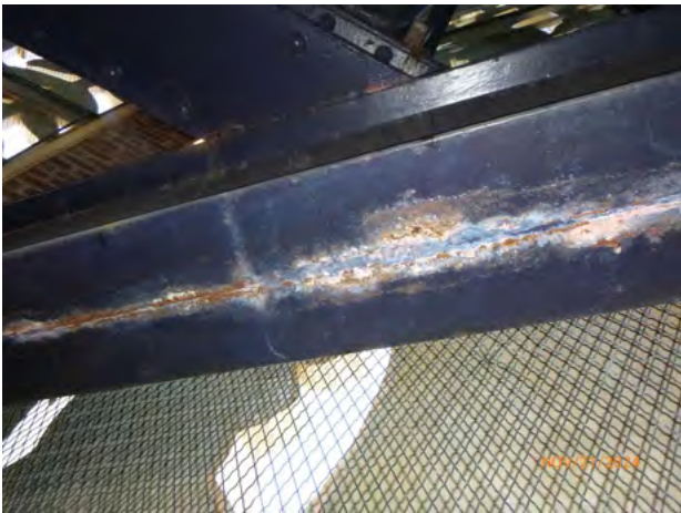
657-144 ArchMetal_Coating Coating Failed 2024-4.jpg
