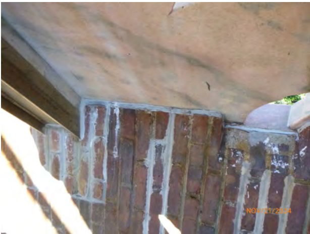
844-184 Brick_Joints Sealant Failed 2024-3.jpg
