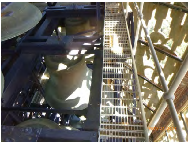
741-169 ArchMetal_Coating Coating Failed 2024-2.jpg
