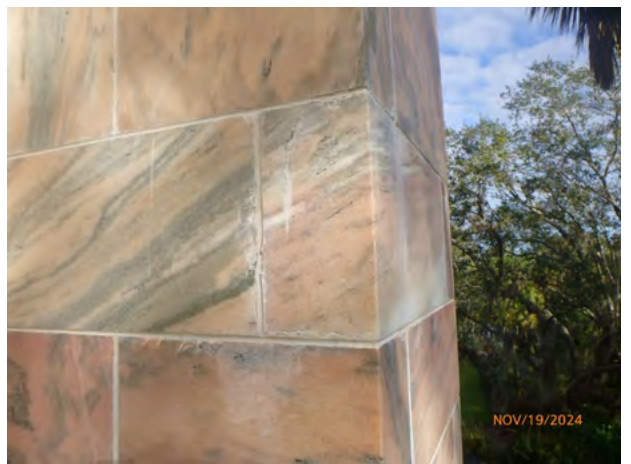
356-37 Stone_SurfLoss Chipped 2024-1.jpg
