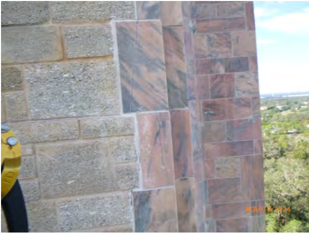
365-107 Stone_Crack System units and joints 2024-1.jpg
