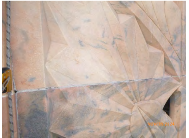
38-188 Stone_Joints Mortar Failed 2024-2.jpg
