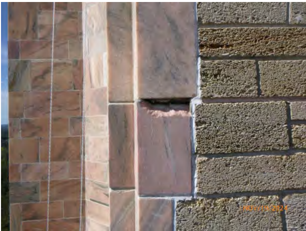
334-98 Stone_Spall Missing + Steel 2024-3.jpg
