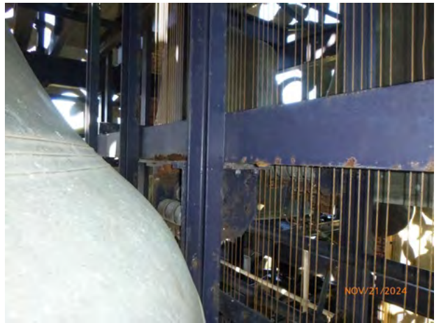
742-150 ArchMetal_Coating Coating Failed 2024-3.jpg
