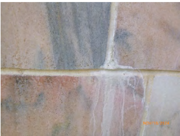
31-59 Stone_SoilStain Leached Salts 2024-2.jpg
