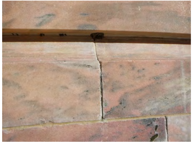
255-28 Stone_Joints Mortar Failed 2024-1.jpg
