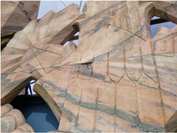
237-193 Stone_Spall Missing 2024-1.jpg
