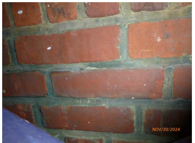
548-143 Brick_Joints Mortar Failed 2024-2.jpg
