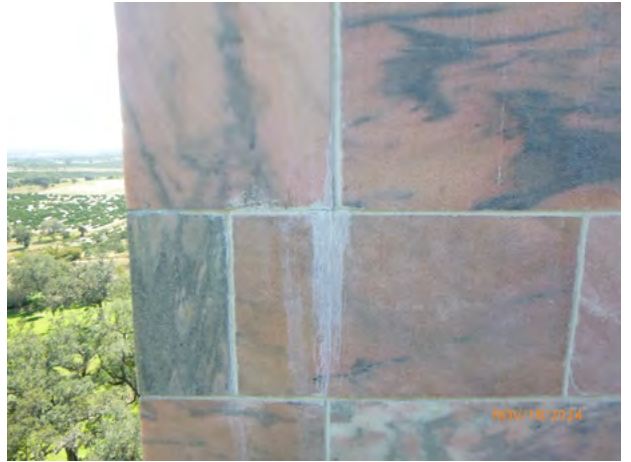
30-136 Stone_SoilStain Leached Salts 2024-1.jpg
