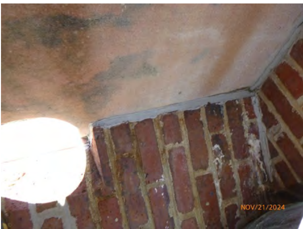
757-184 Brick_Joints Sealant Failed 2024-2.jpg
