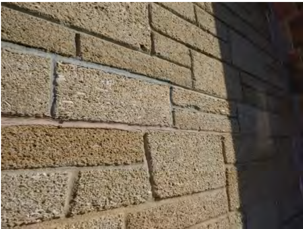
250-66 Stone_Joints Sealant Failed 2024-2.jpg
