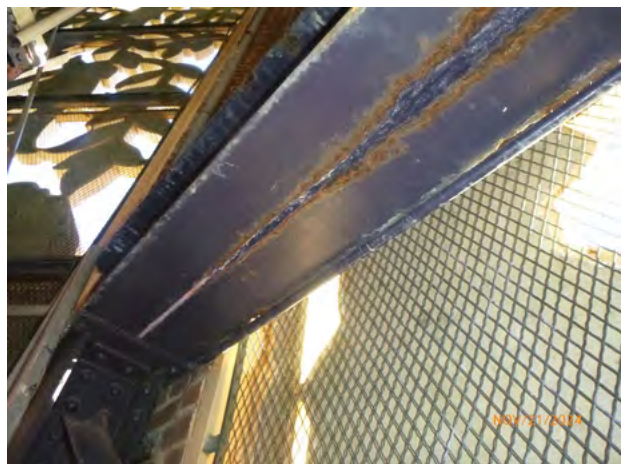
861-145 ArchMetal_Coating Coating Failed 2024-3.jpg
