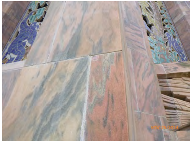
59-142 Stone_SurfLoss Chipped 2024-1.jpg
