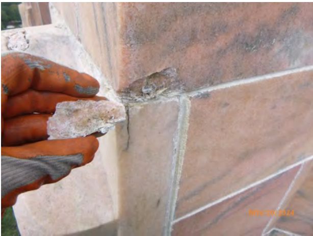
131-162 Stone_SurfLoss Chipped 2024-3.jpg
