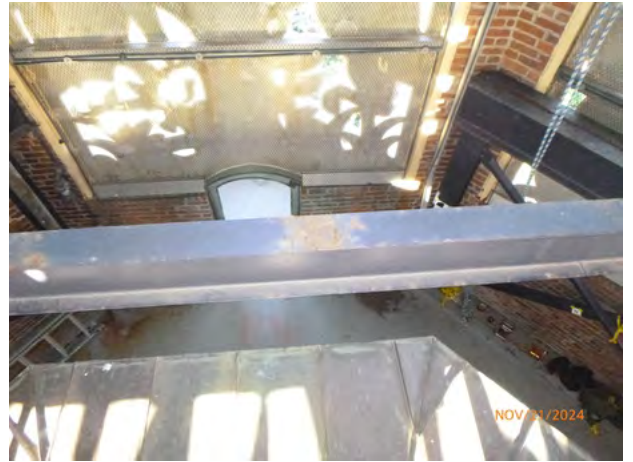
663-148 ArchMetal_Coating Coating Failed 2024-2.jpg
