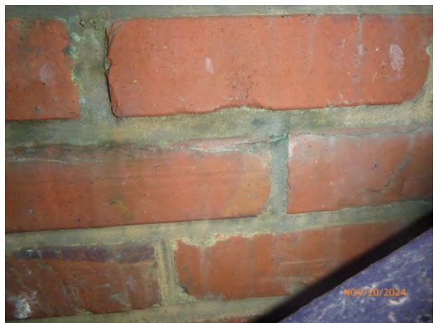
854-143 Brick_Crack System units and joints 2024-1.jpg
