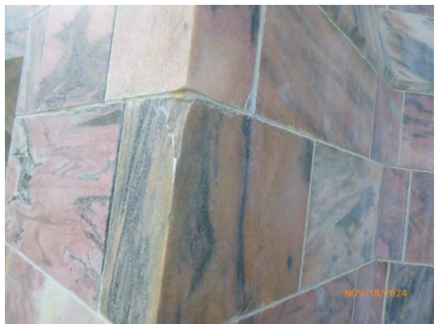
29-119 Stone_SurfLoss Chipped 2024-2.jpg
