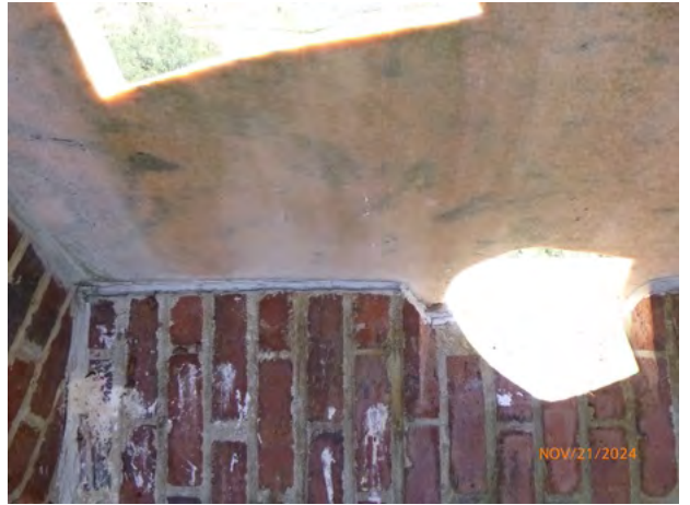
757-184 Brick_Joints Sealant Failed 2024-5.jpg
