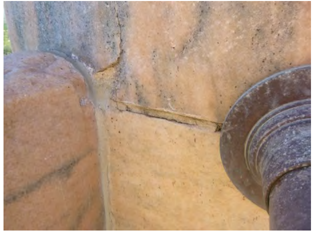
539-193 Stone_Joints Mortar Failed 2024-4.jpg
