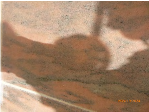
357-45 Stone_SoilStain Leached Salts 2024-6.jpg
