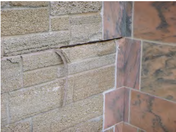
150-90 Stone_Joints Sealant Failed 2024-3.jpg
