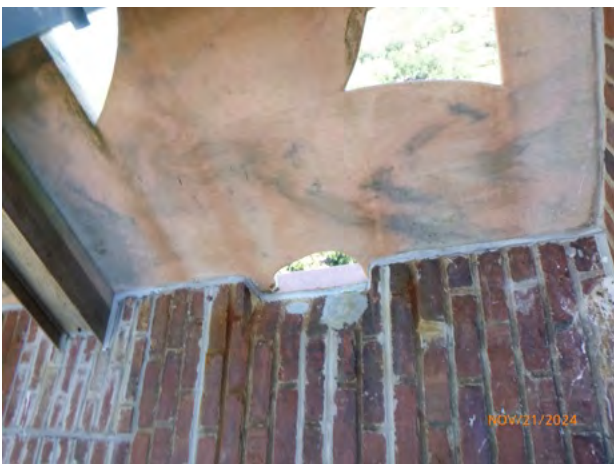
860-184 Brick_Joints Sealant Failed 2024-2.jpg
