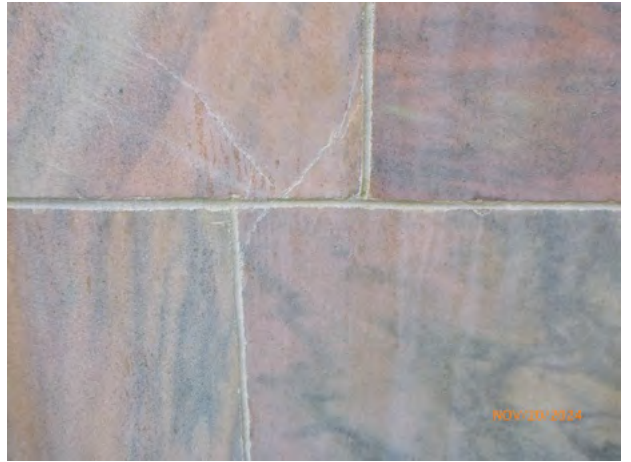
129-70 Stone_Crack System units and joints 2024-1.jpg
