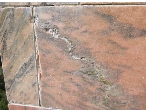
330-128 Stone_Crack Single unit 2024-1.jpg
