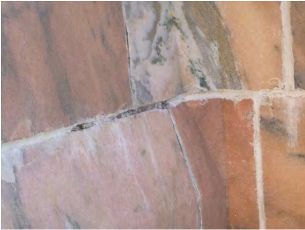
256-138 Stone_Joints Mortar Failed 2024-1.jpg
