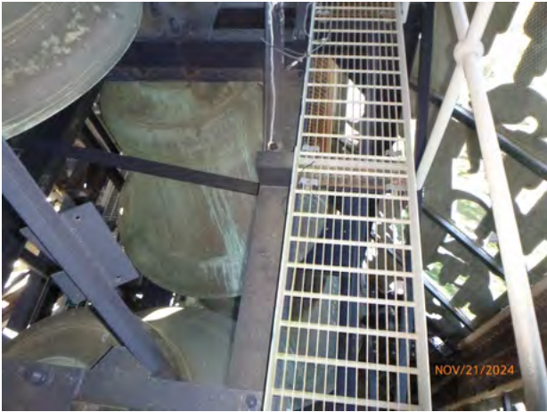
538-170 ArchMetal_Coating Coating Failed 2024-1.jpg
