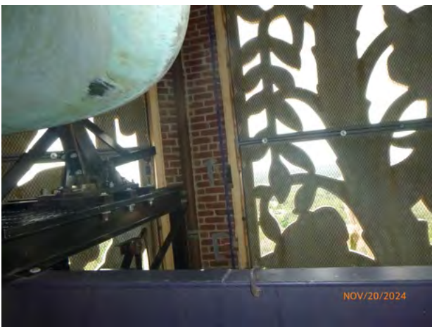
658-149 Brick_Unsecured Missing 2024-1.jpg
