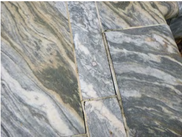
55-1 Stone_Joints Mortar Failed 2024-2.jpg
