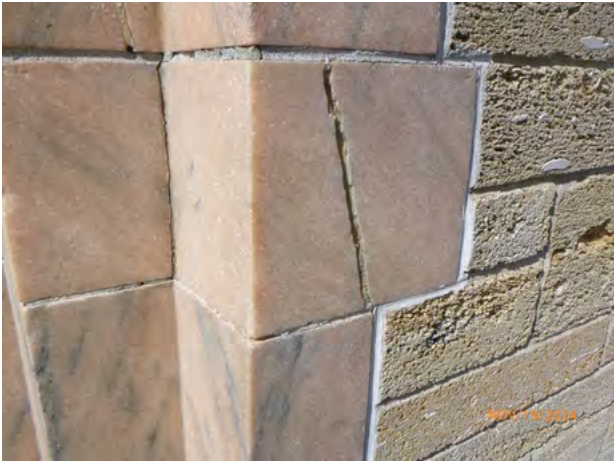
336-132 Stone_Crack Repair failed 2024-2.jpg
