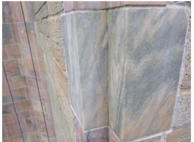
135-108 Stone_Crack Single unit 2024-1.jpg
