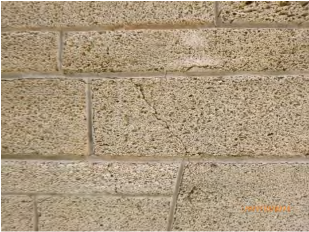
336-13 Stone_Crack System units and joints 2024-2.jpg
