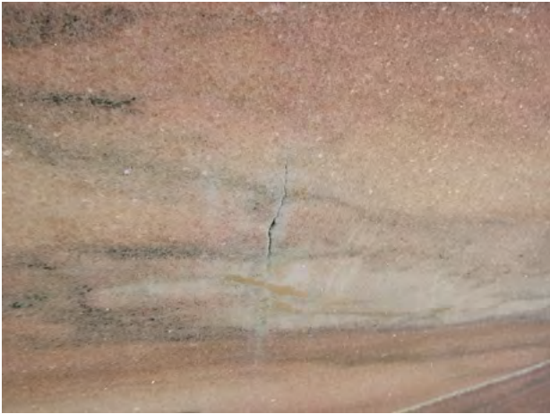
286-103 Stone_Crack Single unit 2024-1.jpg
