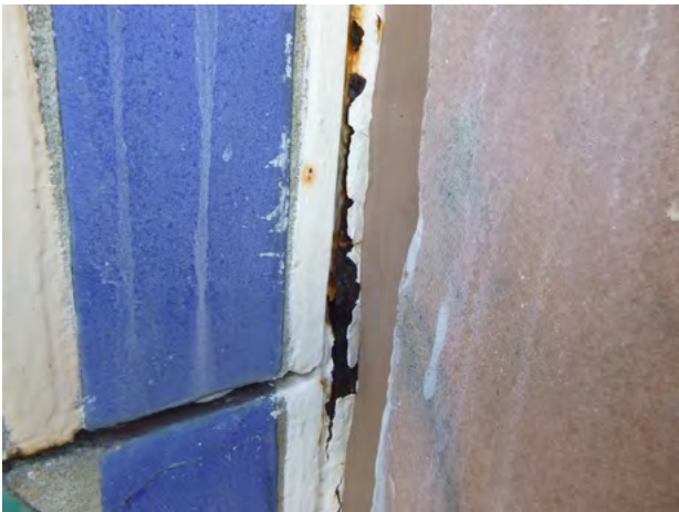
18-169 ArchMetal_Corrosion Pitted 2024-1.jpg
