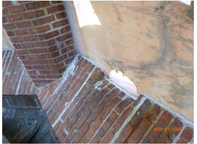
860-184 Brick_Joints Sealant Failed 2024-5.jpg
