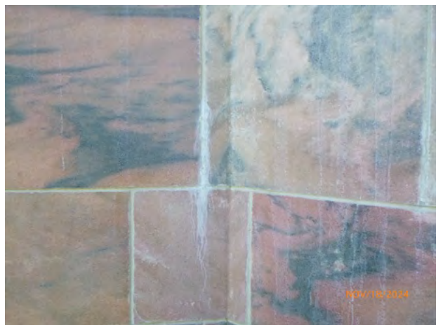
32-136 Stone_SoilStain Leached Salts 2024-1.jpg
