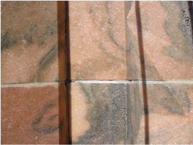
336-188 Stone_Joints Mortar Failed 2024-2.jpg
