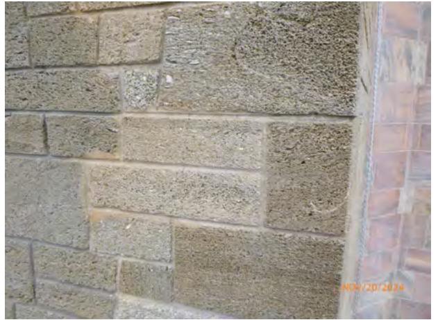
66-77 Stone_Crack Single unit 2024-1.jpg
