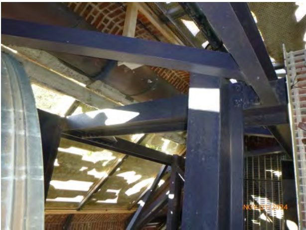
764-157 ArchMetal_Coating Coating Failed 2024-1.jpg
