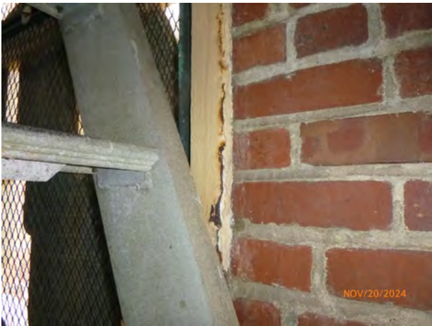
653-163 ArchMetal_Coating Coating Failed 2024-1.jpg
