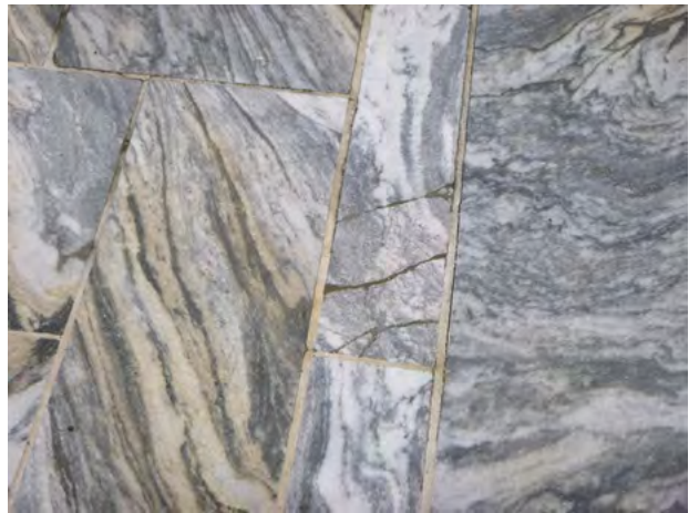
55-1 Stone_Joints Mortar Failed 2024-3.jpg
