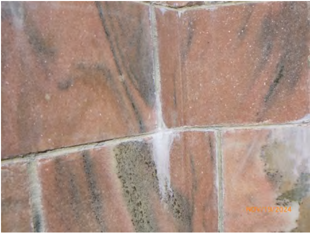
342-131 Stone_SoilStain Leached Salts 2024-3.jpg
