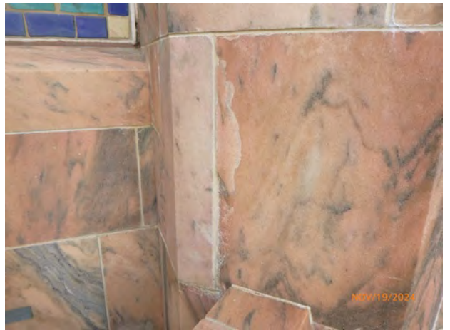
167-142 Stone_SurfLoss Chipped 2024-1.jpg
