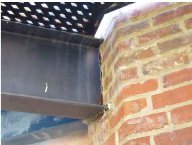
643-193 ArchMetal_Corrosion Surface 2024-1.jpg
