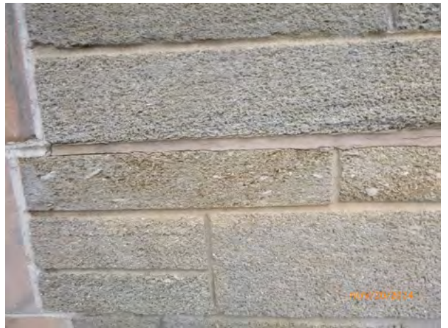
62-81 Stone_Joints Sealant Failed 2024-2.jpg
