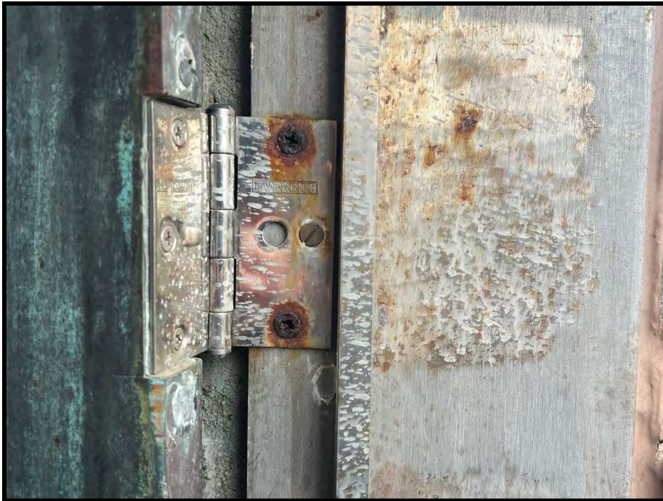
Figure 40 Corroded fasteners require replacement
