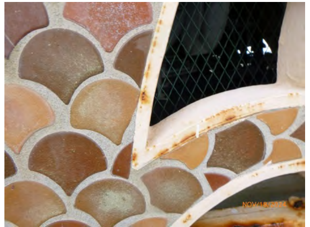
392-174 ArchMetal_Coating Coating Failed 2024-4.jpg
