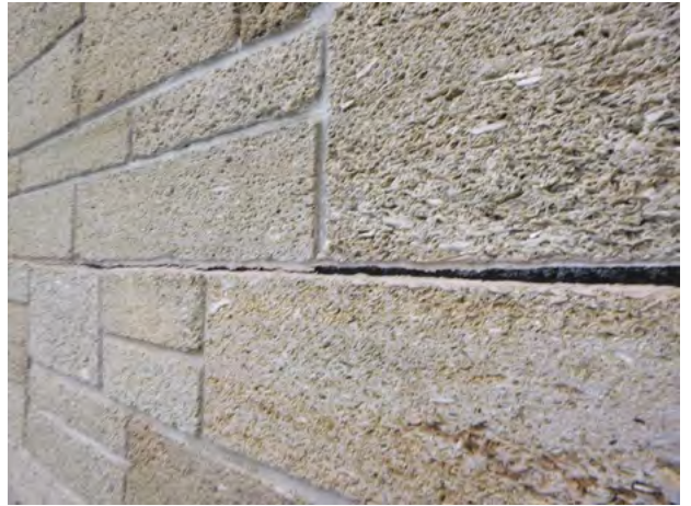
139-121 Stone_Joints Sealant Failed 2024-1.jpg
