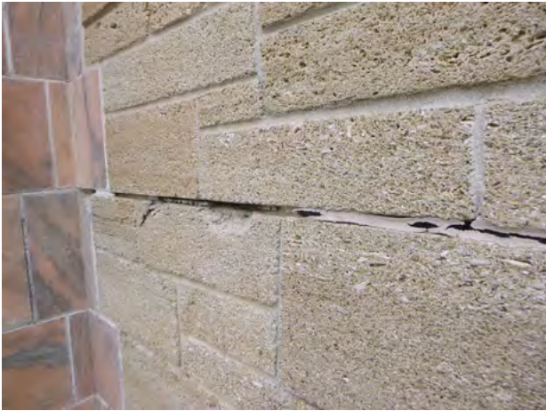
150-90 Stone_Joints Sealant Failed 2024-1.jpg
