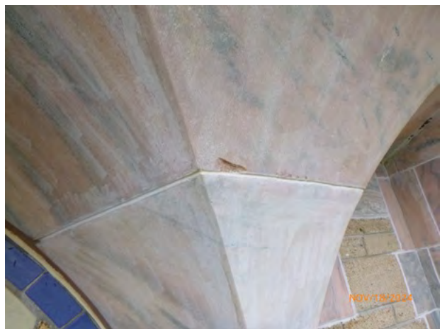
353-119 Stone_SurfLoss Chipped 2024-1.jpg
