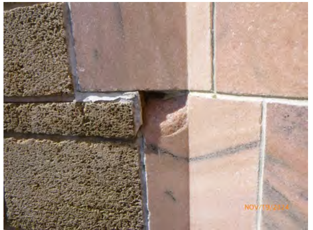
340-90 Stone_Spall Missing + Steel 2024-1.jpg
