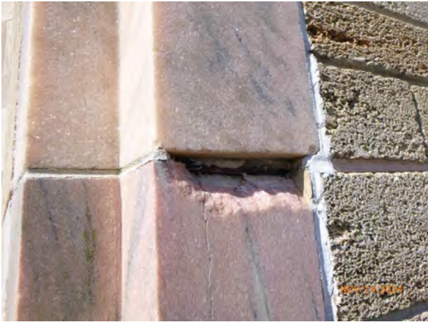
334-98 Stone_Spall Missing + Steel 2024-1.jpg
