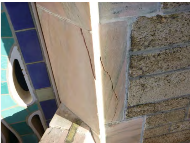
253-105 Stone_Crack Single unit 2024-1.jpg
