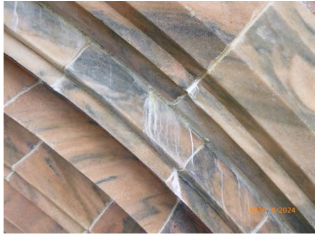
241-178 Stone_SoilStain Leached Salts 2024-2.jpg
