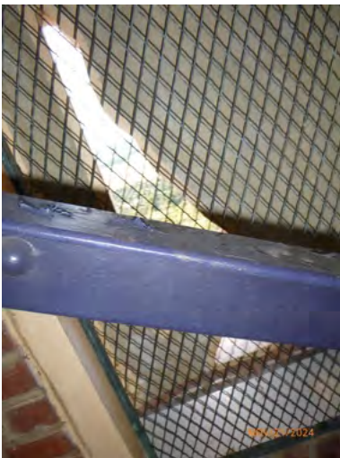
746-144 ArchMetal_Coating Coating Failed 2024-3.jpg
