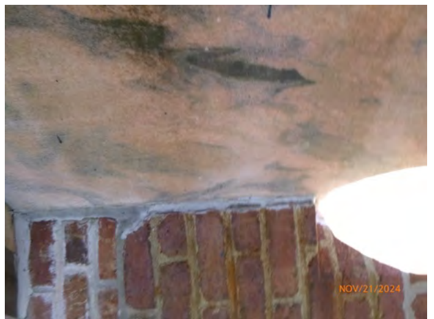
757-184 Brick_Joints Sealant Failed 2024-3.jpg
