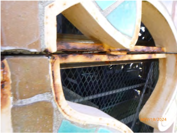
12-163 ArchMetal_Corrosion Pitted 2024-2.jpg
