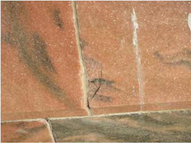
253-184 Stone_Spall Missing 2024-1.jpg
