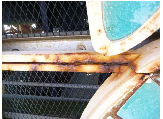
15-163 ArchMetal_Corrosion Pitted 2024-1.jpg
