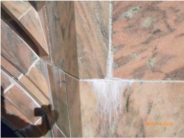
341-176 Stone_SoilStain Leached Salts 2024-2.jpg
