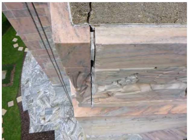
135-32 Stone_Crack System units and joints 2024-4.jpg
