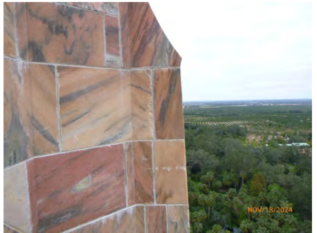
355-181 Stone_SurfLoss Chipped 2024-1.jpg
