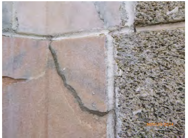
60-70 Stone_Crack Single unit 2024-3.jpg
