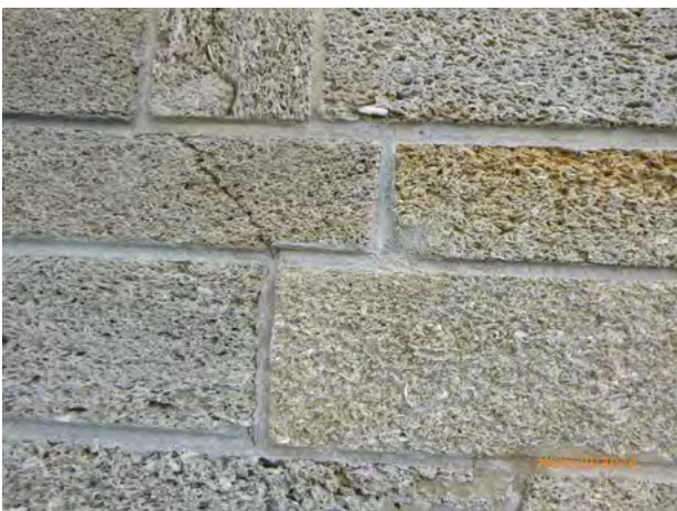
65-116 Stone_Crack System units and joints 2024-3.jpg
