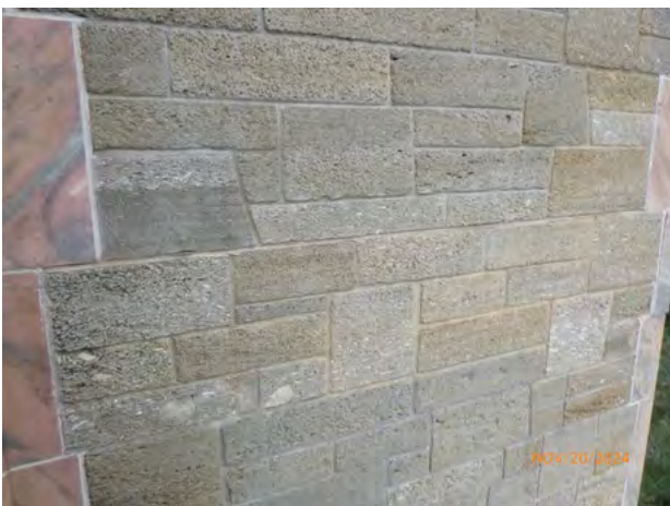
61-127 Stone_Joints Sealant Failed 2024-1.jpg
