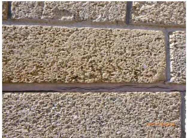
340-68 Stone_Joints Sealant Failed 2024-3.jpg
