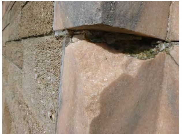
334-135 Stone_Spall Missing 2024-1.jpg
