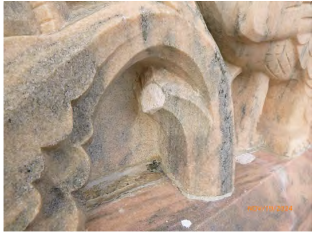
237-139 Stone_Spall Missing 2024-2.jpg
