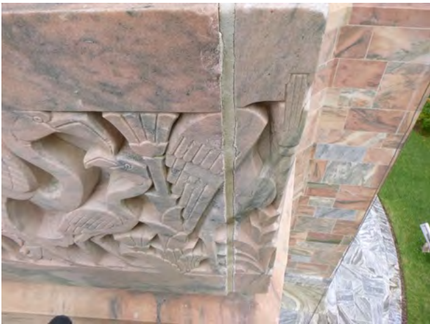
167-29 Stone_Joints Mortar Failed 2024-1.jpg
