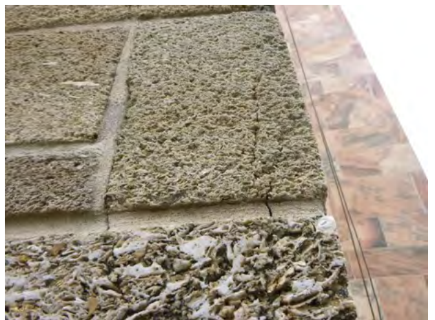
166-33 Stone_Crack System units and joints 2024-1.jpg
