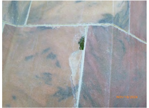
35-160 Stone_Spall Removed 2024-4.jpg
