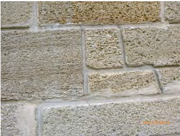
235-33 Stone_Crack System units and joints 2024-3.jpg
