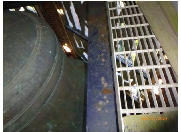
561-157 ArchMetal_Coating Coating Failed 2024-2.jpg
