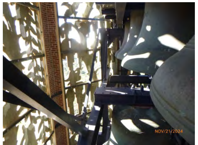
743-157 ArchMetal_Coating Coating Failed 2024-4.jpg
