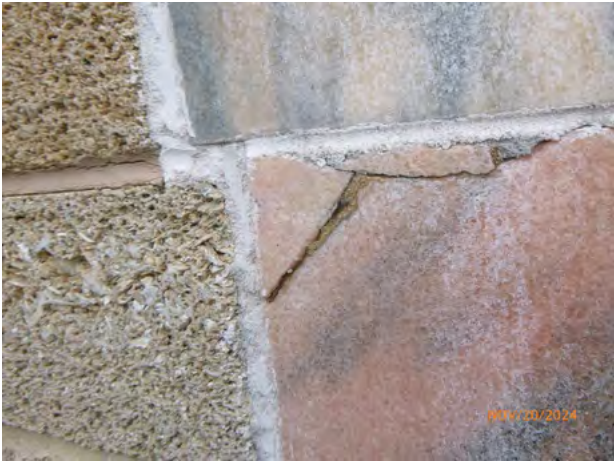
67-101 Stone_Crack Repair failed 2024-2.jpg
