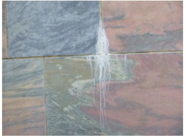
372-11 Stone_SoilStain Leached Salts 2024-1.jpg
