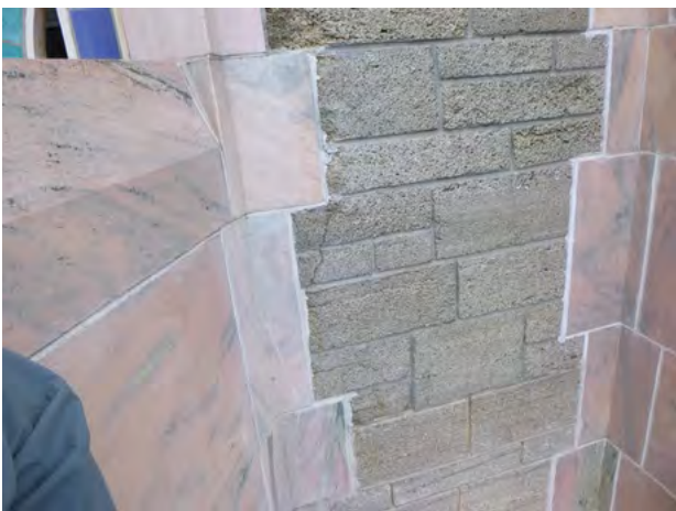
53-103 Stone_Crack System units and joints 2024-1.jpg
