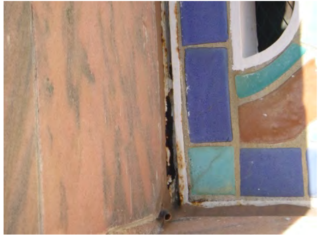
308-145 ArchMetal_Corrosion Pitted 2024-1.jpg
