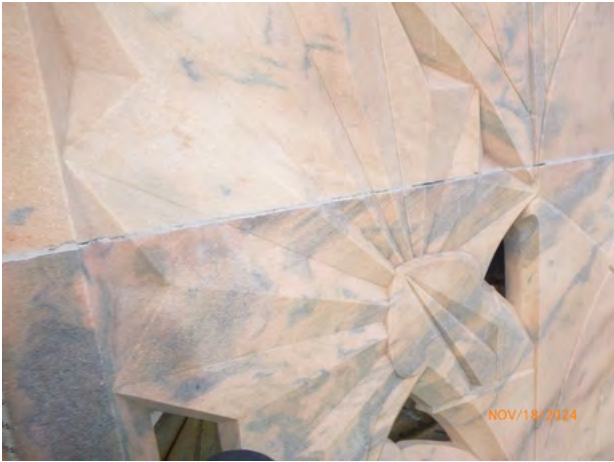
38-188 Stone_Joints Mortar Failed 2024-1.jpg
