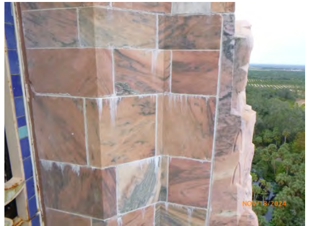
397-156 Stone_SoilStain Leached Salts 2024-2.jpg
