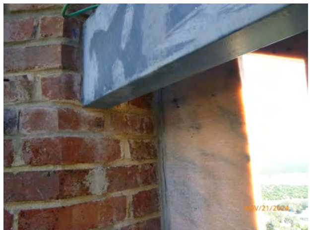
734-190 Brick_Joints Mortar Failed 2024-2.jpg
