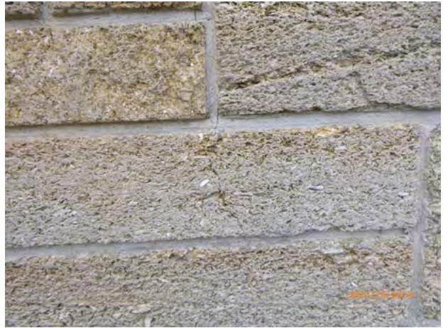
366-55 Stone_Crack System units and joints 2024-4.jpg
