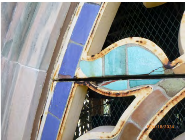
9-173 TerraCotta_Spall Missing 2024-2.jpg
