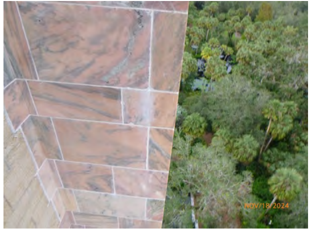
356-110 Stone_SoilStain Leached Salts 2024-1.jpg
