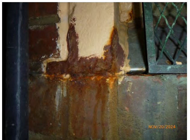
555-143 ArchMetal_Corrosion Pitted 2024-1.jpg
