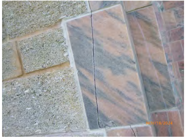
365-107 Stone_Crack System units and joints 2024-2.jpg
