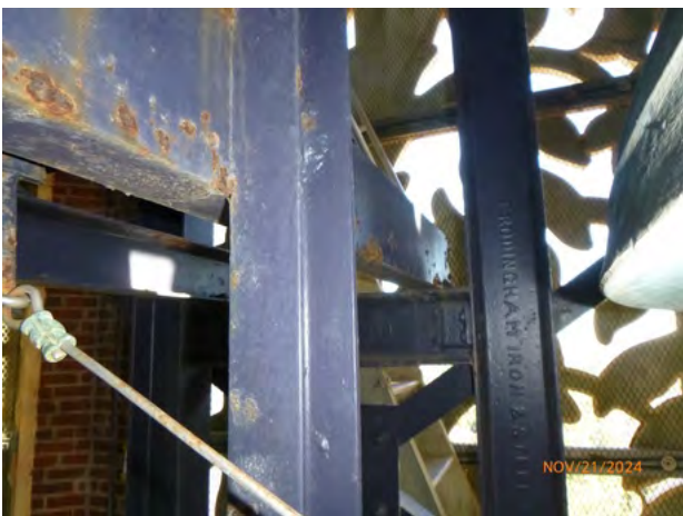
742-150 ArchMetal_Coating Coating Failed 2024-4.jpg
