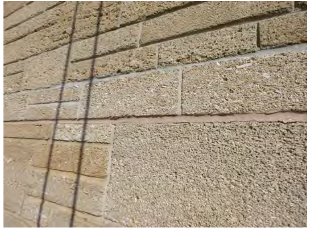
250-66 Stone_Joints Sealant Failed 2024-1.jpg
