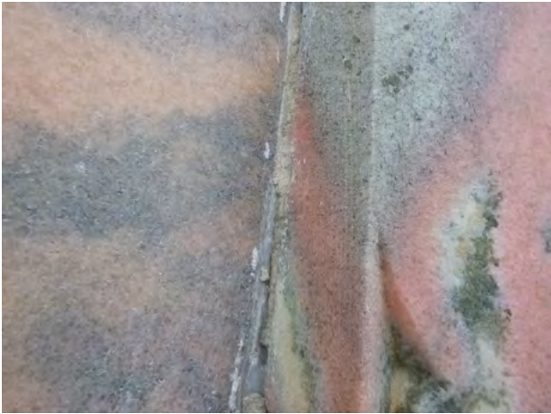
141-188 Stone_Joints Mortar Failed 2024-3.jpg
