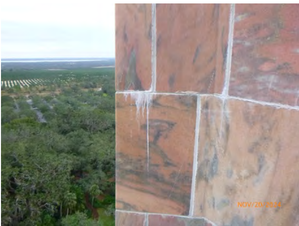
136-170 Stone_SoilStain Leached Salts 2024-4.jpg
