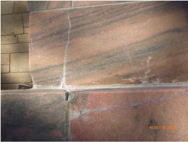
356-32 Stone_Crack Single unit 2024-2.jpg
