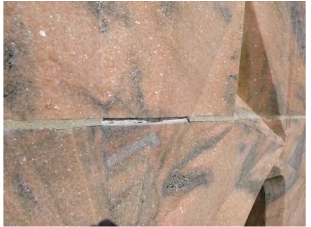
336-188 Stone_Joints Mortar Failed 2024-3.jpg
