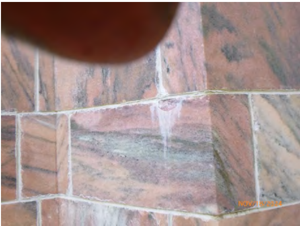
345-168 Stone_SoilStain Leached Salts 2024-2.jpg
