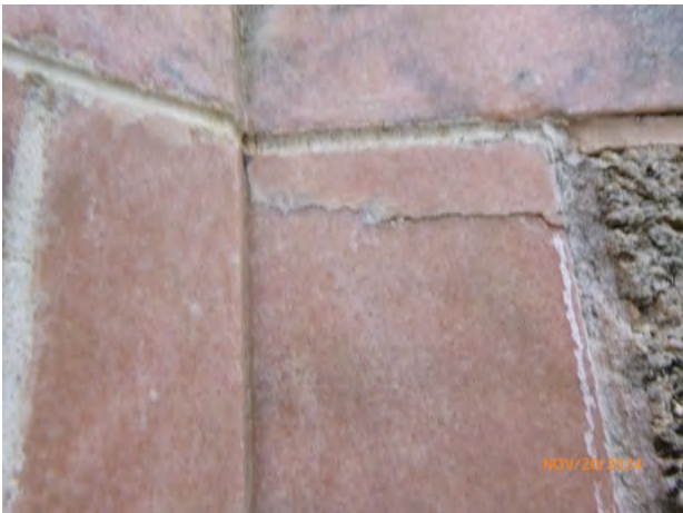
59-128 Stone_Crack Single unit 2024-3.jpg
