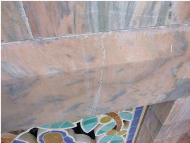
54-138 Stone_Crack Single unit 2024-1.jpg
