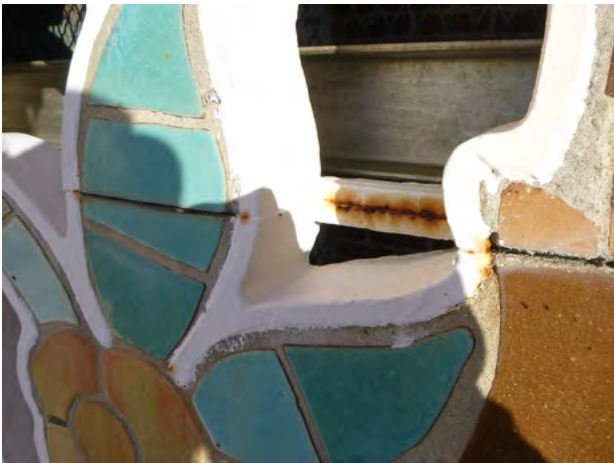
287-133 ArchMetal_Corrosion Surface 2024-1.jpg
