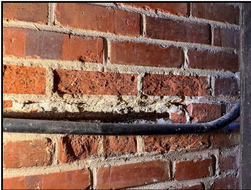
Figure 26 Spalled interior masonry and exposed embedded steel
