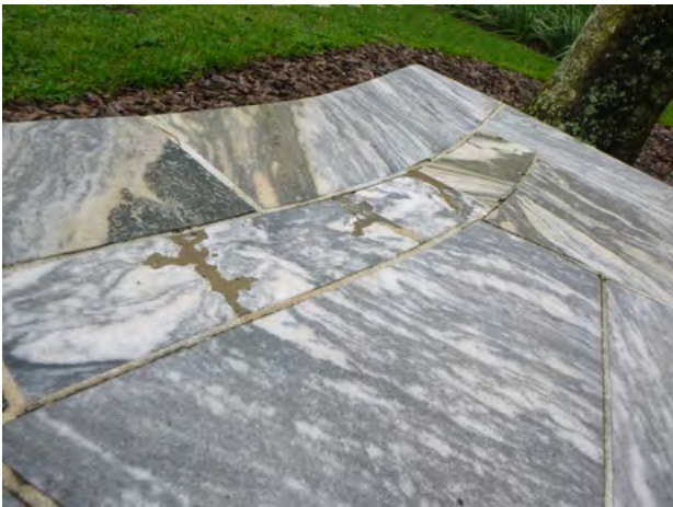
31-1 Stone_Repair Patch Failed 2024-1.jpg
