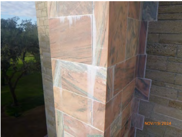
344-52 Stone_SoilStain Leached Salts 2024-2.jpg
