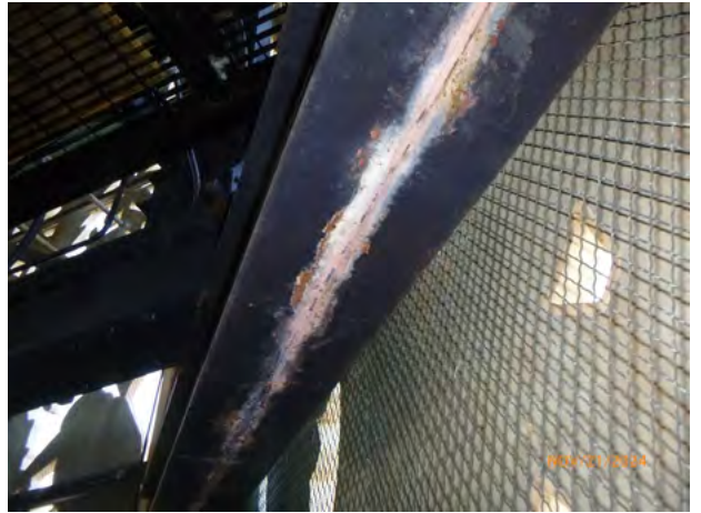
657-144 ArchMetal_Coating Coating Failed 2024-3.jpg
