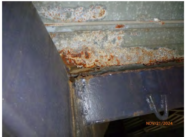
765-182 SheetMetal_Corrosion Perforated 2024-4.jpg
