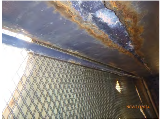
861-145 ArchMetal_Coating Coating Failed 2024-5.jpg
