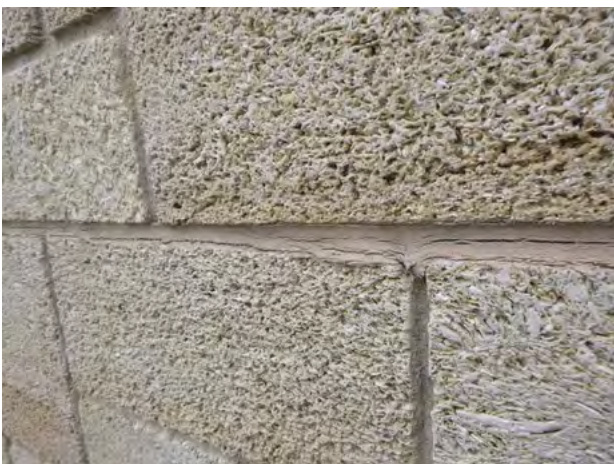
138-106 Stone_Joints Sealant Failed 2024-2.jpg
