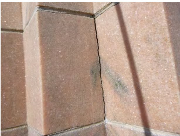
336-125 Stone_Crack Single unit 2024-1.jpg
