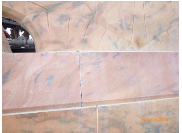
37-184 Stone_Joints Mortar Failed 2024-2.jpg
