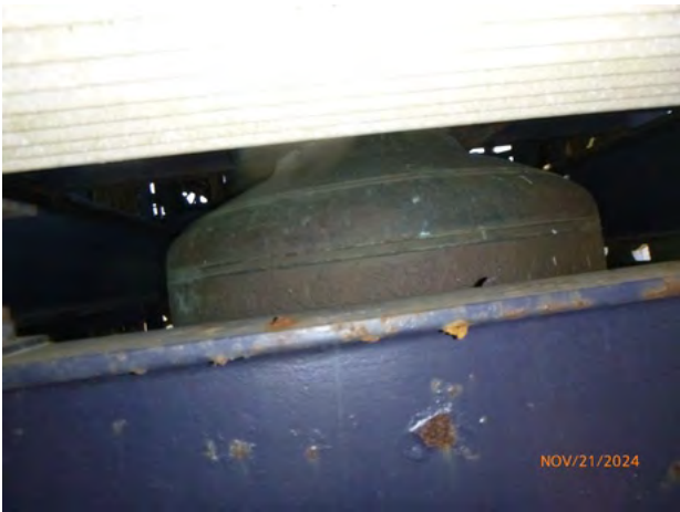
561-157 ArchMetal_Coating Coating Failed 2024-3.jpg
