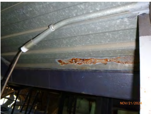
765-182 SheetMetal_Corrosion Perforated 2024-5.jpg
