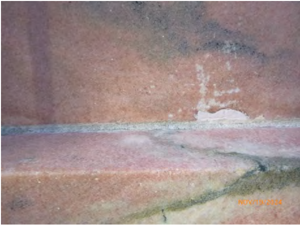
343-32 Stone_Repair Patch Failed 2024-3.jpg
