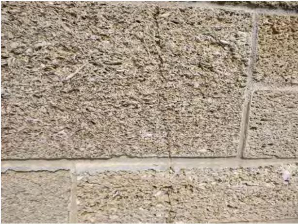
264-132 Stone_Crack System units and joints 2024-1.jpg
