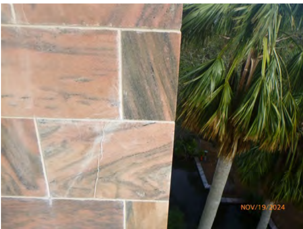
357-45 Stone_SoilStain Leached Salts 2024-2.jpg
