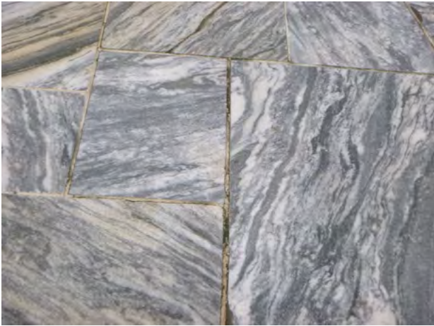
355-1 Stone_Joints Mortar Failed 2024-1.jpg
