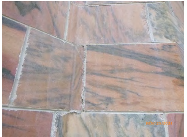
133-148 Stone_SurfLoss Chipped 2024-1.jpg
