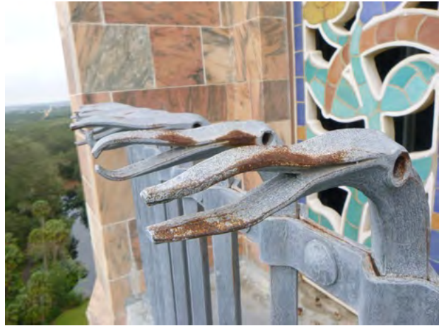
186-128 ArchMetal_Corrosion Surface 2024-1.jpg
