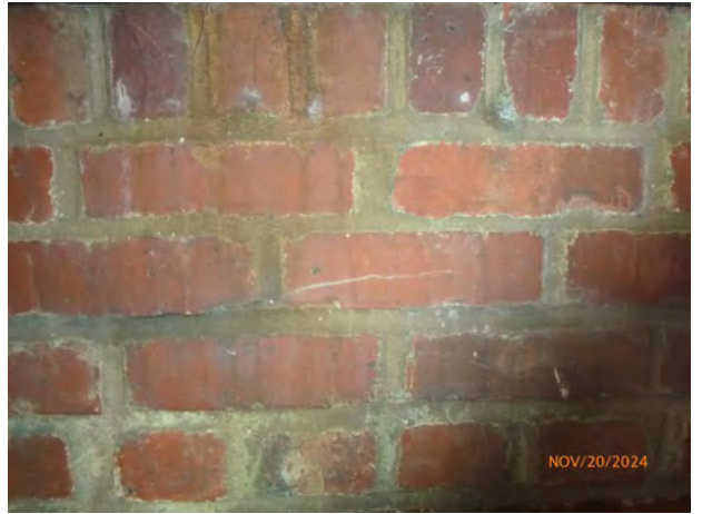
753-143 Brick_Crack System units and joints 2024-1.jpg
