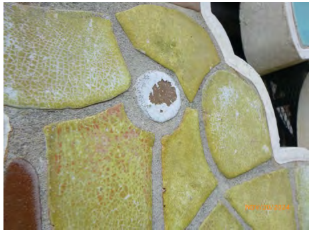
116-171 TerraCotta_SurfLoss Glaze loss 2024-3.jpg
