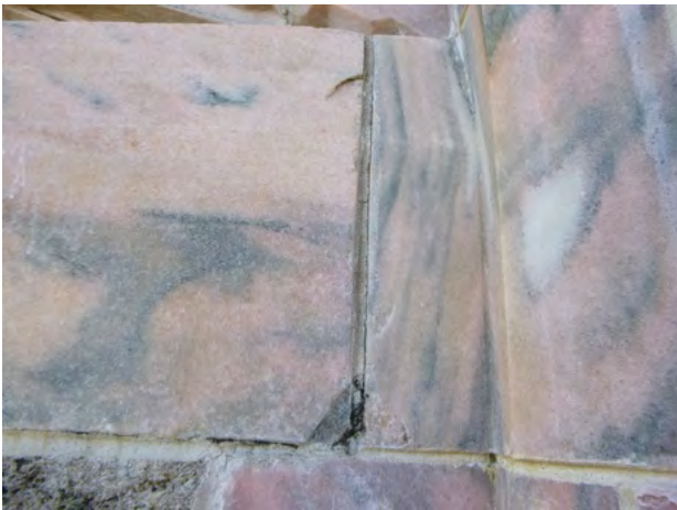
41-138 Stone_SurfLoss Chipped 2024-1.jpg
