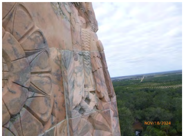
356-197 Stone_Spall Missing 2024-1.jpg
