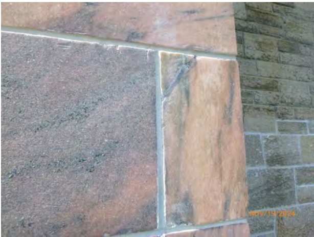
344-88 Stone_Crack System units and joints 2024-3.jpg
