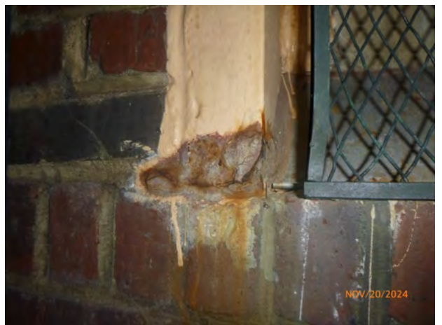
847-143 ArchMetal_Corrosion Pitted 2024-1.jpg
