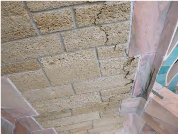
146-108 Stone_Crack System units and joints 2024-3.jpg
