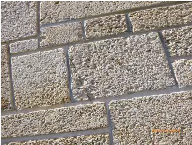
336-82 Stone_Crack Single unit 2024-1.jpg
