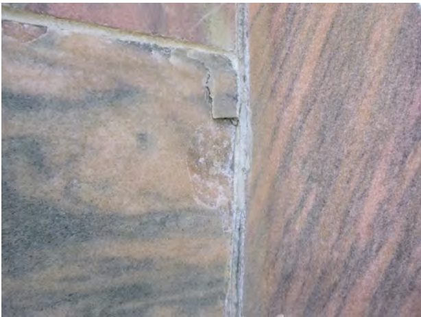
42-180 Stone_Spall Missing 2024-1.jpg
