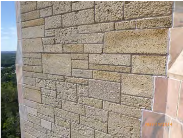
341-122 Stone_Joints Sealant Failed 2024-1.jpg
