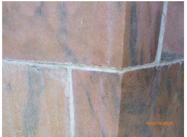
32-169 Stone_SurfLoss Chipped 2024-1.jpg
