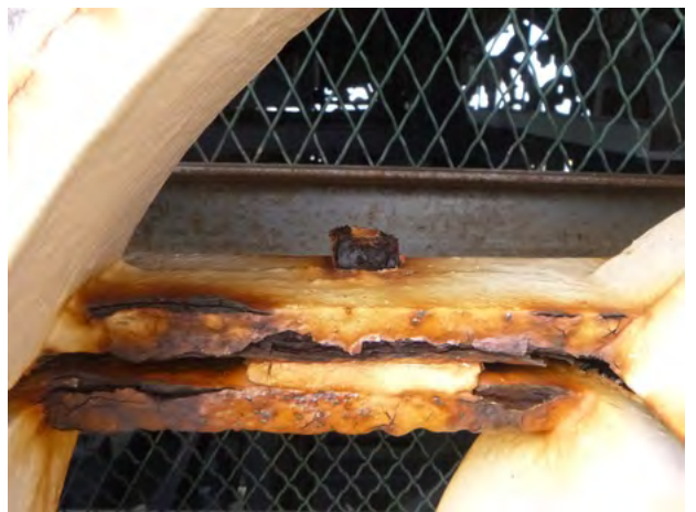
15-173 ArchMetal_Corrosion Fastener rusted 2024-1.jpg
