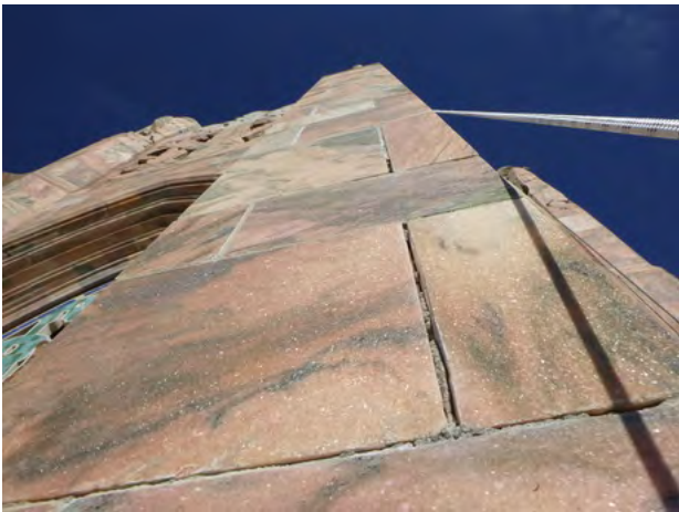
257-166 Stone_Joints Mortar Failed 2024-1.jpg
