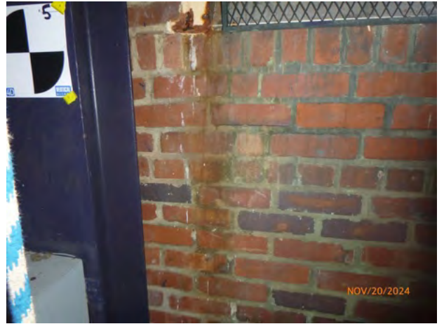
542-142 Brick_SoilStain Rust 2024-1.jpg
