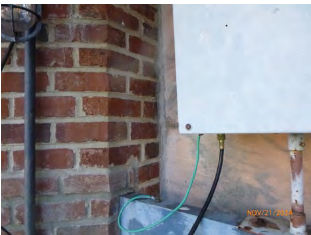
734-190 Brick_Joints Mortar Failed 2024-1.jpg
