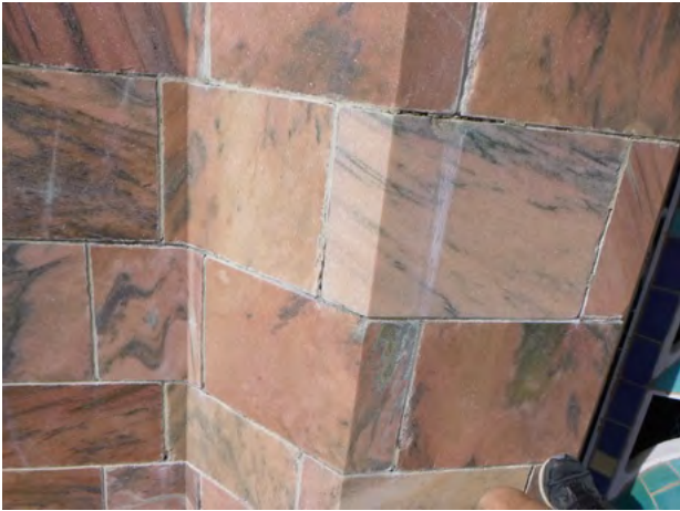
305-156 Stone_Joints Mortar Failed 2024-2.jpg
