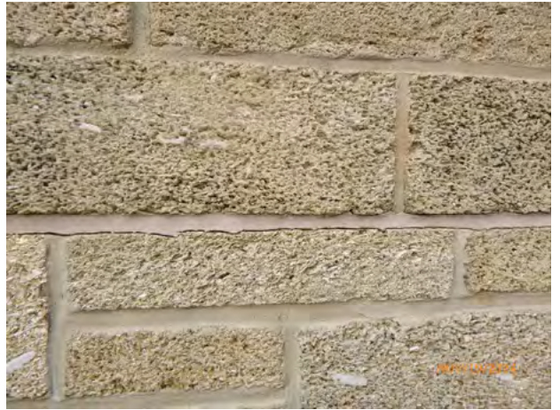
240-101 Stone_Joints Sealant Failed 2024-3.jpg
