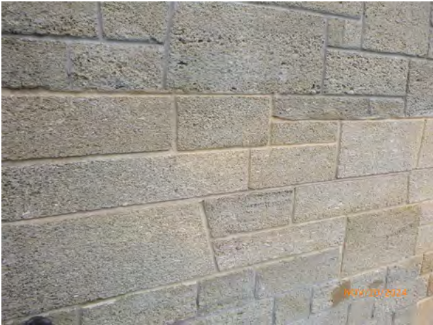
61-71 Stone_Joints Sealant Failed 2024-1.jpg
