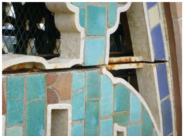
90-173 ArchMetal_Corrosion Pitted 2024-1.jpg
