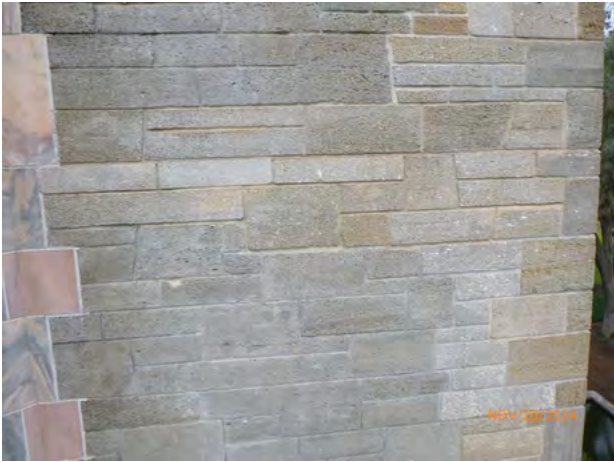
61-37 Stone_Joints Sealant Failed 2024-1.jpg
