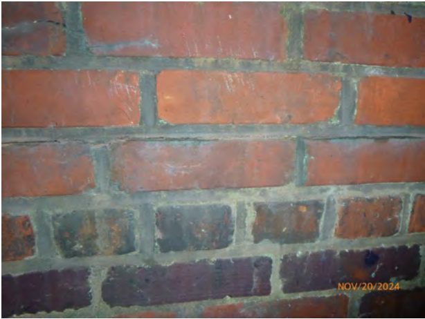
548-143 Brick_Joints Mortar Failed 2024-3.jpg
