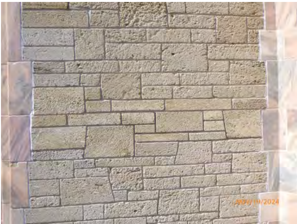
340-106 Stone_Joints Sealant Failed 2024-3.jpg
