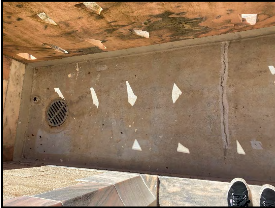
Figure 41 Large split in a balcony roof membrane
