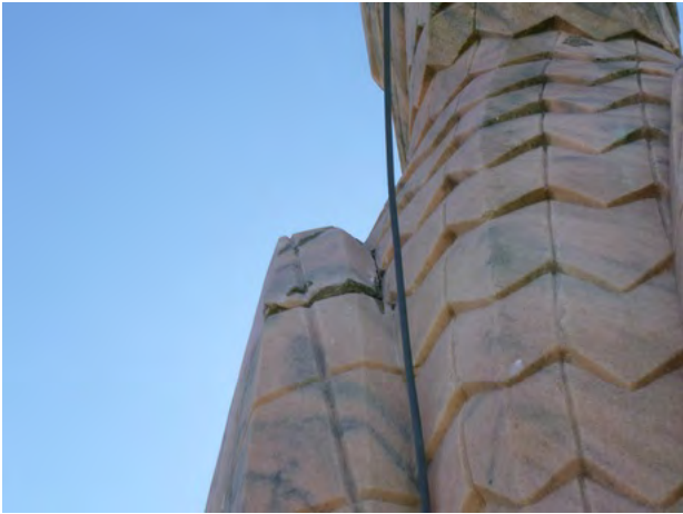
868-203 Stone_Repair Patch Failed 2024-2.jpg
