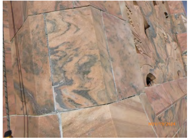
245-185 Stone_Joints Mortar Failed 2024-1.jpg
