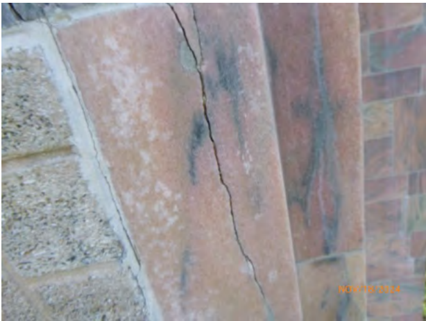
365-107 Stone_Crack System units and joints 2024-3.jpg
