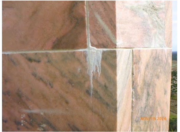
170-170 Stone_SoilStain Leached Salts 2024-1.jpg
