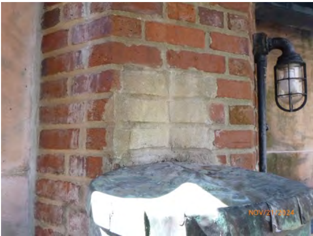
756-190 Brick_Repair Patch Failed 2024-1.jpg
