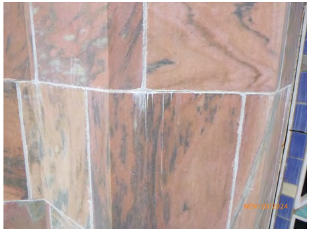
136-170 Stone_SoilStain Leached Salts 2024-3.jpg
