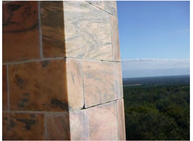
258-89 Stone_Joints Mortar Failed 2024-1.jpg
