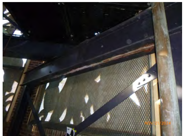
657-144 ArchMetal_Coating Coating Failed 2024-1.jpg
