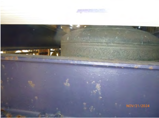
561-157 ArchMetal_Coating Coating Failed 2024-7.jpg
