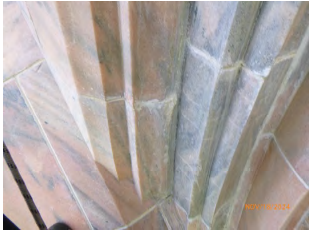
36-179 Stone_SoilStain Leached Salts 2024-2.jpg
