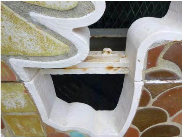
188-163 ArchMetal_Coating Coating Failed 2024-1.jpg
