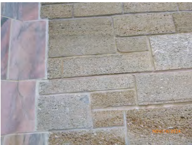
361-96 Stone_Joints Sealant Failed 2024-1.jpg
