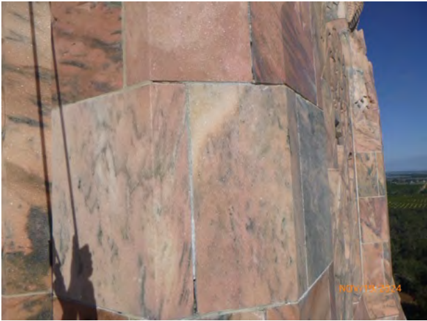
343-185 Stone_Joints Mortar Failed 2024-2.jpg
