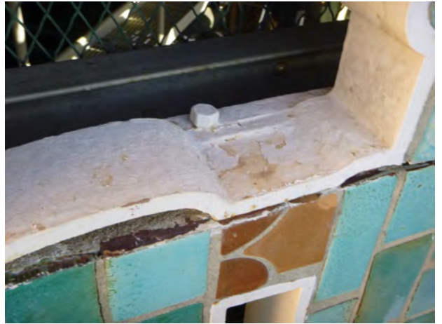
290-173 ArchMetal_Coating Coating Failed 2024-1.jpg
