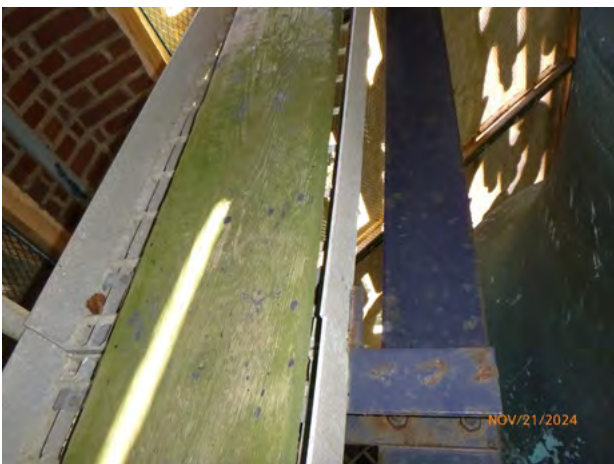
561-157 ArchMetal_Coating Coating Failed 2024-5.jpg
