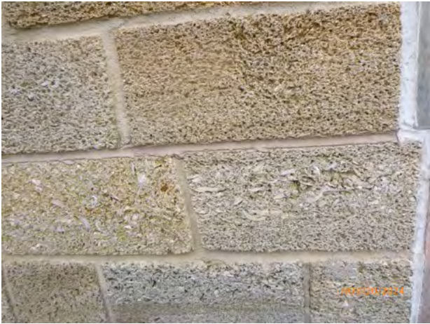
61-101 Stone_Joints Sealant Failed 2024-4.jpg
