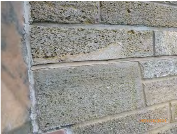
61-121 Stone_Joints Sealant Failed 2024-4.jpg
