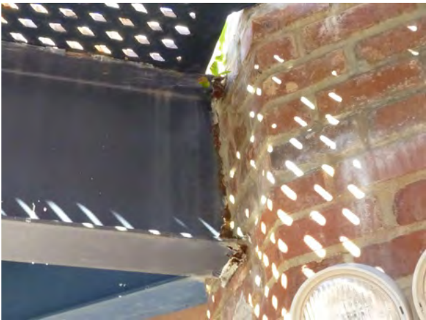
536-193 ArchMetal_Corrosion Surface 2024-1.jpg
