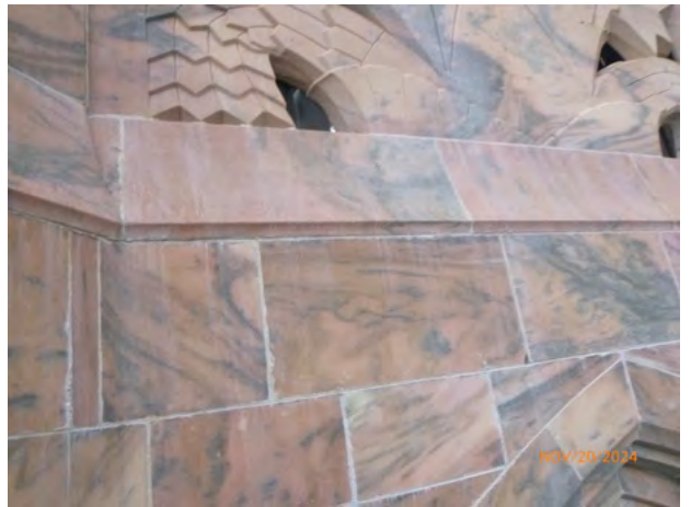
138-179 Stone_SoilStain Leached Salts 2024-1.jpg
