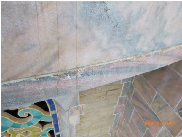
351-122 Stone_SurfLoss Chipped 2024-3.jpg
