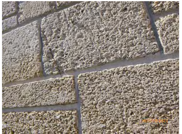
336-82 Stone_Crack Single unit 2024-2.jpg
