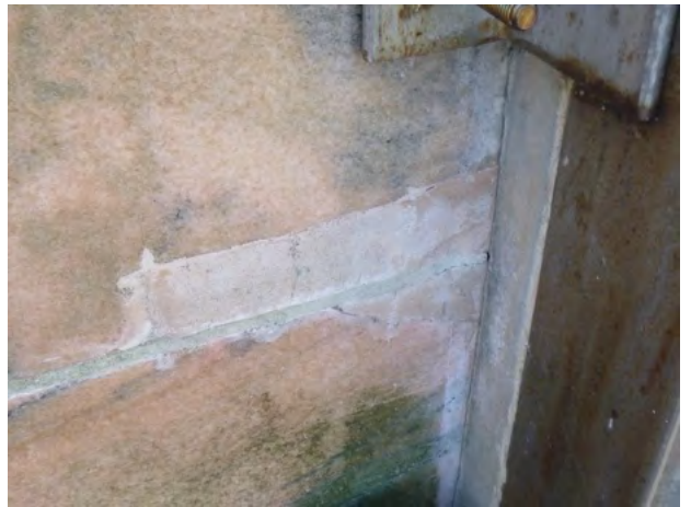
637-193 Stone_Repair Patch Failed 2024-2.jpg
