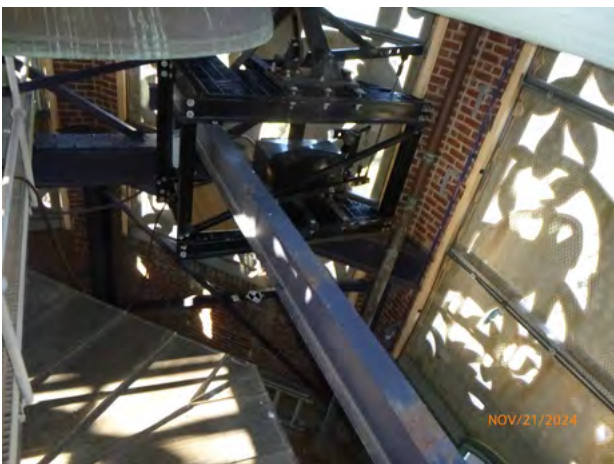
663-148 ArchMetal_Coating Coating Failed 2024-5.jpg
