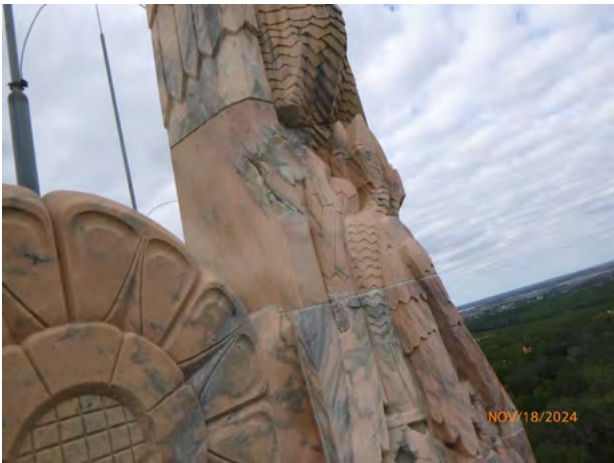
356-201 Stone_Spall Missing 2024-2.jpg
