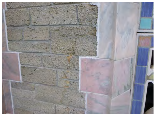
47-110 Stone_Crack System units and joints 2024-3.jpg
