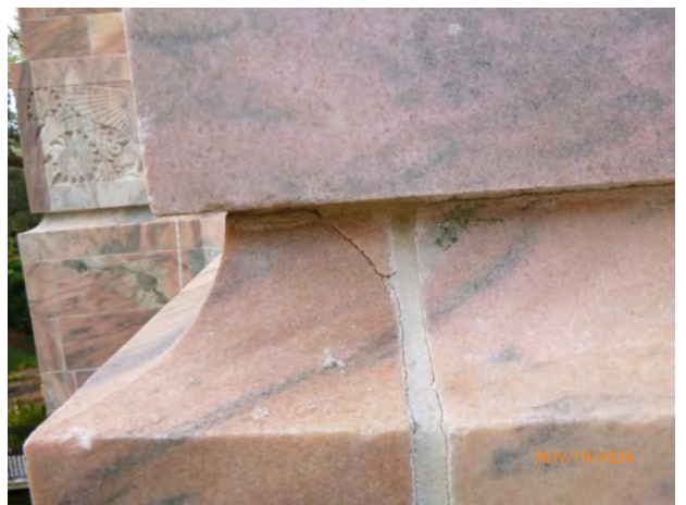
235-28 Stone_Crack Single unit 2024-2.jpg
