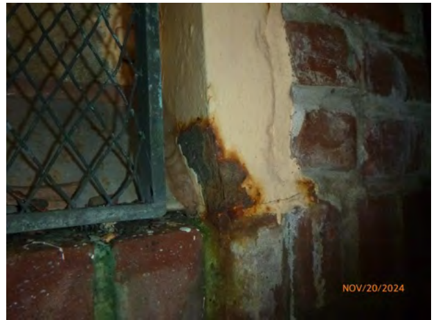
857-143 ArchMetal_Corrosion Pitted 2024-1.jpg
