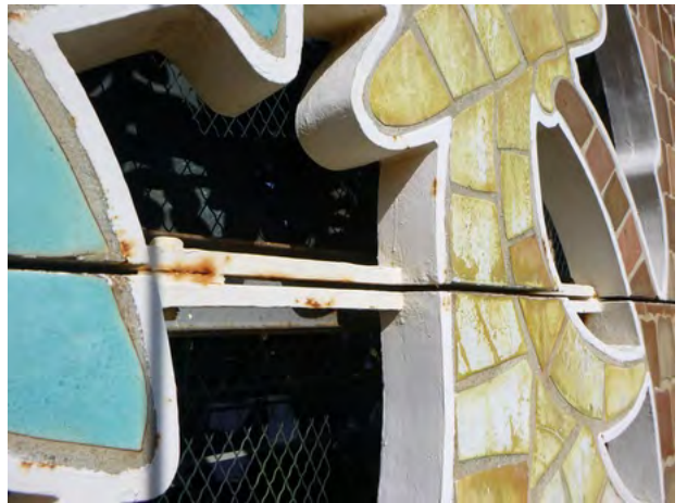
313-152 ArchMetal_Coating Coating Failed 2024-2.jpg
