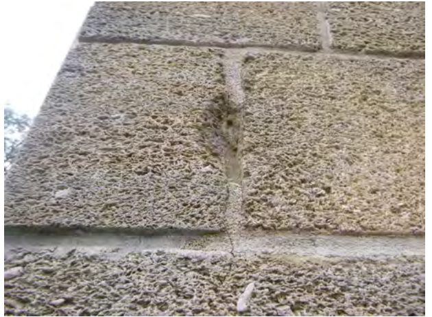
135-11 Stone_Spall Missing 2024-1.jpg
