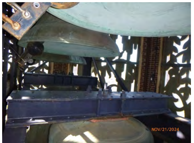
540-158 ArchMetal_Coating Coating Failed 2024-2.jpg
