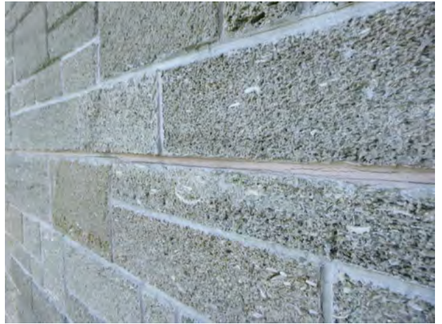
37-82 Stone_Joints Sealant Failed 2024-1.jpg
