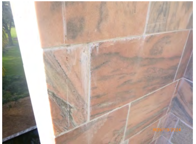
344-52 Stone_SoilStain Leached Salts 2024-3.jpg
