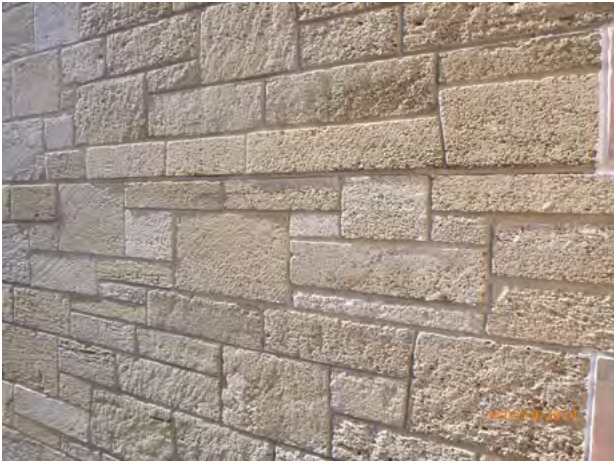
341-45 Stone_Joints Sealant Failed 2024-1.jpg
