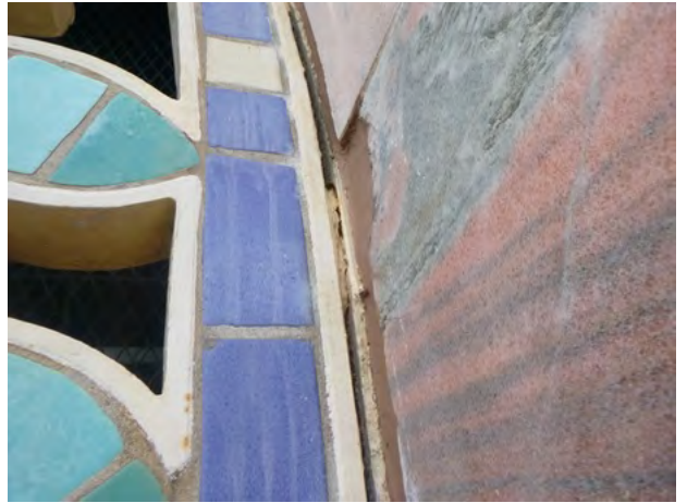
118-167 ArchMetal_Corrosion Pitted 2024-1.jpg
