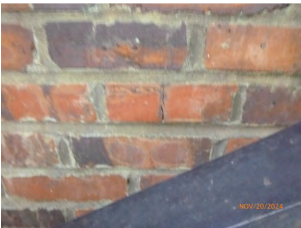
544-142 Brick_Crack Single unit 2024-1.jpg
