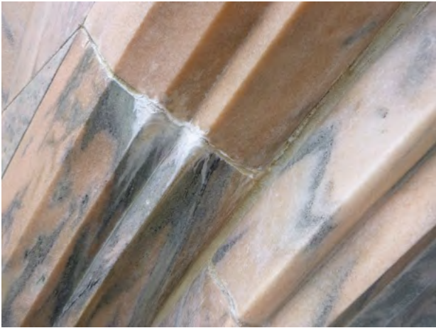
187-180 Stone_SoilStain Leached Salts 2024-2.jpg
