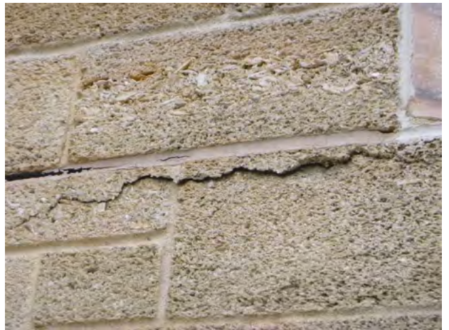
146-101 Stone_Joints Sealant Failed 2024-2.jpg
