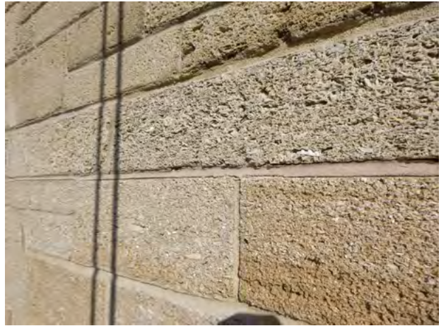
251-81 Stone_Joints Sealant Failed 2024-2.jpg
