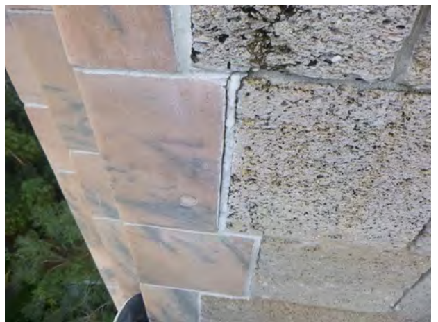
135-133 Stone_Joints Mortar Failed 2024-3.jpg
