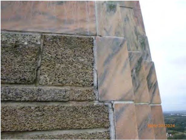
66-132 Stone_Crack System units and joints 2024-2.jpg
