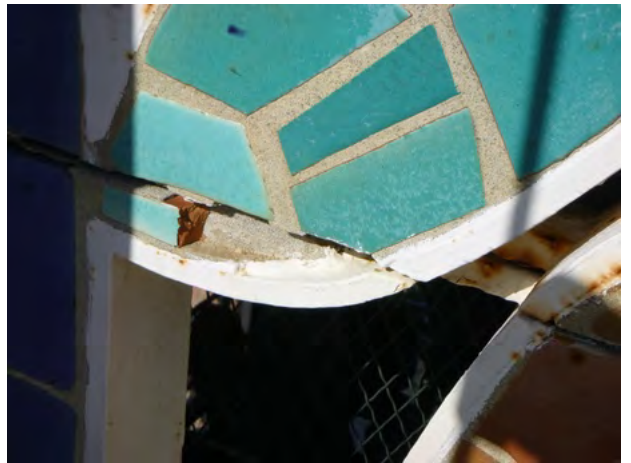
309-158 TerraCotta_Spall Missing 2024-1.jpg
