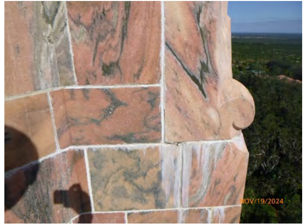
272-156 Stone_SoilStain Leached Salts 2024-2.jpg
