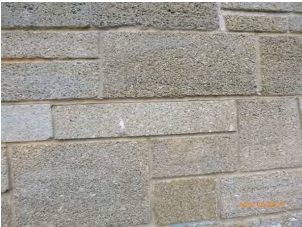
61-37 Stone_Joints Sealant Failed 2024-3.jpg
