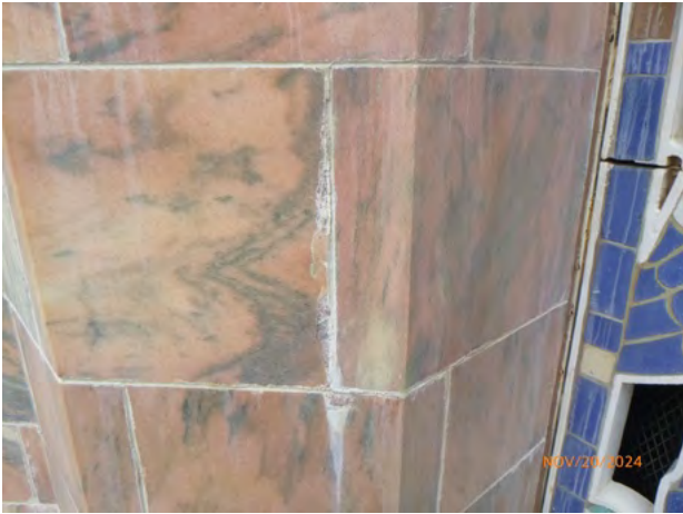
134-146 Stone_SurfLoss Chipped 2024-1.jpg
