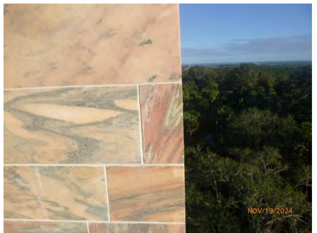
355-78 Stone_Crack Single unit 2024-1.jpg
