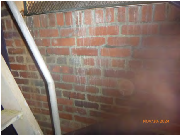
849-142 Brick_SoilStain Leached Salts 2024-1.jpg
