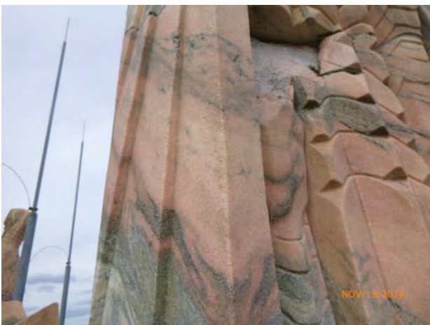
244-201 Stone_Spall Missing 2024-2.jpg
