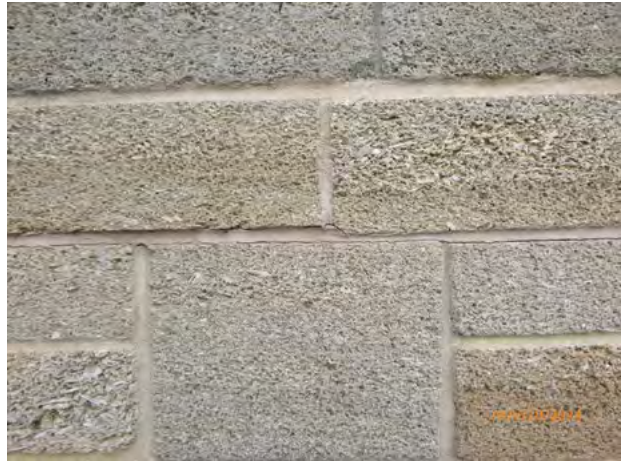
61-90 Stone_Joints Sealant Failed 2024-3.jpg
