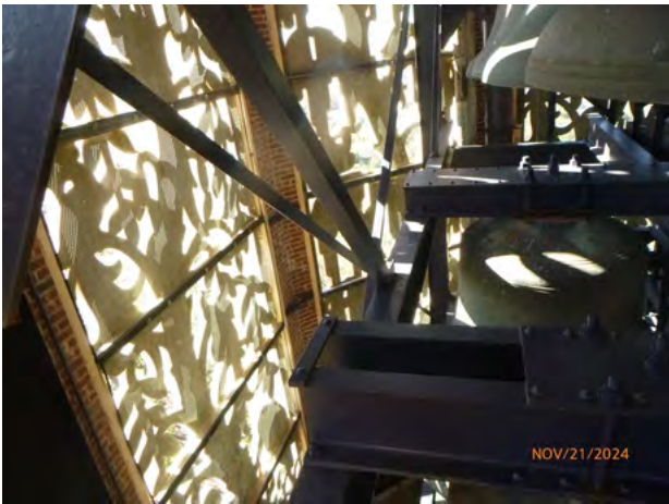
743-157 ArchMetal_Coating Coating Failed 2024-1.jpg
