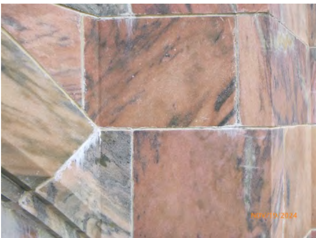
241-178 Stone_SoilStain Leached Salts 2024-5.jpg
