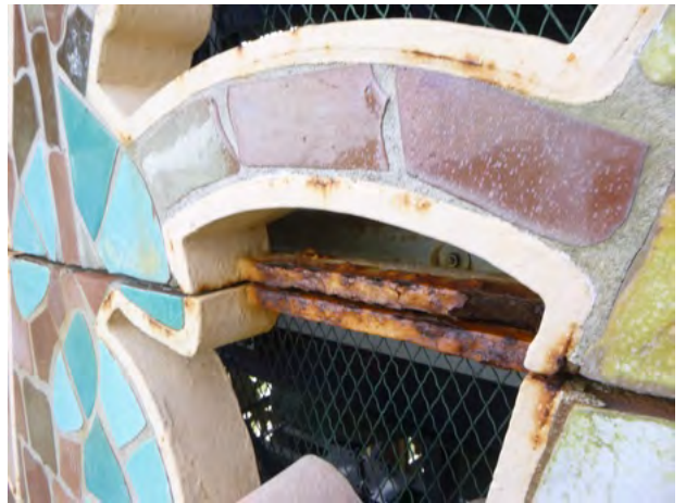
15-167 ArchMetal_Corrosion Pitted 2024-1.jpg
