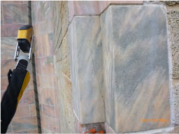
134-105 Stone_Crack Single unit 2024-1.jpg
