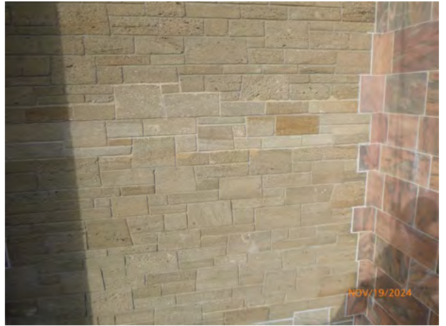
356-52 Stone_Joints Sealant Failed 2024-1.jpg
