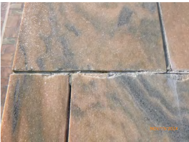
344-141 Stone_Joints Mortar Failed 2024-2.jpg
