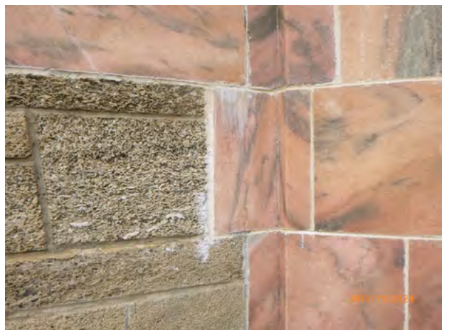
240-137 Stone_SoilStain Leached Salts 2024-1.jpg
