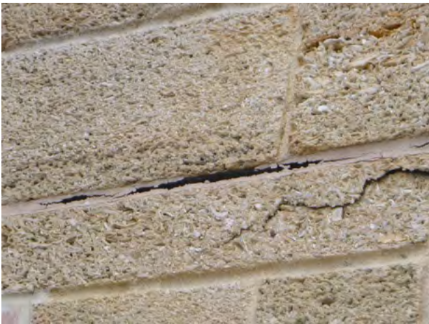
146-101 Stone_Joints Sealant Failed 2024-1.jpg
