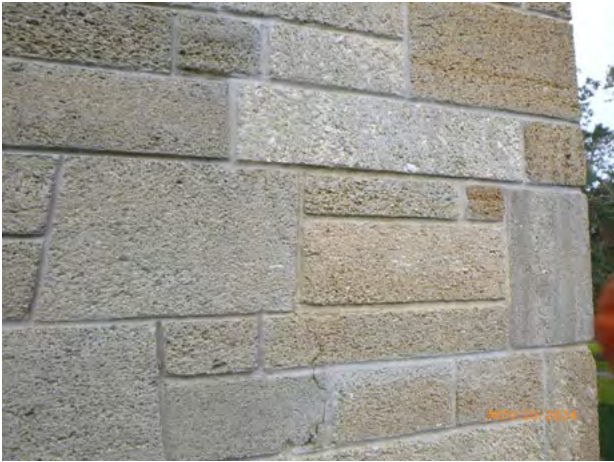
66-32 Stone_Crack System units and joints 2024-2.jpg
