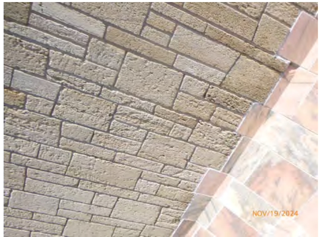
341-89 Stone_Joints Sealant Failed 2024-1.jpg
