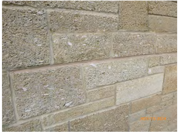
240-57 Stone_Joints Sealant Failed 2024-4.jpg
