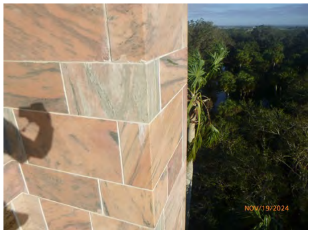
356-71 Stone_SoilStain Leached Salts 2024-1.jpg
