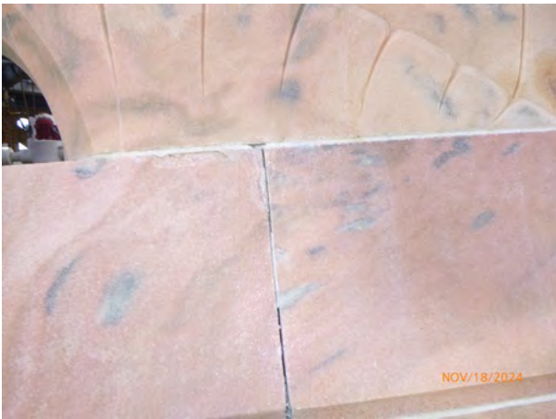
37-184 Stone_Joints Mortar Failed 2024-1.jpg
