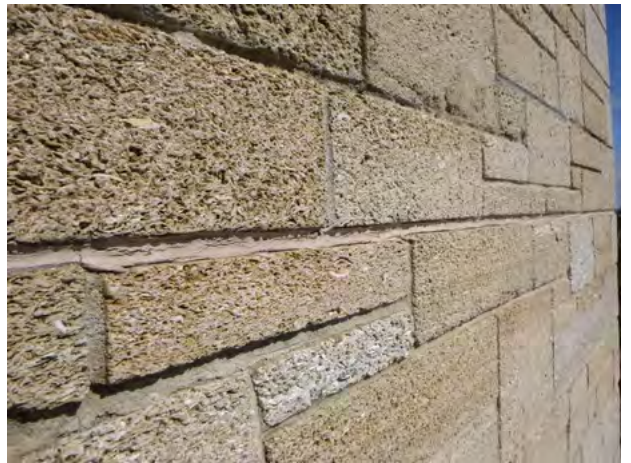
264-66 Stone_Joints Sealant Failed 2024-1.jpg
