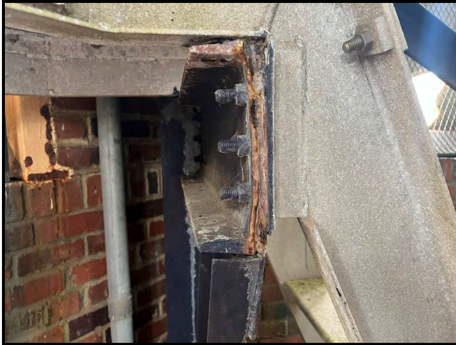
Figure 32 Corrosion at Carillon access stair
