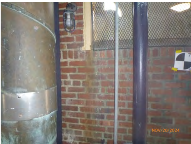
759-141 Brick_SoilStain Rust 2024-1.jpg
