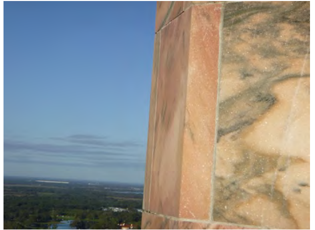
243-189 Stone_Joints Mortar Failed 2024-1.jpg
