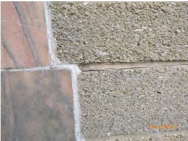
61-109 Stone_Joints Sealant Failed 2024-2.jpg
