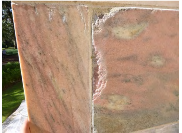
328-14 Stone_SurfLoss Chipped 2024-1.jpg
