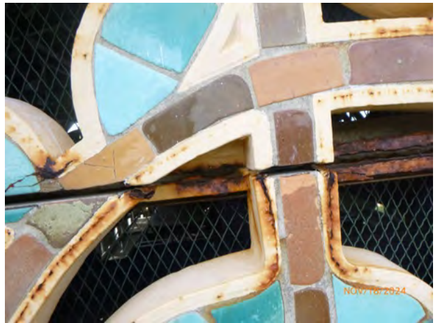
13-173 ArchMetal_Corrosion Pitted 2024-3.jpg
