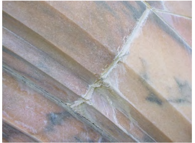
17-179 Stone_SoilStain Leached Salts 2024-1.jpg
