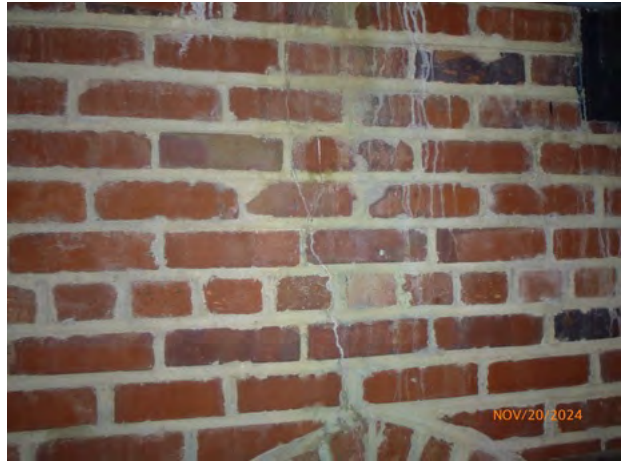
546-181 Brick_Crack System units and joints 2024-1.jpg
