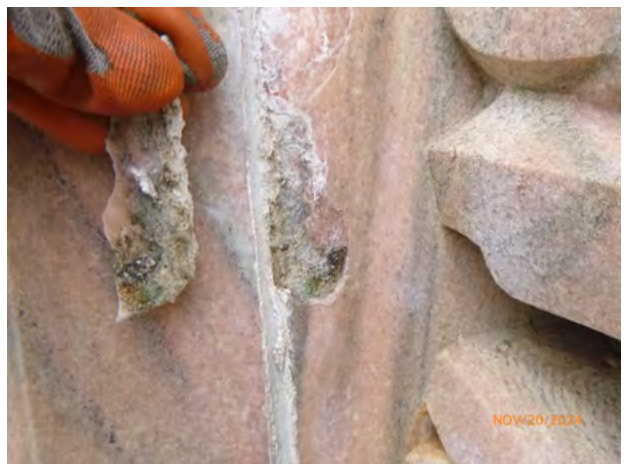
133-139 Stone_SurfLoss Chipped 2024-3.jpg
