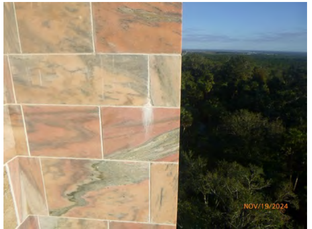
355-86 Stone_SoilStain Leached Salts 2024-1.jpg
