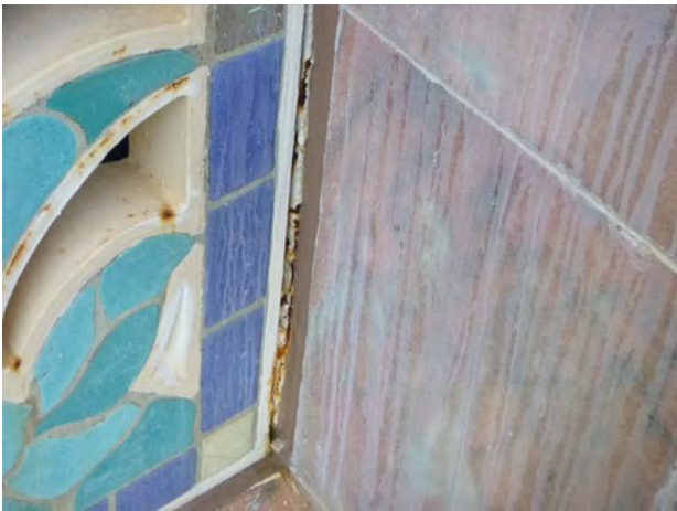
18-145 ArchMetal_Corrosion Pitted 2024-1.jpg
