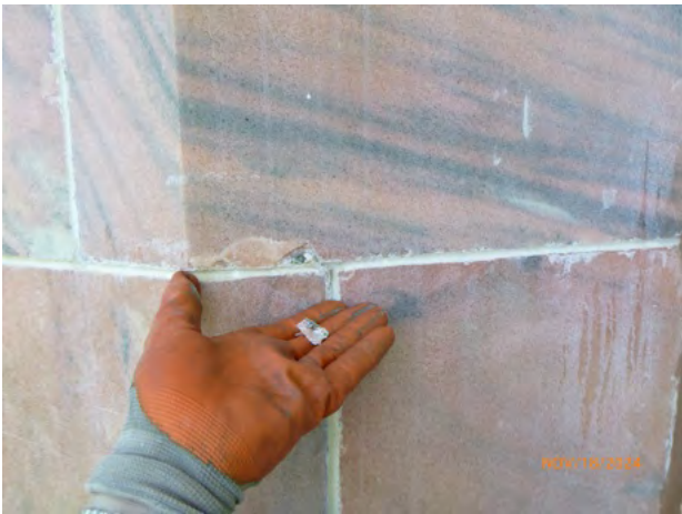
36-162 Stone_SurfLoss Chipped 2024-2.jpg
