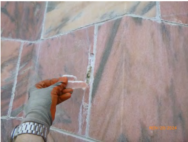
132-161 Stone_Spall Removed 2024-1.jpg
