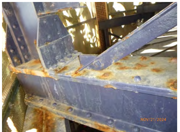
844-147 ArchMetal_Corrosion Fastener rusted 2024-1.jpg
