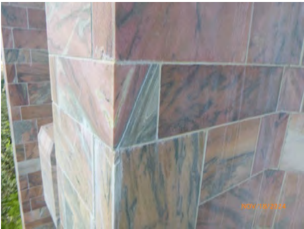
28-103 Stone_Crack Single unit 2024-1.jpg
