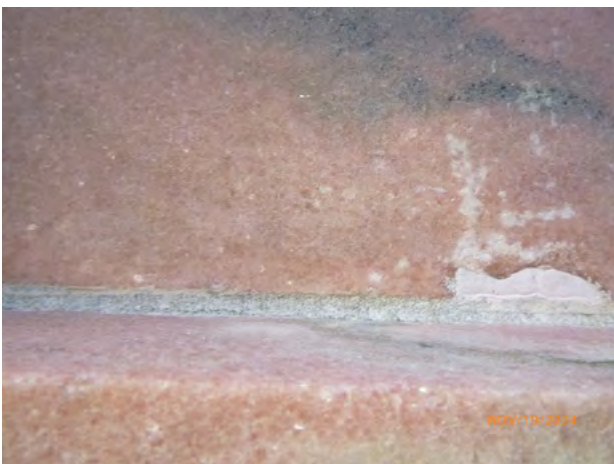
343-32 Stone_Repair Patch Failed 2024-1.jpg
