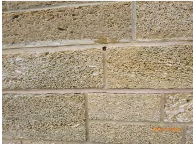
241-130 Stone_Joints Sealant Failed 2024-4.jpg
