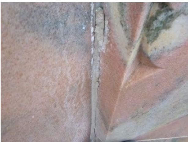
141-188 Stone_Joints Mortar Failed 2024-1.jpg
