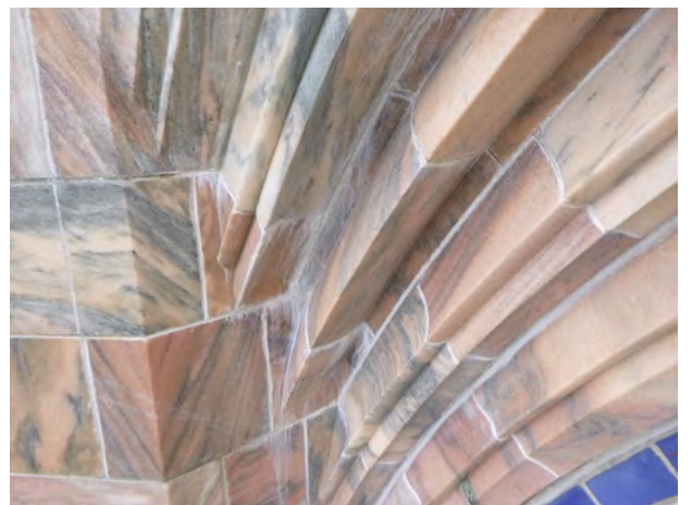
187-180 Stone_SoilStain Leached Salts 2024-1.jpg
