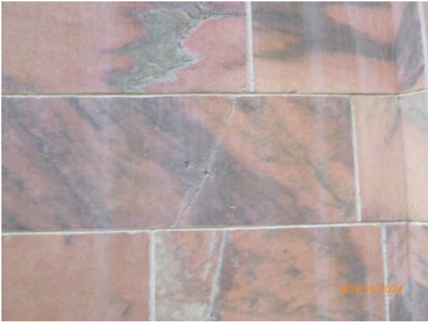
130-23 Stone_Crack Single unit 2024-1.jpg
