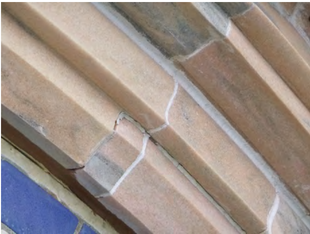
89-178 Stone_Joints Mortar Failed 2024-1.jpg
