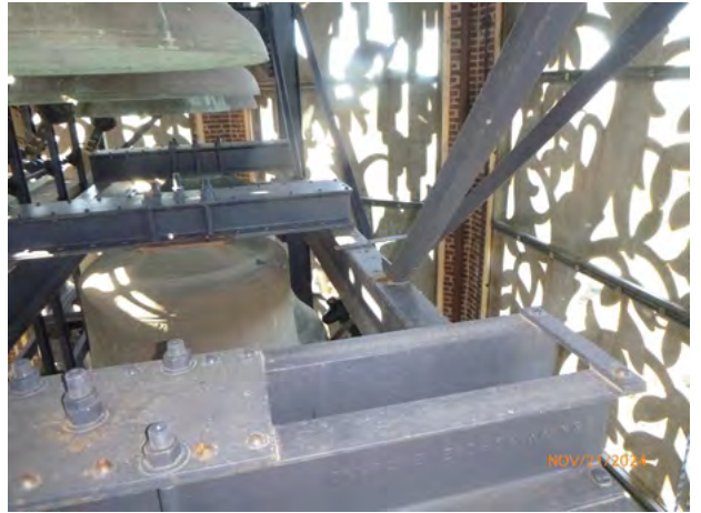
540-158 ArchMetal_Coating Coating Failed 2024-4.jpg
