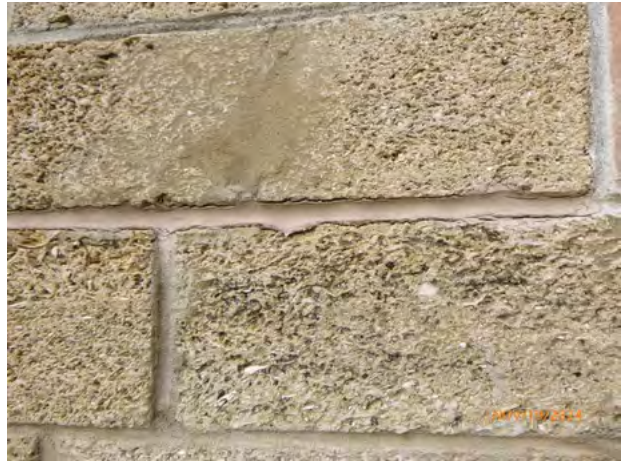
241-80 Stone_Joints Sealant Failed 2024-2.jpg
