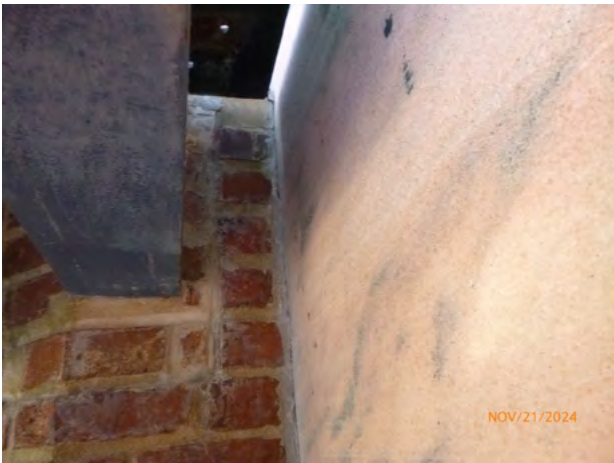
734-190 Brick_Joints Mortar Failed 2024-5.jpg
