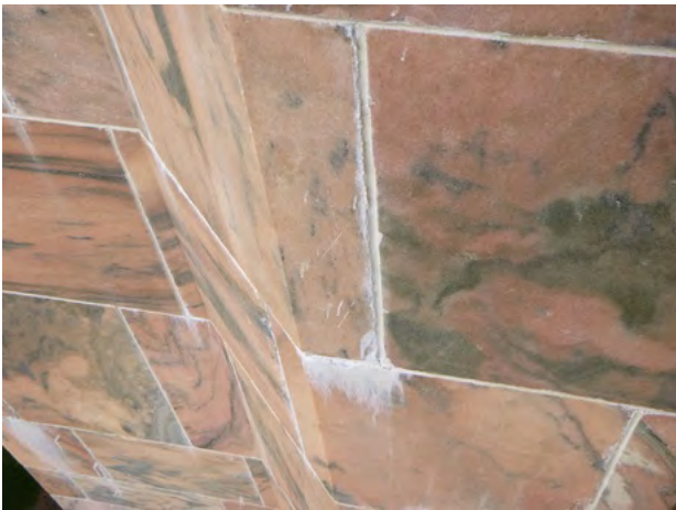
204-157 Stone_SoilStain Leached Salts 2024-3.jpg
