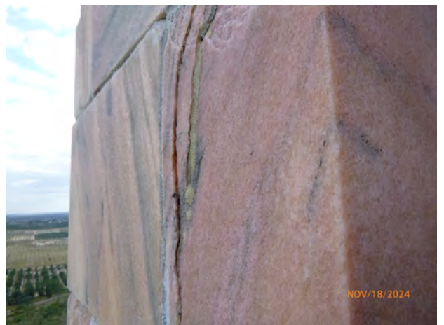
343-150 Stone_Crack Single unit 2024-3.jpg
