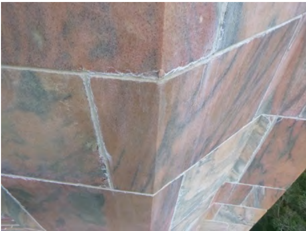
141-182 Stone_SoilStain Leached Salts 2024-3.jpg
