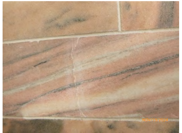
356-41 Stone_Crack Single unit 2024-3.jpg
