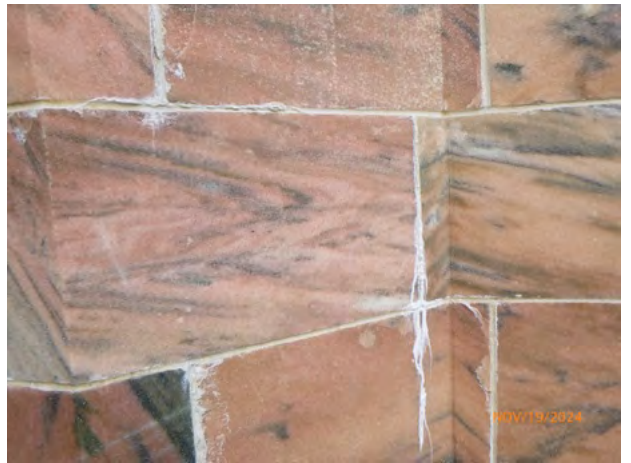
242-164 Stone_SoilStain Leached Salts 2024-1.jpg
