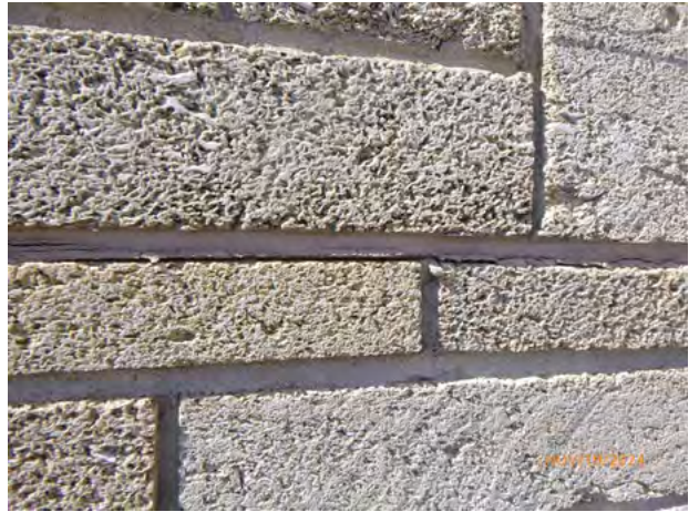
341-89 Stone_Joints Sealant Failed 2024-5.jpg
