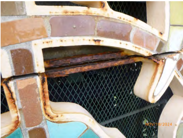
13-173 ArchMetal_Corrosion Pitted 2024-2.jpg
