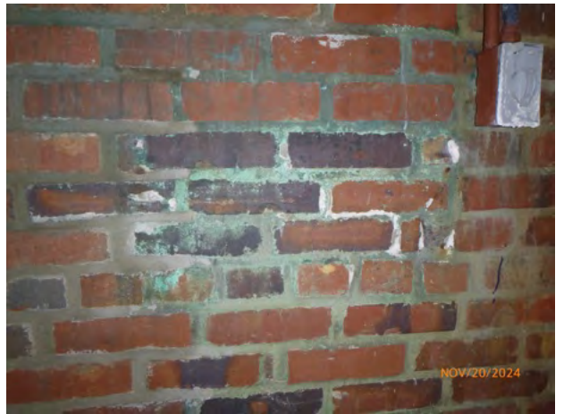
867-140 Brick_SoilStain Copper 2024-2.jpg
