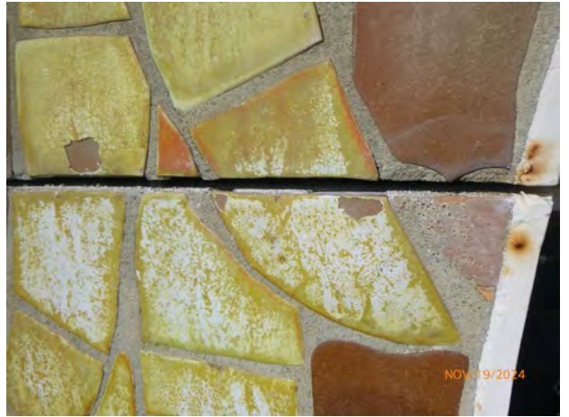
313-164 TerraCotta_SurfLoss Glaze loss 2024-3.jpg
