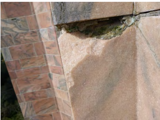
334-135 Stone_Spall Removed 2024-1.jpg
