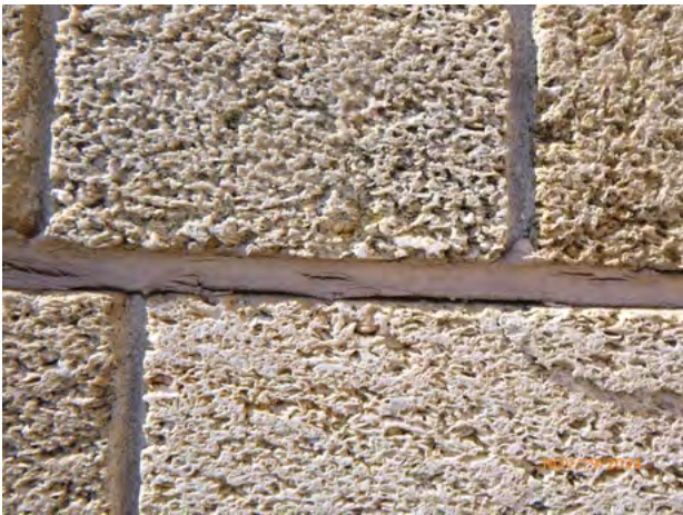
340-68 Stone_Joints Sealant Failed 2024-2.jpg
