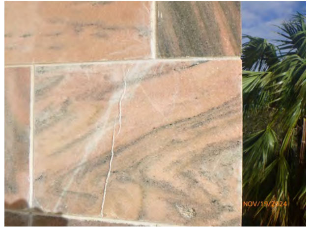
357-45 Stone_SoilStain Leached Salts 2024-5.jpg
