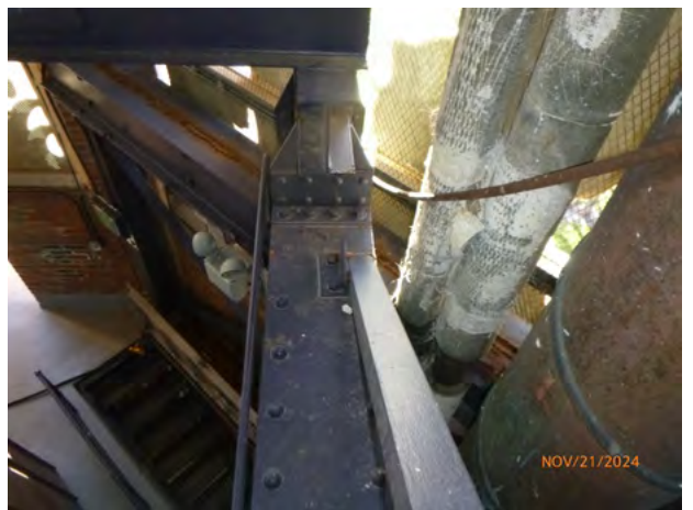
763-147 ArchMetal_Coating Coating Failed 2024-6.jpg
