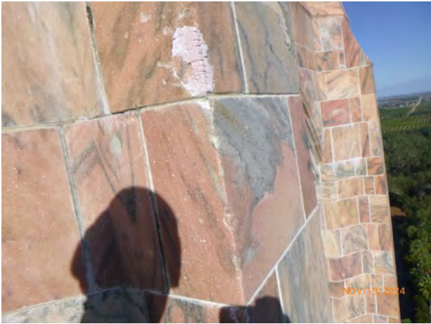
342-182 Stone_Repair Patch Failed 2024-3.jpg
