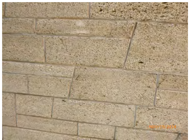
336-13 Stone_Crack System units and joints 2024-1.jpg
