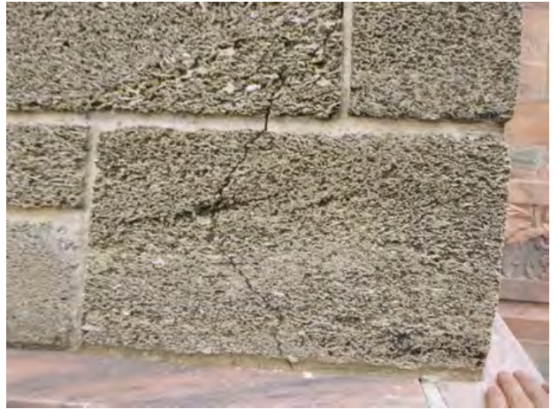
166-33 Stone_Crack System units and joints 2024-3.jpg
