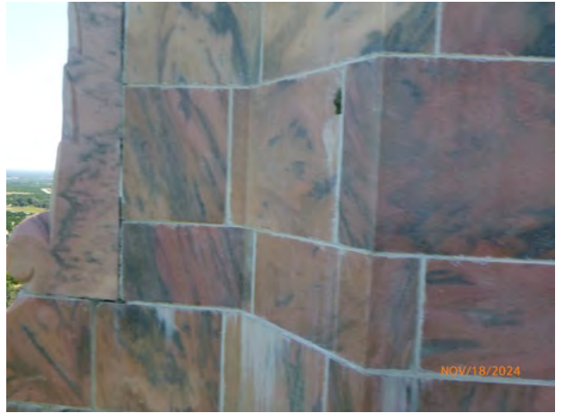
31-158 Stone_Joints Mortar Failed 2024-2.jpg
