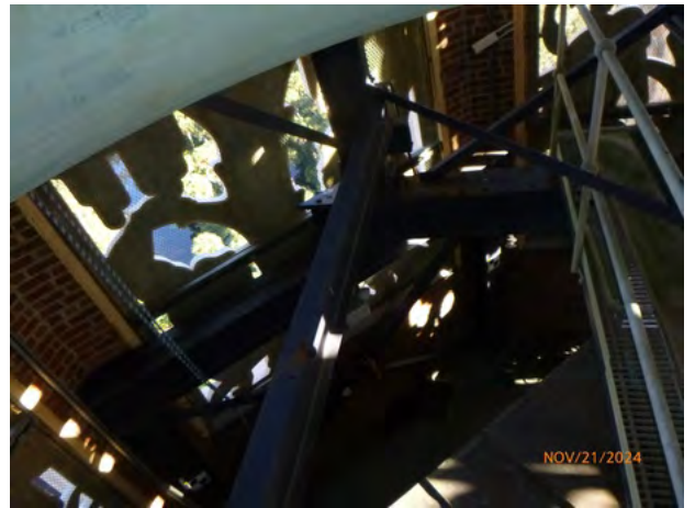
663-148 ArchMetal_Coating Coating Failed 2024-4.jpg
