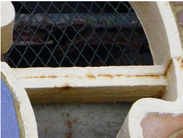
86-149 ArchMetal_Corrosion Surface 2024-2.jpg
