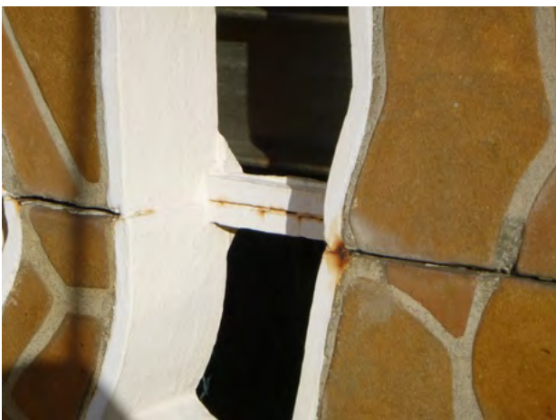
287-133 ArchMetal_Corrosion Surface 2024-3.jpg
