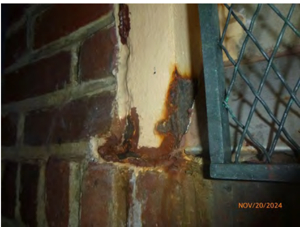
541-144 ArchMetal_Corrosion Pitted 2024-2.jpg
