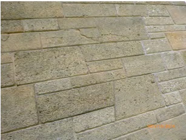
364-13 Stone_Crack System units and joints 2024-2.jpg
