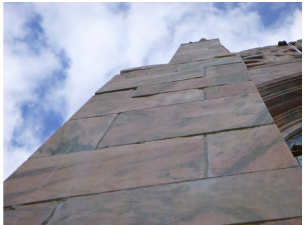
43-154 Stone_Joints Mortar Failed 2024-2.jpg
