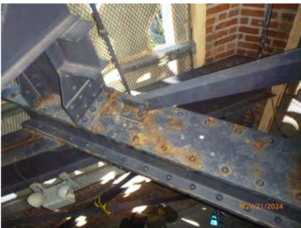
844-147 ArchMetal_Corrosion Fastener rusted 2024-6.jpg
