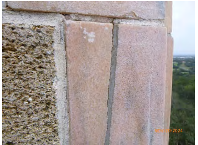
67-108 Stone_Crack Repair failed 2024-3.jpg
