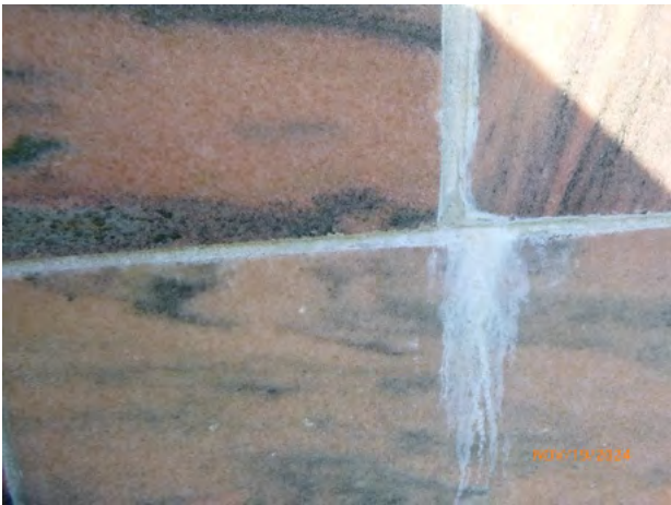
343-154 Stone_SoilStain Leached Salts 2024-3.jpg
