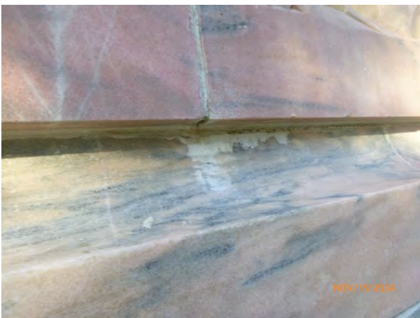
345-28 Stone_SoilStain Leached Salts 2024-1.jpg
