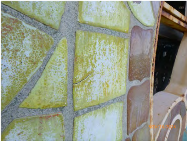
13-163 TerraCotta_Crack Single unit 2024-2.jpg
