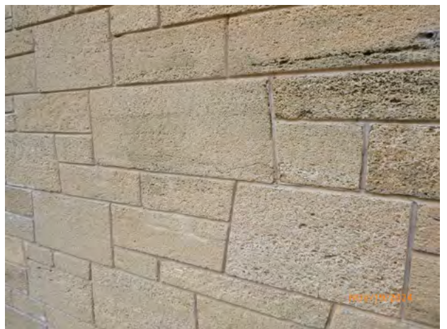
237-15 Stone_Crack Single unit 2024-1.jpg
