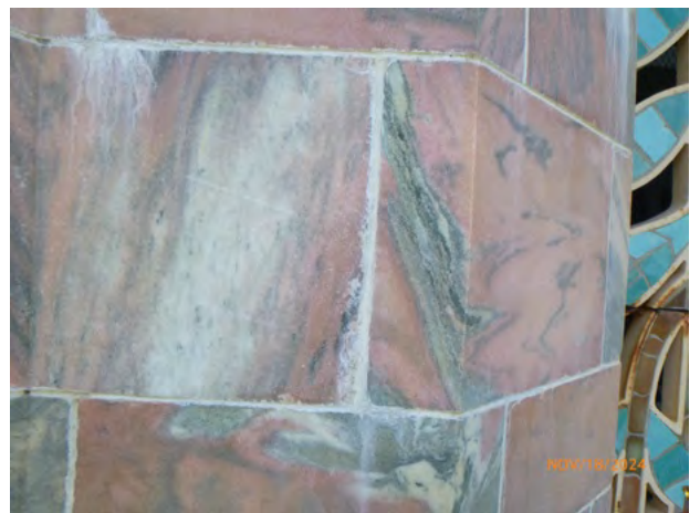
35-164 Stone_SurfLoss Chipped 2024-1.jpg
