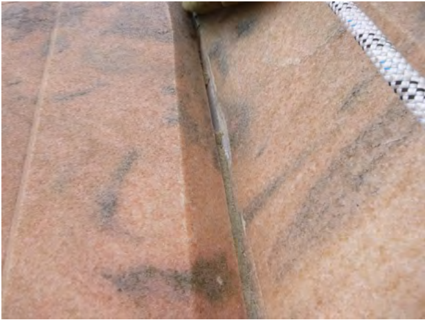
235-194 Stone_Joints Mortar Failed 2024-1.jpg
