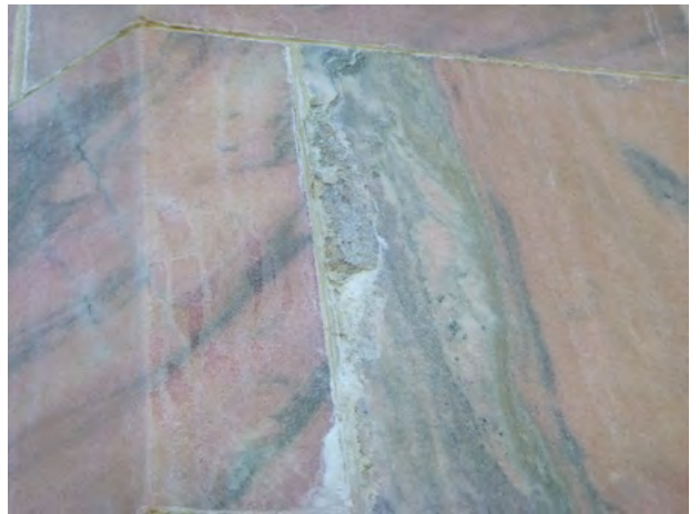
42-147 Stone_SurfLoss Chipped 2024-1.jpg
