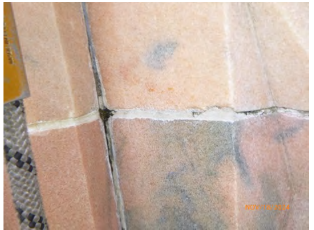
38-188 Stone_Joints Mortar Failed 2024-4.jpg
