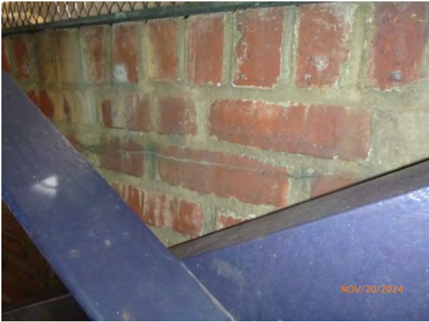
751-143 Brick_Crack System units and joints 2024-2.jpg
