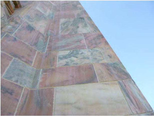
42-128 Stone_SoilStain Efflorescence 2024-1.jpg
