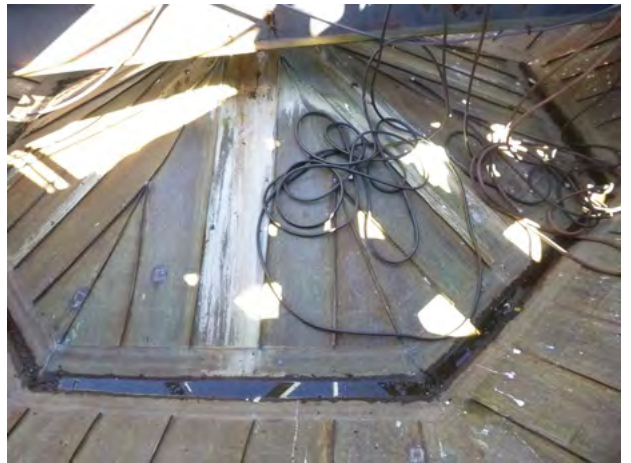
640-182 SheetMetal_Note Photo-active leak 2024-1.jpg
