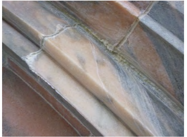
140-178 Stone_SoilStain Leached Salts 2024-2.jpg
