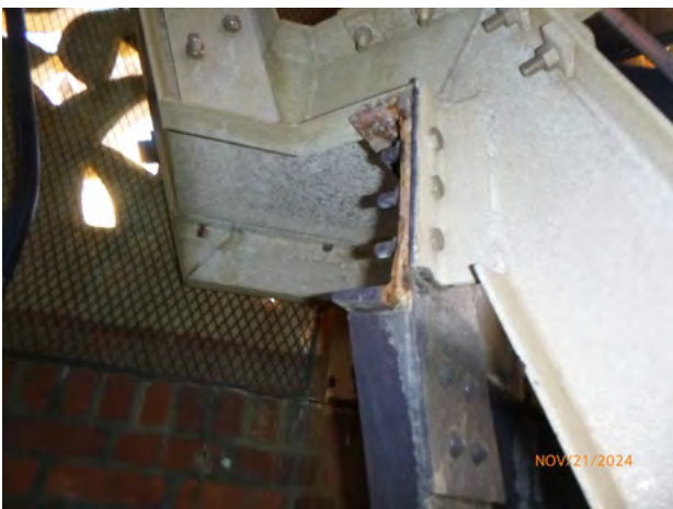
846-142 ArchMetal_Coating Coating Failed 2024-3.jpg
