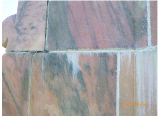
34-157 Stone_SoilStain Leached Salts 2024-4.jpg
