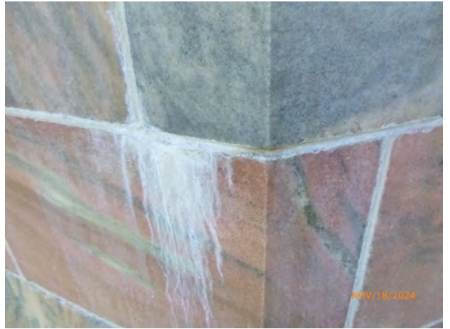
33-150 Stone_SoilStain Leached Salts 2024-3.jpg
