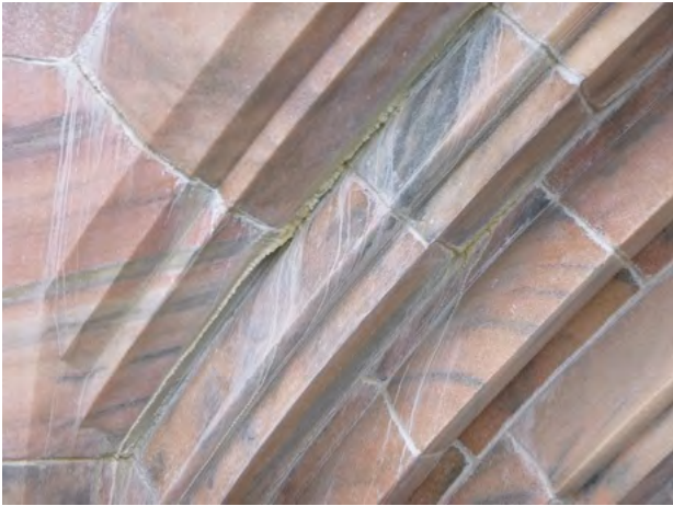
85-179 Stone_SoilStain Leached Salts 2024-1.jpg
