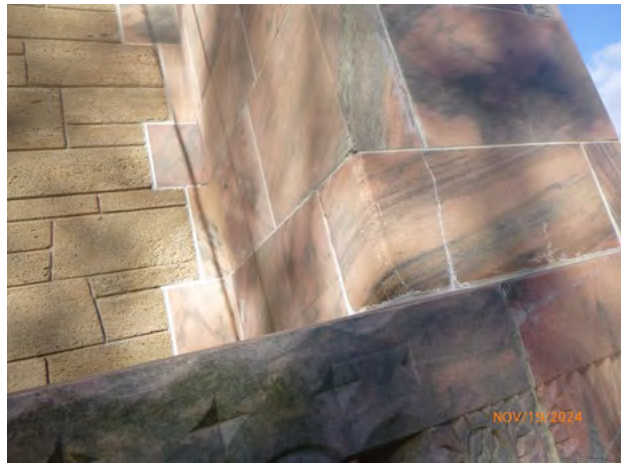
356-32 Stone_Spall Missing 2024-3.jpg
