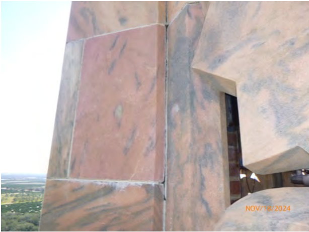
36-185 Stone_Joints Mortar Failed 2024-5.jpg
