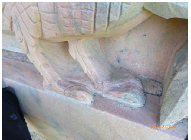
361-138 Stone_Crack Single unit 2024-3.jpg
