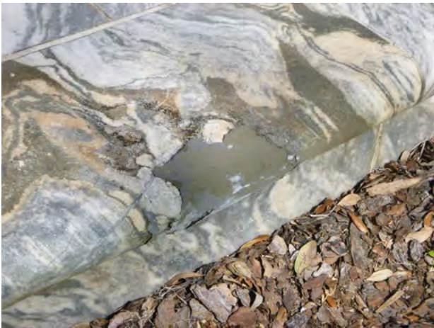
243-1 Stone_Repair Patch Failed 2024-1.jpg
