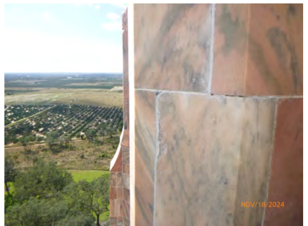
33-188 Stone_Spall Missing 2024-2.jpg
