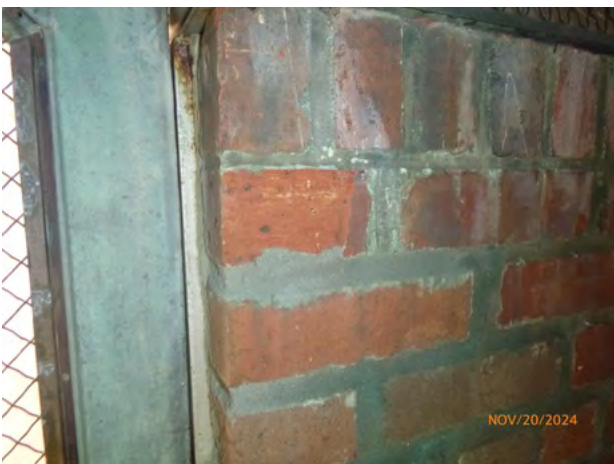
639-143 Brick_Spall Missing 2024-1.jpg
