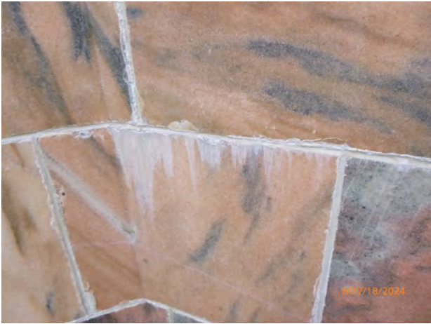
350-182 Stone_SoilStain Leached Salts 2024-3.jpg
