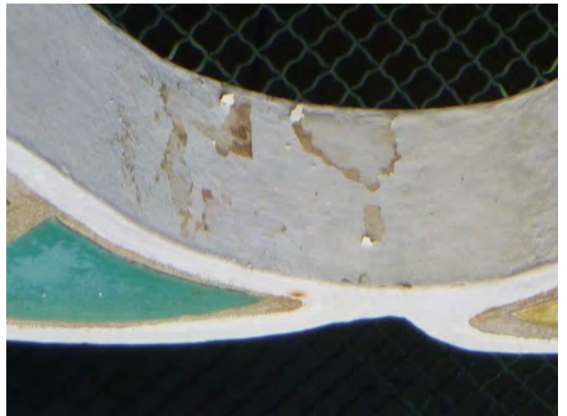
212-151 ArchMetal_Coating Coating Failed 2024-1.jpg
