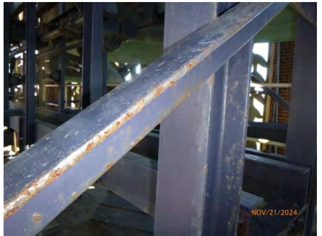
560-148 ArchMetal_Corrosion Surface 2024-2.jpg
