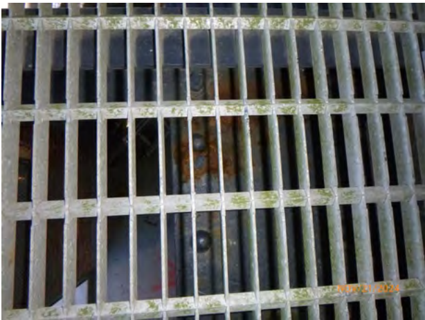
763-147 ArchMetal_Coating Coating Failed 2024-3.jpg
