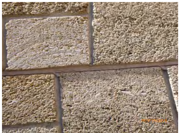
340-53 Stone_Joints Sealant Failed 2024-3.jpg
