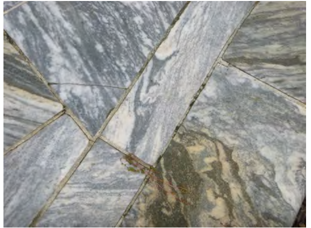
355-1 Stone_Joints Mortar Failed 2024-2.jpg
