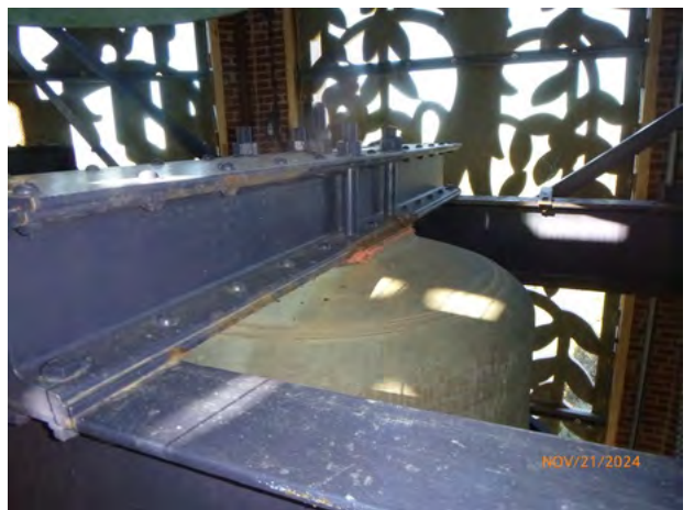
555-160 ArchMetal_Coating Coating Failed 2024-3.jpg
