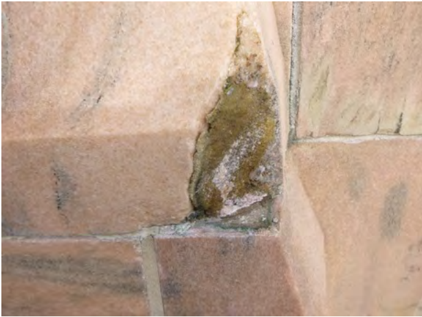
164-142 Stone_Spall Removed 2024-1.jpg
