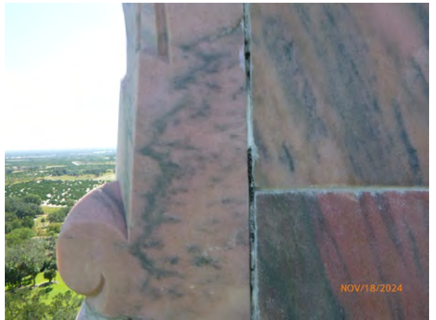
31-158 Stone_Joints Mortar Failed 2024-4.jpg
