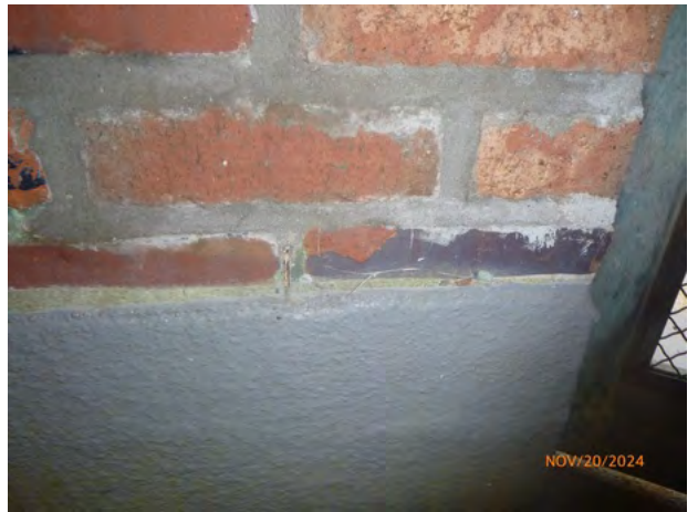
533-139 Brick_Spall Missing 2024-1.jpg
