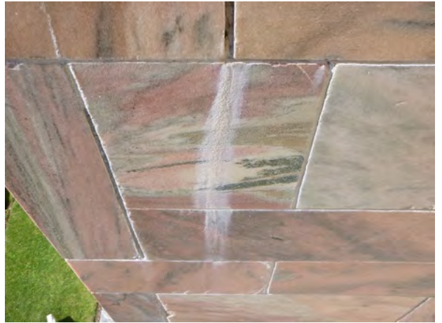
330-38 Stone_SoilStain Leached Salts 2024-1.jpg
