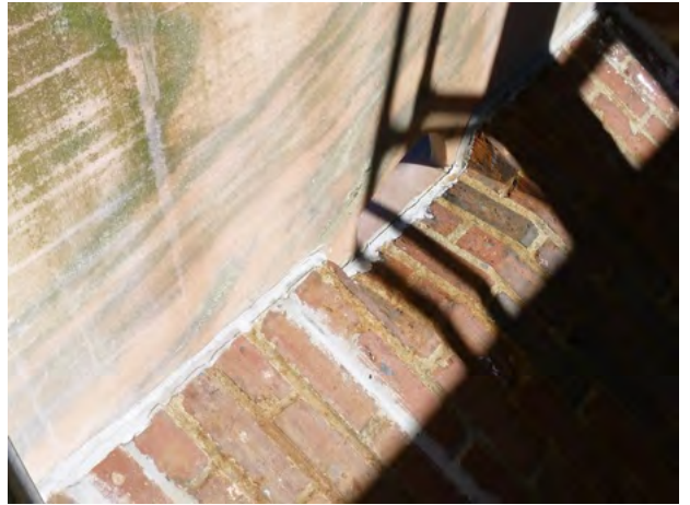
543-185 Brick_Joints Sealant Failed 2024-2.jpg
