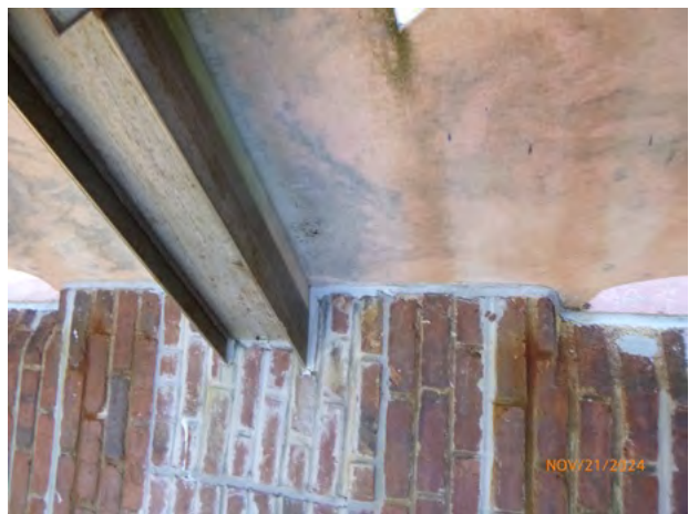
860-184 Brick_Joints Sealant Failed 2024-3.jpg
