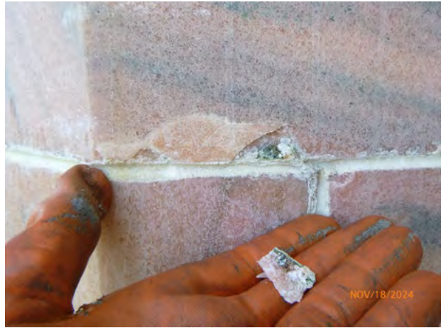
36-162 Stone_SurfLoss Chipped 2024-1.jpg
