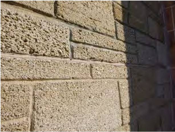
251-81 Stone_Joints Sealant Failed 2024-1.jpg
