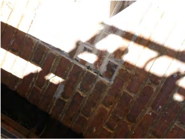
535-185 Brick_Joints Sealant Failed 2024-2.jpg
