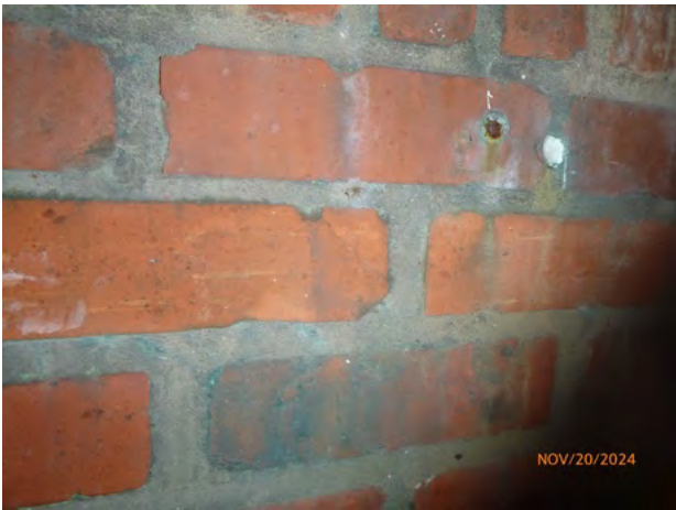
559-143 Brick_Crack Single unit 2024-1.jpg
