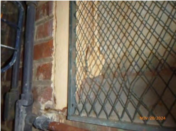
861-143 ArchMetal_Corrosion Pitted 2024-1.jpg
