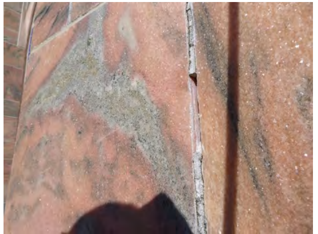
257-166 Stone_Joints Mortar Failed 2024-2.jpg
