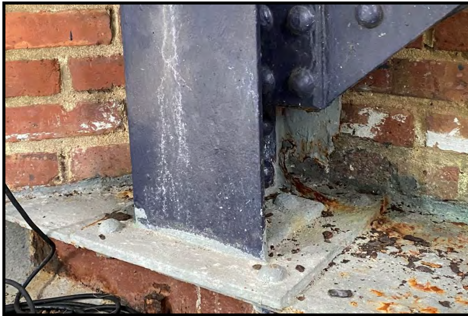
Figure 27 Section loss at base of bell tower column
