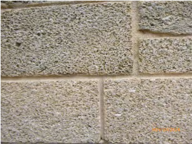
61-71 Stone_Joints Sealant Failed 2024-2.jpg
