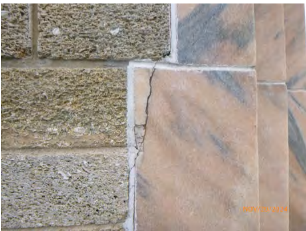
66-132 Stone_Crack System units and joints 2024-6.jpg
