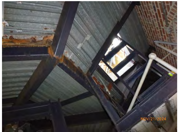
848-180 ArchMetal_Corrosion Perforated 2024-4.jpg
