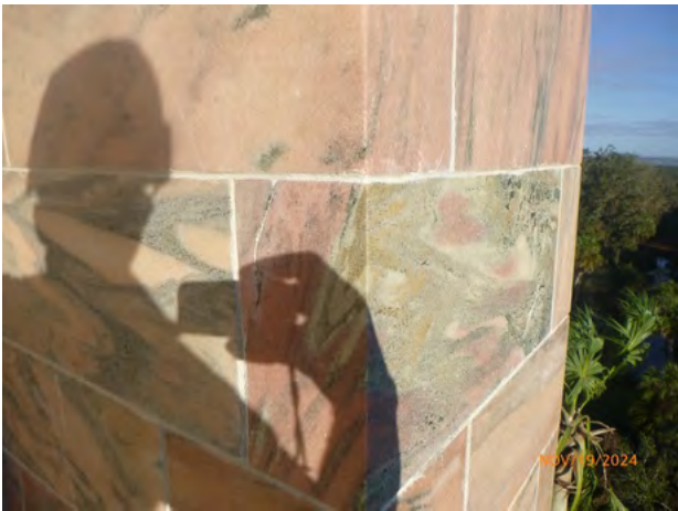
355-78 Stone_Crack Single unit 2024-4.jpg
