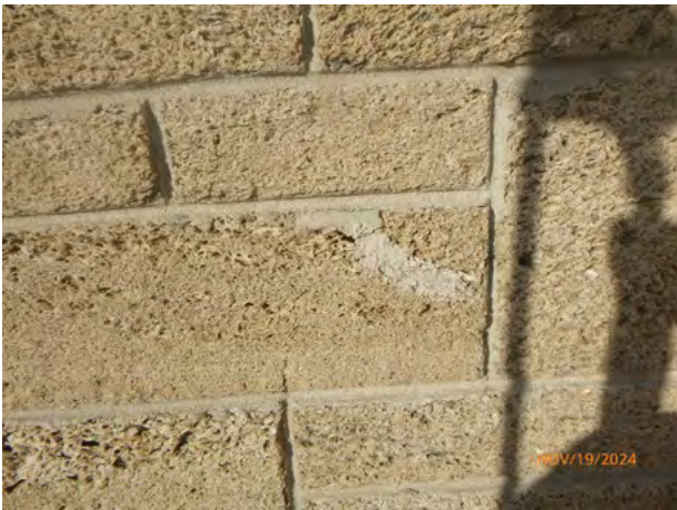
354-71 Stone_Repair Patch Failed 2024-2.jpg
