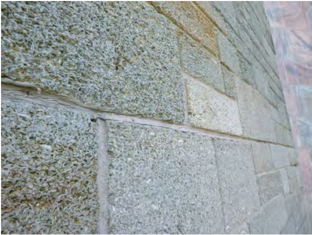
37-71 Stone_Joints Sealant Failed 2024-1.jpg
