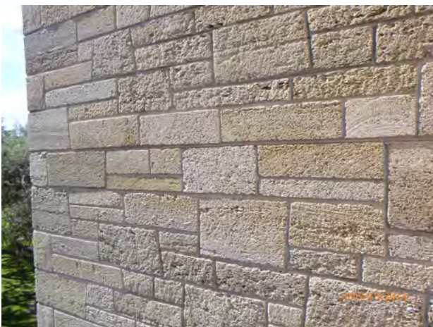
340-53 Stone_Joints Sealant Failed 2024-2.jpg
