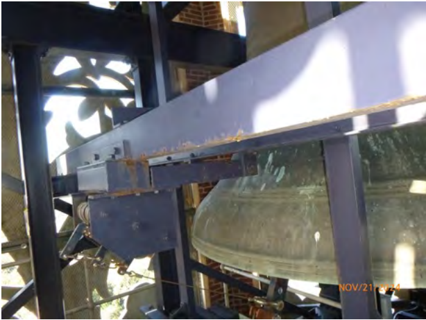
742-150 ArchMetal_Coating Coating Failed 2024-6.jpg
