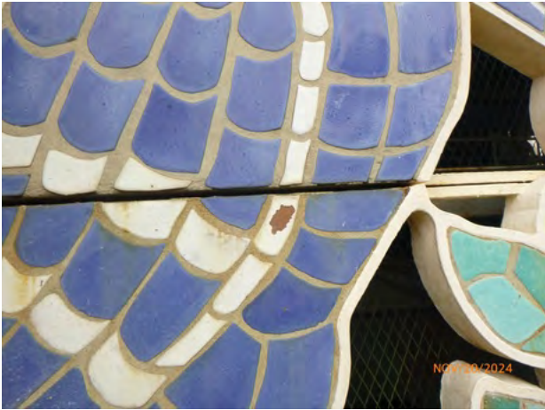
111-149 TerraCotta_SurfLoss Glaze loss 2024-1.jpg
