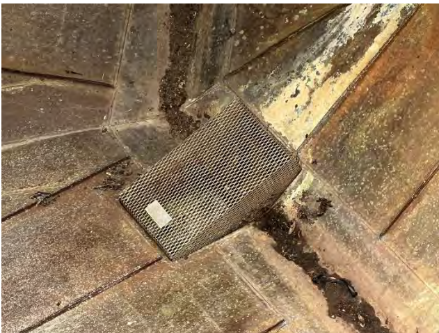
6 Single upper roof drain
