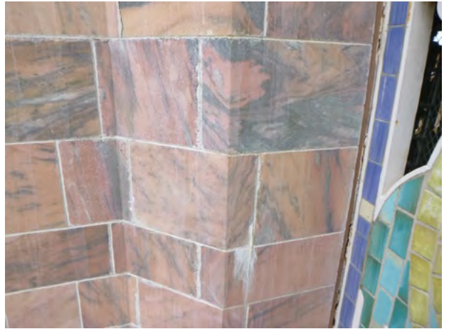
80-162 Stone_SoilStain Leached Salts 2024-2.jpg
