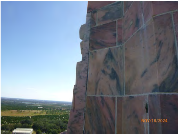
31-158 Stone_Joints Mortar Failed 2024-3.jpg
