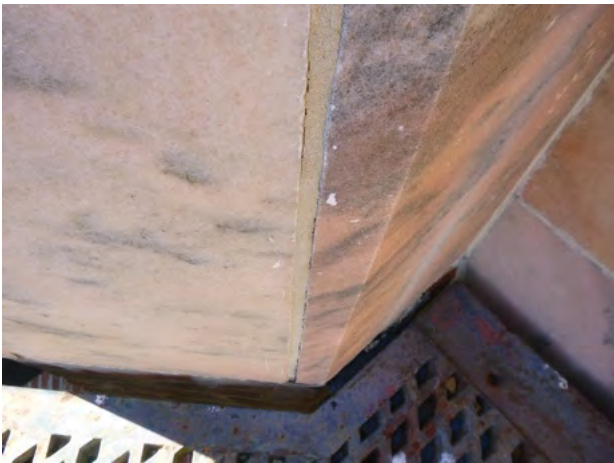
643-196 Stone_Joints Mortar Failed 2024-3.jpg
