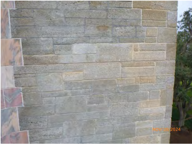
61-59 Stone_Joints Sealant Failed 2024-3.jpg
