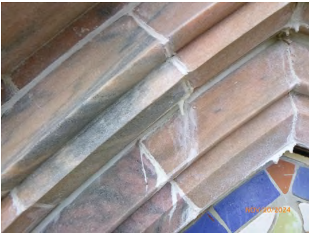
138-179 Stone_SoilStain Leached Salts 2024-6.jpg
