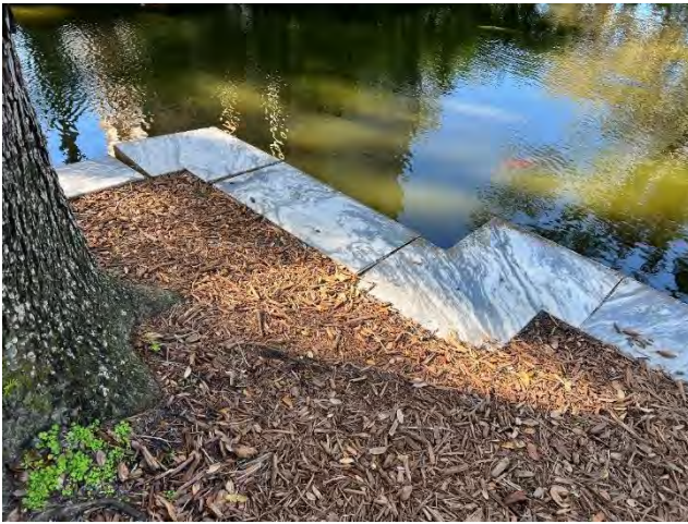
24 Moat edge stones out of plumb.
