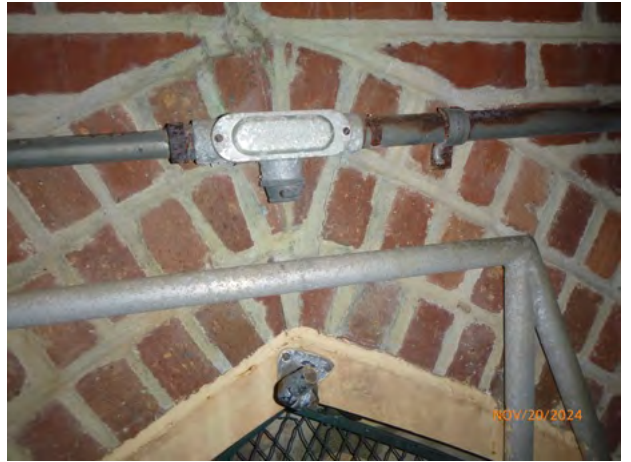
547-178 Brick_Joints Mortar Failed 2024-1.jpg
