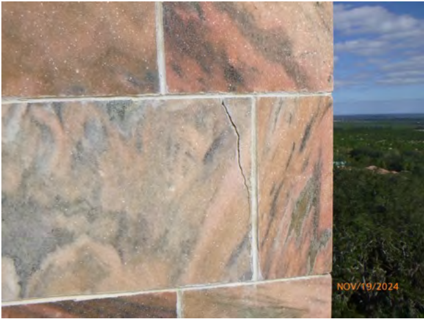
271-147 Stone_Crack Single unit 2024-1.jpg
