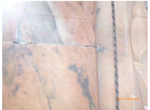
35-191 Stone_Joints Mortar Failed 2024-1.jpg
