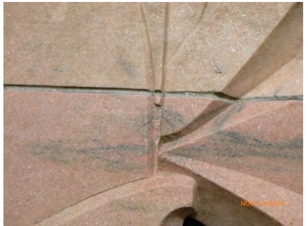
239-188 Stone_Spall Missing 2024-1.jpg
