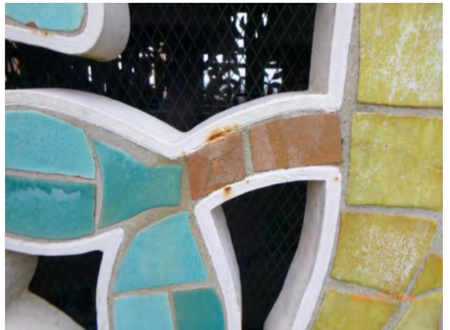
113-161 TerraCotta_SurfLoss Glaze loss 2024-1.jpg
