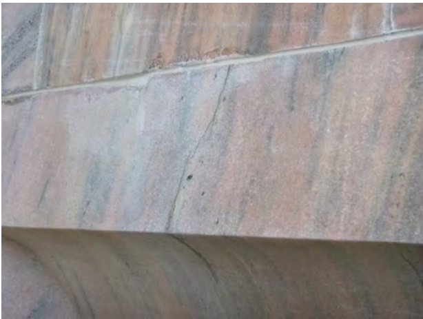
48-101 Stone_Crack Single unit 2024-1.jpg
