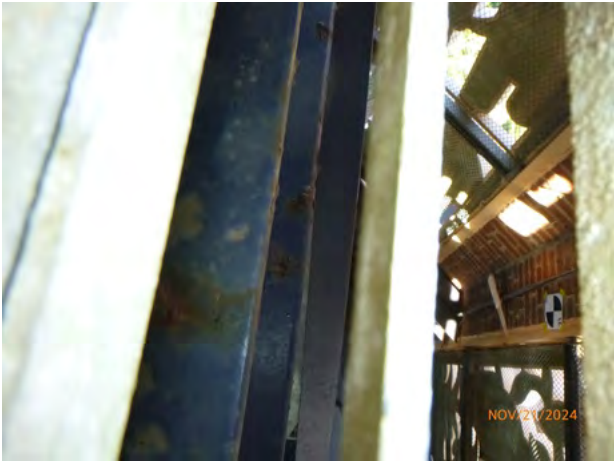
561-157 ArchMetal_Coating Coating Failed 2024-1.jpg
