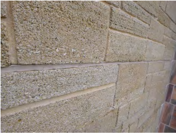
151-79 Stone_Joints Sealant Failed 2024-2.jpg
