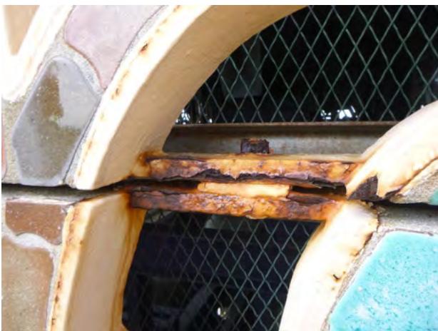
15-172 ArchMetal_Corrosion Pitted 2024-1.jpg
