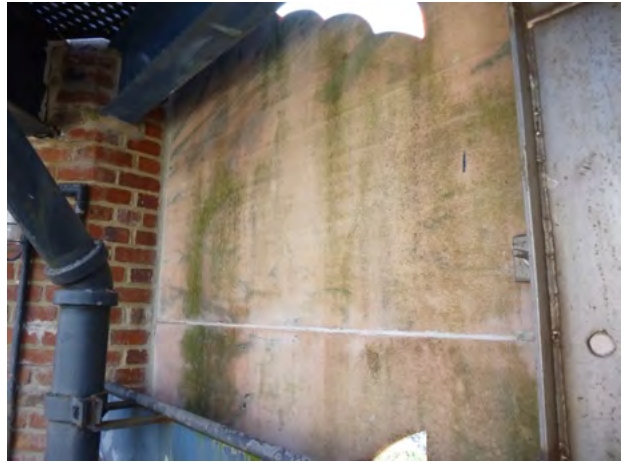
636-189 Brick_SoilStain Biological 2024-1.jpg
