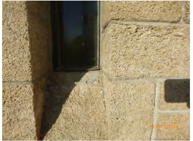
351-86 Stone_Joints Mortar Failed 2024-1.jpg
