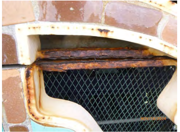
13-173 ArchMetal_Corrosion Pitted 2024-1.jpg
