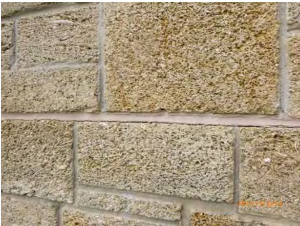
241-80 Stone_Joints Sealant Failed 2024-3.jpg
