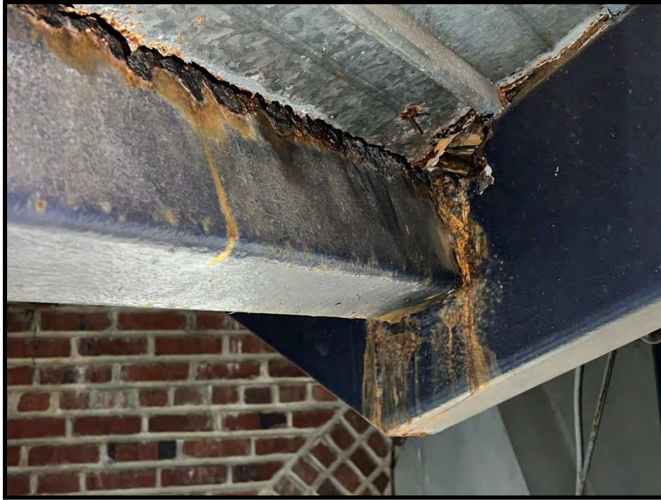
Figure 15 Corrosion of roof steel framing
