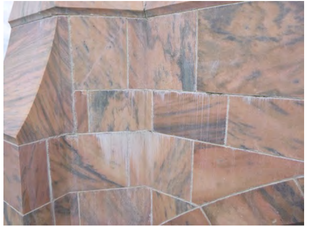
84-181 Stone_SoilStain Leached Salts 2024-1.jpg
