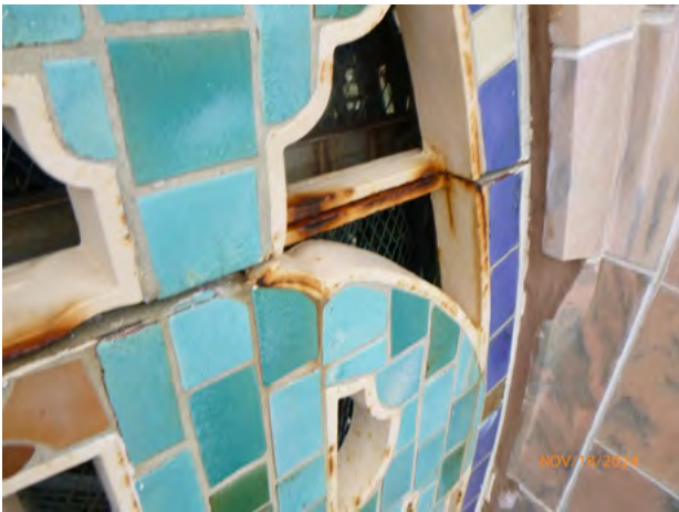
392-174 ArchMetal_Coating Coating Failed 2024-9.jpg
