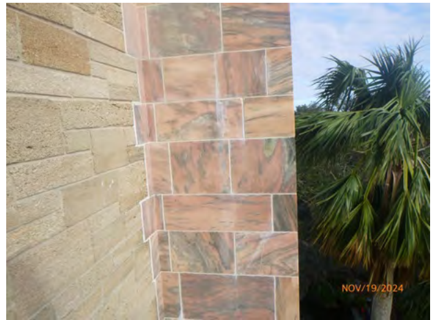
357-45 Stone_SoilStain Leached Salts 2024-1.jpg
