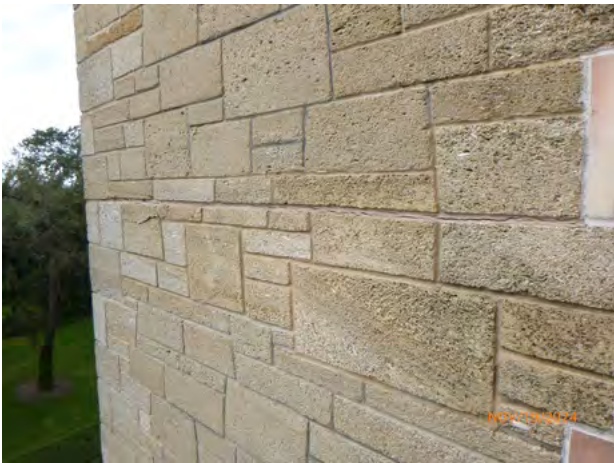
241-44 Stone_Joints Sealant Failed 2024-1.jpg
