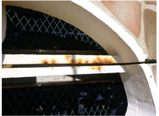
311-158 ArchMetal_Coating Coating Failed 2024-1.jpg
