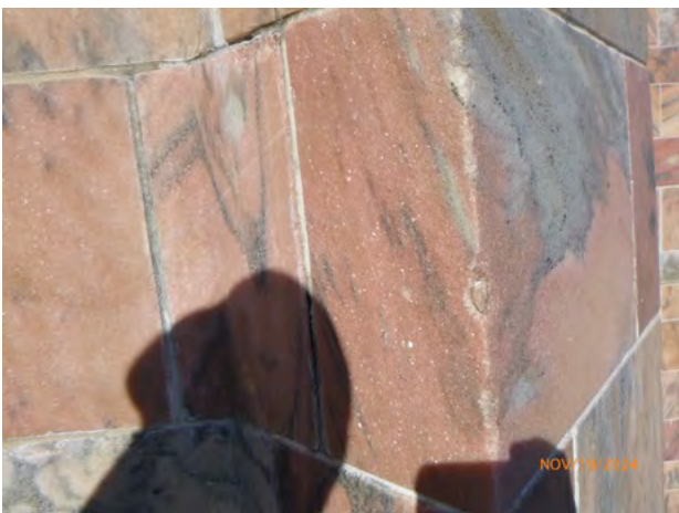
342-182 Stone_Repair Patch Failed 2024-1.jpg
