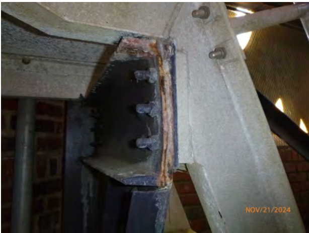
846-142 ArchMetal_Coating Coating Failed 2024-1.jpg
