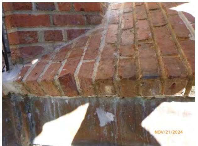
836-184 Brick_Spall Missing 2024-1.jpg
