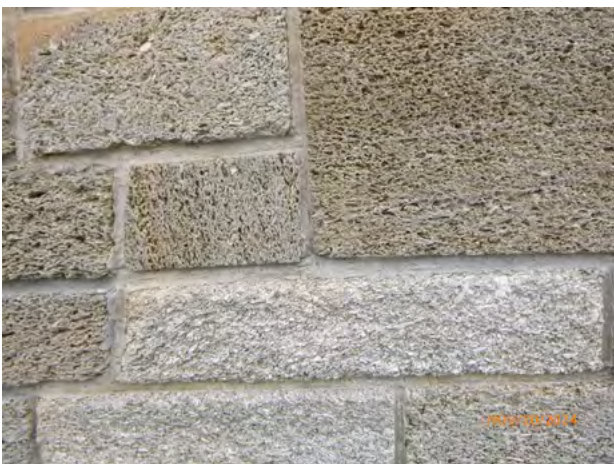
66-77 Stone_Crack Single unit 2024-4.jpg
