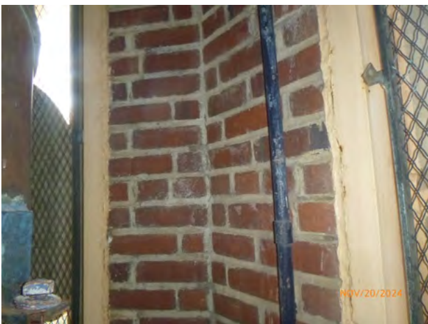
745-154 Brick_SoilStain Cementitious 2024-2.jpg
