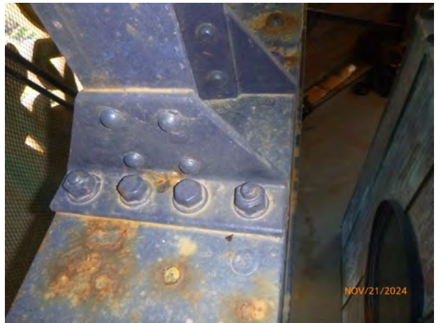
844-147 ArchMetal_Corrosion Fastener rusted 2024-5.jpg
