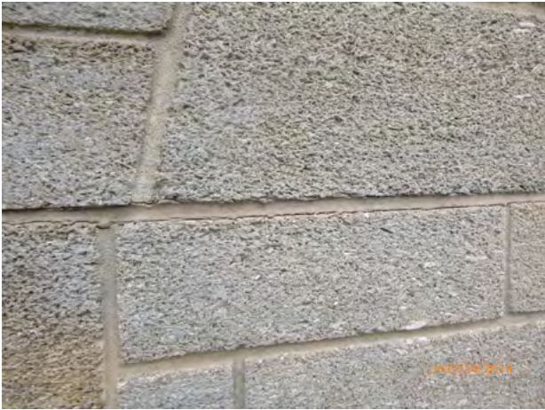
62-46 Stone_Joints Sealant Failed 2024-3.jpg
