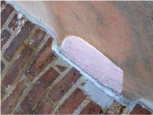
645-185 Brick_Joints Sealant Failed 2024-1.jpg
