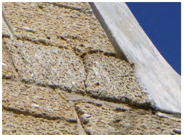
266-90 Stone_Crack System units and joints 2024-2.jpg
