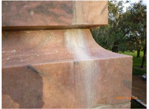
174-26 Stone_SoilStain Leached Salts 2024-2.jpg
