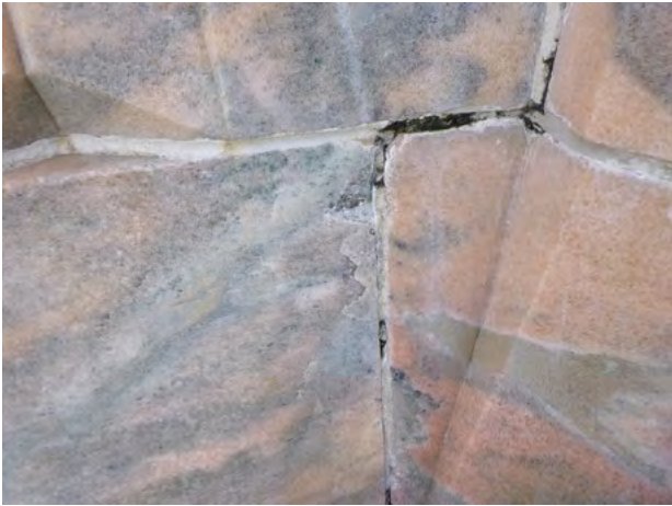
40-183 Stone_SurfLoss Chipped 2024-1.jpg
