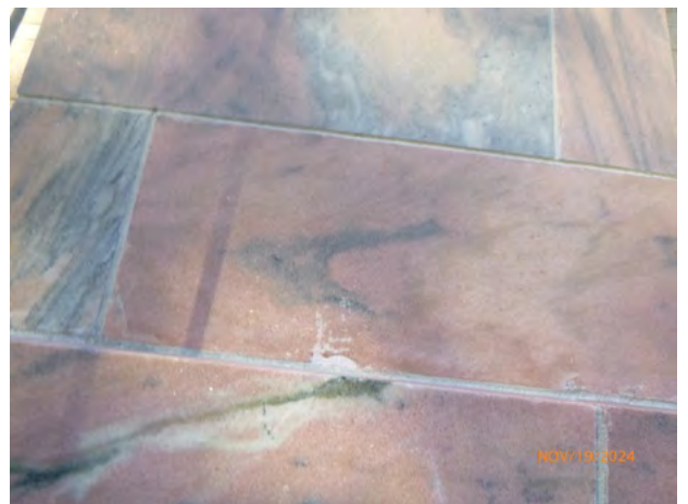
343-32 Stone_Repair Patch Failed 2024-2.jpg
