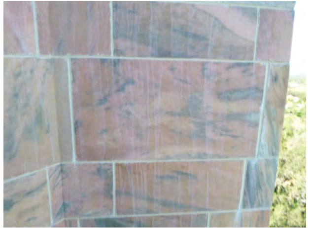
42-128 Stone_SoilStain Efflorescence 2024-2.jpg
