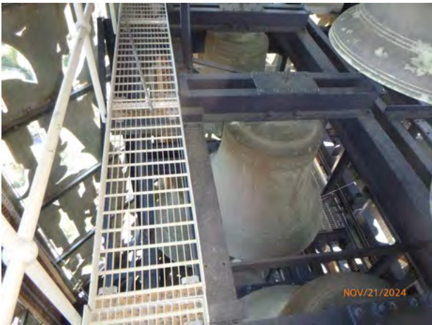
538-170 ArchMetal_Coating Coating Failed 2024-3.jpg
