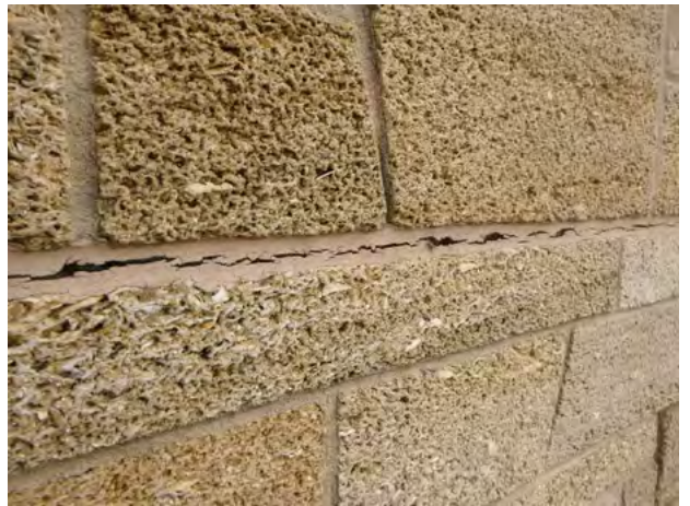
163-46 Stone_Joints Sealant Failed 2024-2.jpg
