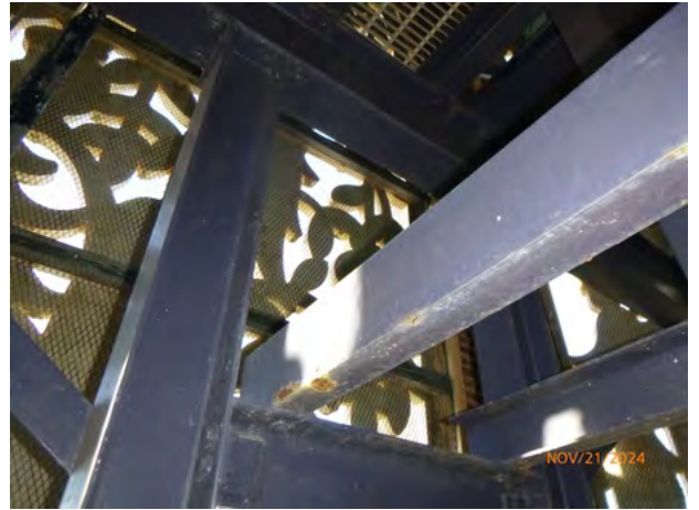
742-150 ArchMetal_Coating Coating Failed 2024-7.jpg
