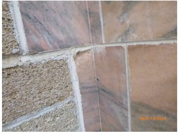
355-90 Stone_Spall Missing 2024-3.jpg
