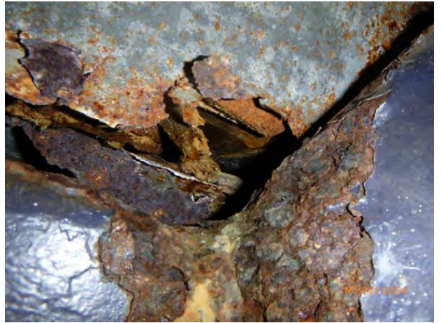
765-182 SheetMetal_Corrosion Perforated 2024-2.jpg
