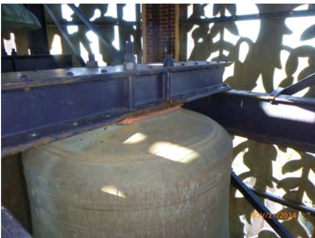
555-160 ArchMetal_Coating Coating Failed 2024-2.jpg
