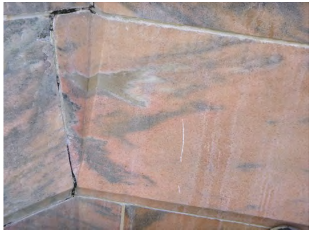
42-184 Stone_SoilStain Efflorescence 2024-1.jpg
