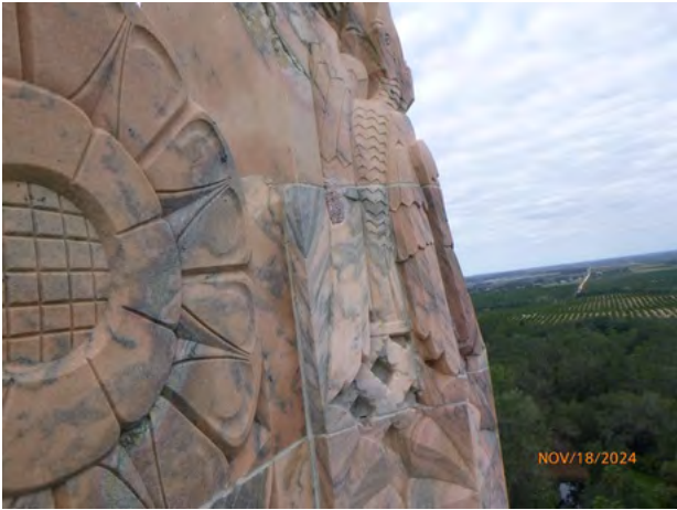
356-197 Stone_Spall Missing 2024-2.jpg
