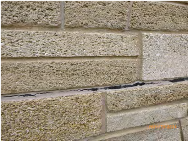
241-37 Stone_Joints Sealant Failed 2024-3.jpg
