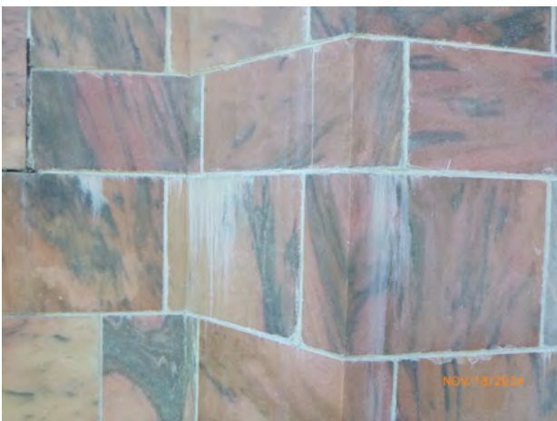
34-157 Stone_SoilStain Leached Salts 2024-1.jpg
