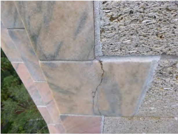
135-123 Stone_Crack System units and joints 2024-2.jpg
