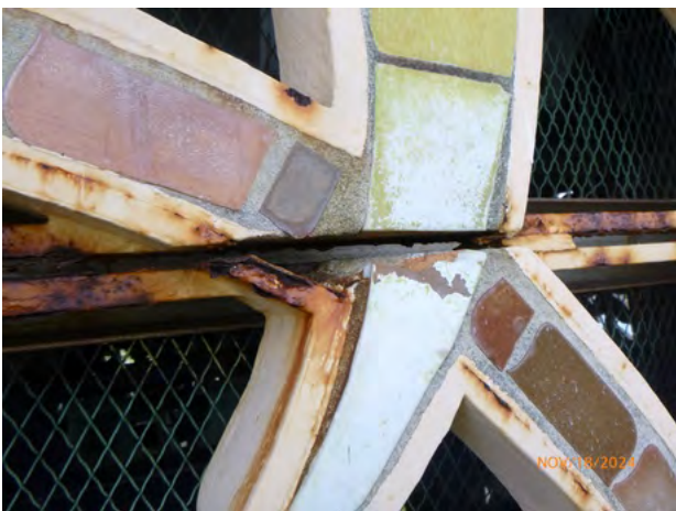
13-173 TerraCotta_Spall Missing 2024-1.jpg
