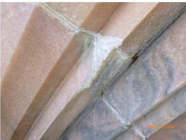
37-180 Stone_SoilStain Leached Salts 2024-2.jpg
