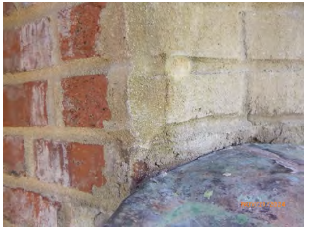
756-190 Brick_Repair Patch Failed 2024-2.jpg
