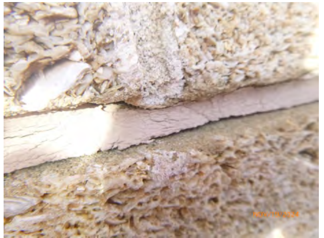
356-52 Stone_Joints Sealant Failed 2024-3.jpg
