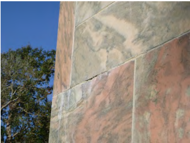
242-10 Stone_Joints Mortar Failed 2024-1.jpg
