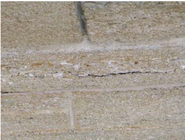
146-108 Stone_Crack System units and joints 2024-5.jpg
