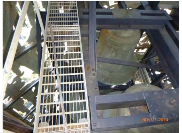
538-170 ArchMetal_Coating Coating Failed 2024-4.jpg
