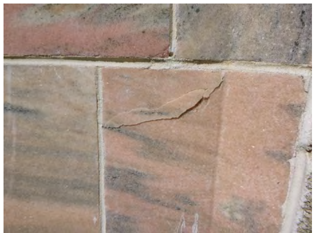
331-48 Stone_Spall Removed 2024-1.jpg
