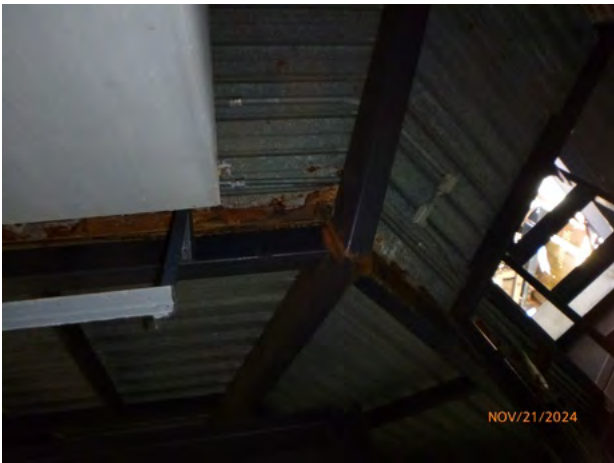
848-180 ArchMetal_Corrosion Perforated 2024-3.jpg
