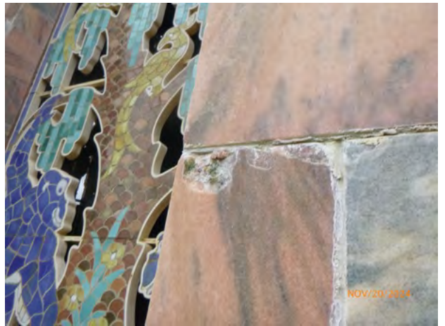
129-149 Stone_Spall Removed 2024-2.jpg
