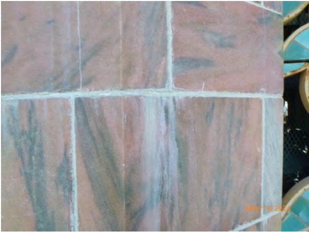
34-157 Stone_SoilStain Leached Salts 2024-3.jpg
