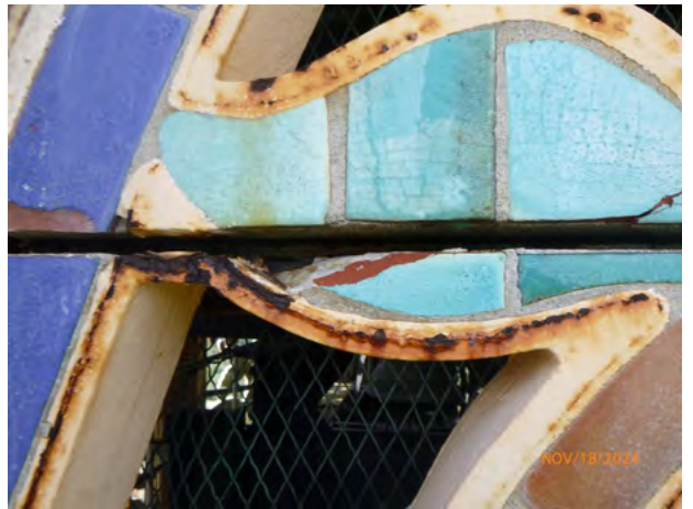
9-173 TerraCotta_Spall Missing 2024-1.jpg
