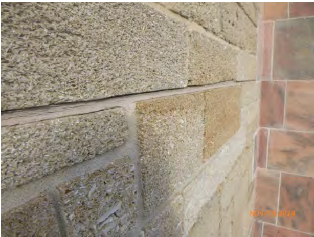
356-52 Stone_Joints Sealant Failed 2024-2.jpg
