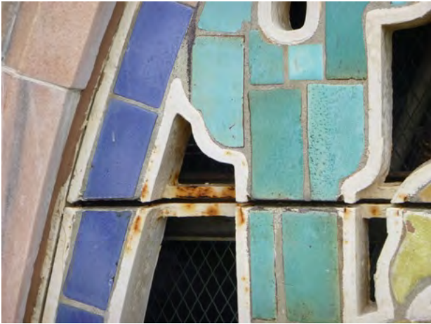
83-173 ArchMetal_Corrosion Pitted 2024-1.jpg
