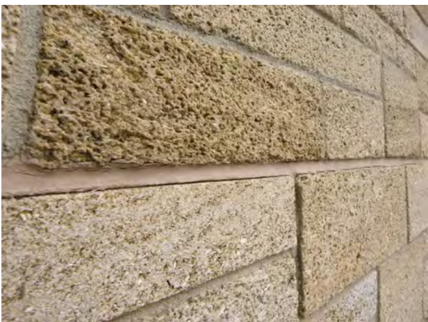
164-78 Stone_Joints Sealant Failed 2024-1.jpg
