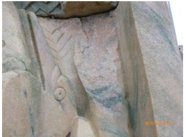
134-200 Stone_Spall Missing 2024-2.jpg
