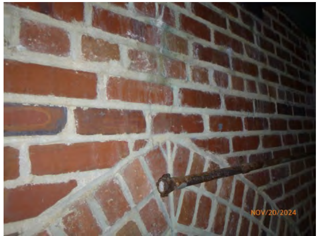
651-179 Brick_Crack System units and joints 2024-2.jpg
