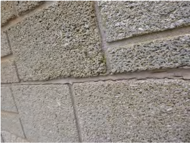
137-68 Stone_Joints Sealant Failed 2024-2.jpg
