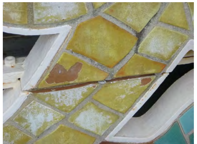
116-158 TerraCotta_SurfLoss Glaze loss 2024-1.jpg
