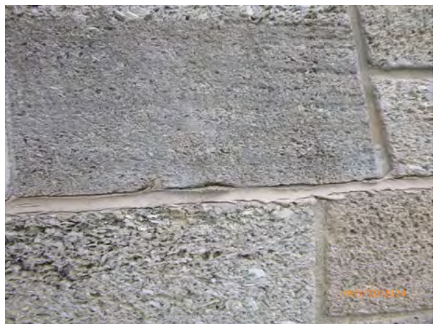
61-127 Stone_Joints Sealant Failed 2024-2.jpg
