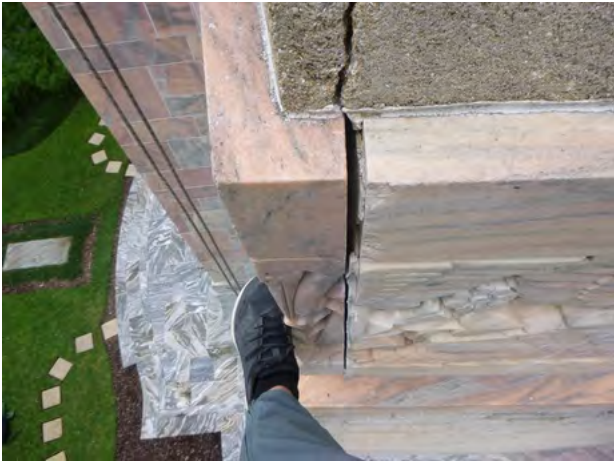
135-32 Stone_Crack System units and joints 2024-5.jpg
