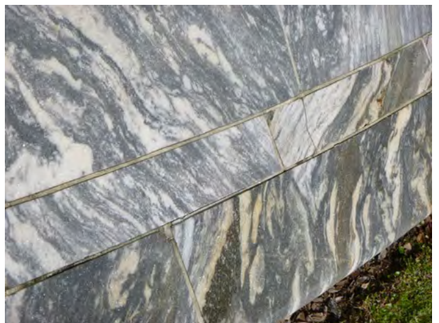
250-1 Stone_Joints Mortar Failed 2024-1.jpg
