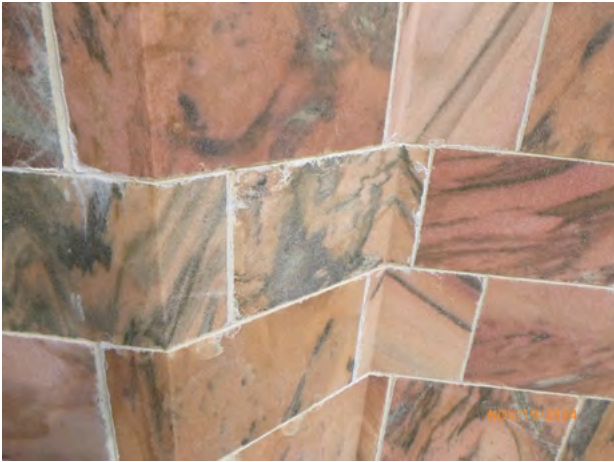
243-154 Stone_SurfLoss Chipped 2024-1.jpg
