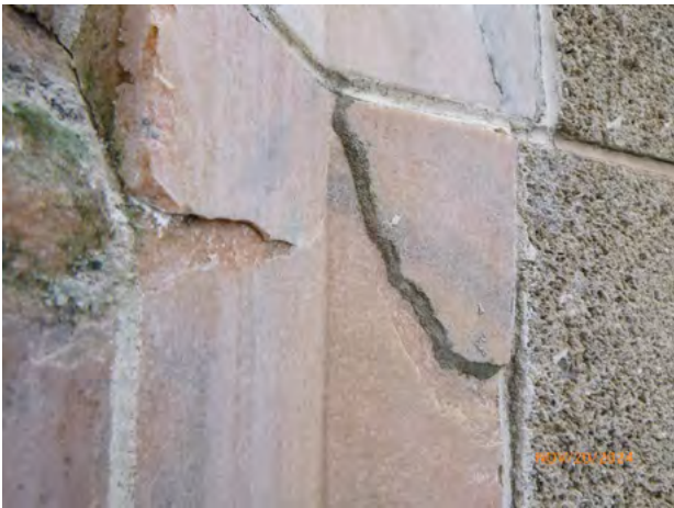
60-70 Stone_Crack Single unit 2024-2.jpg
