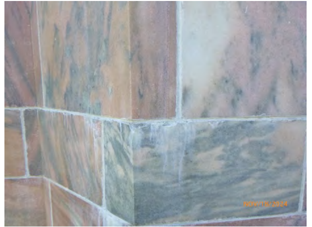
34-152 Stone_SurfLoss Chipped 2024-2.jpg
