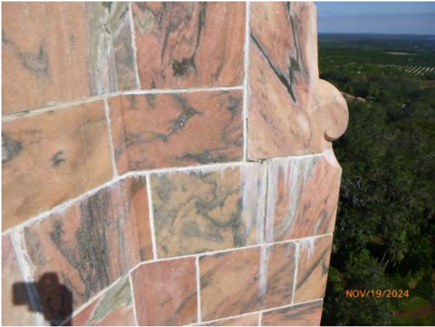
272-156 Stone_SoilStain Leached Salts 2024-1.jpg
