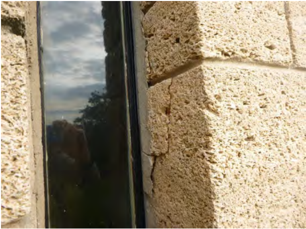
164-55 Stone_Spall Removed 2024-1.jpg
