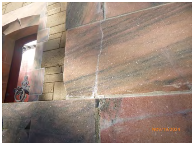
356-32 Stone_Crack Single unit 2024-1.jpg
