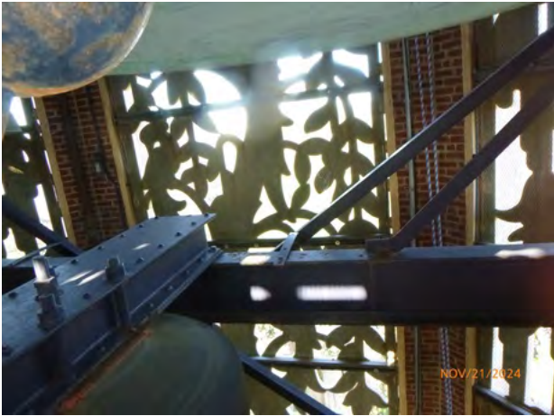
540-158 ArchMetal_Coating Coating Failed 2024-3.jpg
