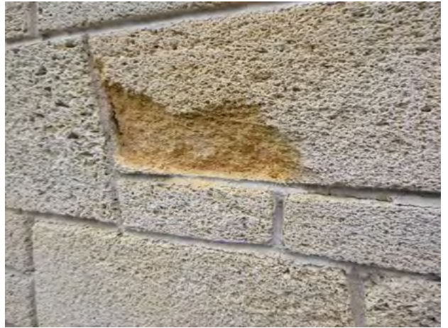
137-17 Stone_Spall Removed 2024-3.jpg
