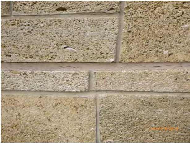
240-57 Stone_Joints Sealant Failed 2024-3.jpg
