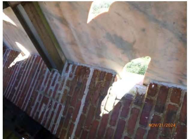
741-184 Brick_Joints Sealant Failed 2024-2.jpg
