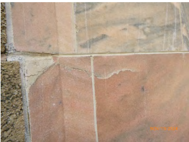
241-70 Stone_Crack System units and joints 2024-1.jpg
