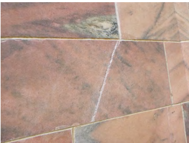
230-23 Stone_Crack Single unit 2024-1.jpg
