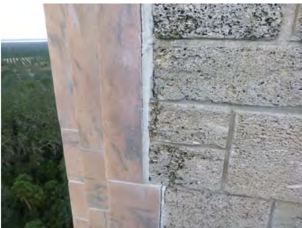
135-133 Stone_Joints Mortar Failed 2024-2.jpg
