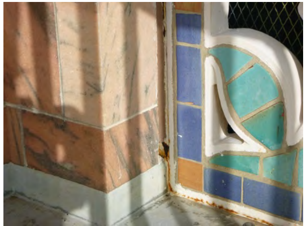
283-129 ArchMetal_Corrosion Pitted 2024-1.jpg
