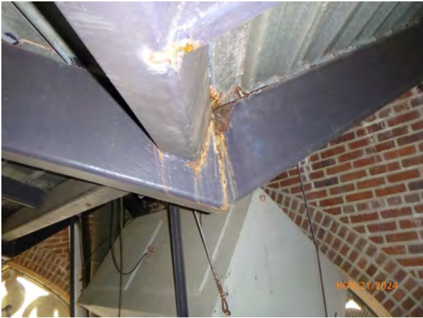
763-180 ArchMetal_Corrosion Surface 2024-1.jpg
