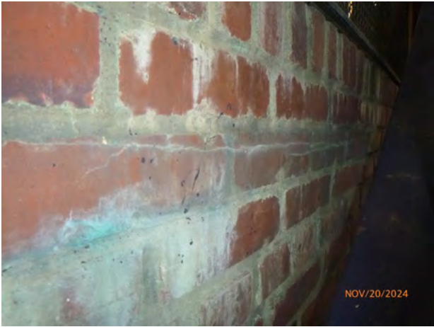
651-142 Brick_Crack System units and joints 2024-2.jpg
