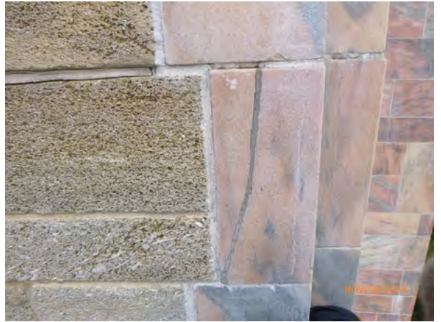
67-108 Stone_Crack Repair failed 2024-1.jpg
