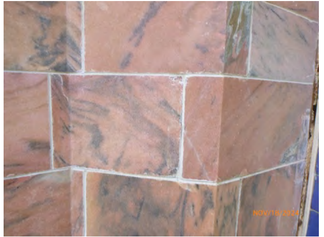
346-162 Stone_SurfLoss Chipped 2024-1.jpg
