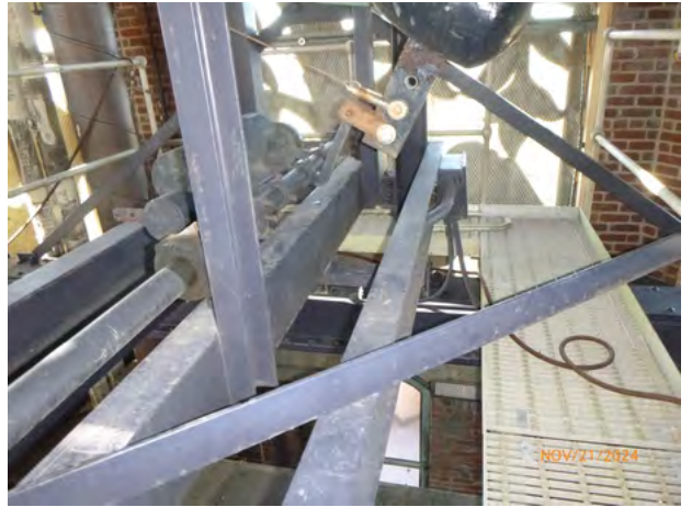
664-149 ArchMetal_Coating Coating Failed 2024-3.jpg
