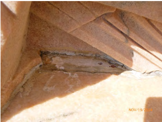
341-139 Stone_Joints Mortar Failed 2024-3.jpg
