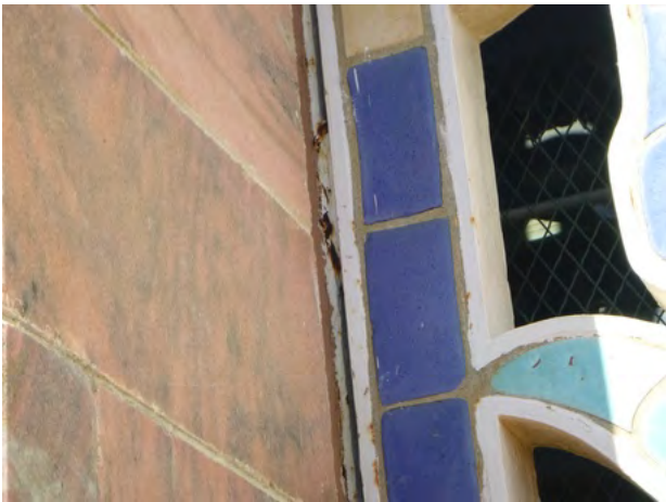
308-145 ArchMetal_Corrosion Pitted 2024-2.jpg
