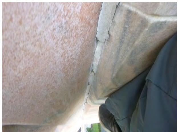
141-188 Stone_Joints Mortar Failed 2024-2.jpg
