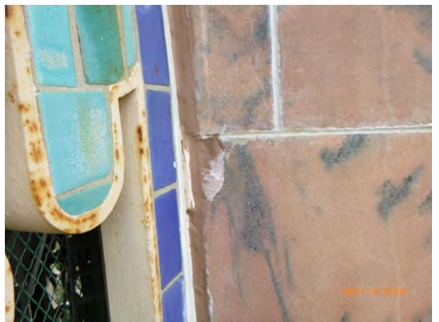
355-172 Stone_Repair Patch Failed 2024-1.jpg
