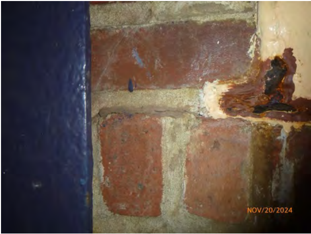
541-144 Brick_Crack Repair failed 2024-2.jpg
