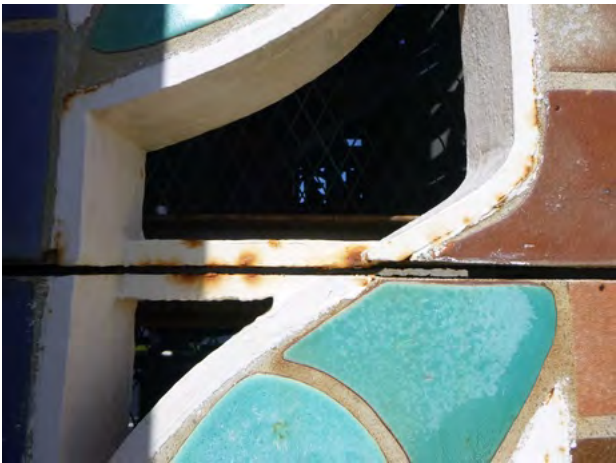
313-152 ArchMetal_Coating Coating Failed 2024-1.jpg
