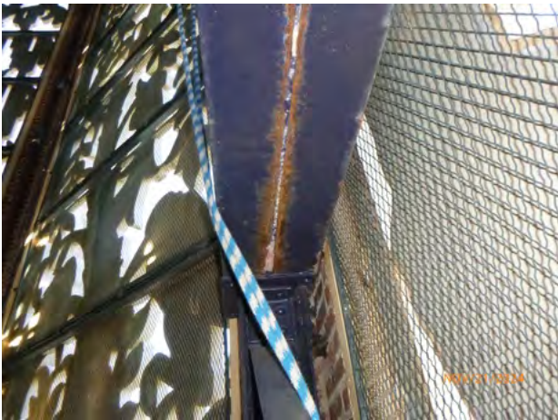
555-145 ArchMetal_Coating Coating Failed 2024-3.jpg
