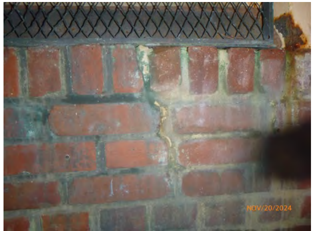
856-143 Brick_Repair Patch Failed 2024-1.jpg
