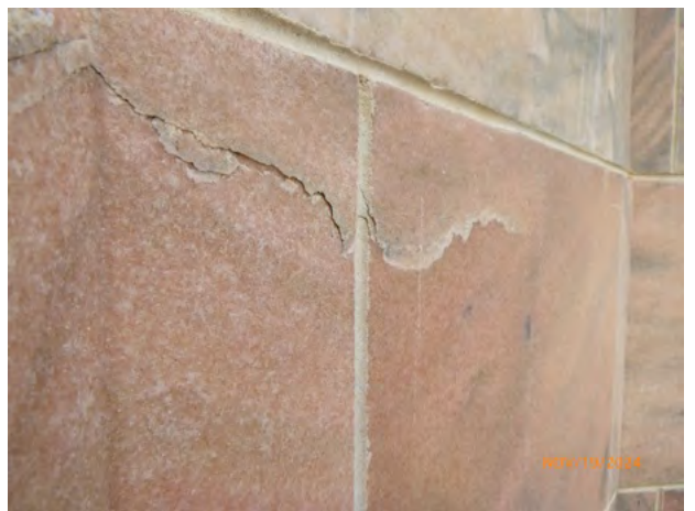
241-70 Stone_Crack System units and joints 2024-2.jpg
