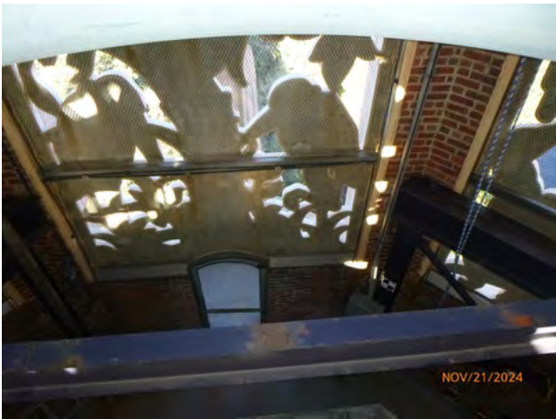
663-148 ArchMetal_Coating Coating Failed 2024-3.jpg
