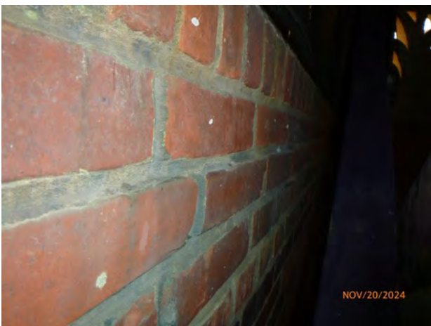
548-143 Brick_Joints Mortar Failed 2024-1.jpg
