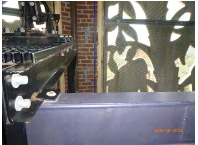
658-146 Brick_Unsecured Missing 2024-2.jpg
