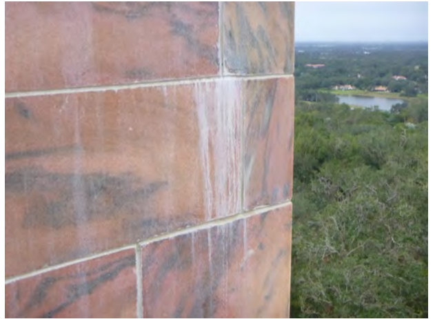
70-97 Stone_SoilStain Leached Salts 2024-1.jpg
