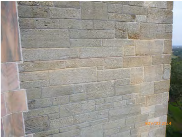
62-81 Stone_Joints Sealant Failed 2024-1.jpg
