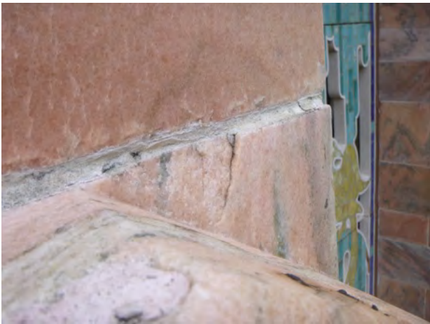
158-163 Stone_Spall Missing 2024-1.jpg
