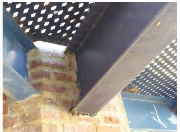
643-193 ArchMetal_Corrosion Surface 2024-2.jpg
