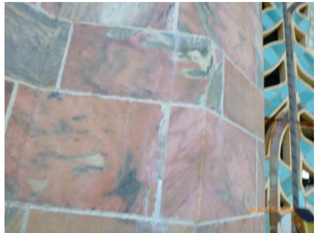
35-163 Stone_Spall Missing 2024-2.jpg
