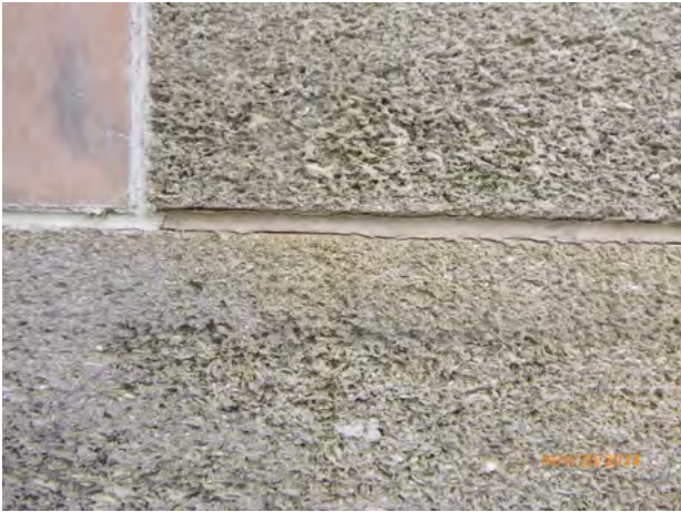
61-90 Stone_Joints Sealant Failed 2024-2.jpg
