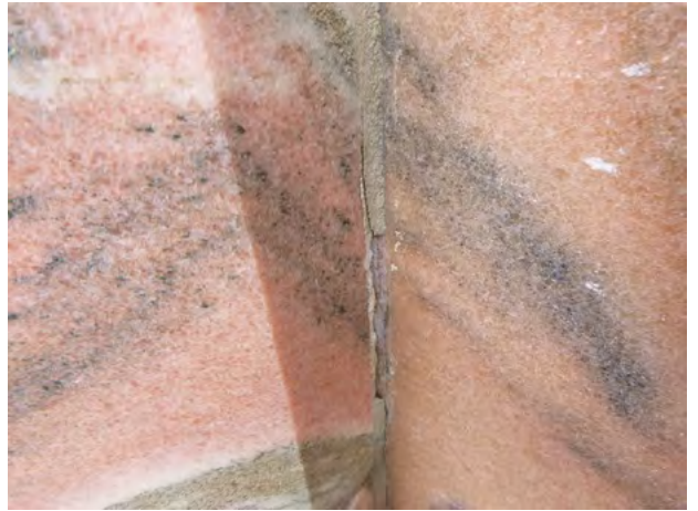
235-194 Stone_Joints Mortar Failed 2024-2.jpg
