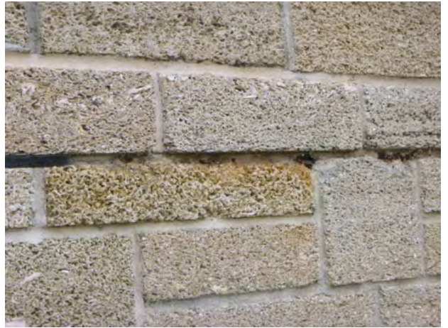
151-91 Stone_Spall Missing + Steel 2024-1.jpg
