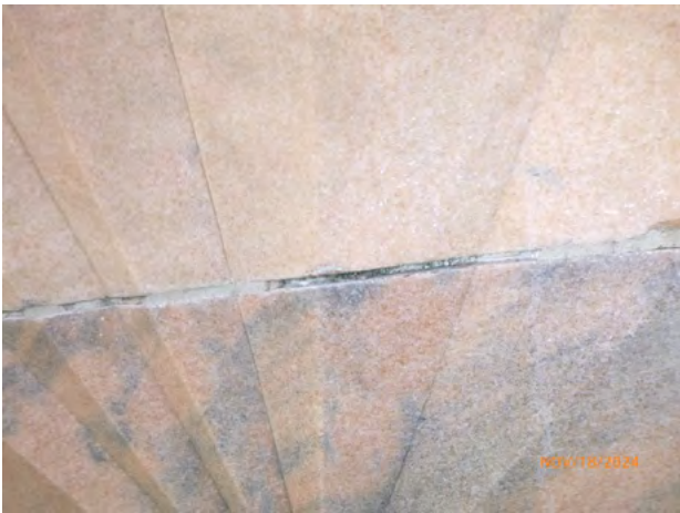
38-188 Stone_Joints Mortar Failed 2024-3.jpg
