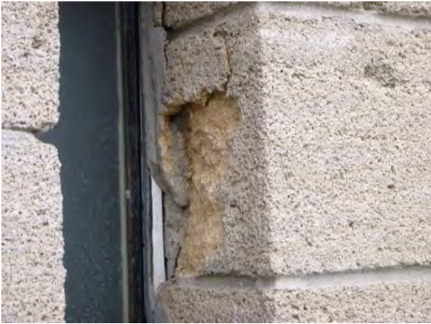
50-88 Stone_Spall Removed 2024-3.jpg
