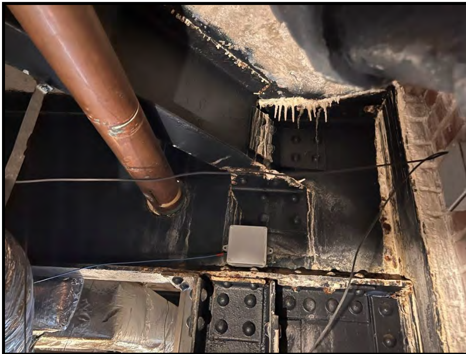
Figure 19 Efflorescence and stalactites forming below seventh level slab
