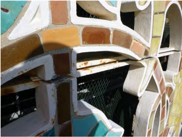
310-173 ArchMetal_Corrosion Surface 2024-2.jpg
