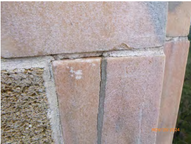
67-108 Stone_Crack Repair failed 2024-2.jpg
