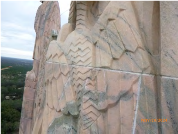
134-196 Stone_Repair Dutchman Failed 2024-2.jpg
