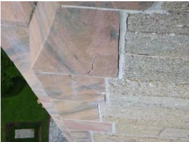
135-123 Stone_Crack System units and joints 2024-4.jpg
