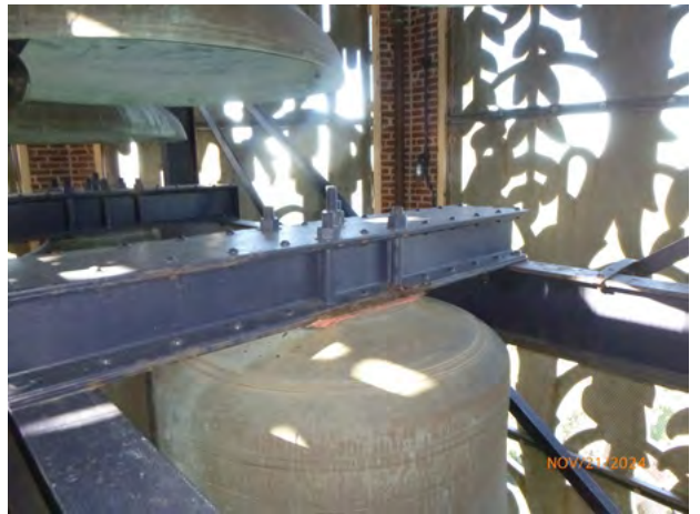
555-160 ArchMetal_Coating Coating Failed 2024-1.jpg
