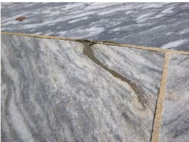
45-0 Stone_Crack Repair failed 2024-1.jpg
