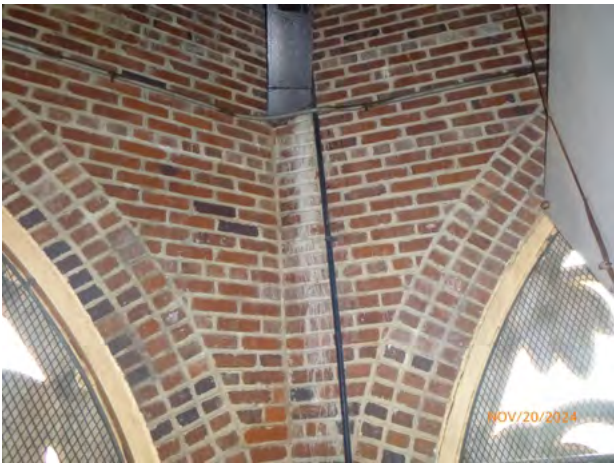
860-177 Brick_SoilStain Leached Salts 2024-1.jpg
