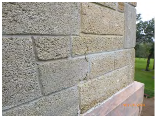
66-32 Stone_Crack System units and joints 2024-1.jpg
