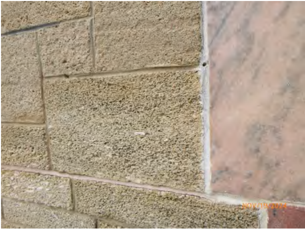
241-130 Stone_Joints Sealant Failed 2024-3.jpg
