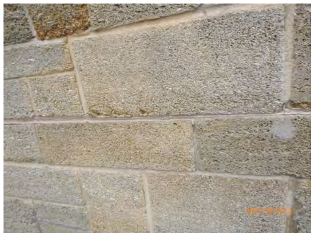
62-81 Stone_Joints Sealant Failed 2024-4.jpg
