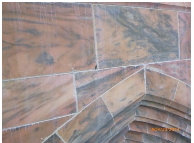
137-182 Stone_Spall Removed 2024-3.jpg
