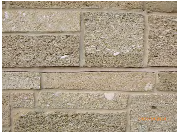
240-90 Stone_Joints Sealant Failed 2024-3.jpg
