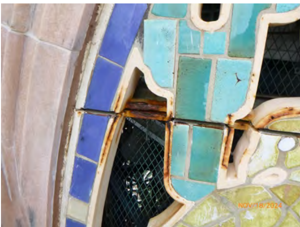
392-174 ArchMetal_Coating Coating Failed 2024-5.jpg
