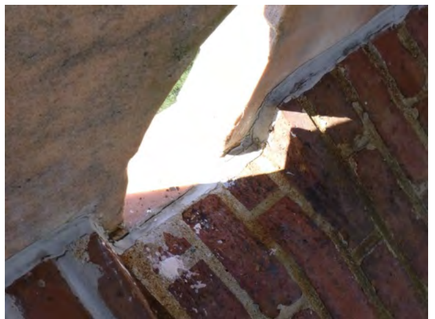
639-185 Brick_Joints Sealant Failed 2024-1.jpg
