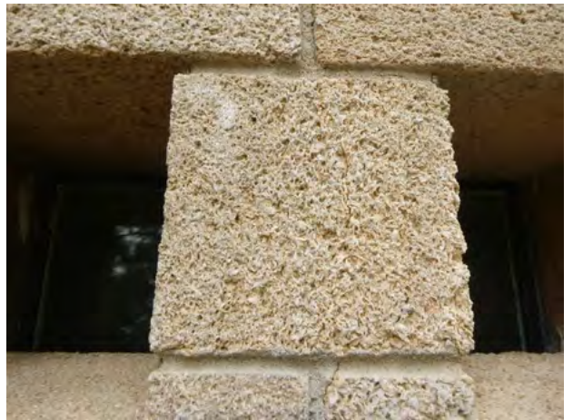
262-11 Stone_Crack Single unit 2024-1.jpg
