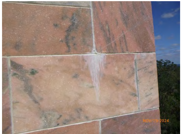
272-71 Stone_SoilStain Leached Salts 2024-1.jpg
