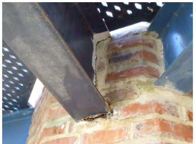
634-193 ArchMetal_Corrosion Surface 2024-1.jpg
