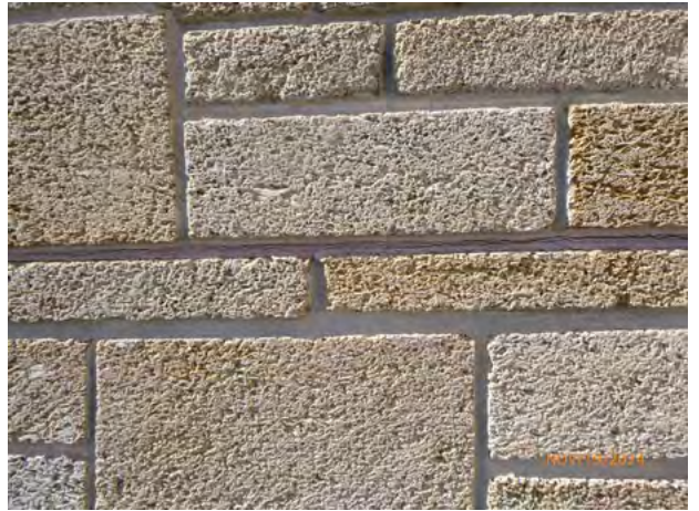
340-80 Stone_Joints Sealant Failed 2024-3.jpg
