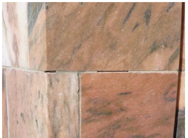
336-188 Stone_Joints Mortar Failed 2024-1.jpg
