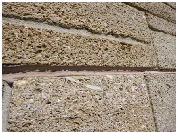
264-82 Stone_Joints Sealant Failed 2024-2.jpg
