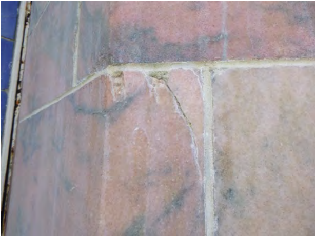
41-169 Stone_Crack Single unit 2024-1.jpg
