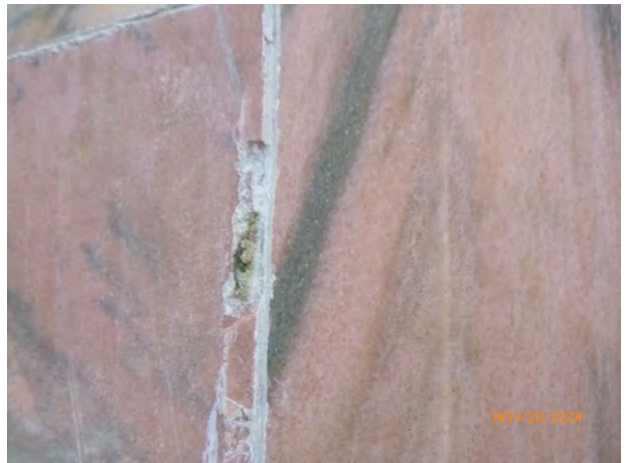
132-161 Stone_Spall Removed 2024-2.jpg
