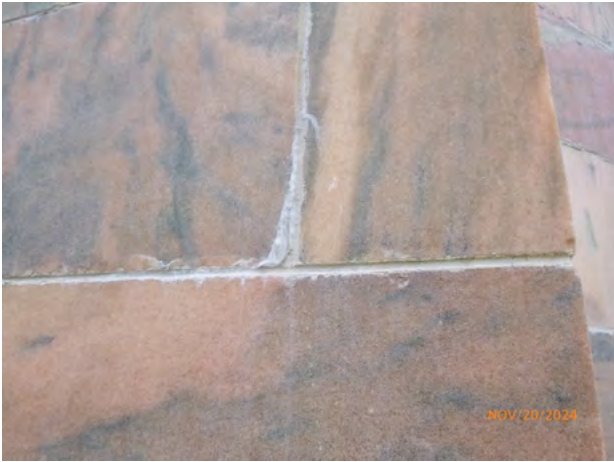
59-177 Stone_SoilStain Leached Salts 2024-2.jpg
