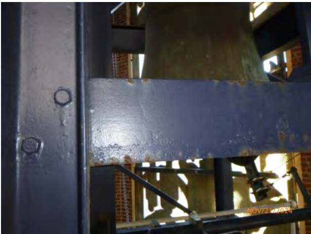
742-150 ArchMetal_Coating Coating Failed 2024-2.jpg
