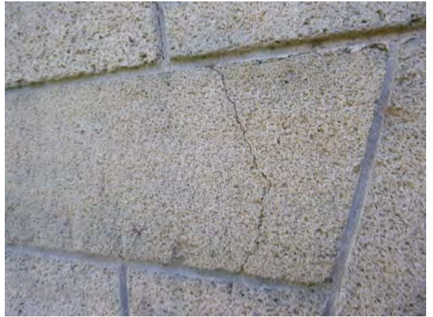
37-15 Stone_Crack Single unit 2024-1.jpg
