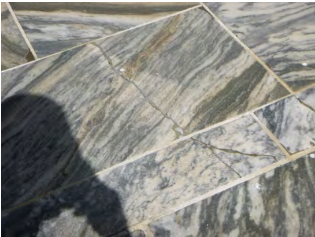
226-1 Stone_Crack Repair failed 2024-1.jpg
