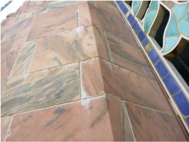
204-157 Stone_SoilStain Leached Salts 2024-1.jpg
