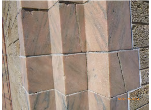
333-132 Stone_Crack Repair failed 2024-1.jpg
