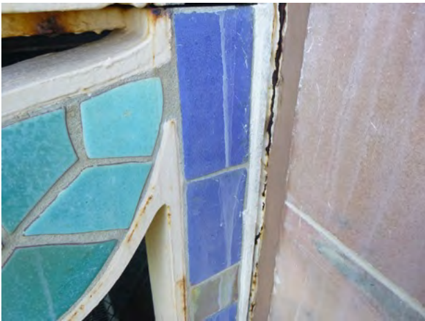
19-159 ArchMetal_Corrosion Pitted 2024-2.jpg
