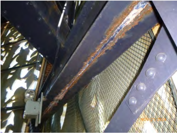
555-145 ArchMetal_Coating Coating Failed 2024-1.jpg
