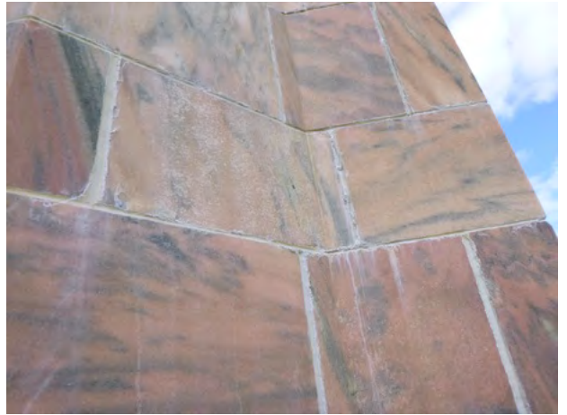
42-172 Stone_SoilStain Leached Salts 2024-1.jpg
