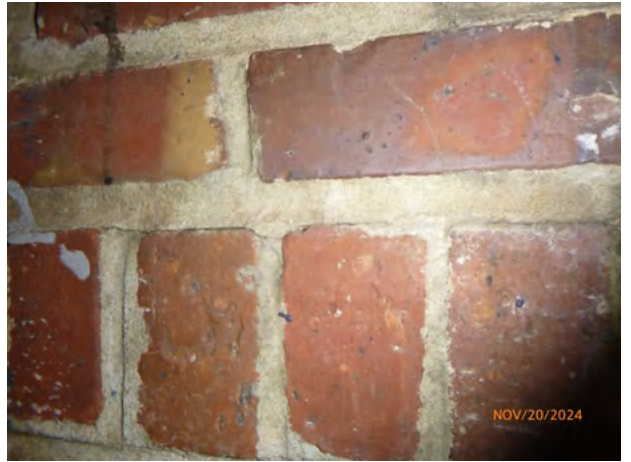
759-143 Brick_Joints Mortar Failed 2024-2.jpg
