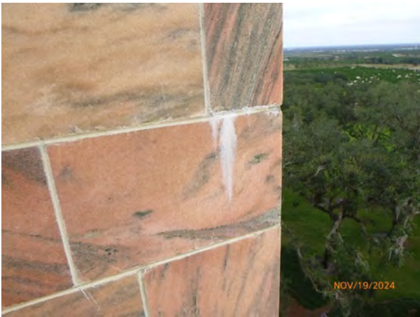
172-88 Stone_SoilStain Leached Salts 2024-1.jpg
