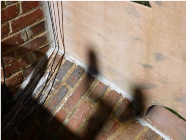
543-185 Brick_Joints Sealant Failed 2024-1.jpg
