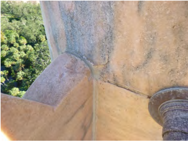
551-195 Stone_Spall Missing 2024-1.jpg
