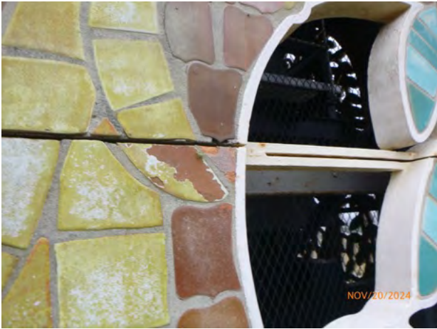
114-163 TerraCotta_SurfLoss Glaze loss 2024-1.jpg
