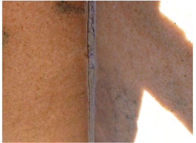
531-191 Stone_Joints Mortar Failed 2024-2.jpg
