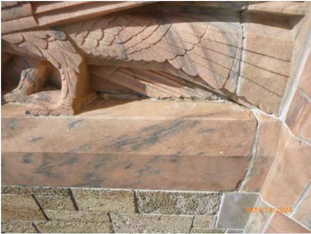
341-139 Stone_Joints Mortar Failed 2024-1.jpg
