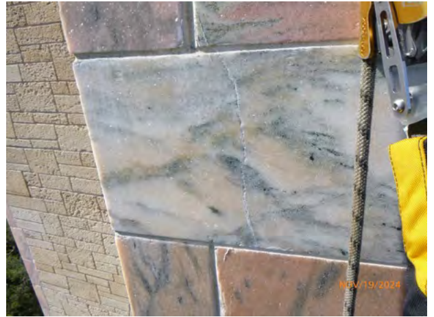
343-117 Stone_Crack Single unit 2024-1.jpg
