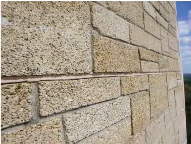
263-125 Stone_Joints Sealant Failed 2024-1.jpg
