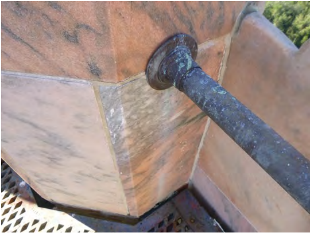
643-196 Stone_Joints Mortar Failed 2024-1.jpg
