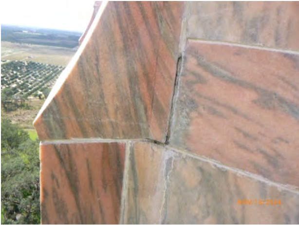
32-181 Stone_Joints Mortar Failed 2024-1.jpg
