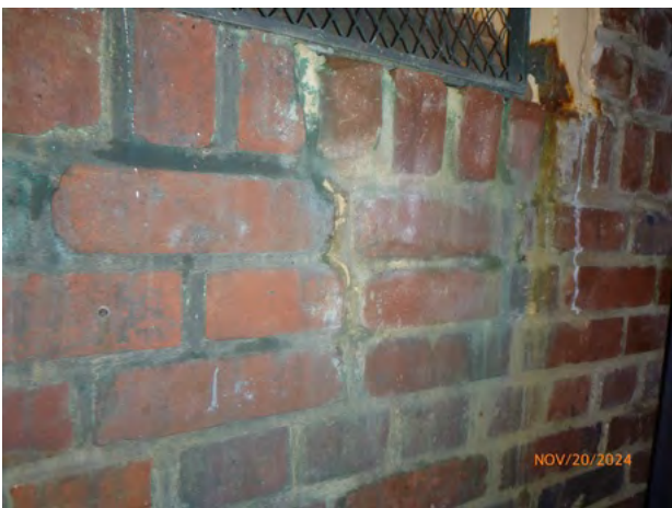
856-143 Brick_Repair Patch Failed 2024-2.jpg
