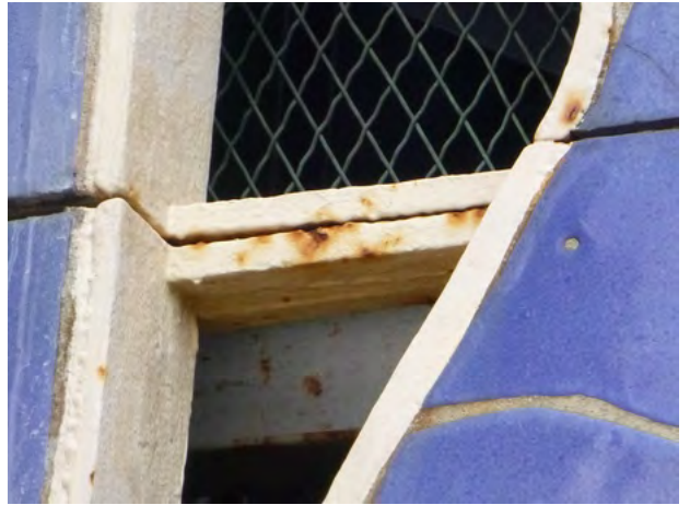
86-149 ArchMetal_Corrosion Surface 2024-1.jpg
