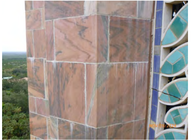
136-170 Stone_SoilStain Leached Salts 2024-1.jpg
