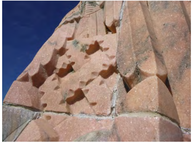
334-192 Stone_Joints Mortar Failed 2024-2.jpg
