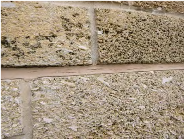
164-90 Stone_Joints Sealant Failed 2024-2.jpg
