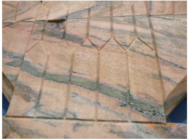
237-193 Stone_Spall Missing 2024-2.jpg
