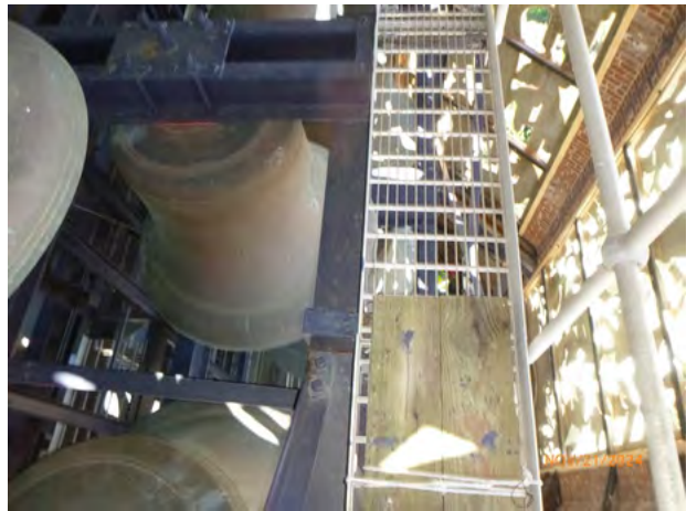
741-169 ArchMetal_Coating Coating Failed 2024-1.jpg
