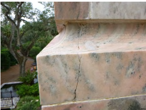
228-27 Stone_Crack Single unit 2024-1.jpg
