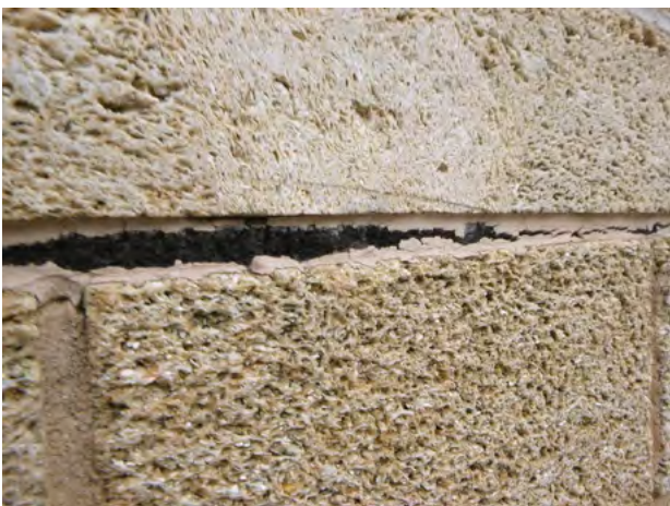
164-40 Stone_Joints Sealant Failed 2024-1.jpg
