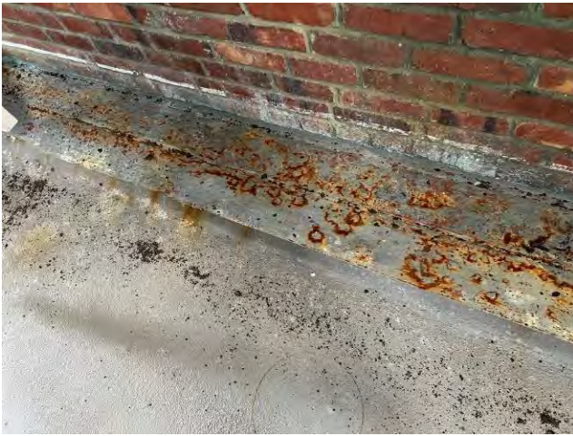
11 Lower Roof surface degradation
