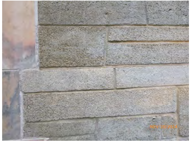
61-37 Stone_Joints Sealant Failed 2024-2.jpg
