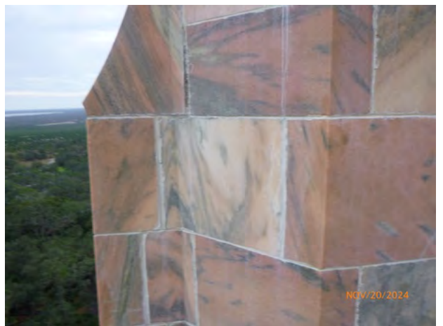
138-179 Stone_SoilStain Leached Salts 2024-3.jpg
