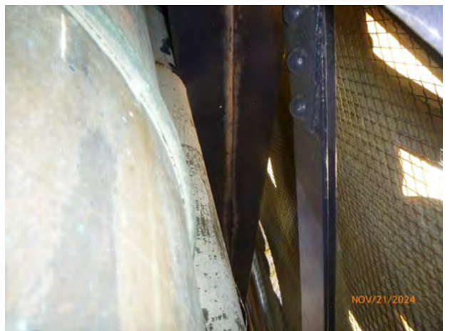
760-145 ArchMetal_Coating Coating Failed 2024-4.jpg
