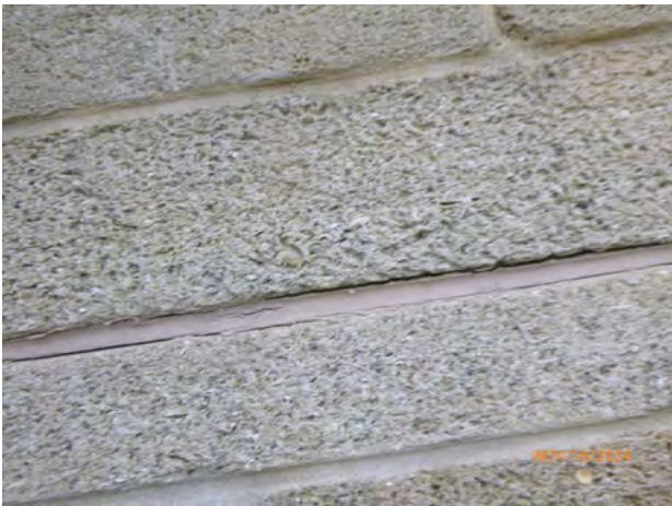
361-96 Stone_Joints Sealant Failed 2024-5.jpg
