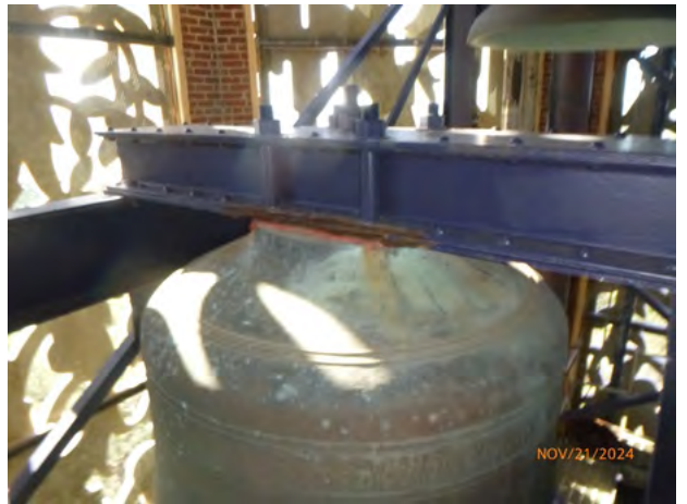
561-160 ArchMetal_Coating Coating Failed 2024-1.jpg
