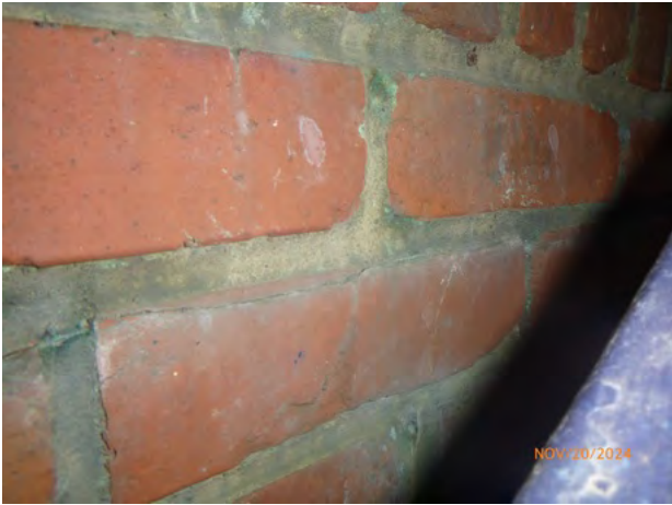
854-143 Brick_Crack System units and joints 2024-2.jpg
