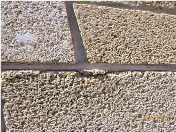
341-89 Stone_Joints Sealant Failed 2024-4.jpg
