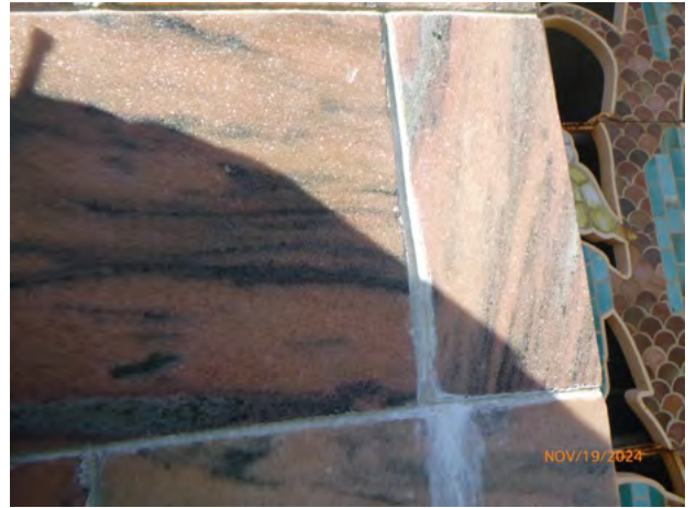
343-154 Stone_SoilStain Leached Salts 2024-2.jpg
