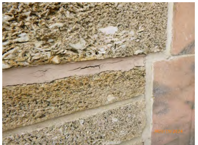
240-112 Stone_Joints Sealant Failed 2024-3.jpg
