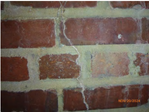
546-181 Brick_Crack System units and joints 2024-2.jpg
