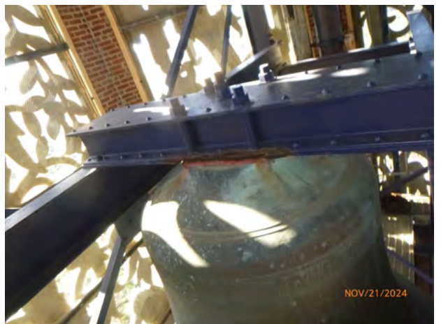
561-160 ArchMetal_Coating Coating Failed 2024-3.jpg
