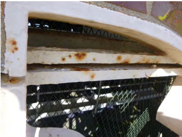
311-172 ArchMetal_Coating Coating Failed 2024-1.jpg
