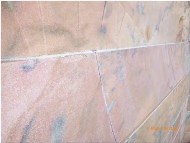
37-184 Stone_SurfLoss Chipped 2024-3.jpg
