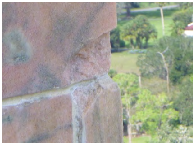
41-168 Stone_Spall Missing 2024-1.jpg
