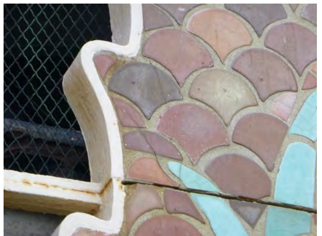
88-150 TerraCotta_Crack Single unit 2024-1.jpg
