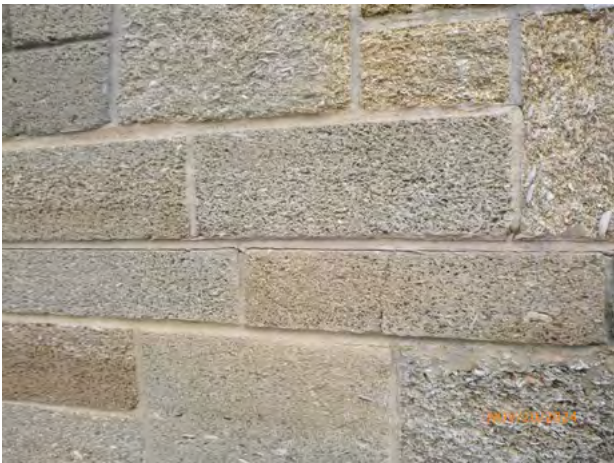
61-90 Stone_Joints Sealant Failed 2024-4.jpg
