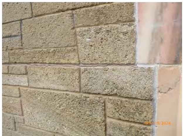
241-44 Stone_Joints Sealant Failed 2024-4.jpg
