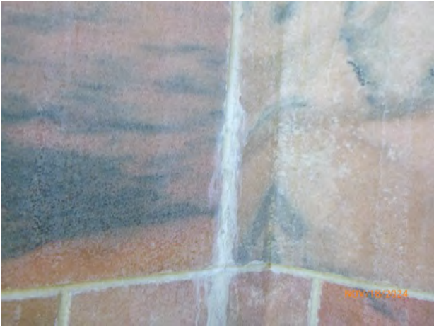
32-136 Stone_SoilStain Leached Salts 2024-2.jpg
