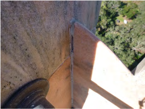
531-191 Stone_Joints Mortar Failed 2024-1.jpg
