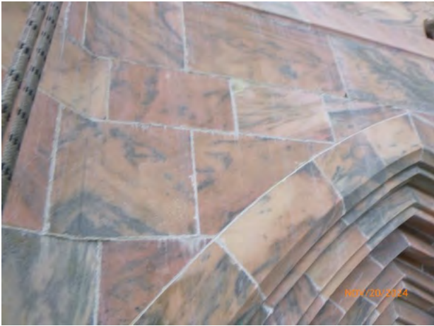
138-179 Stone_SoilStain Leached Salts 2024-4.jpg
