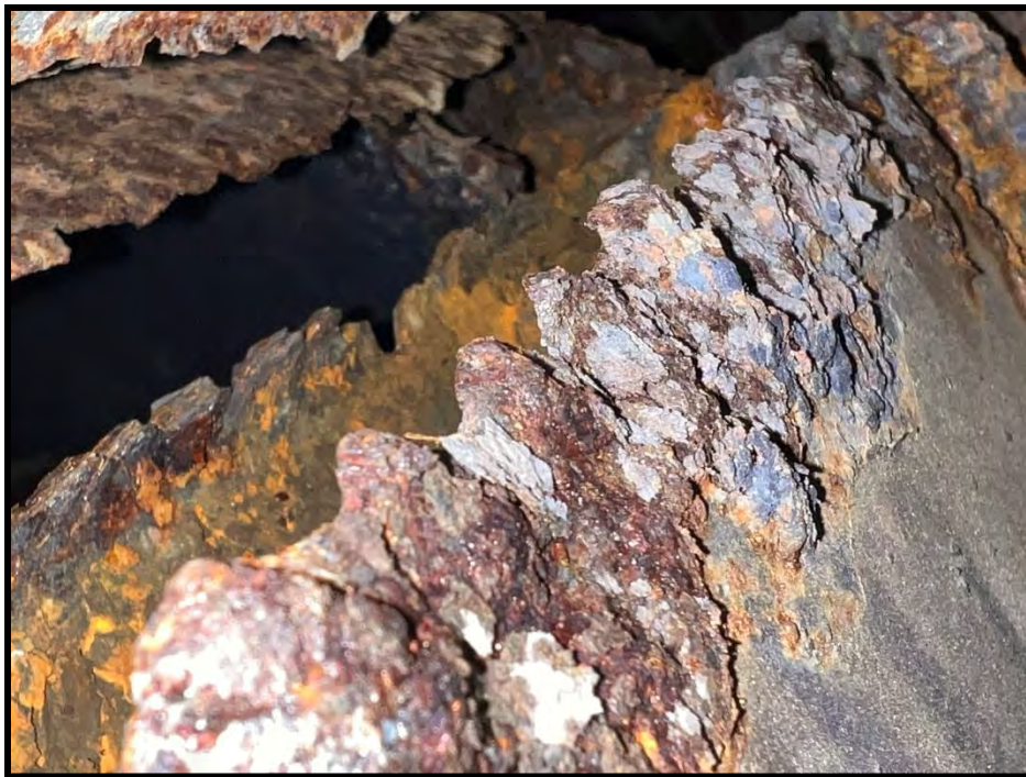
Figure 16 Corrosion of roof steel framing
