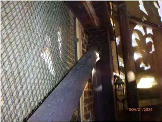
656-144 ArchMetal_Coating Coating Failed 2024-1.jpg
