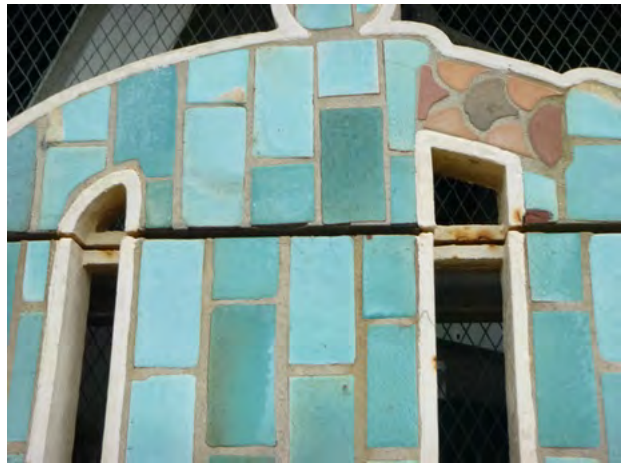
87-167 ArchMetal_Coating Coating Failed 2024-2.jpg
