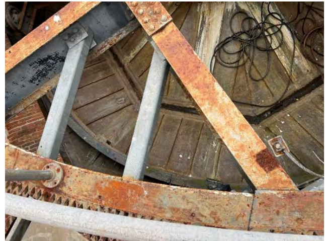
17 Corrosion at roof steel structure
