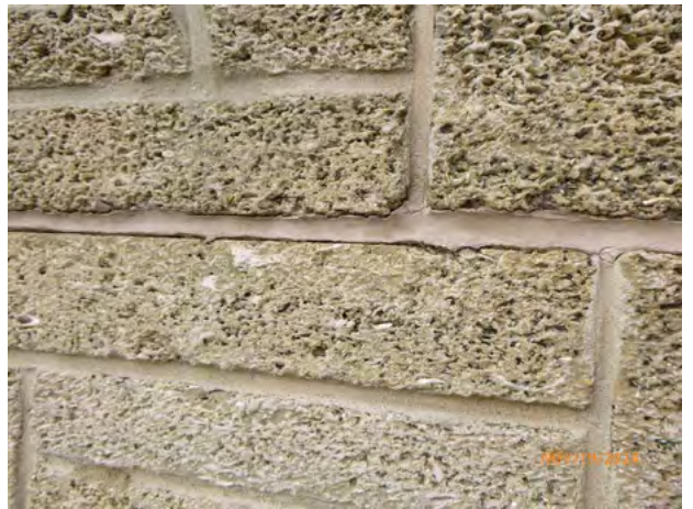
240-69 Stone_Joints Sealant Failed 2024-2.jpg
