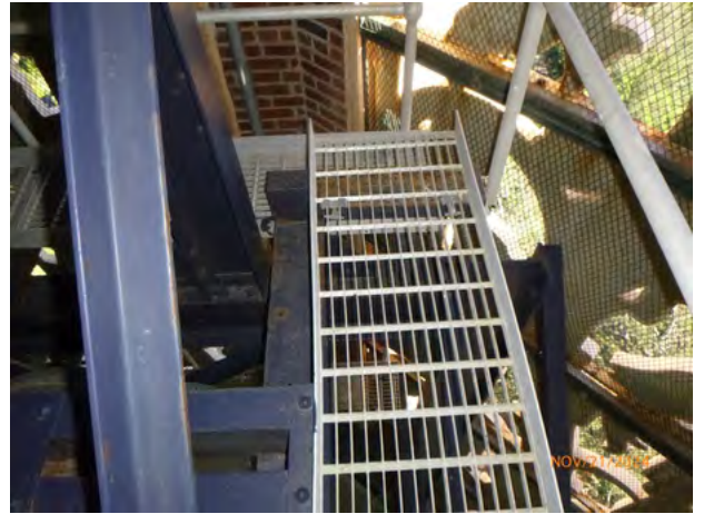
741-169 ArchMetal_Coating Coating Failed 2024-5.jpg
