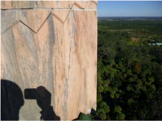
538-201 Stone_Crack Repair failed 2024-2.jpg
