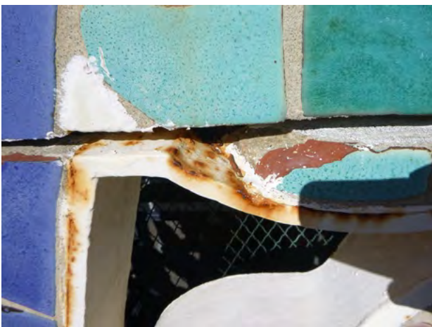
309-173 TerraCotta_Spall Missing 2024-1.jpg
