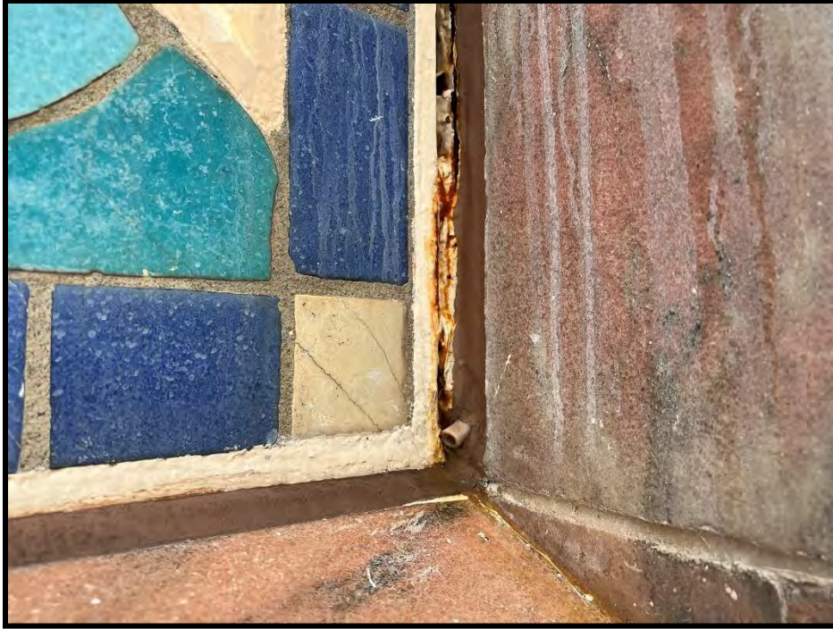
Figure 39 Failed sealant joint at perimeter of the mosaic
