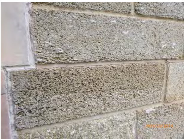
61-101 Stone_Joints Sealant Failed 2024-2.jpg
