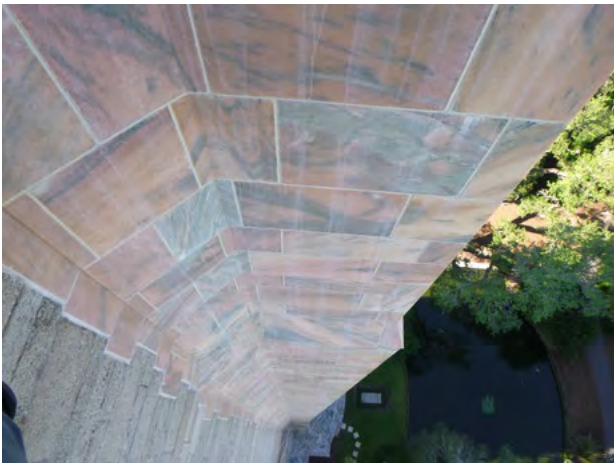
42-128 Stone_SoilStain Efflorescence 2024-3.jpg
