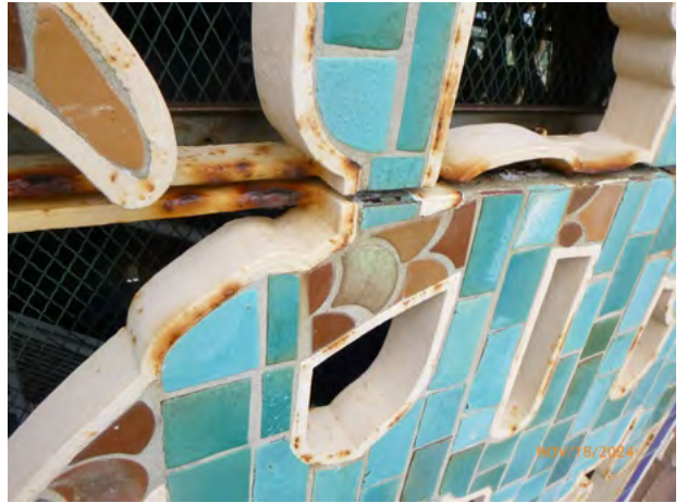
392-174 ArchMetal_Coating Coating Failed 2024-8.jpg
