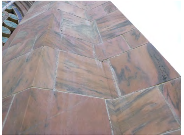
125-164 Stone_SoilStain Leached Salts 2024-1.jpg
