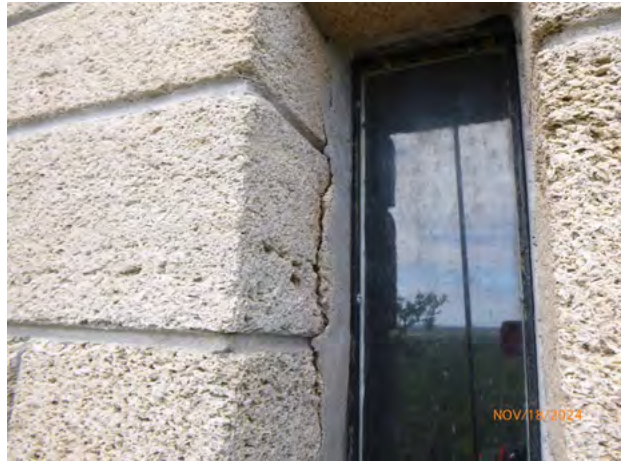
34-56 Stone_Joints Mortar Failed 2024-1.jpg
