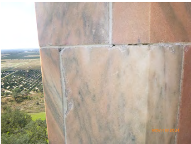
33-188 Stone_Spall Missing 2024-1.jpg
