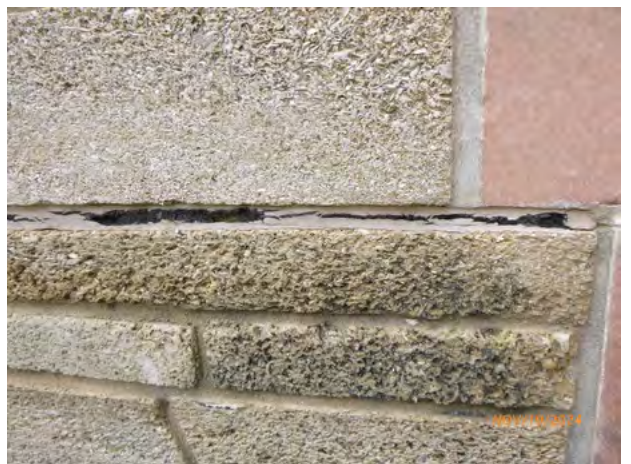
241-37 Stone_Joints Sealant Failed 2024-2.jpg
