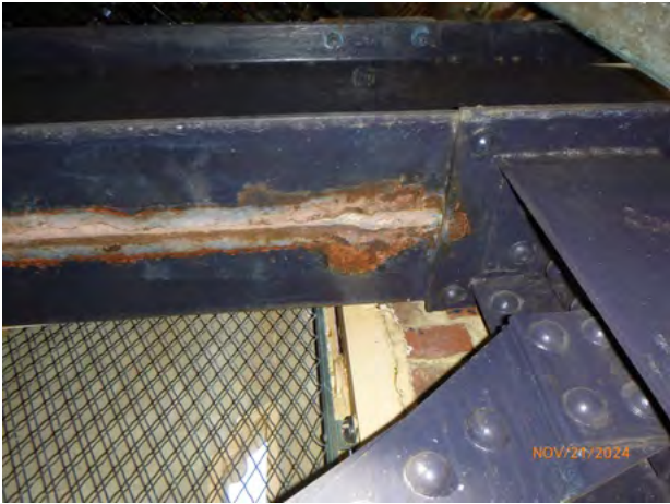
657-144 ArchMetal_Coating Coating Failed 2024-2.jpg
