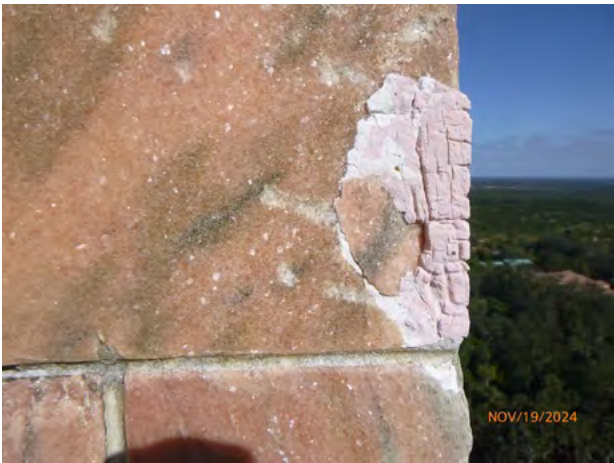
342-183 Stone_Repair Patch Failed 2024-2.jpg
