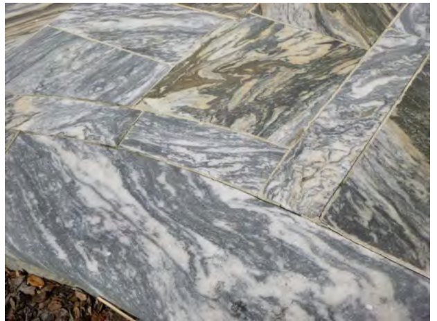
265-1 Stone_Joints Mortar Failed 2024-1.jpg
