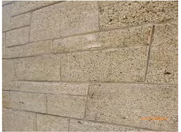
336-13 Stone_Crack System units and joints 2024-3.jpg
