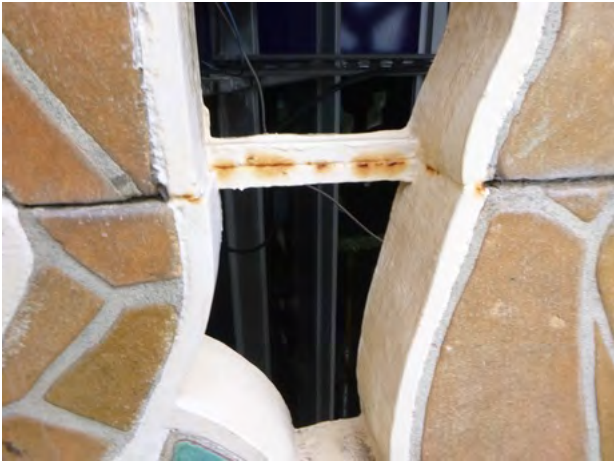
87-133 ArchMetal_Corrosion Surface 2024-1.jpg
