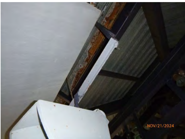
848-180 ArchMetal_Corrosion Perforated 2024-5.jpg
