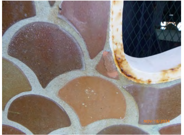
388-151 TerraCotta_Coating Coating Failed 2024-2.jpg
