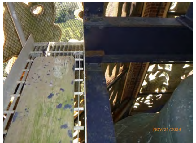
561-157 ArchMetal_Coating Coating Failed 2024-6.jpg
