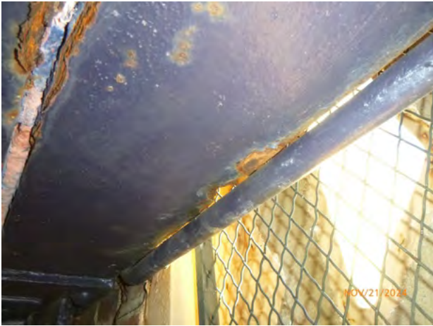
861-145 ArchMetal_Coating Coating Failed 2024-4.jpg
