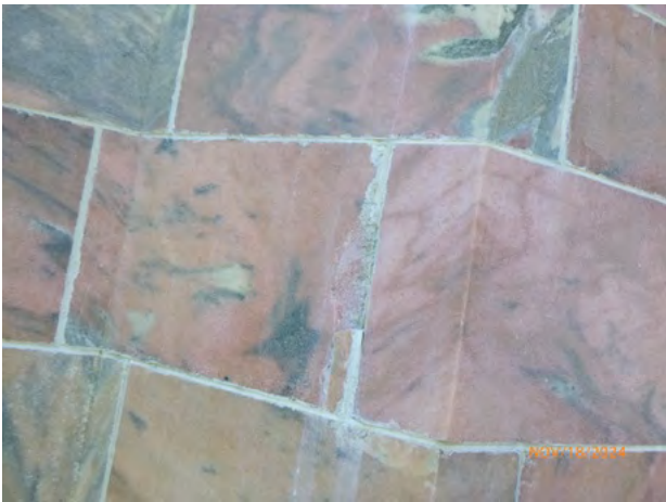
35-163 Stone_Spall Missing 2024-1.jpg
