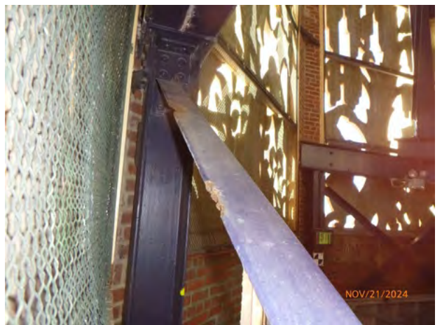
859-145 ArchMetal_Damaged Dented 2024-3.jpg
