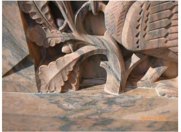
341-139 Stone_Joints Mortar Failed 2024-2.jpg
