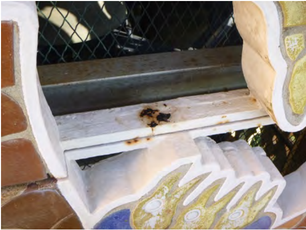
289-168 ArchMetal_Corrosion Surface 2024-1.jpg
