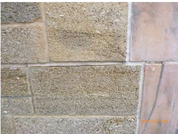
61-109 Stone_Joints Sealant Failed 2024-4.jpg
