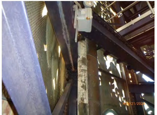
760-145 ArchMetal_Coating Coating Failed 2024-2.jpg
