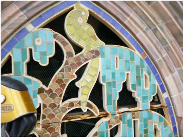
392-174 ArchMetal_Coating Coating Failed 2024-1.jpg
