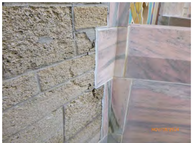
346-104 Stone_Crack System units and joints 2024-4.jpg
