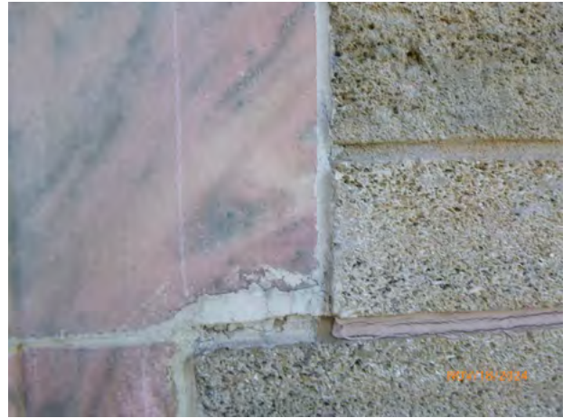
360-131 Stone_Repair Patch Failed 2024-2.jpg
