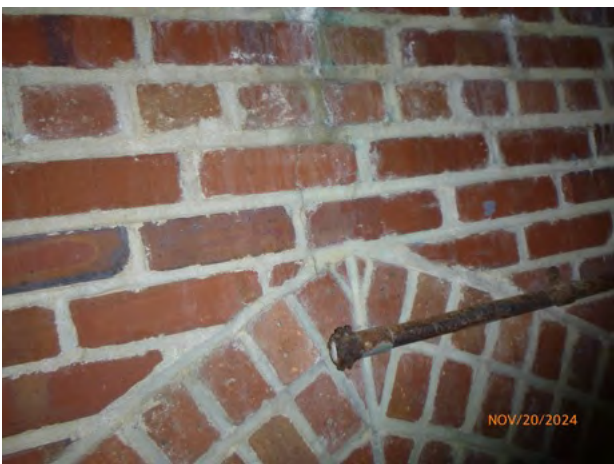
651-179 Brick_Crack System units and joints 2024-3.jpg
