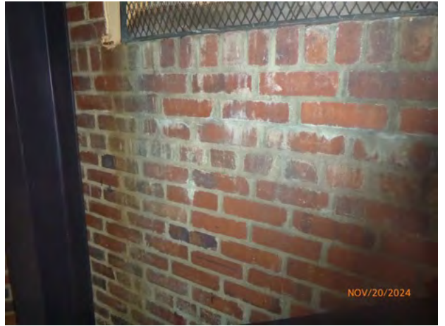
646-139 Brick_SoilStain Leached Salts 2024-1.jpg
