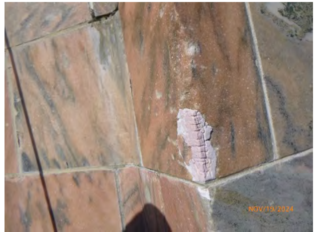
342-183 Stone_Repair Patch Failed 2024-3.jpg
