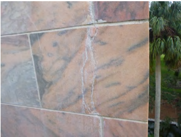
72-46 Stone_Crack Single unit 2024-1.jpg
