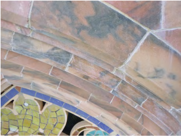
15-179 Stone_SoilStain Efflorescence 2024-1.jpg
