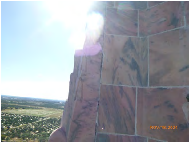
31-158 Stone_Joints Mortar Failed 2024-1.jpg
