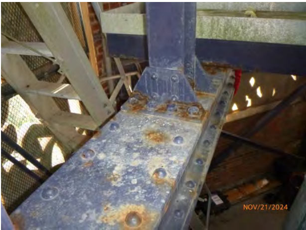
844-147 ArchMetal_Corrosion Fastener rusted 2024-4.jpg
