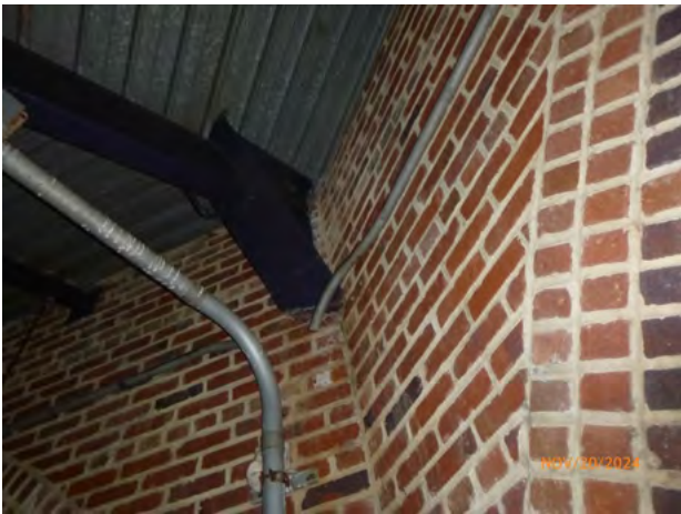
847-178 Brick_SoilStain Leached Salts 2024-1.jpg
