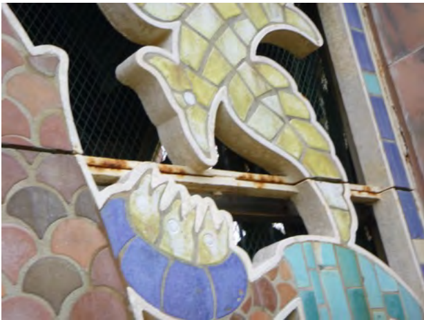
87-167 ArchMetal_Coating Coating Failed 2024-1.jpg
