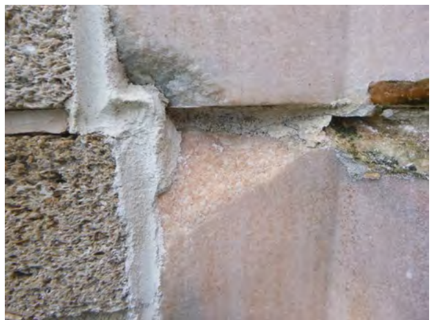
140-69 Stone_Spall Missing 2024-1.jpg
