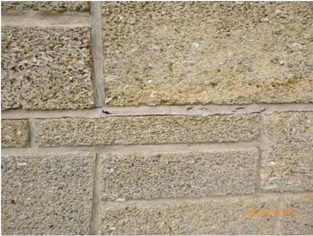
240-112 Stone_Joints Sealant Failed 2024-4.jpg
