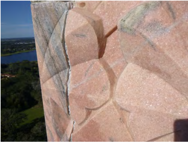
334-192 Stone_Joints Mortar Failed 2024-1.jpg
