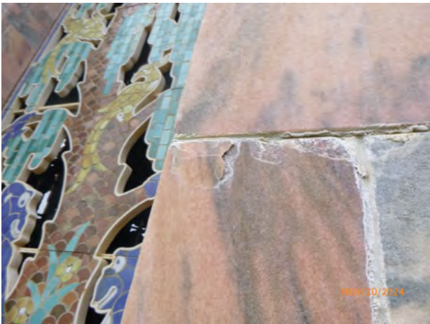
129-149 Stone_Spall Removed 2024-1.jpg
