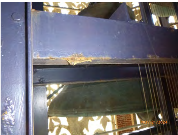
664-151 ArchMetal_Coating Coating Failed 2024-2.jpg
