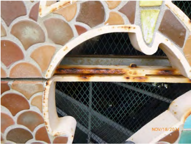
392-174 ArchMetal_Coating Coating Failed 2024-7.jpg
