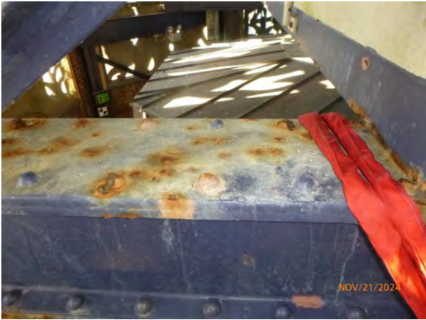
844-147 ArchMetal_Corrosion Fastener rusted 2024-2.jpg
