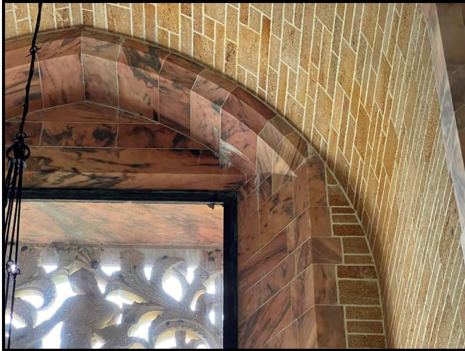
Figure 22 Efflorescence in the Founders Room at Level 1, just below an exterior balcony
