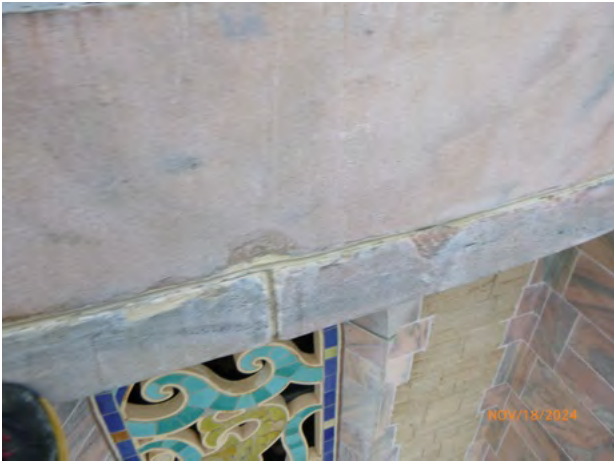
351-122 Stone_SurfLoss Chipped 2024-1.jpg
