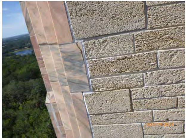
335-128 Stone_Crack Repair failed 2024-2.jpg
