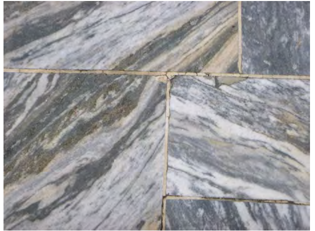
55-1 Stone_Joints Mortar Failed 2024-1.jpg
