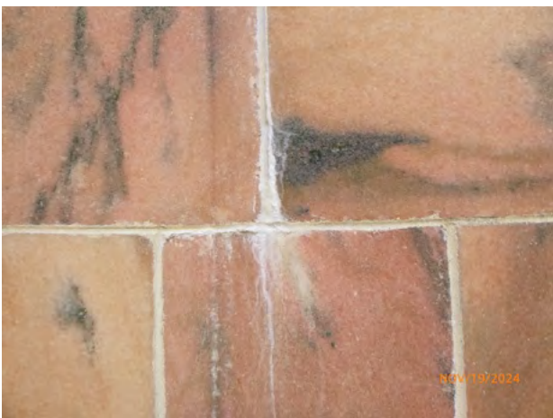
243-142 Stone_SoilStain Leached Salts 2024-2.jpg
