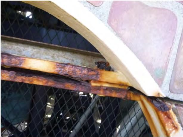
15-158 ArchMetal_Corrosion Fastener rusted 2024-1.jpg
