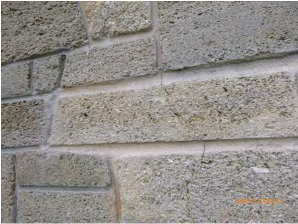
366-55 Stone_Crack System units and joints 2024-3.jpg
