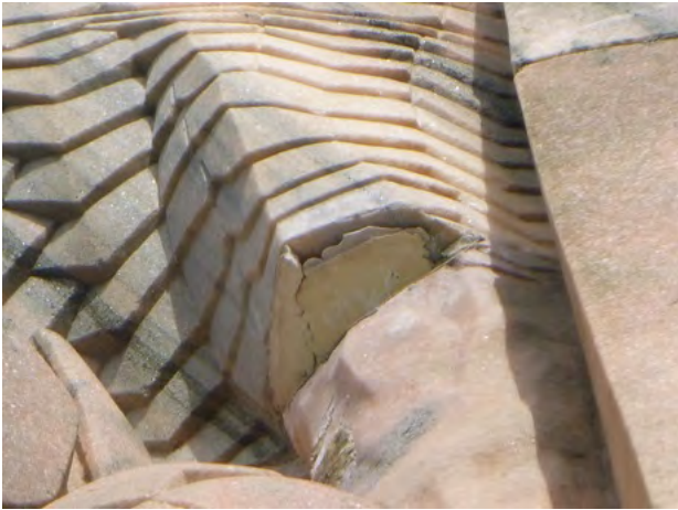
167-202 Stone_Repair Patch Failed 2024-1.jpg
