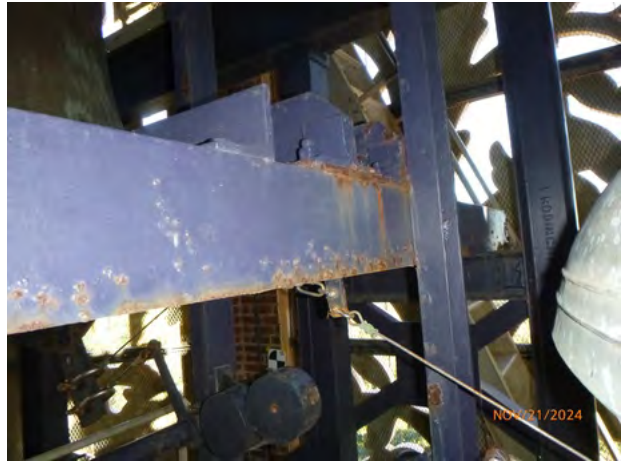
742-150 ArchMetal_Coating Coating Failed 2024-1.jpg
