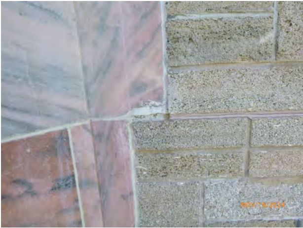
360-131 Stone_Repair Patch Failed 2024-1.jpg
