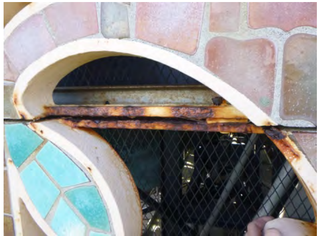
16-158 ArchMetal_Corrosion Pitted 2024-1.jpg
