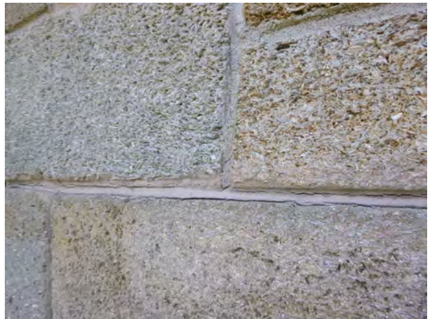
37-43 Stone_Joints Sealant Failed 2024-2.jpg
