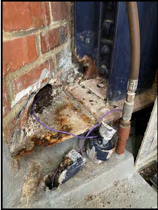
Figure 13 Part of the cathodic protection system visible at Level 7 outside of the Playing Cabin
