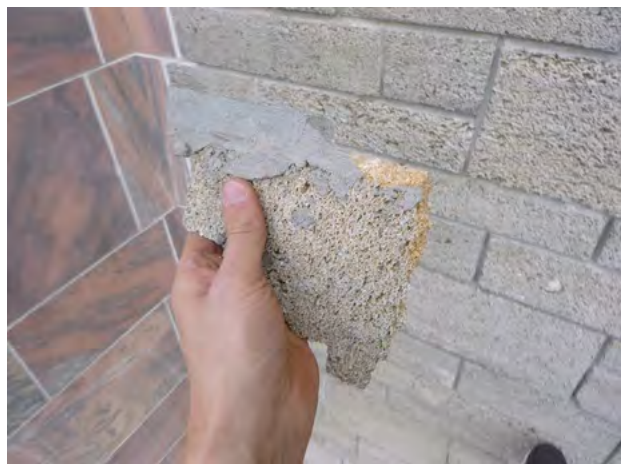
50-88 Stone_Spall Removed 2024-2.jpg
