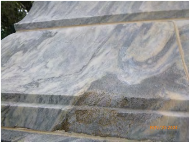
128-4 Stone_Spall Missing 2024-3.jpg
