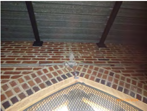
854-180 Brick_SoilStain Leached Salts 2024-1.jpg
