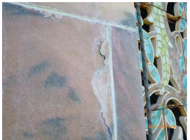
35-160 Stone_Spall Removed 2024-2.jpg
