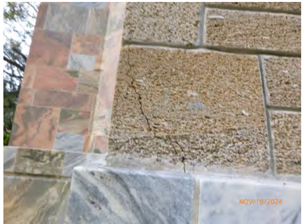
235-11 Stone_Crack Single unit 2024-1.jpg
