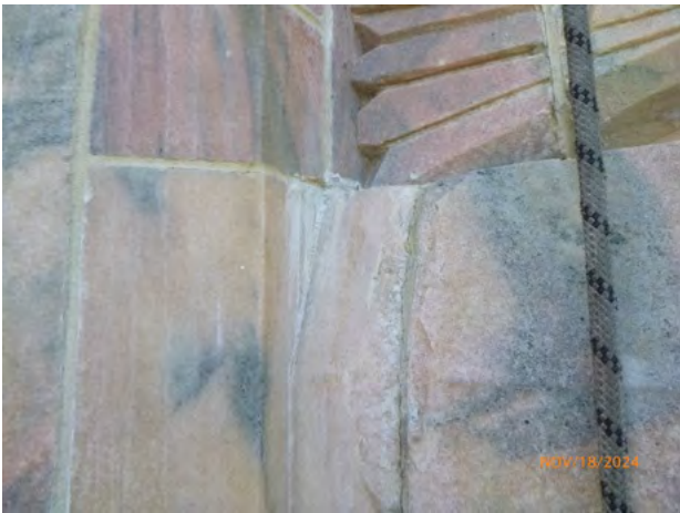
360-138 Stone_SoilStain Leached Salts 2024-1.jpg
