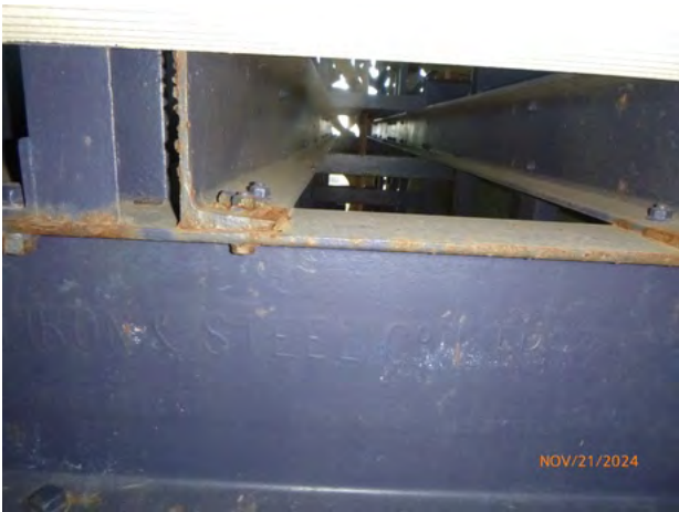
562-170 ArchMetal_Coating Coating Failed 2024-3.jpg
