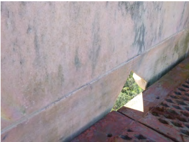
862-194 Stone_Crack System joints 2024-1.jpg
