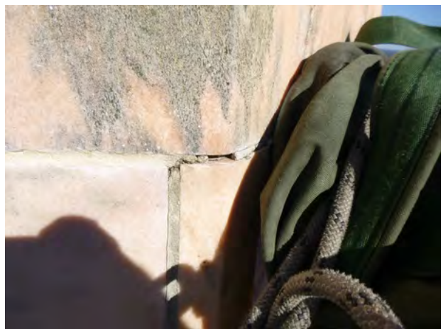
539-193 Stone_Joints Mortar Failed 2024-2.jpg
