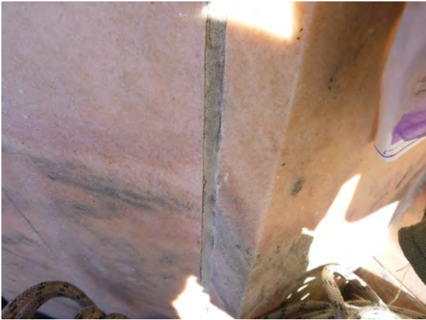
539-193 Stone_Joints Mortar Failed 2024-3.jpg
