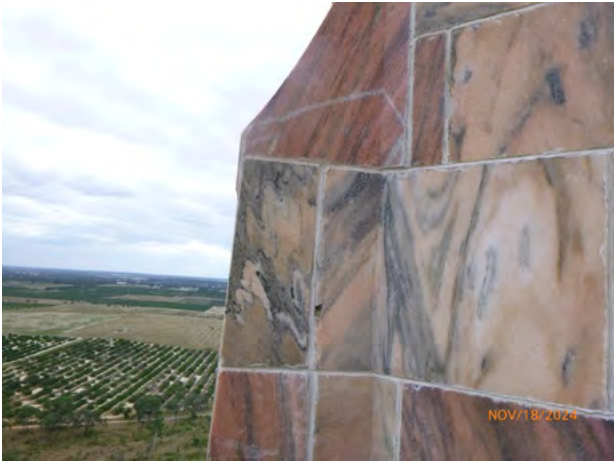
345-181 Stone_Joints Mortar Failed 2024-2.jpg
