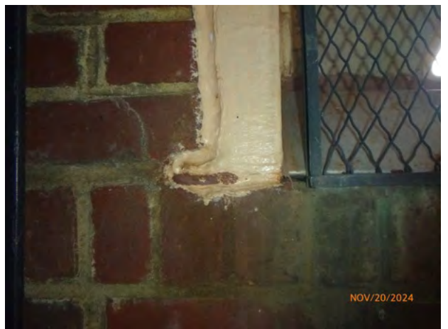
645-144 ArchMetal_Corrosion Surface 2024-1.jpg
