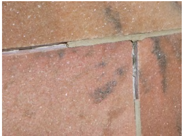
338-184 Stone_Joints Mortar Failed 2024-1.jpg
