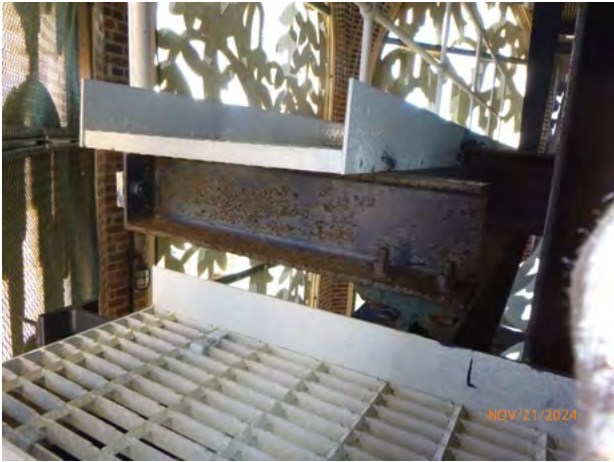
562-172 ArchMetal_Corrosion Surface 2024-1.jpg
