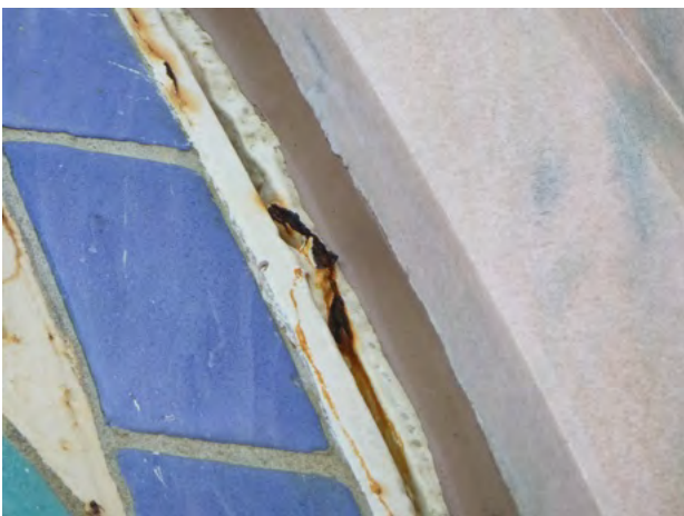
18-169 ArchMetal_Corrosion Pitted 2024-3.jpg
