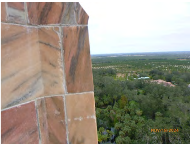
355-181 Stone_SurfLoss Chipped 2024-2.jpg
