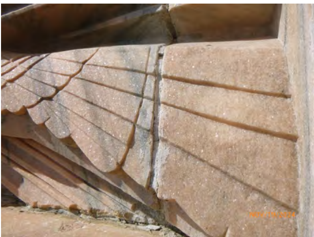
341-139 Stone_Joints Mortar Failed 2024-5.jpg
