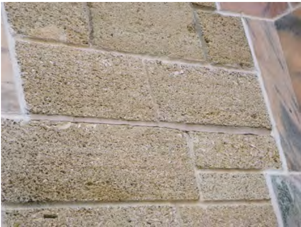
154-101 Stone_Joints Sealant Failed 2024-1.jpg
