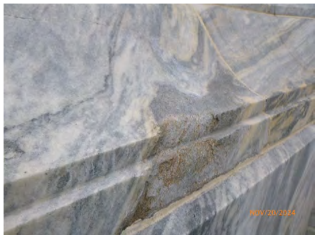
128-4 Stone_Spall Missing 2024-2.jpg
