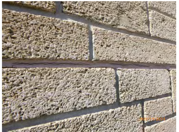
340-106 Stone_Joints Sealant Failed 2024-4.jpg
