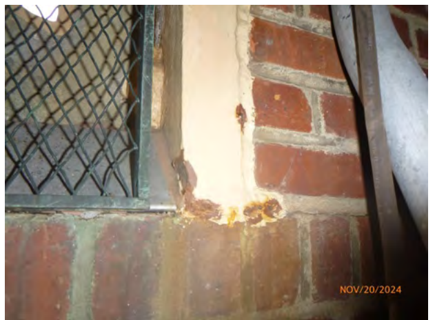
538-143 ArchMetal_Corrosion Pitted 2024-1.jpg
