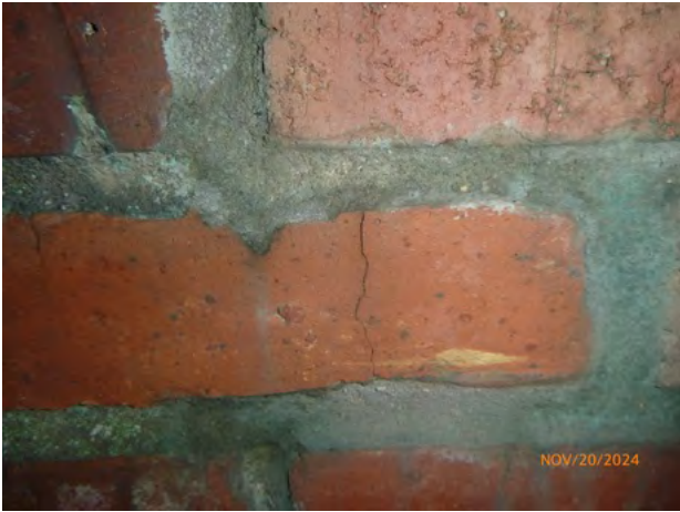
556-140 Brick_Crack Single unit 2024-1.jpg
