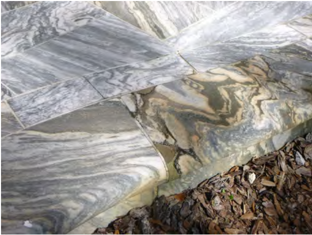
234-0 Stone_Joints Mortar Failed 2024-1.jpg
