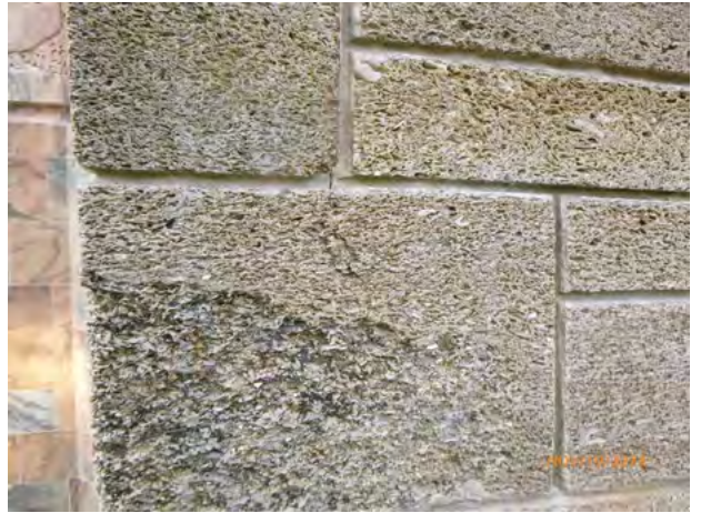
234-26 Stone_Crack System units and joints 2024-1.jpg
