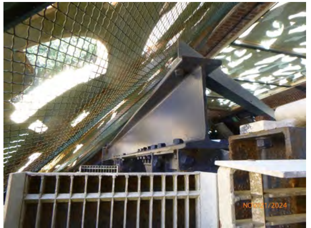
852-160 ArchMetal_Coating Coating Failed 2024-1.jpg
