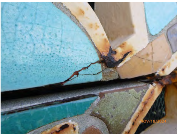
10-173 TerraCotta_Crack System units and joints 2024-2.jpg
