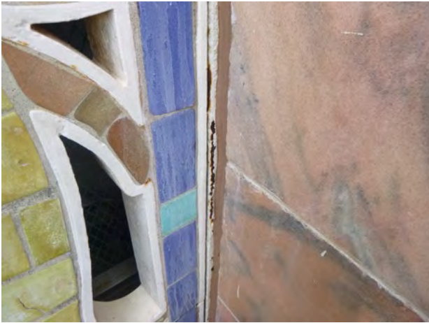
118-158 ArchMetal_Corrosion Pitted 2024-1.jpg
