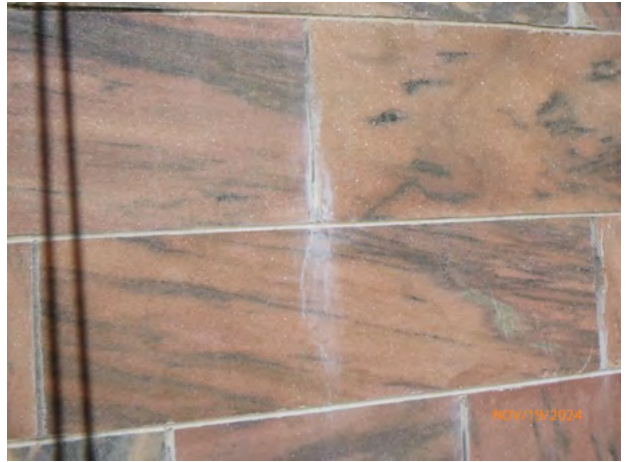
272-35 Stone_SoilStain Leached Salts 2024-1.jpg
