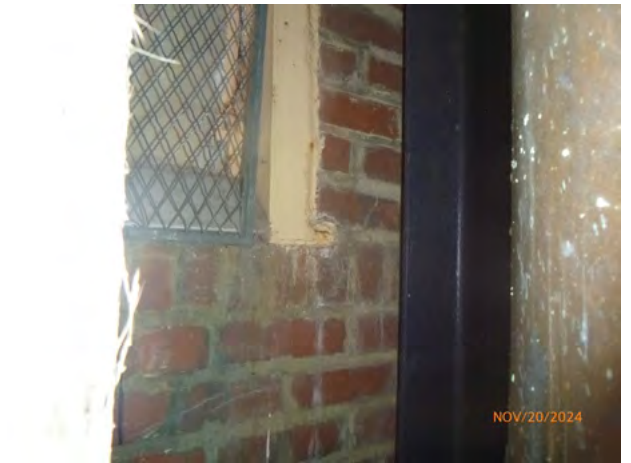
755-143 ArchMetal_Corrosion Surface 2024-1.jpg
