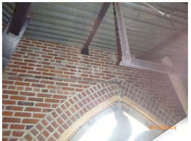
755-178 Brick_SoilStain Leached Salts 2024-1.jpg
