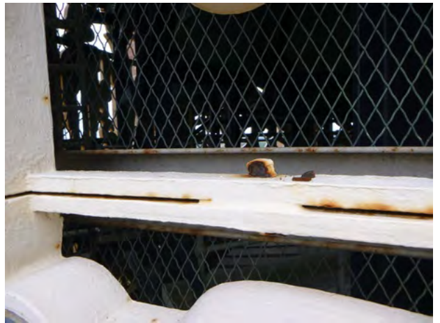
85-154 ArchMetal_Corrosion Surface 2024-1.jpg
