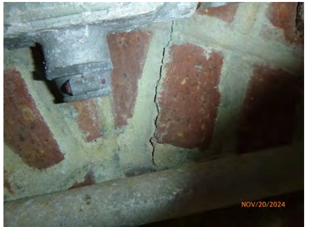
547-178 Brick_Joints Mortar Failed 2024-3.jpg
