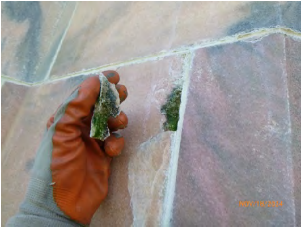
35-160 Stone_Spall Removed 2024-3.jpg
