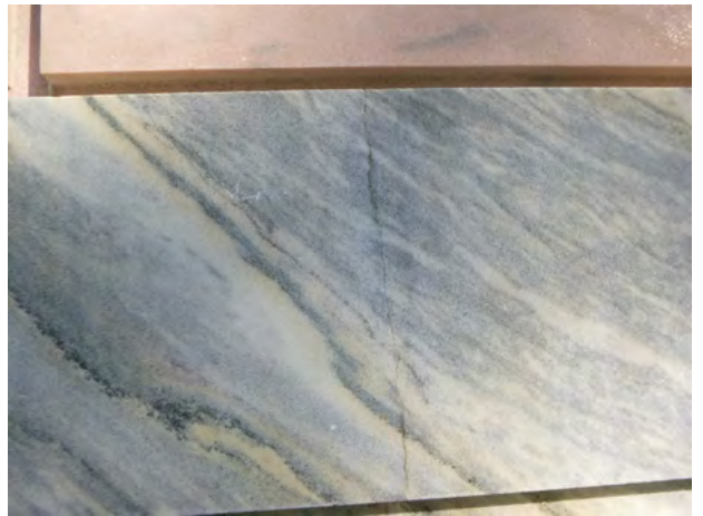
256-7 Stone_Crack Single unit 2024-1.jpg
