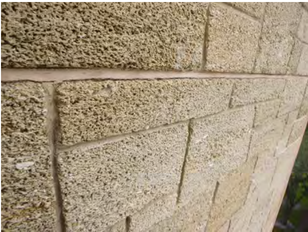
163-130 Stone_Joints Sealant Failed 2024-1.jpg
