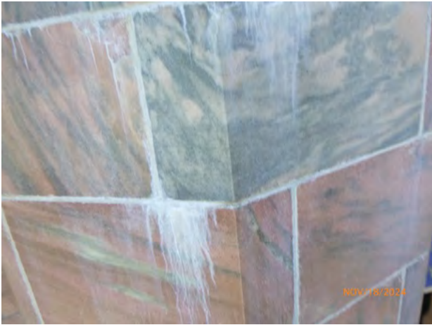
33-150 Stone_SoilStain Leached Salts 2024-2.jpg
