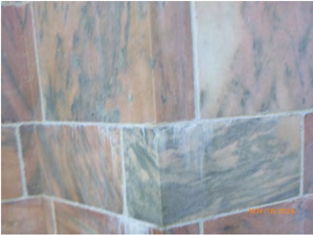
34-152 Stone_SurfLoss Chipped 2024-1.jpg
