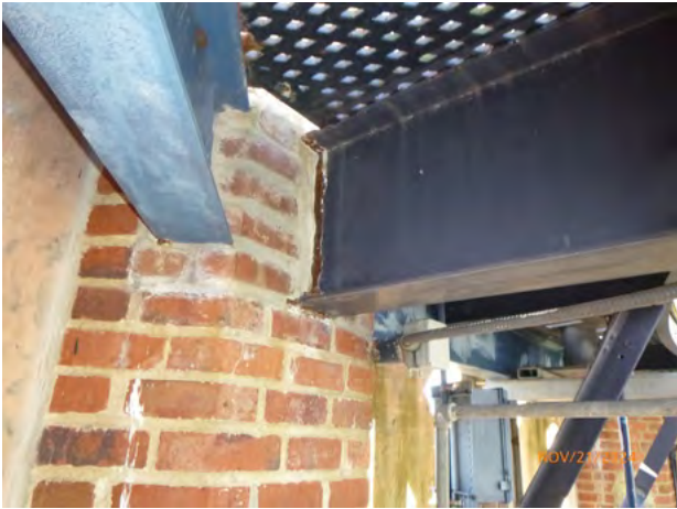
743-190 ArchMetal_Corrosion Surface 2024-1.jpg
