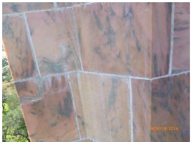
32-169 Stone_SurfLoss Chipped 2024-3.jpg
