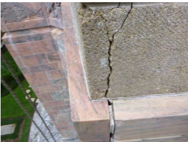
135-32 Stone_Crack System units and joints 2024-3.jpg
