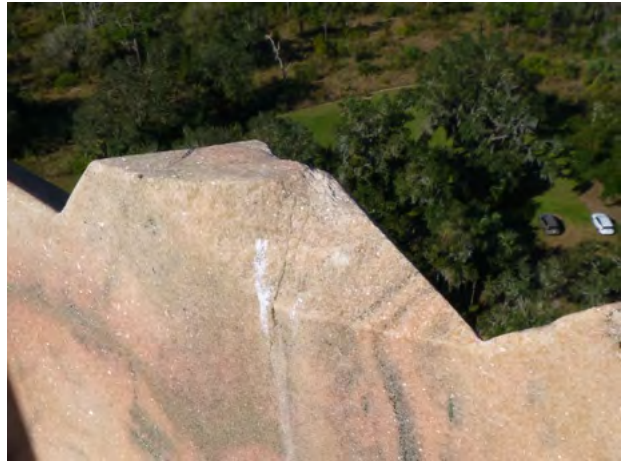
535-196 Stone_Spall Missing 2024-1.jpg
