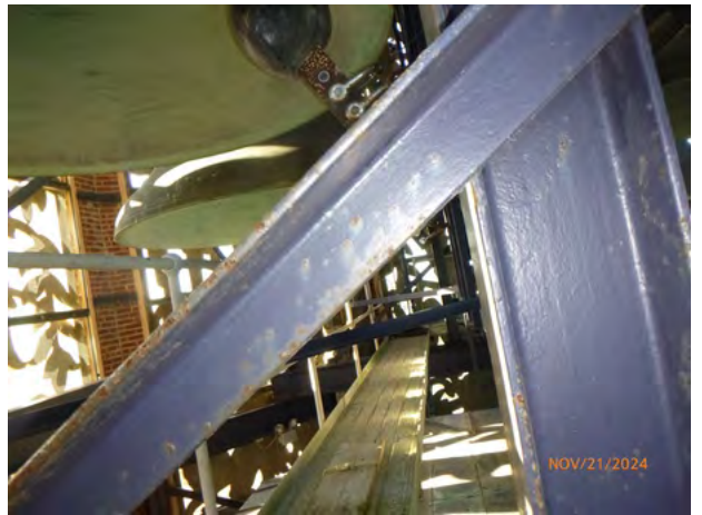
841-150 ArchMetal_Coating Coating Failed 2024-4.jpg
