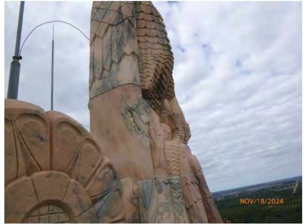
356-201 Stone_Spall Missing 2024-1.jpg
