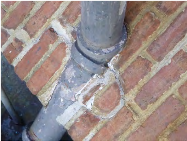
635-185 Brick_Joints Mortar Failed 2024-1.jpg
