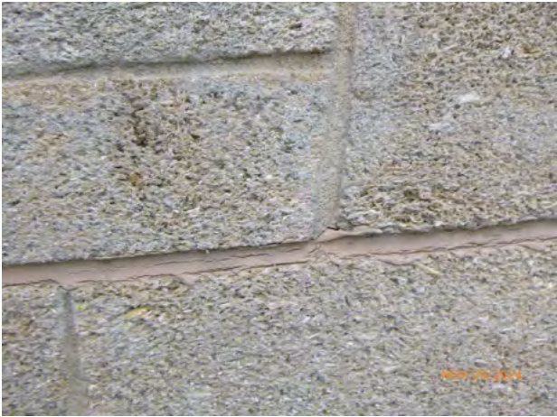
61-59 Stone_Joints Sealant Failed 2024-4.jpg
