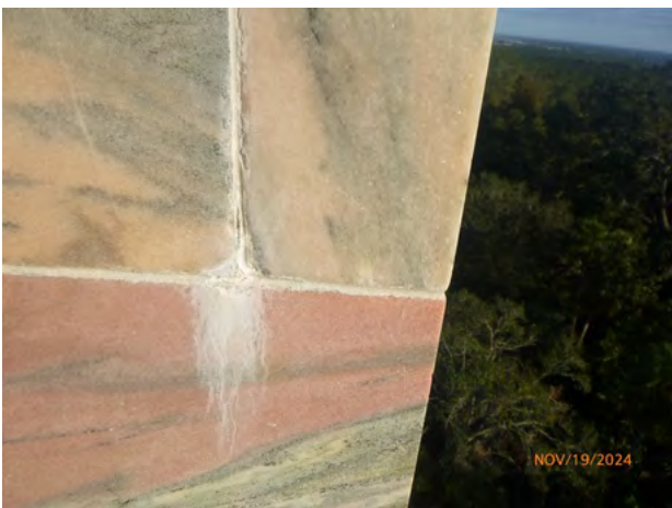
355-86 Stone_SoilStain Leached Salts 2024-2.jpg
