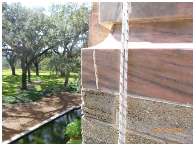
334-28 Stone_Crack Repair failed 2024-2.jpg
