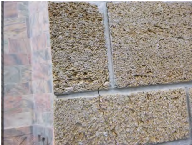
135-32 Stone_Crack System units and joints 2024-1.jpg
