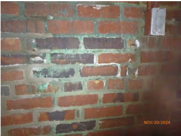
867-140 Brick_SoilStain Copper 2024-1.jpg
