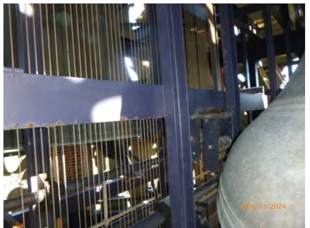
742-150 ArchMetal_Coating Coating Failed 2024-5.jpg
