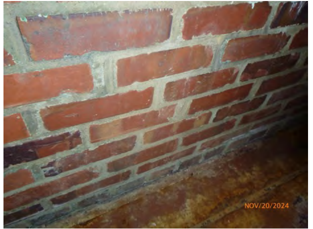
746-139 Brick_Spall Missing 2024-2.jpg
