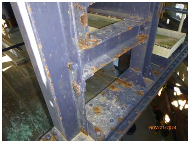
844-147 ArchMetal_Corrosion Fastener rusted 2024-7.jpg
