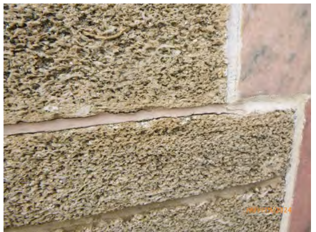
241-130 Stone_Joints Sealant Failed 2024-2.jpg
