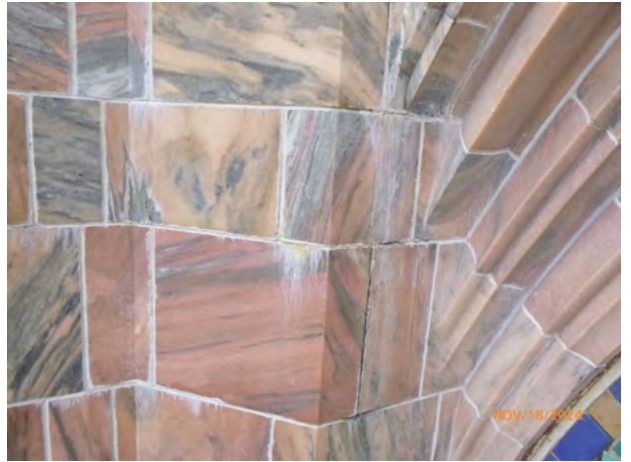
346-176 Stone_SoilStain Leached Salts 2024-1.jpg
