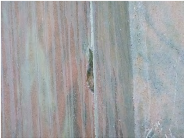
23-146 Stone_Spall Removed 2024-1.jpg
