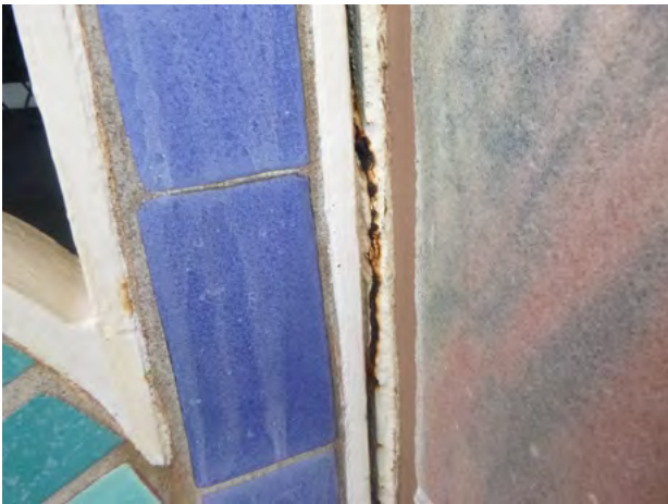
118-167 ArchMetal_Corrosion Pitted 2024-2.jpg
