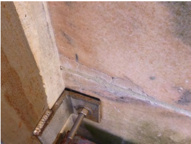
637-193 Stone_Repair Patch Failed 2024-1.jpg
