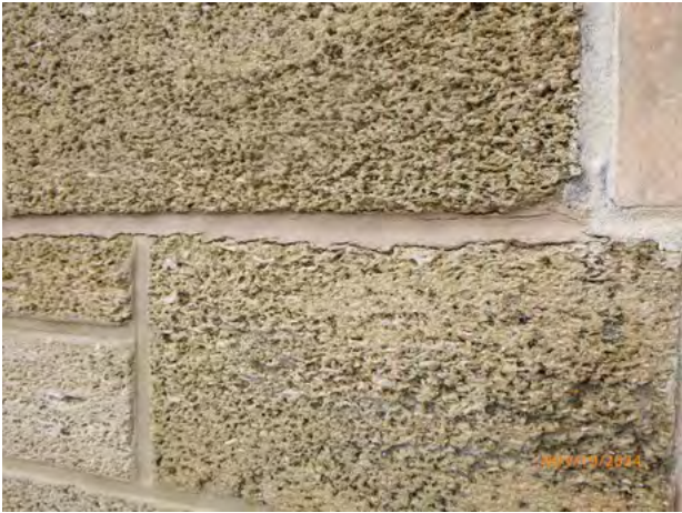
240-101 Stone_Joints Sealant Failed 2024-2.jpg
