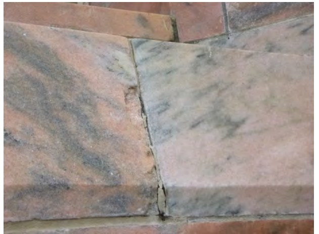
154-142 Stone_Spall Missing 2024-1.jpg
