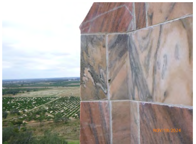
345-181 Stone_Joints Mortar Failed 2024-1.jpg
