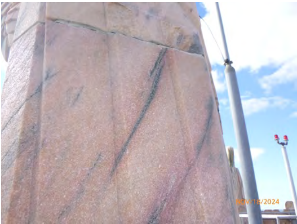
35-198 Stone_Spall Missing 2024-1.jpg
