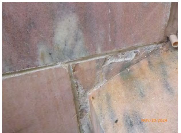
134-142 Stone_Spall Missing 2024-2.jpg
