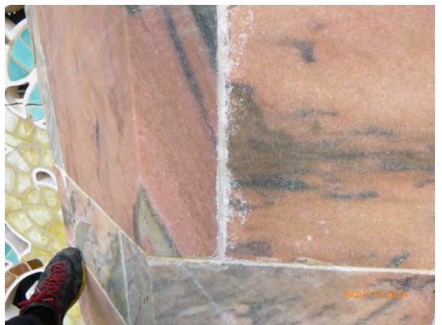
241-164 Stone_SurfLoss Chipped 2024-3.jpg
