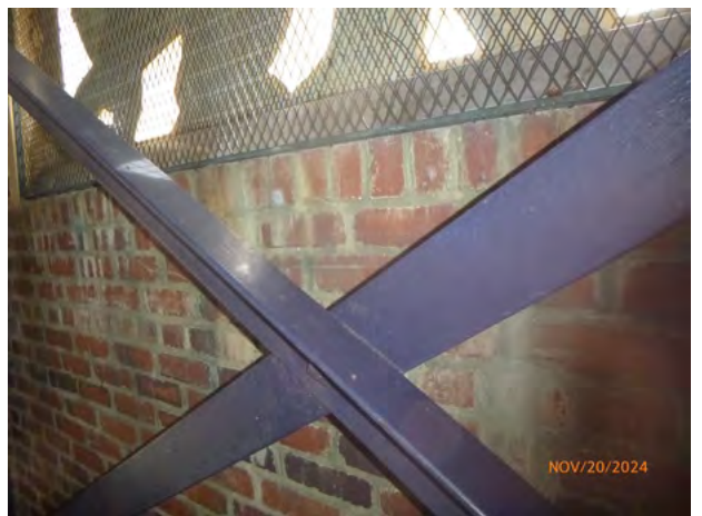
751-143 Brick_Crack System units and joints 2024-1.jpg
