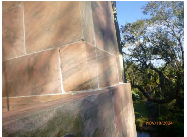
356-32 Stone_Spall Missing 2024-1.jpg
