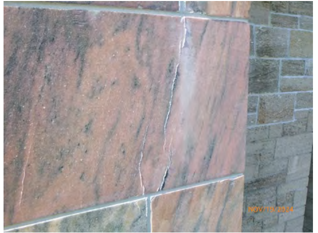
344-88 Stone_Crack System units and joints 2024-2.jpg
