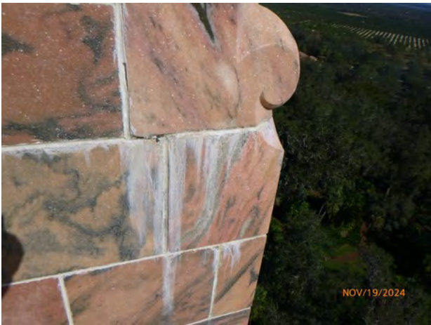
272-156 Stone_SoilStain Leached Salts 2024-3.jpg
