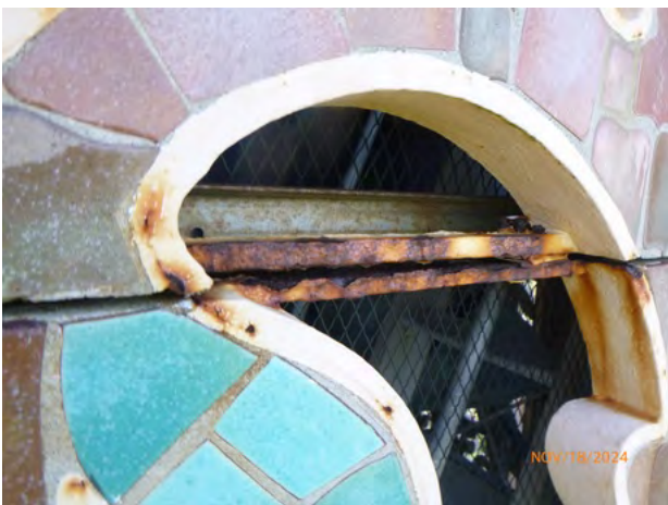
14-158 ArchMetal_Corrosion Pitted 2024-2.jpg
