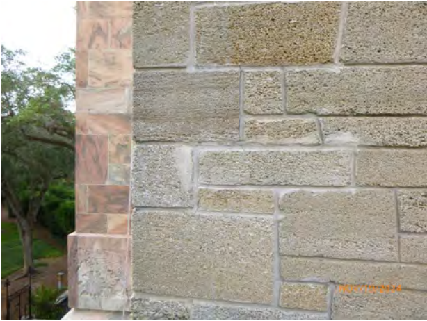
235-33 Stone_Crack System units and joints 2024-1.jpg
