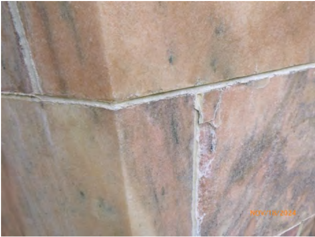
356-174 Stone_SurfLoss Chipped 2024-3.jpg
