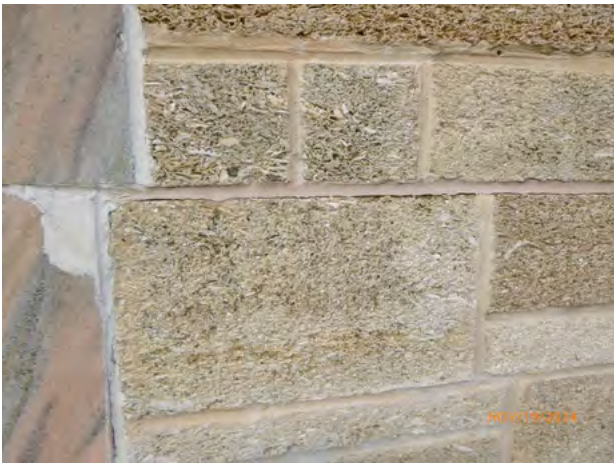
240-101 Stone_Joints Sealant Failed 2024-4.jpg
