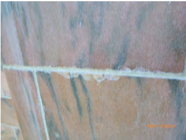
34-156 Stone_SurfLoss Chipped 2024-1.jpg
