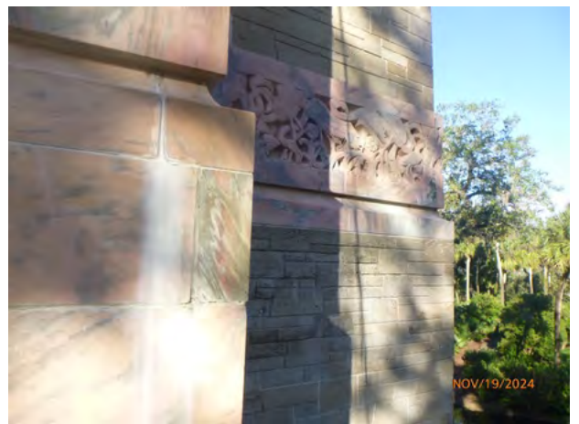
359-21 Stone_SoilStain Leached Salts 2024-2.jpg
