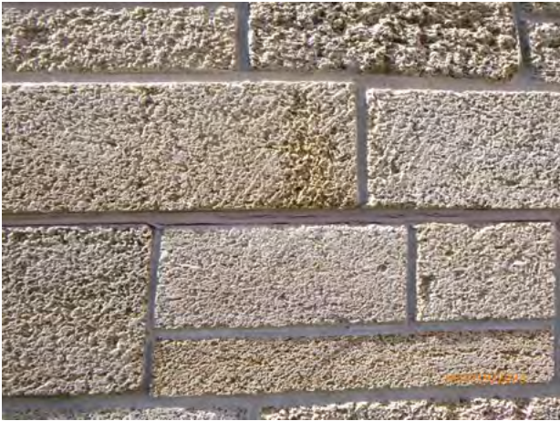
340-53 Stone_Joints Sealant Failed 2024-4.jpg
