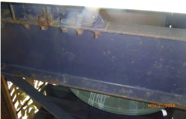
562-170 ArchMetal_Coating Coating Failed 2024-5.jpg
