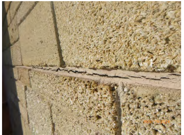
355-68 Stone_Joints Sealant Failed 2024-5.jpg
