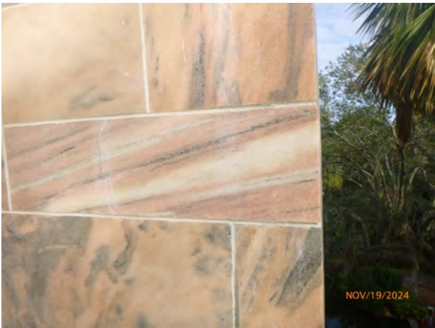
356-41 Stone_Crack Single unit 2024-2.jpg
