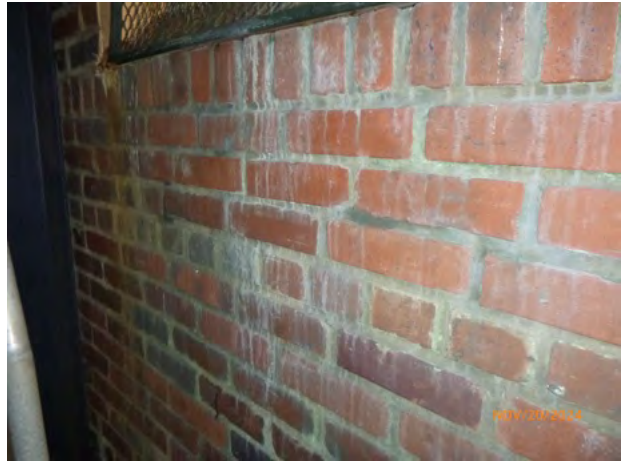
849-142 Brick_SoilStain Leached Salts 2024-2.jpg
