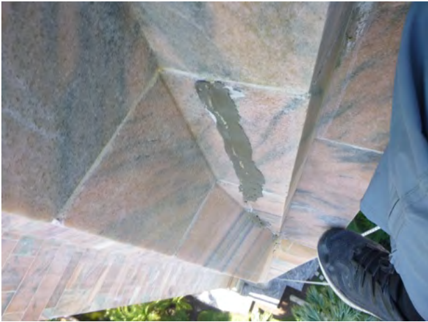
35-122 Stone_Crack Repair failed 2024-1.jpg
