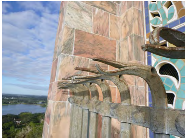
287-128 ArchMetal_Corrosion Surface 2024-1.jpg
