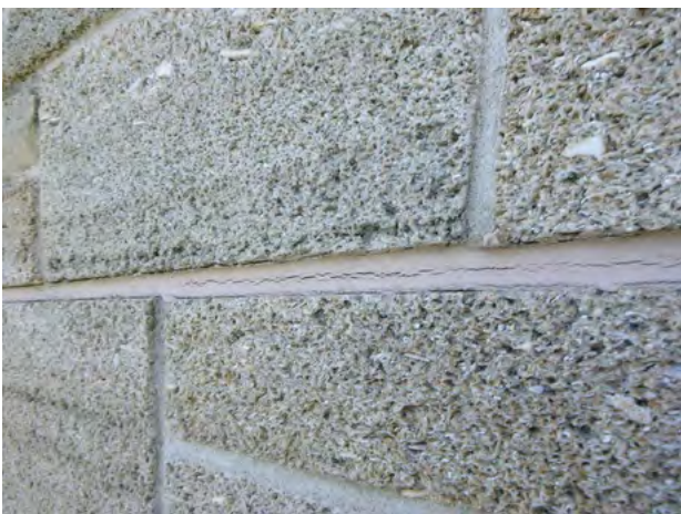
37-90 Stone_Joints Sealant Failed 2024-2.jpg
