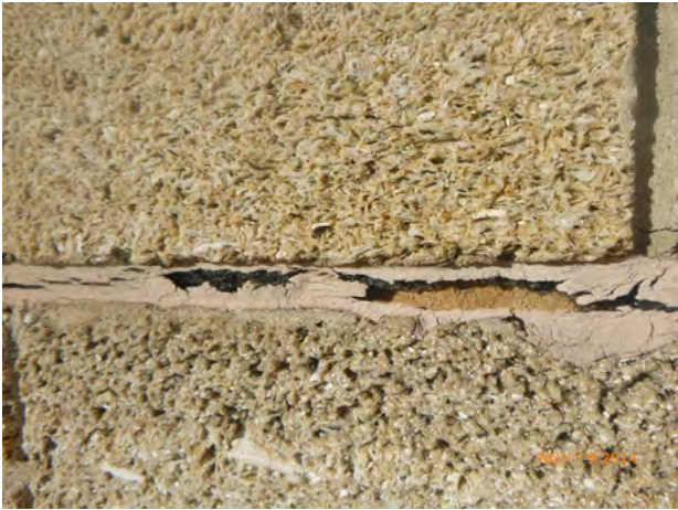
355-68 Stone_Joints Sealant Failed 2024-2.jpg
