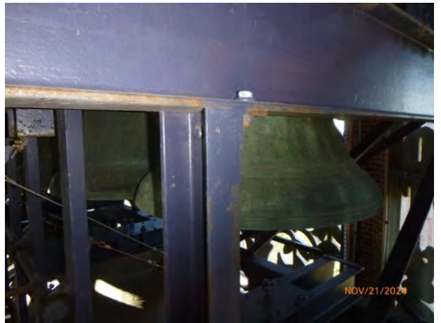
559-162 ArchMetal_Coating Coating Failed 2024-1.jpg
