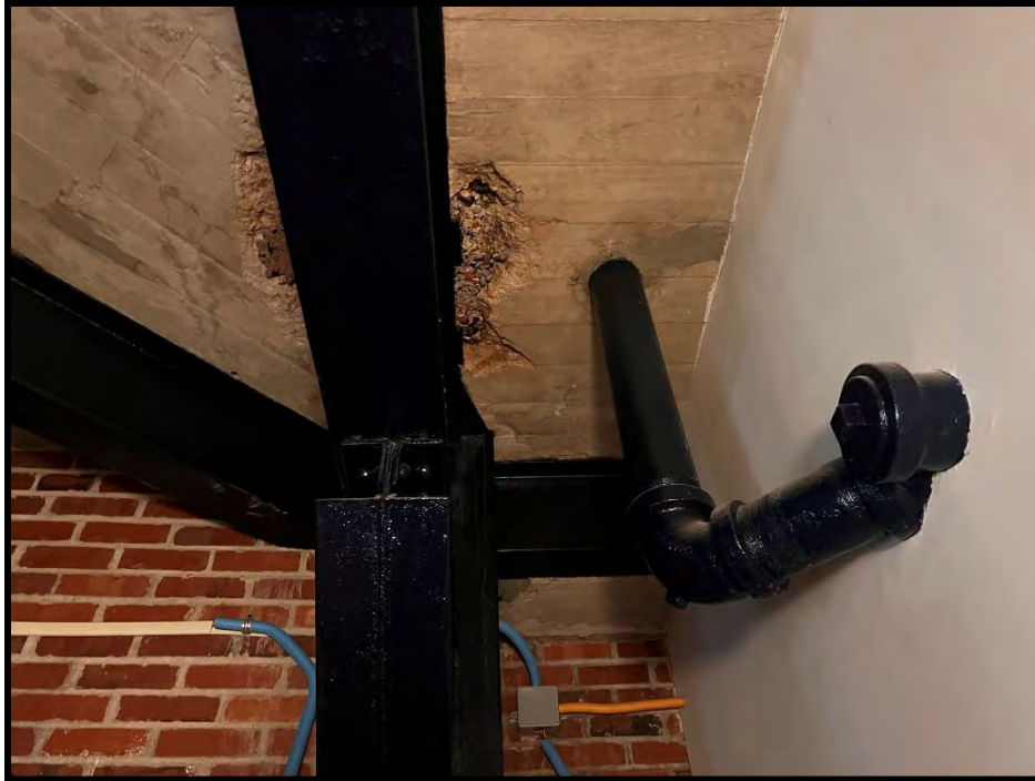
Figure 20 Spalled concrete where steel meets underside of wet slab
