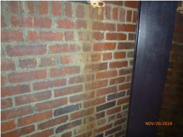
642-140 Brick_SoilStain Rust 2024-1.jpg
