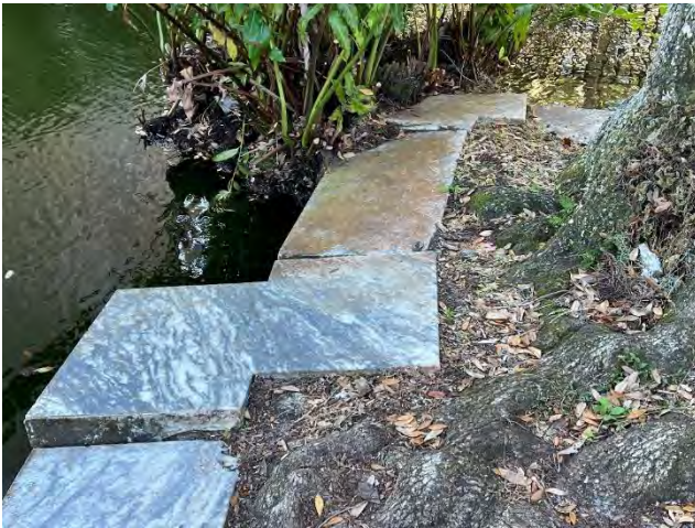
26 Moat coping stones out of plumb.
