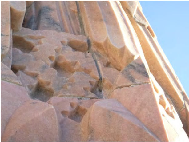
257-192 Stone_Joints Mortar Failed 2024-1.jpg
