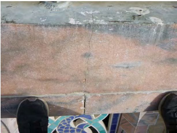
251-122 Stone_Crack System units and joints 2024-1.jpg
