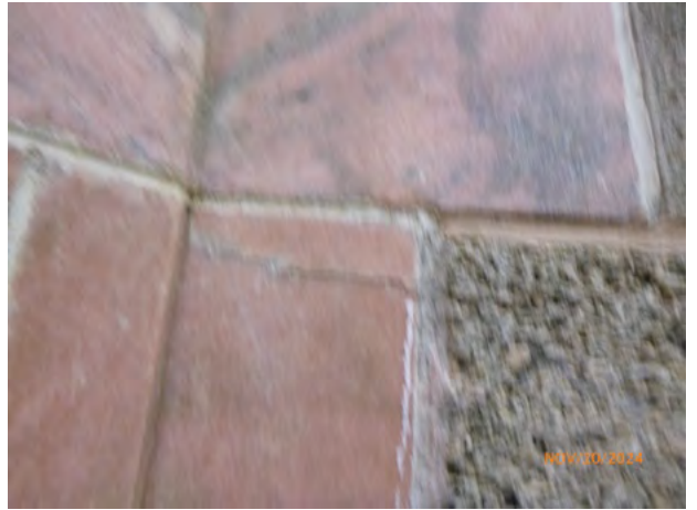
59-128 Stone_Crack Single unit 2024-2.jpg
