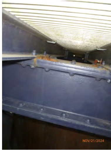
763-147 ArchMetal_Coating Coating Failed 2024-2.jpg
