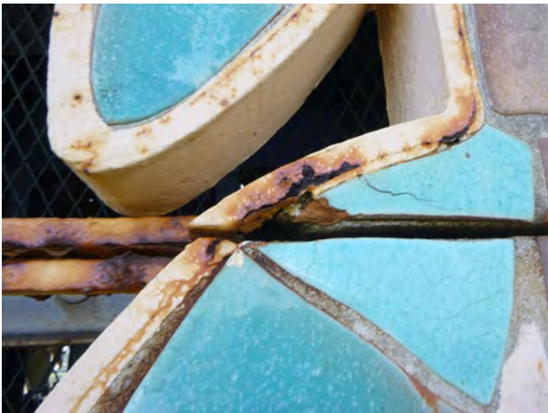
15-164 TerraCotta_Spall Missing 2024-1.jpg
