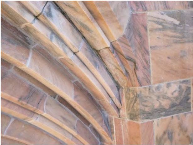
255-177 Stone_SoilStain Leached Salts 2024-1.jpg
