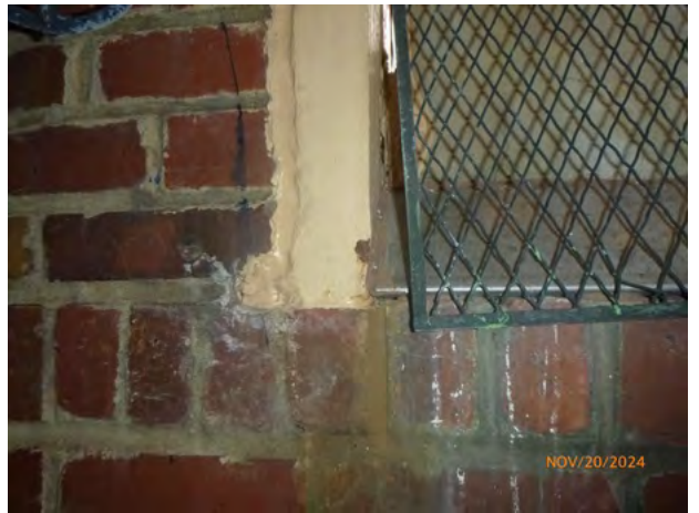
758-143 ArchMetal_Corrosion Surface 2024-1.jpg
