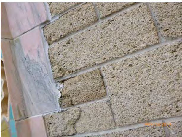
355-108 Stone_Crack System units and joints 2024-3.jpg
