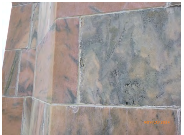
133-179 Stone_SurfLoss Chipped 2024-1.jpg
