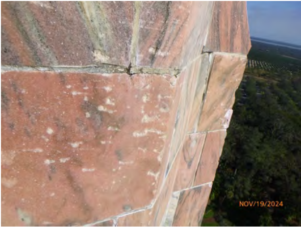
341-181 Stone_SurfLoss Chipped 2024-4.jpg
