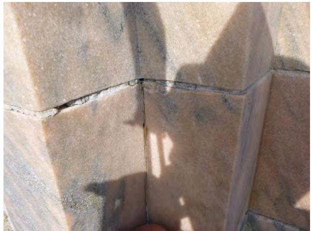
335-136 Stone_Joints Mortar Failed 2024-1.jpg
