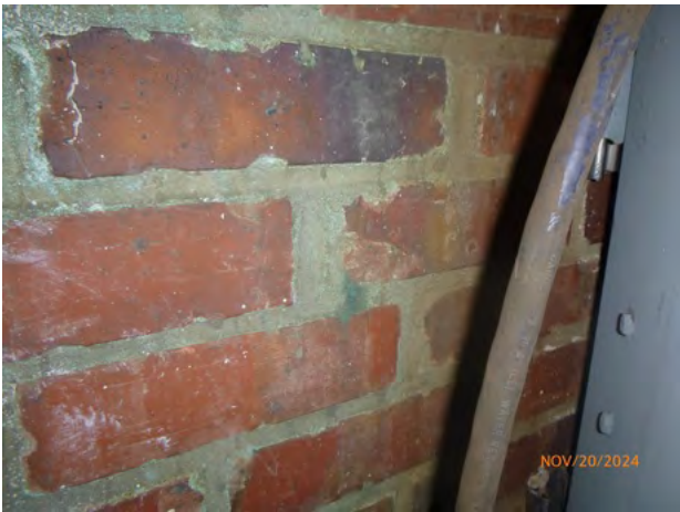
537-141 Brick_Spall Missing 2024-1.jpg
