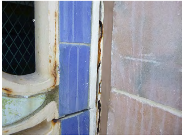
19-159 ArchMetal_Corrosion Pitted 2024-1.jpg
