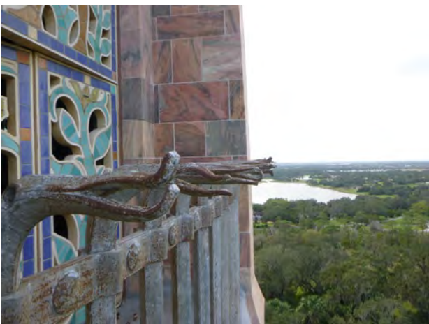
87-127 ArchMetal_Corrosion Surface 2024-1.jpg
