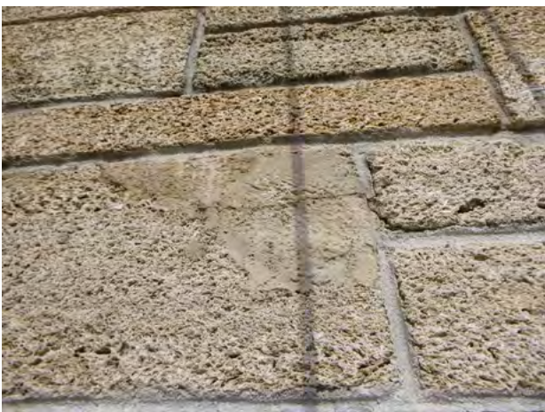
262-120 Stone_Repair Patch Failed 2024-1.jpg
