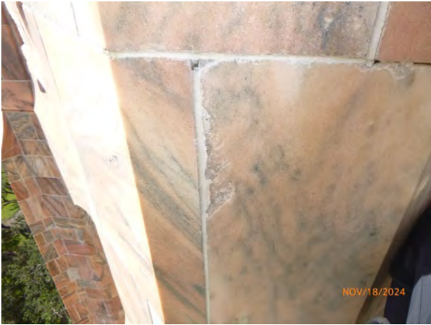
33-188 Stone_Spall Missing 2024-3.jpg
