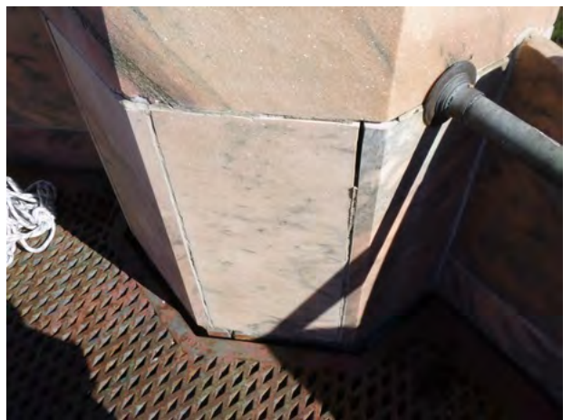
844-193 Stone_Joints Mortar Failed 2024-1.jpg
