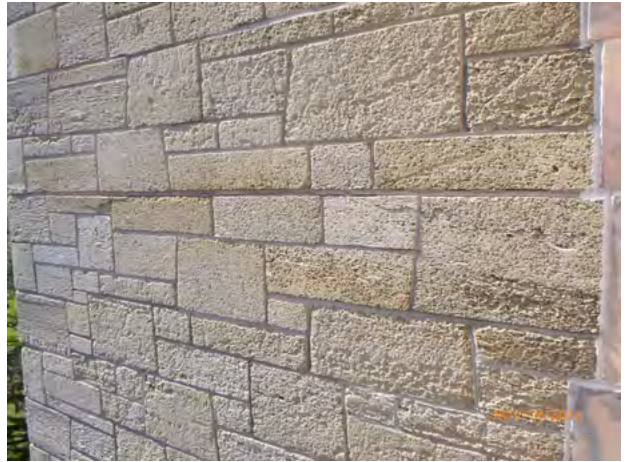
340-68 Stone_Joints Sealant Failed 2024-1.jpg
