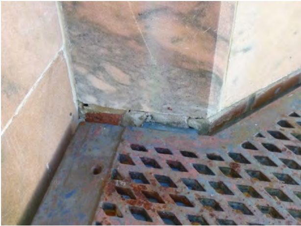
755-193 Stone_Joints Mortar Failed 2024-1.jpg
