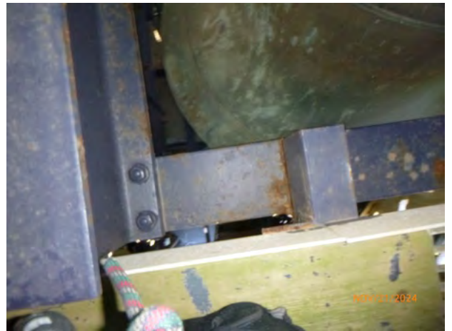
561-157 ArchMetal_Coating Coating Failed 2024-4.jpg
