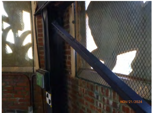
746-144 ArchMetal_Coating Coating Failed 2024-2.jpg
