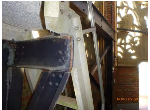
846-142 ArchMetal_Coating Coating Failed 2024-2.jpg
