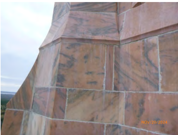
138-179 Stone_SoilStain Leached Salts 2024-2.jpg
