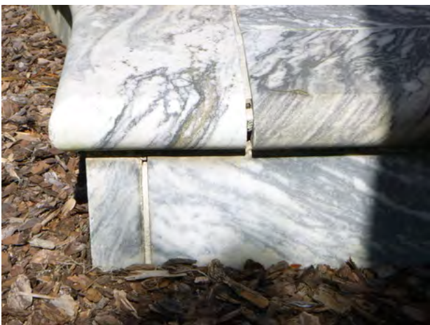
219-1 Stone_Joints Mortar Failed 2024-1.jpg
