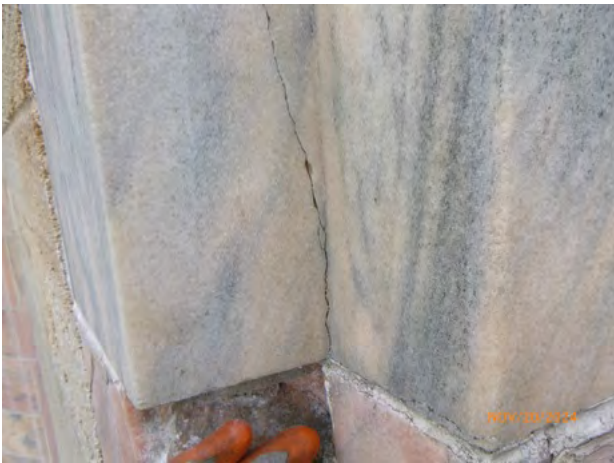
134-105 Stone_Crack Single unit 2024-3.jpg
