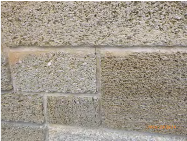
66-77 Stone_Crack Single unit 2024-2.jpg
