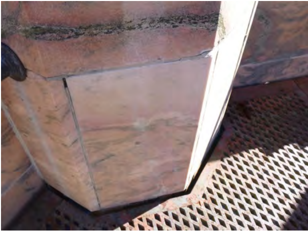
844-193 Stone_Joints Mortar Failed 2024-2.jpg
