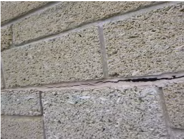
139-121 Stone_Joints Sealant Failed 2024-2.jpg
