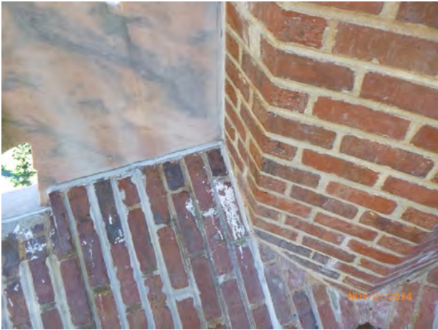
844-184 Brick_Joints Sealant Failed 2024-1.jpg
