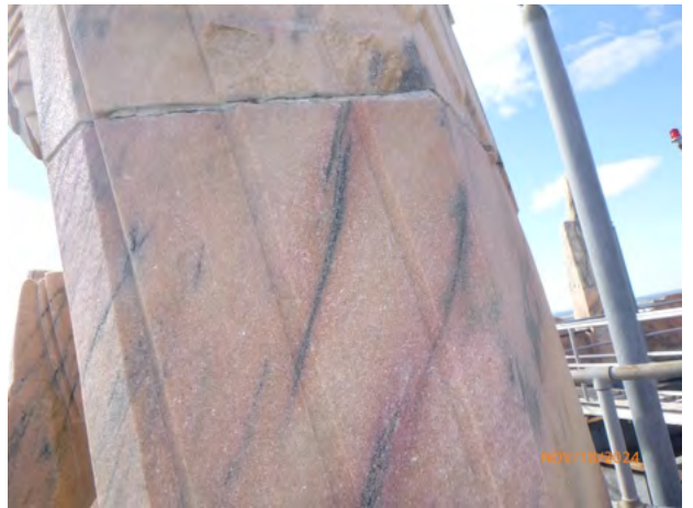
35-198 Stone_Spall Missing 2024-2.jpg
