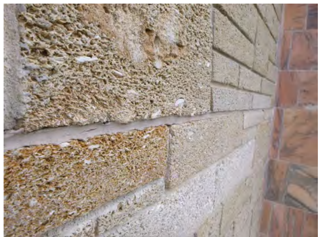
150-41 Stone_Joints Sealant Failed 2024-2.jpg
