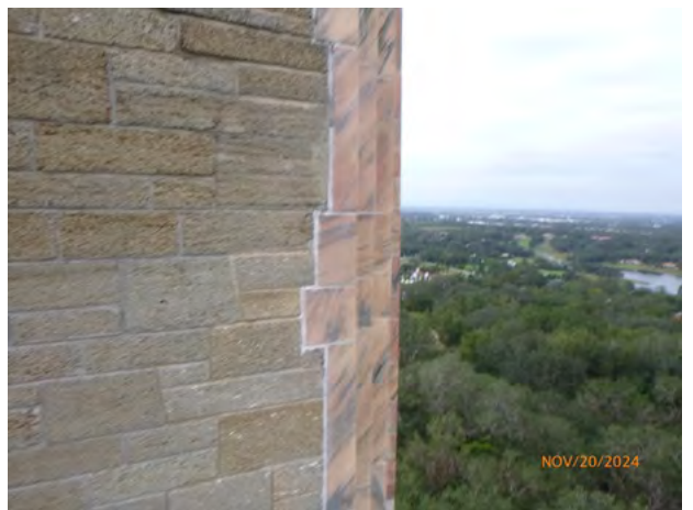
66-132 Stone_Crack System units and joints 2024-1.jpg
