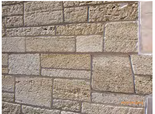
340-53 Stone_Joints Sealant Failed 2024-1.jpg
