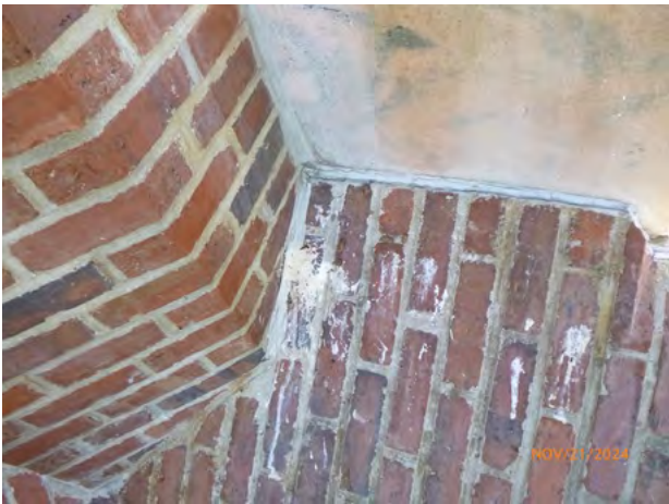
757-184 Brick_Joints Sealant Failed 2024-6.jpg
