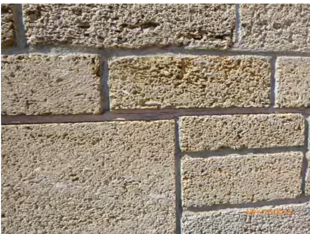
341-122 Stone_Joints Sealant Failed 2024-3.jpg
