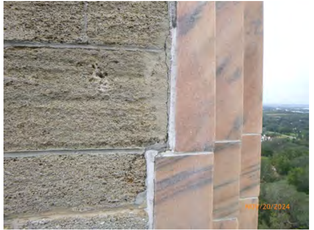
66-132 Stone_Crack System units and joints 2024-3.jpg
