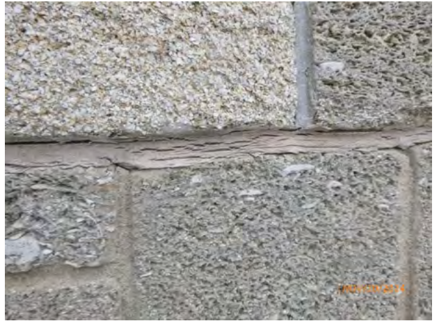
61-121 Stone_Joints Sealant Failed 2024-3.jpg
