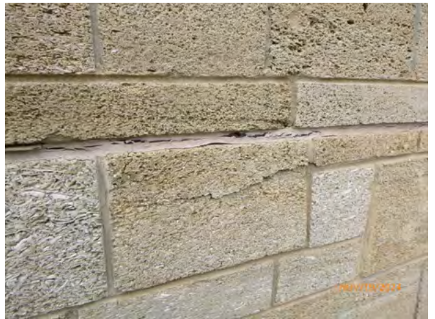
241-44 Stone_Joints Sealant Failed 2024-2.jpg
