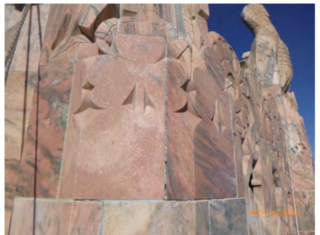
343-185 Stone_Joints Mortar Failed 2024-1.jpg
