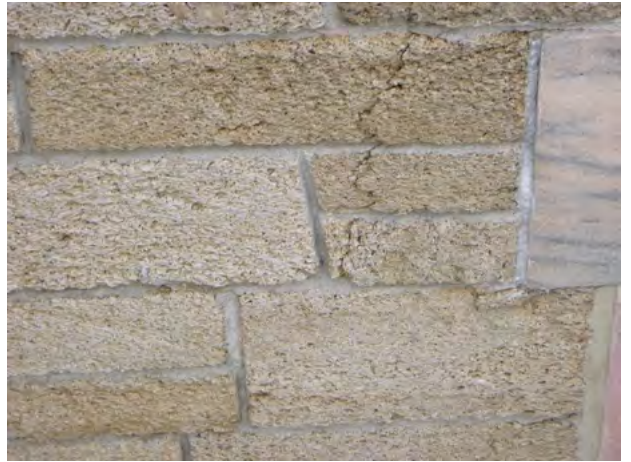
146-108 Stone_Crack System units and joints 2024-4.jpg
