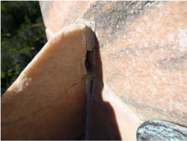
639-194 Stone_Joints Mortar Failed 2024-1.jpg
