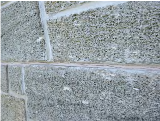
37-82 Stone_Joints Sealant Failed 2024-2.jpg
