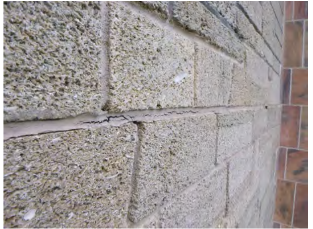
50-92 Stone_Joints Sealant Failed 2024-1.jpg
