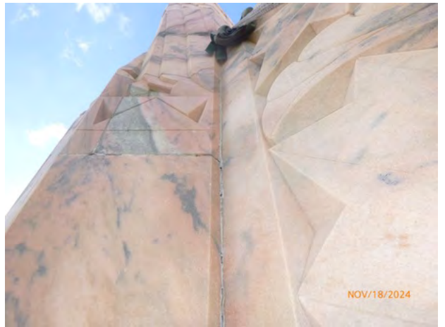
36-185 Stone_Joints Mortar Failed 2024-2.jpg
