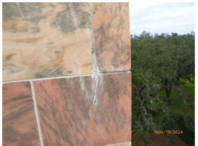
173-68 Stone_SoilStain Leached Salts 2024-1.jpg
