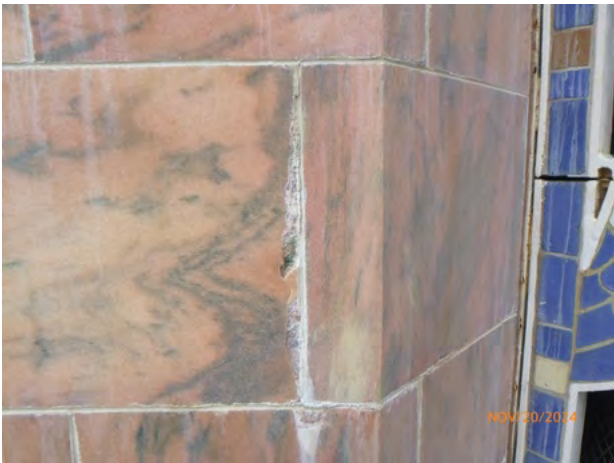
134-146 Stone_SurfLoss Chipped 2024-3.jpg
