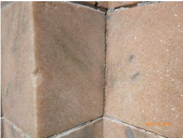
333-132 Stone_Crack Repair failed 2024-2.jpg
