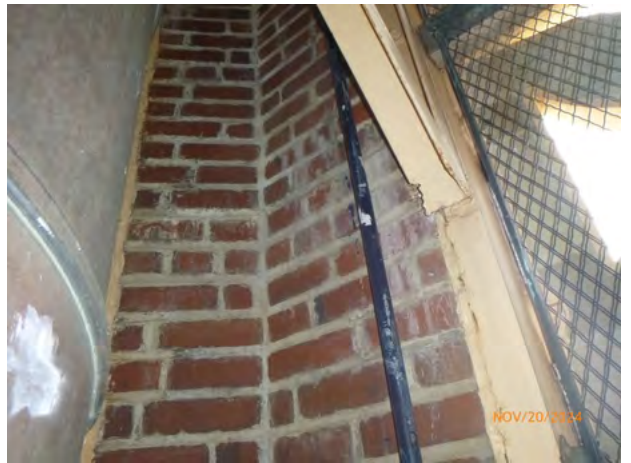
745-154 Brick_SoilStain Cementitious 2024-1.jpg
