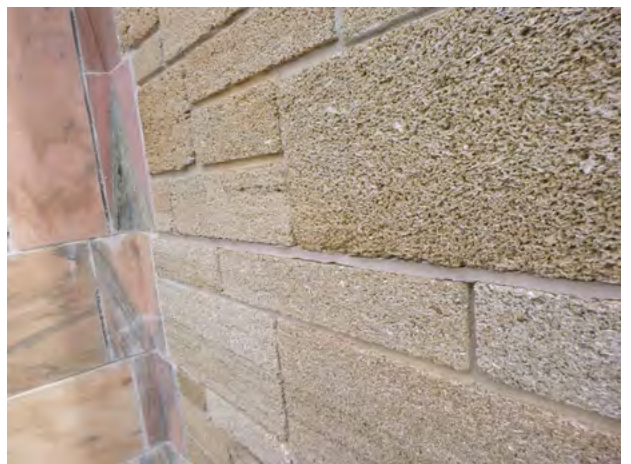
151-79 Stone_Joints Sealant Failed 2024-1.jpg
