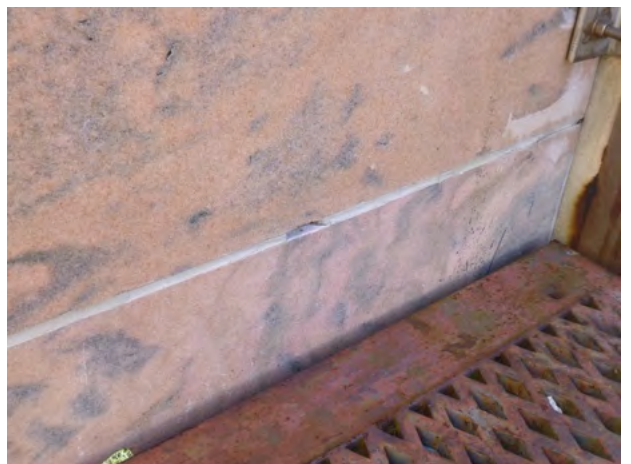
848-194 Stone_Joints Mortar Failed 2024-1.jpg
