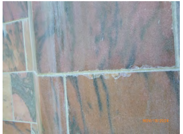
34-156 Stone_SurfLoss Chipped 2024-2.jpg
