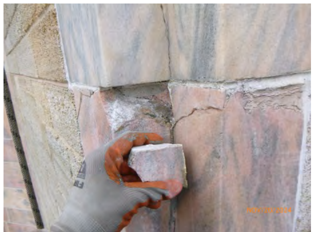
134-102 Stone_Spall Removed 2024-3.jpg
