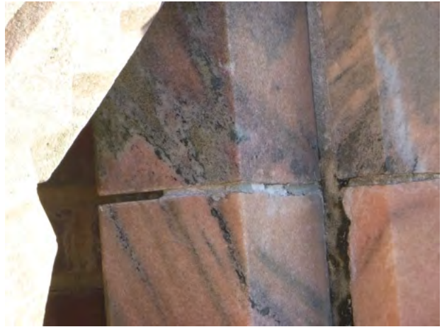
255-188 Stone_Joints Mortar Failed 2024-1.jpg
