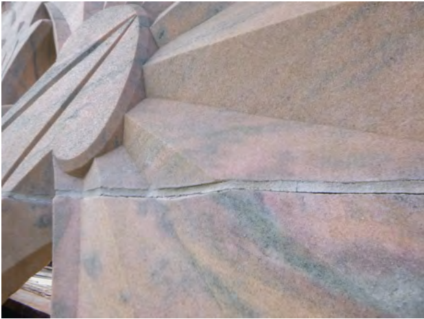
40-193 Stone_Joints Mortar Failed 2024-1.jpg
