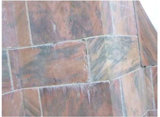
141-182 Stone_SoilStain Leached Salts 2024-2.jpg
