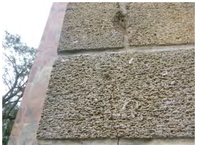
135-10 Stone_Crack System units and joints 2024-1.jpg
