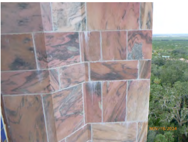
355-144 Stone_SoilStain Leached Salts 2024-1.jpg
