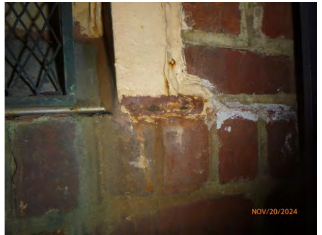
655-144 ArchMetal_Corrosion Pitted 2024-1.jpg
