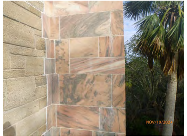
356-41 Stone_Crack Single unit 2024-1.jpg
