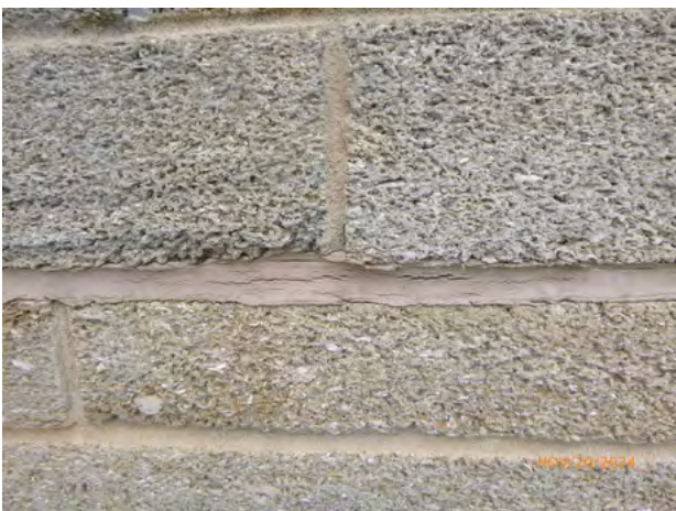
62-81 Stone_Joints Sealant Failed 2024-3.jpg
