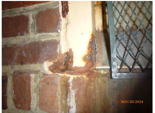
541-144 ArchMetal_Corrosion Pitted 2024-1.jpg
