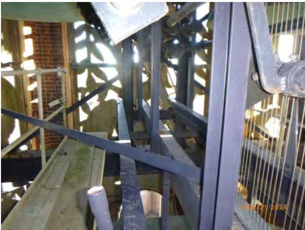
664-149 ArchMetal_Coating Coating Failed 2024-4.jpg
