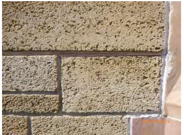
341-122 Stone_Joints Sealant Failed 2024-2.jpg
