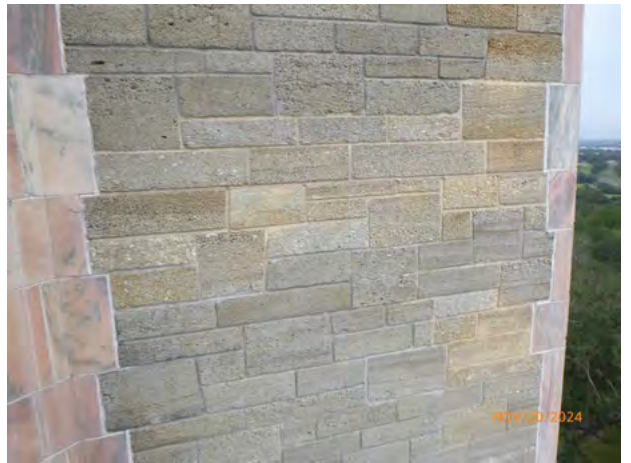
61-101 Stone_Joints Sealant Failed 2024-1.jpg
