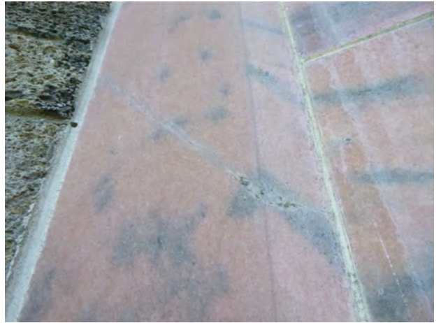
41-83 Stone_Crack Single unit 2024-1.jpg
