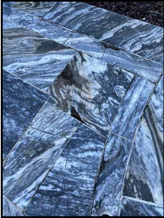
Figure 35 Cracks and staining of Creole marble at tower exterior
