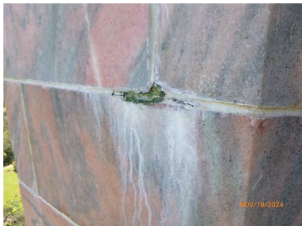
36-165 Stone_SoilStain Leached Salts 2024-3.jpg
