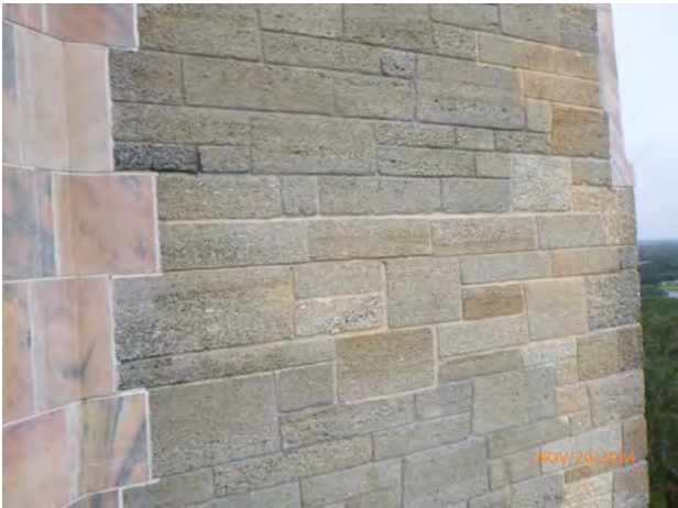
61-90 Stone_Joints Sealant Failed 2024-1.jpg
