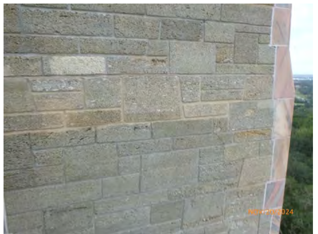
61-121 Stone_Joints Sealant Failed 2024-1.jpg
