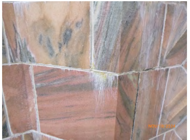
346-176 Stone_SoilStain Leached Salts 2024-3.jpg
