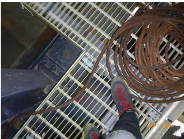
763-147 ArchMetal_Coating Coating Failed 2024-5.jpg
