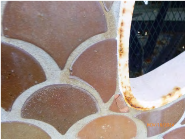
388-151 TerraCotta_Coating Coating Failed 2024-1.jpg
