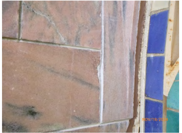
344-173 Stone_SurfLoss Chipped 2024-1.jpg
