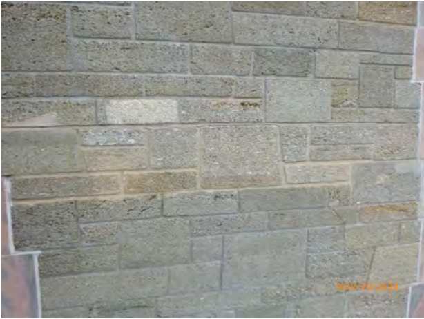
61-121 Stone_Joints Sealant Failed 2024-2.jpg
