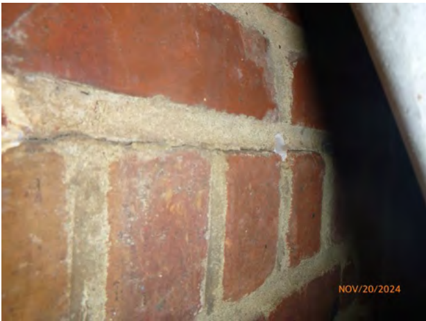
539-144 Brick_Joints Mortar Failed 2024-1.jpg
