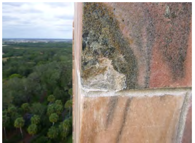
229-157 Stone_Spall Removed 2024-1.jpg
