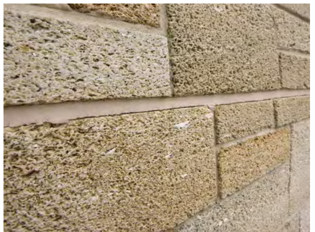
163-66 Stone_Joints Sealant Failed 2024-1.jpg
