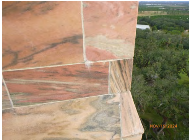
172-125 Stone_SoilStain Leached Salts 2024-1.jpg
