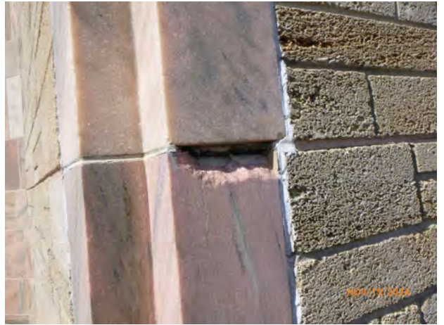
334-98 Stone_Spall Missing + Steel 2024-2.jpg
