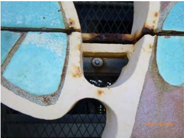
12-168 ArchMetal_Corrosion Pitted 2024-1.jpg
