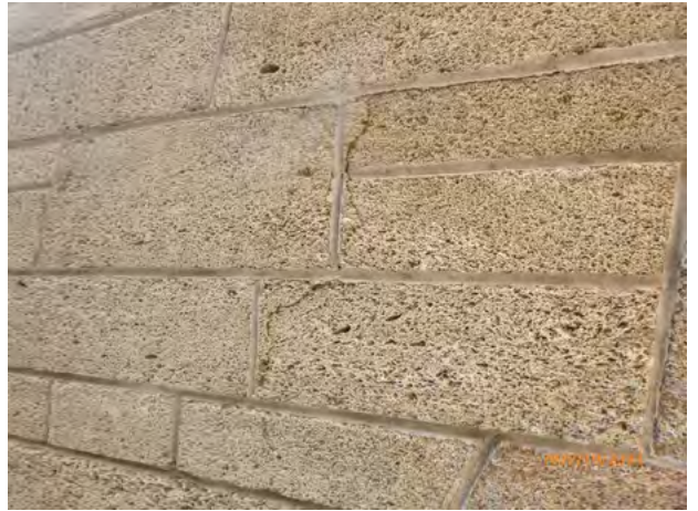
339-14 Stone_Crack System units and joints 2024-1.jpg
