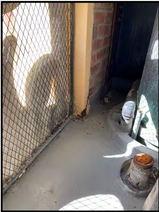
Figure 38 Corrosion at interior mosaic frame
