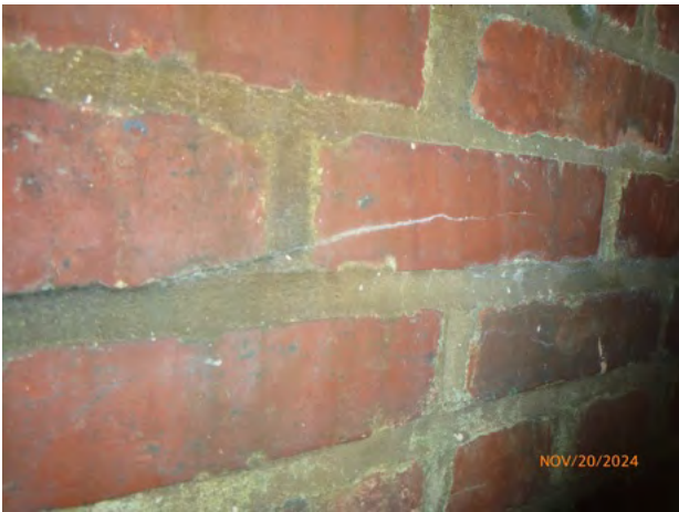
753-143 Brick_Crack System units and joints 2024-2.jpg
