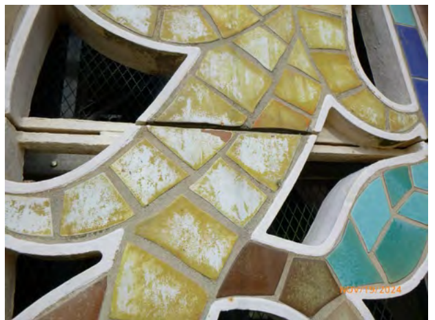
217-157 TerraCotta_SurfLoss Glaze loss 2024-1.jpg
