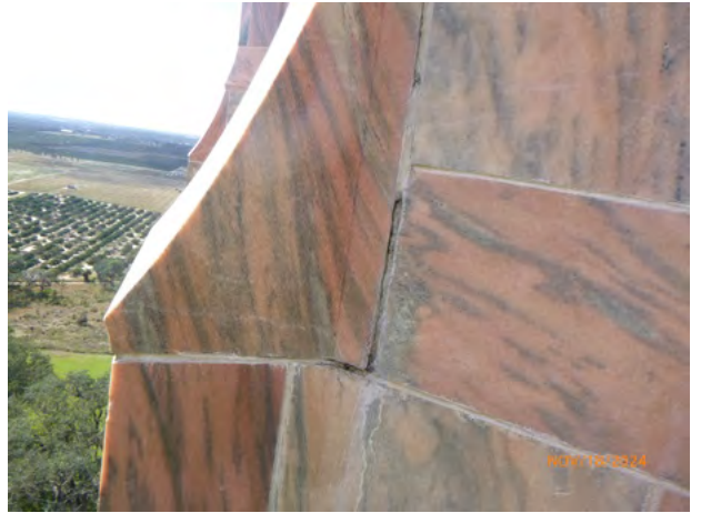
32-181 Stone_Joints Mortar Failed 2024-2.jpg
