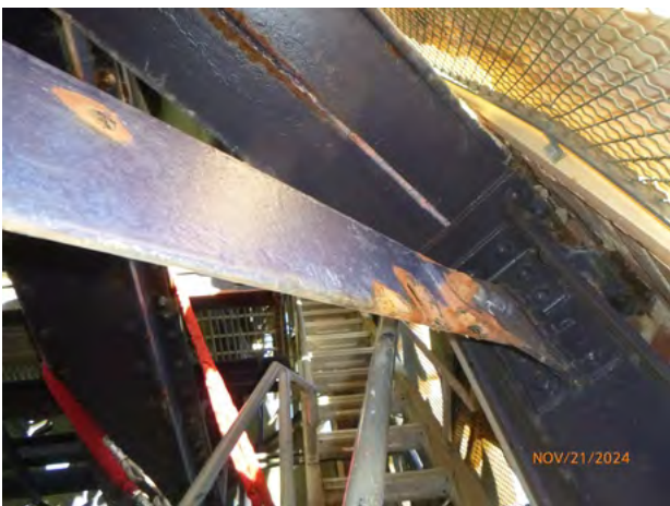
861-137 ArchMetal_Coating Coating Failed 2024-2.jpg
