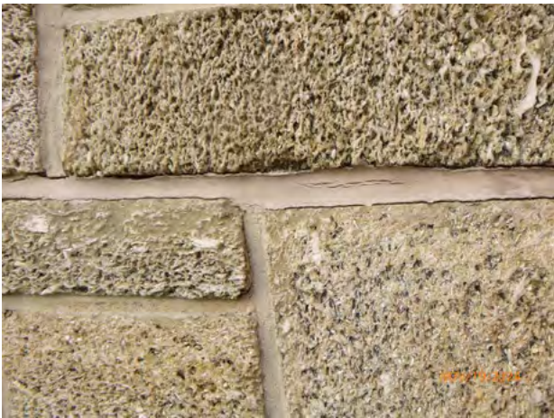
240-90 Stone_Joints Sealant Failed 2024-2.jpg
