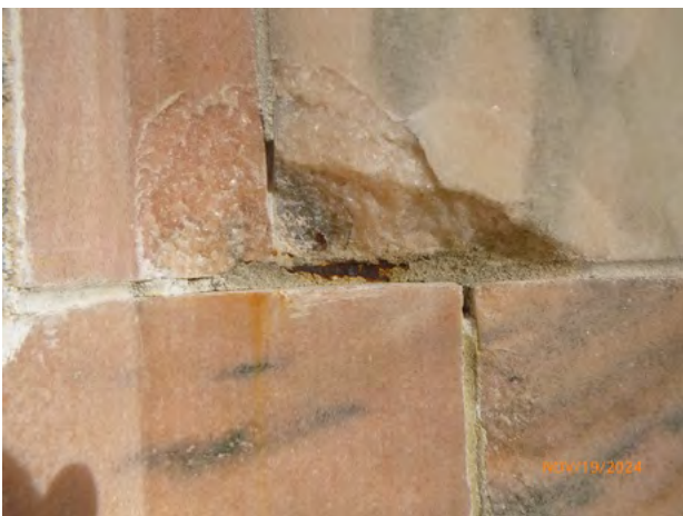
355-38 Stone_Spall Missing + Steel 2024-3.jpg
