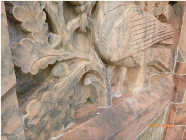
237-139 Stone_Spall Missing 2024-1.jpg
