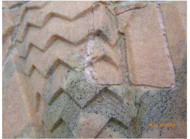
134-196 Stone_Repair Dutchman Failed 2024-3.jpg
