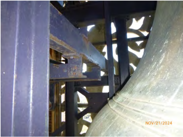
664-151 ArchMetal_Coating Coating Failed 2024-4.jpg
