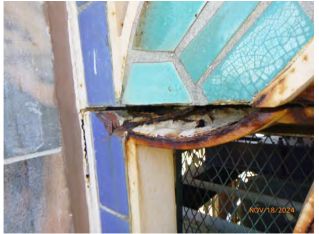
9-164 TerraCotta_Spall Missing + Steel 2024-2.jpg
