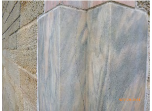
134-105 Stone_Crack Single unit 2024-2.jpg
