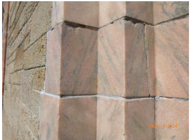
333-132 Stone_Crack Repair failed 2024-3.jpg
