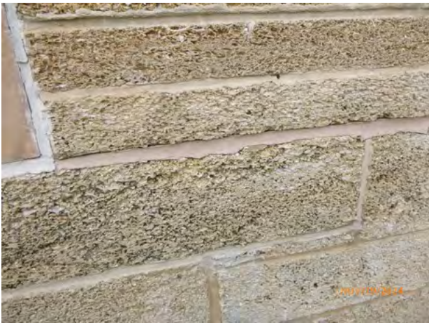
241-130 Stone_Joints Sealant Failed 2024-5.jpg
