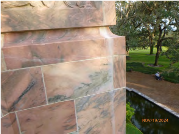
174-26 Stone_SoilStain Leached Salts 2024-1.jpg
