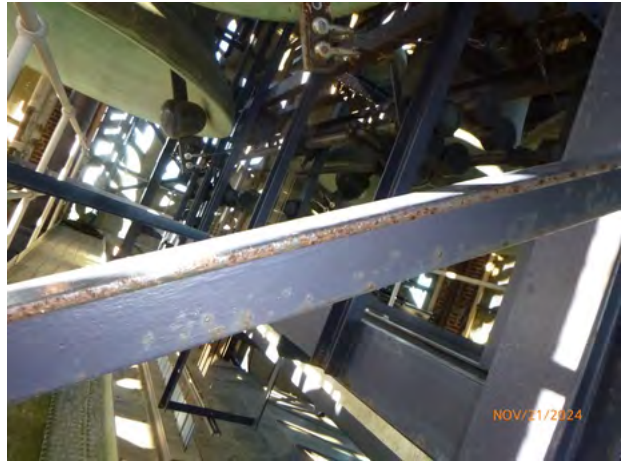
841-150 ArchMetal_Coating Coating Failed 2024-2.jpg
