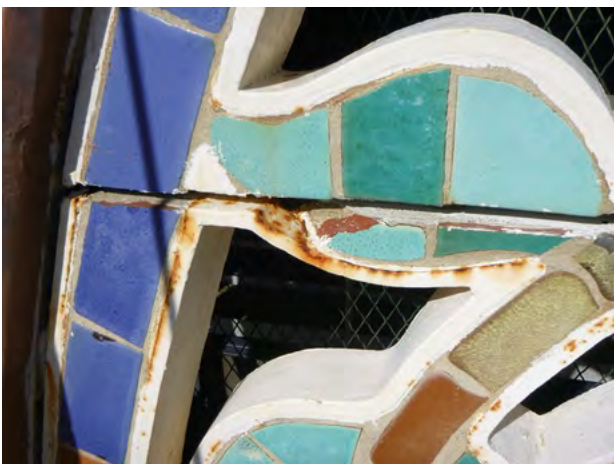
311-172 ArchMetal_Coating Coating Failed 2024-3.jpg
