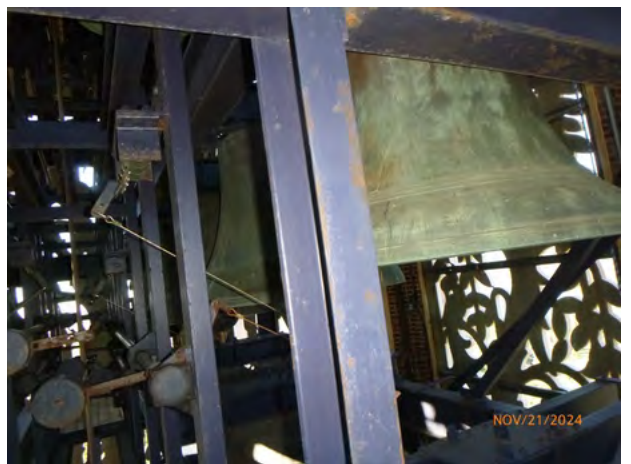
559-162 ArchMetal_Coating Coating Failed 2024-3.jpg
