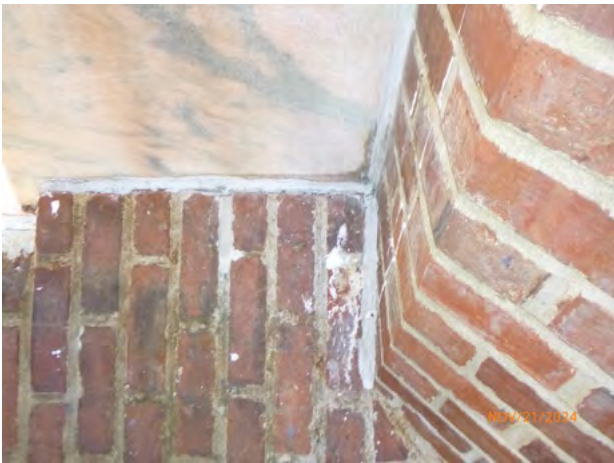
741-184 Brick_Joints Sealant Failed 2024-1.jpg
