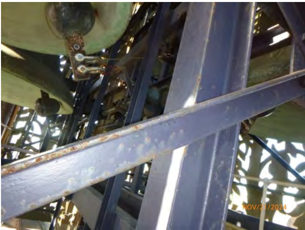
841-150 ArchMetal_Coating Coating Failed 2024-3.jpg
