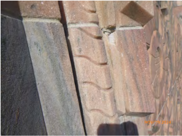
343-198 Stone_Spall Missing 2024-2.jpg
