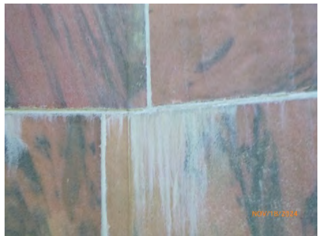
34-157 Stone_SoilStain Leached Salts 2024-2.jpg
