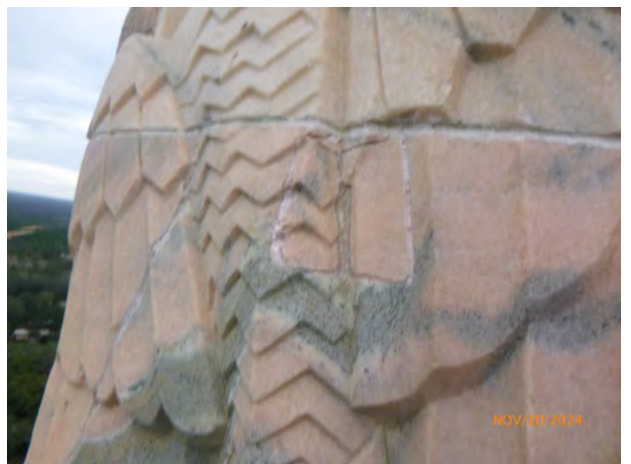
134-196 Stone_Repair Dutchman Failed 2024-1.jpg
