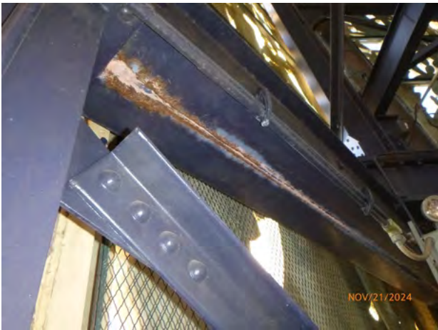
760-145 ArchMetal_Coating Coating Failed 2024-1.jpg
