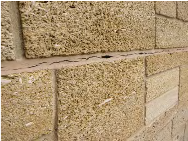
163-46 Stone_Joints Sealant Failed 2024-1.jpg
