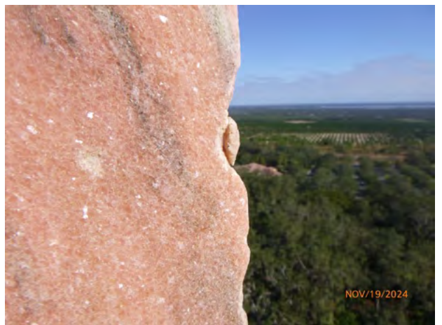
342-182 Stone_Repair Patch Failed 2024-2.jpg
